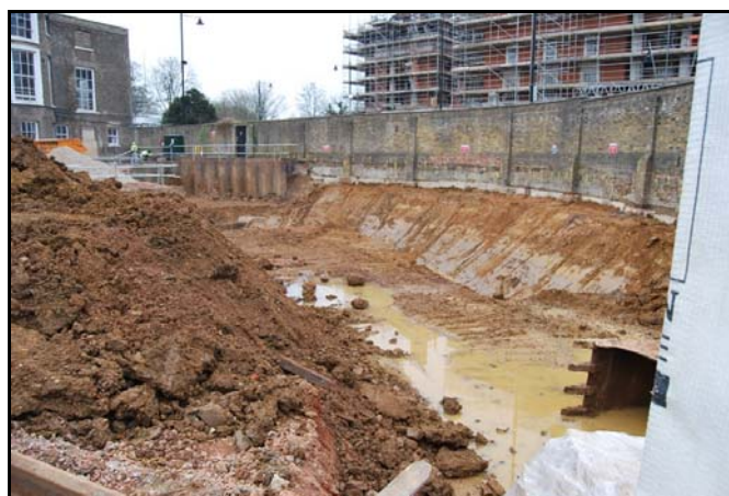
Plate 1: General shot of excavation area to north-west of Ancaster House, looking south-east
