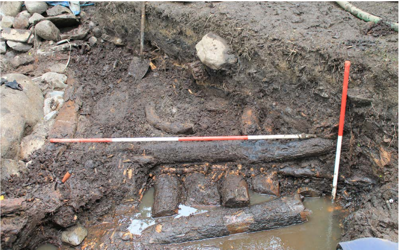
2. The foundation framework [277] after the removal of the brash and branchwood, exposing the stepped facade created by the alternating layers of logs set at right angles to each other
