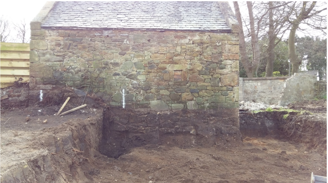
Plate 12: General view of the north-west elevation of the outbuilding, showing the extent of the wall foundations. Note also the small blocked window now exposed after the removal of the vegetation
