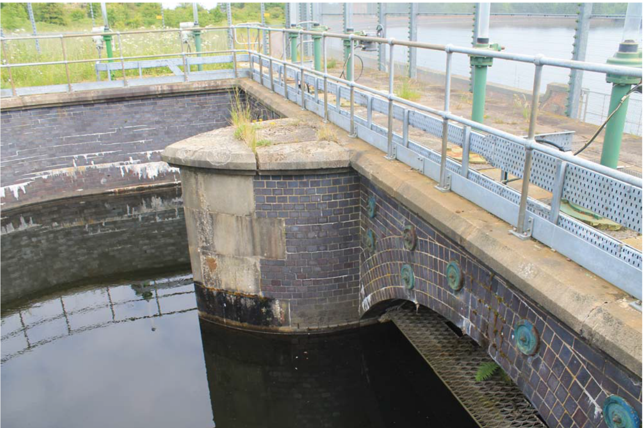
Plate 58: Inlet House, detail of the breakwater to the inlet basin from the west
