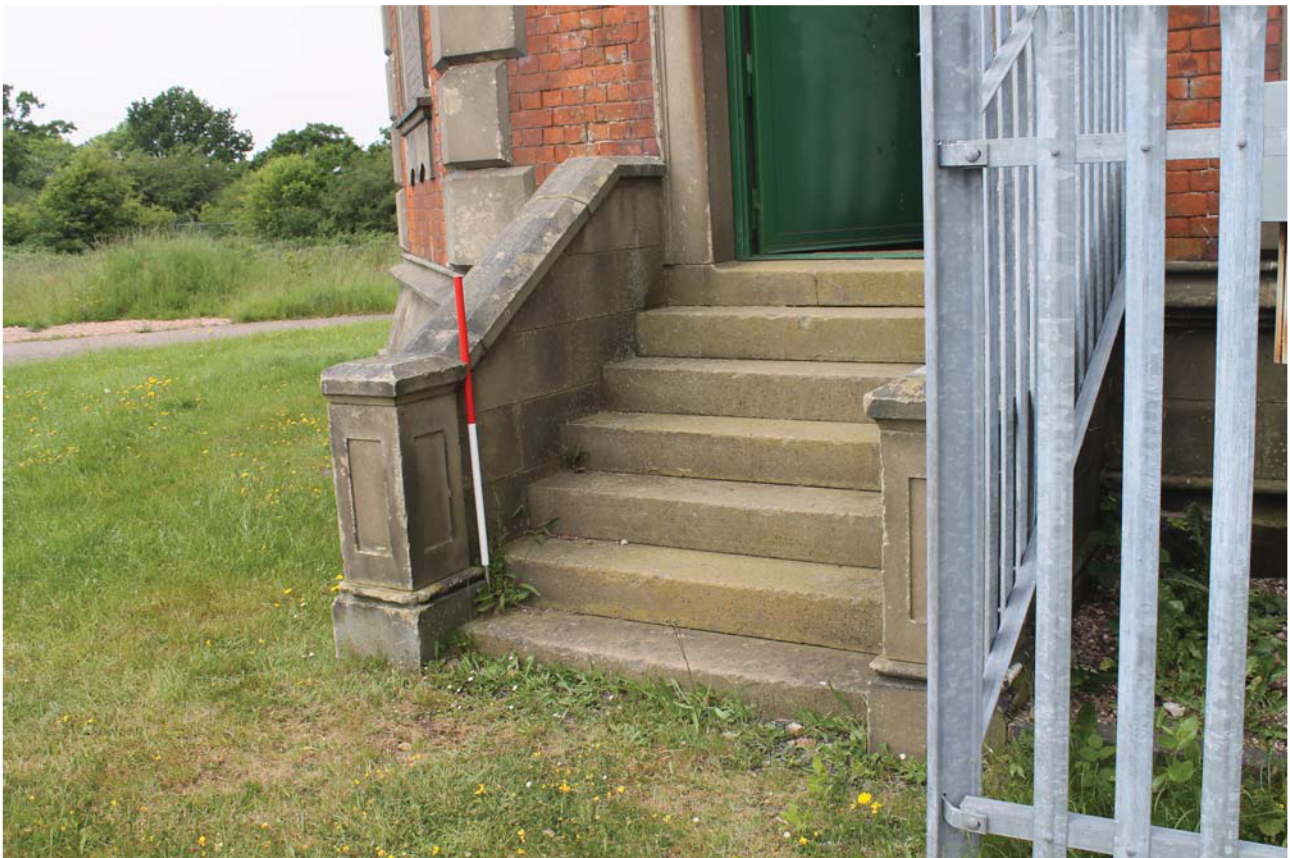
Plate 38: Outlet House 2, detail of the stone steps to the main entrance from the east
