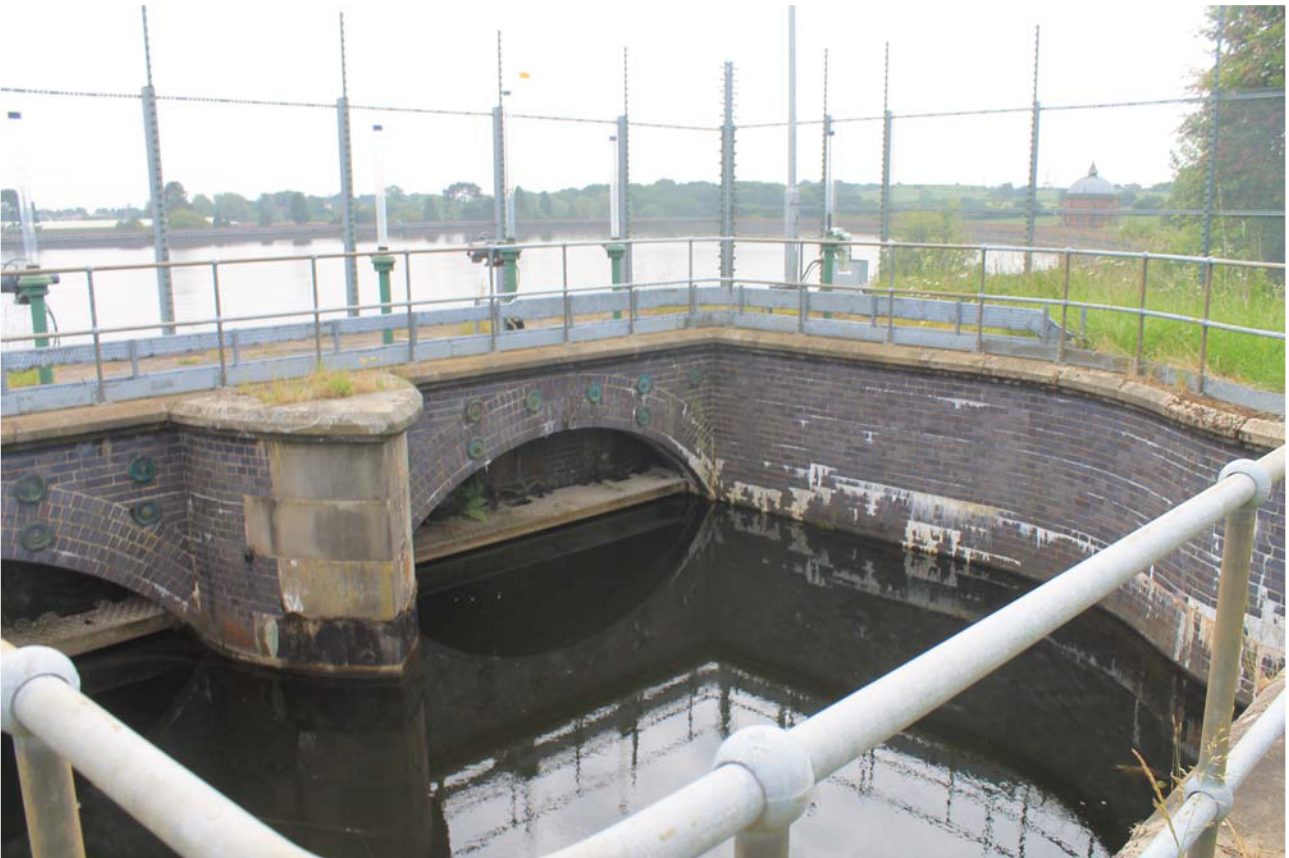
Plate 56: Inlet House, general view of small arches to the inlet basin from the north
