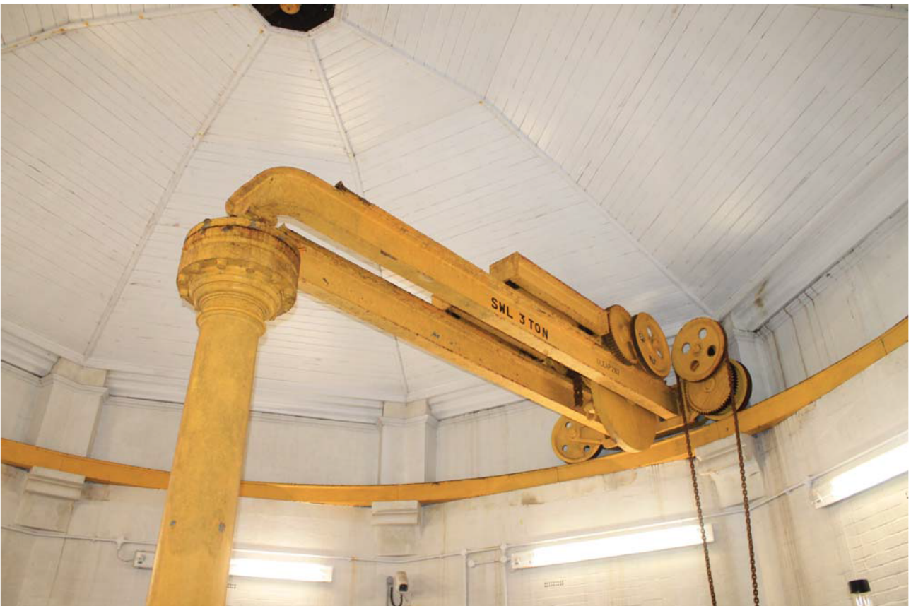
Plate 32: Outlet House 1 Interior, detail of machinery in the roof supporting the main pump from the south
