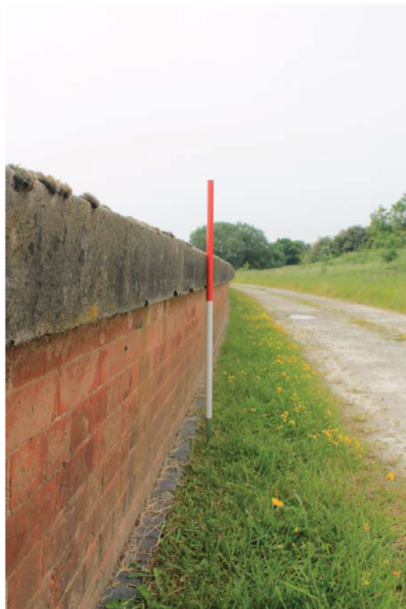
Plate 4: Reservoir, detail of the parapet wall on the north-west side from the north
