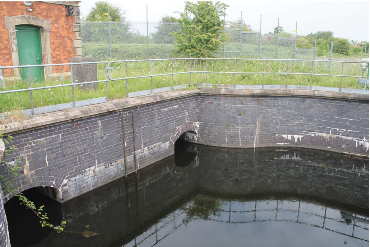
Plate 57: Inlet House, general view of larger arches to the inlet basin leading to reservoir from the south
