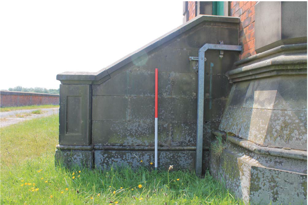
Plate 24: Outlet House 1, detail of steps to the main entrance from the north-east
