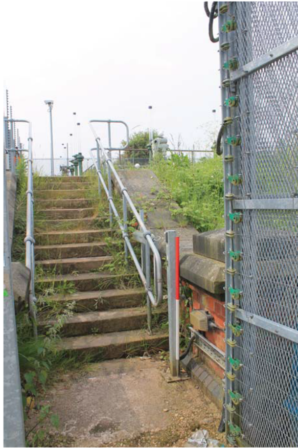
Plate 61: Inlet House, detail of the north-east steps to the main compound from the north-east
