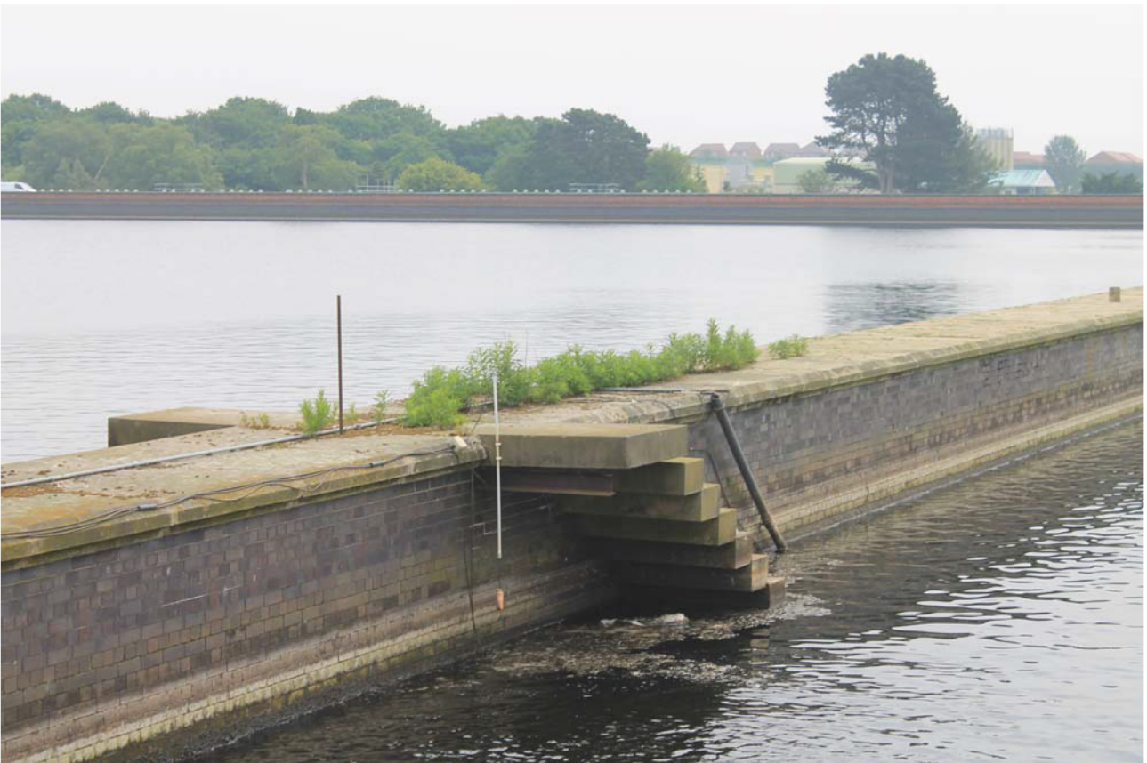
Plate 12: Reservoir, detail of steps on the central dividing wall from the west
