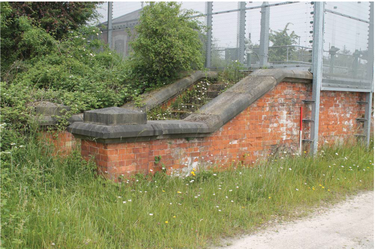
Plate 60: Inlet House, detail of south-west steps to the main compound from the south
