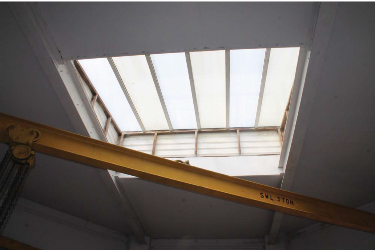
Plate 44: Outlet House 2 Interior, detail of ceiling and skylight, a modern intervention completed in the 1970s from the south-east
