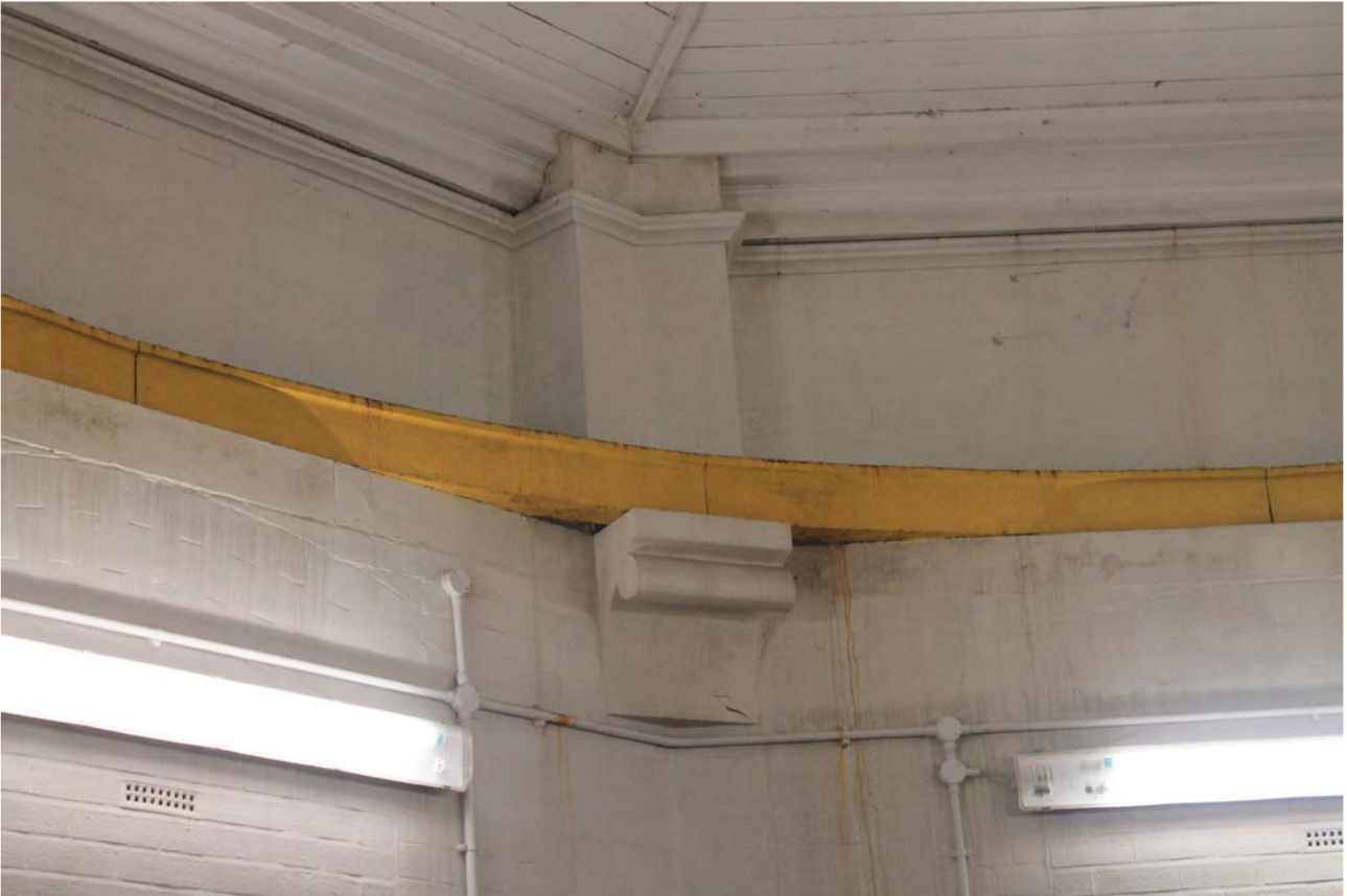
Plate 31: Outlet House 1 Interior, detail of roof support and steel beam from the east
