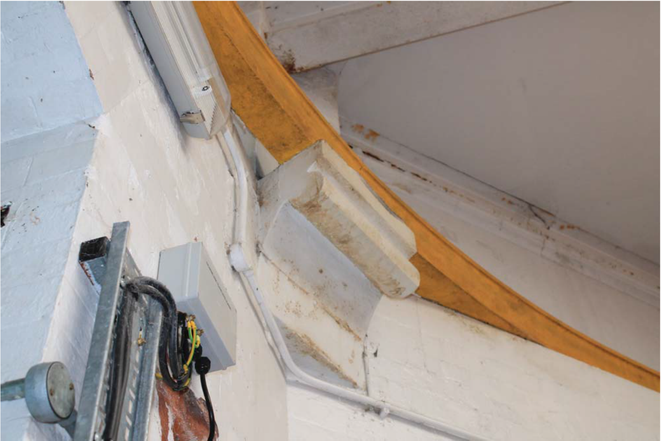
Plate 43: Outlet House 2 Interior, detail of corbel supporting the steel beam from the east
