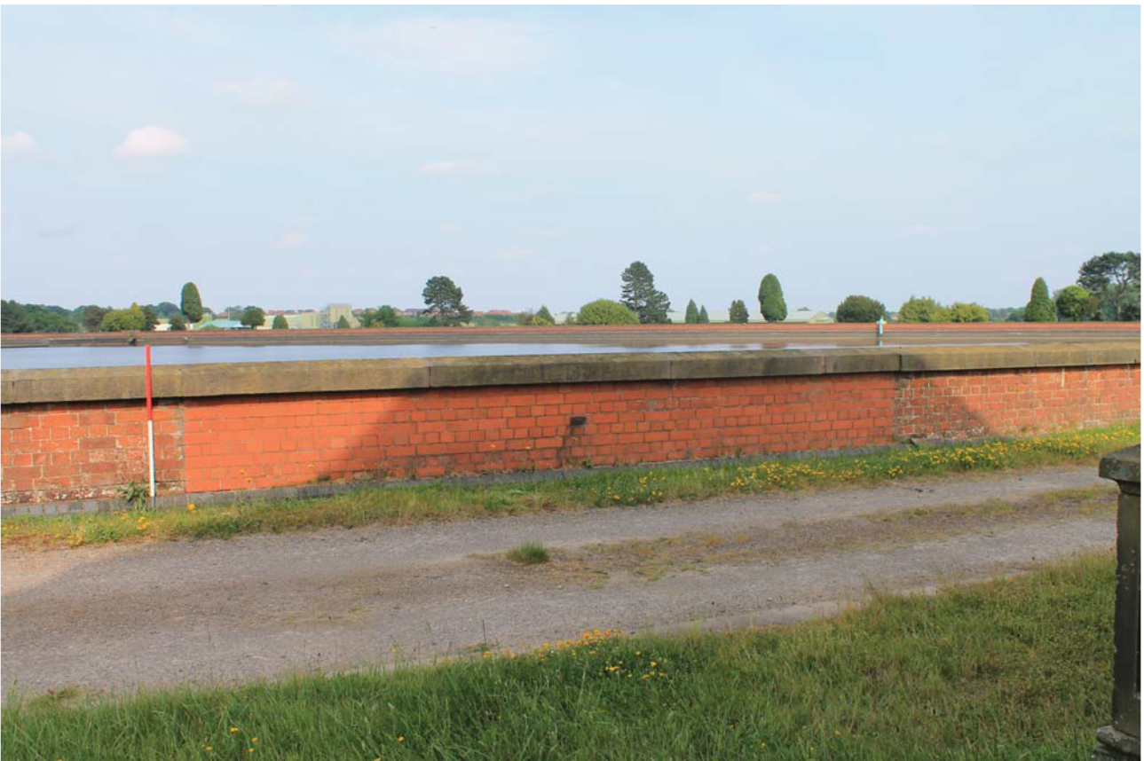
Plate 8: Reservoir, detail of brick repair on the north-west side from the north
