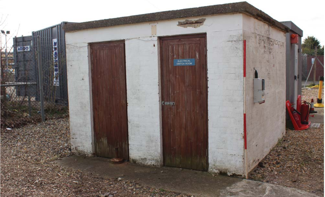
Plate 21: Sea Street, Herne Bay, general view of the Electrical Switch Room from the NNW
