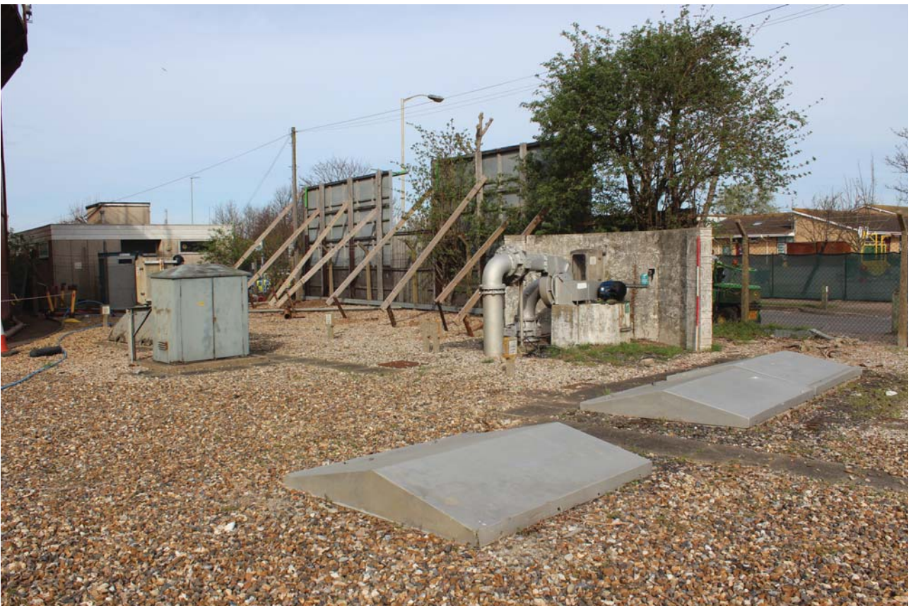
Plate 24: Sea Street, Herne Bay, general view of pipe inlet/outlet from the south
