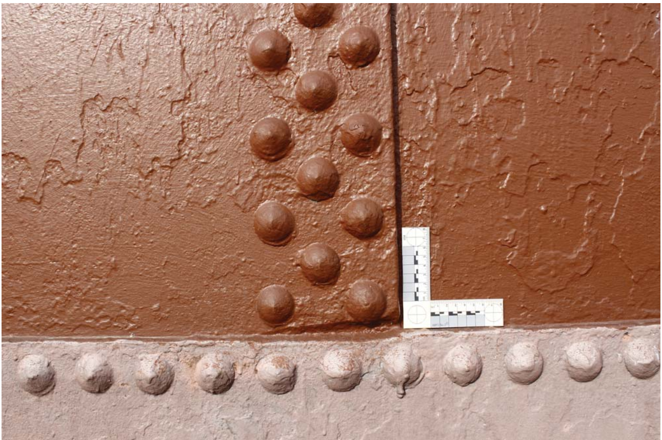
Plate 8: Sea Street, Herne Bay, close detail of the riveted plates from the east
