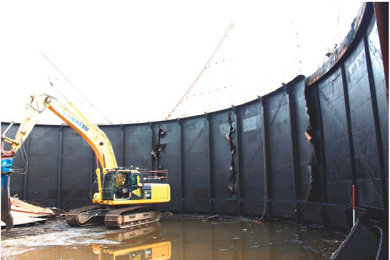
Plate 18: Sea Street, Herne Bay, general view of the interior of the gasholder from the south
