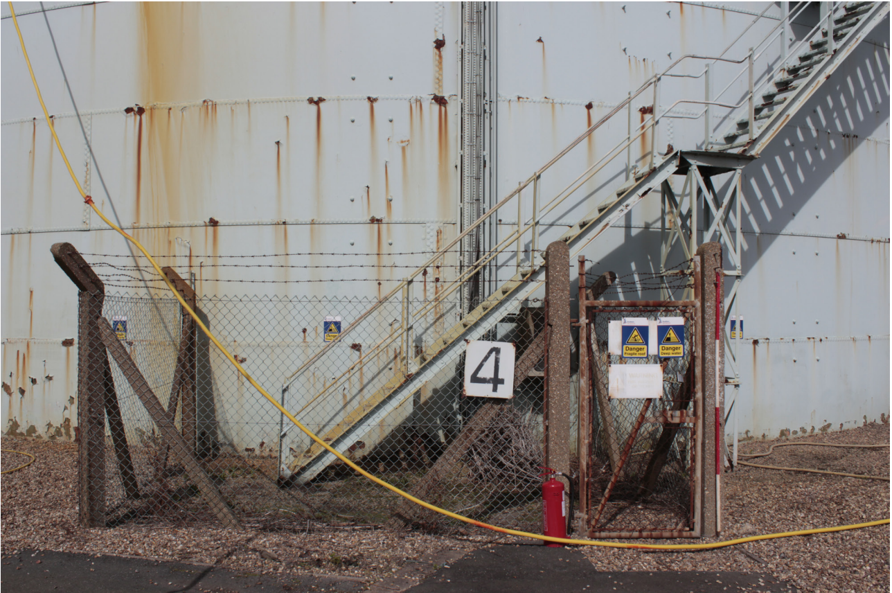
Plate 11: Gasholder No 4, detail of the base of the stair from the south
