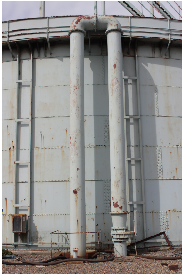
Plate 25: Gasholder No 5, detail of pipes on the north-east side from the north-east
