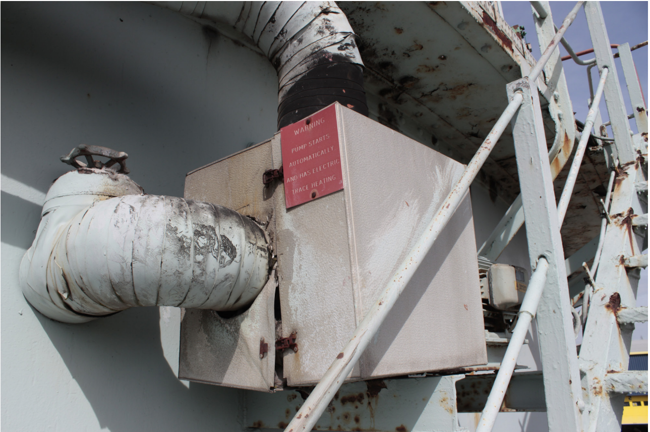
Plate 13: Gasholder No 4, detail of electric motor and pump at the top of the stair from the south-west
