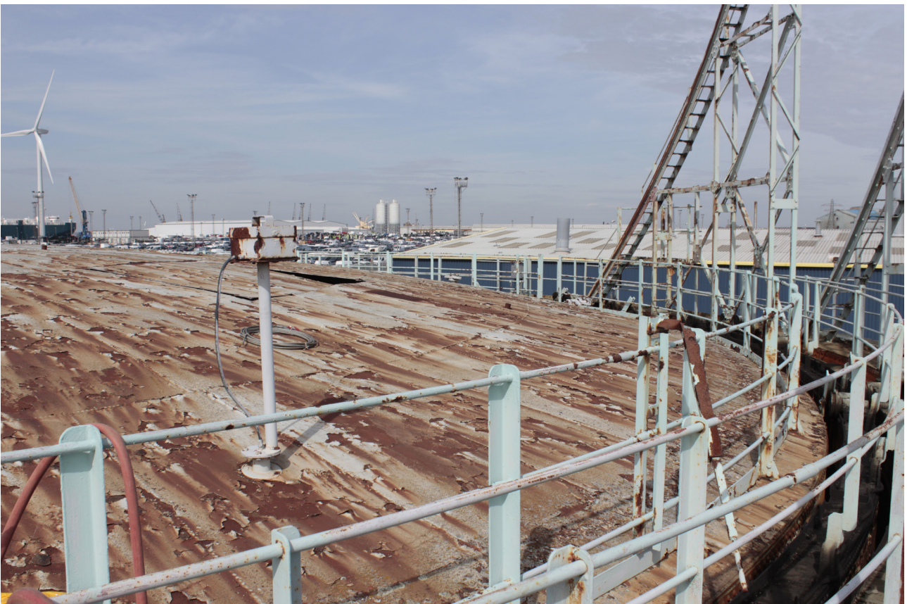
Plate 16: Gasholder No 4, general view of the top of the gasholder from the south
