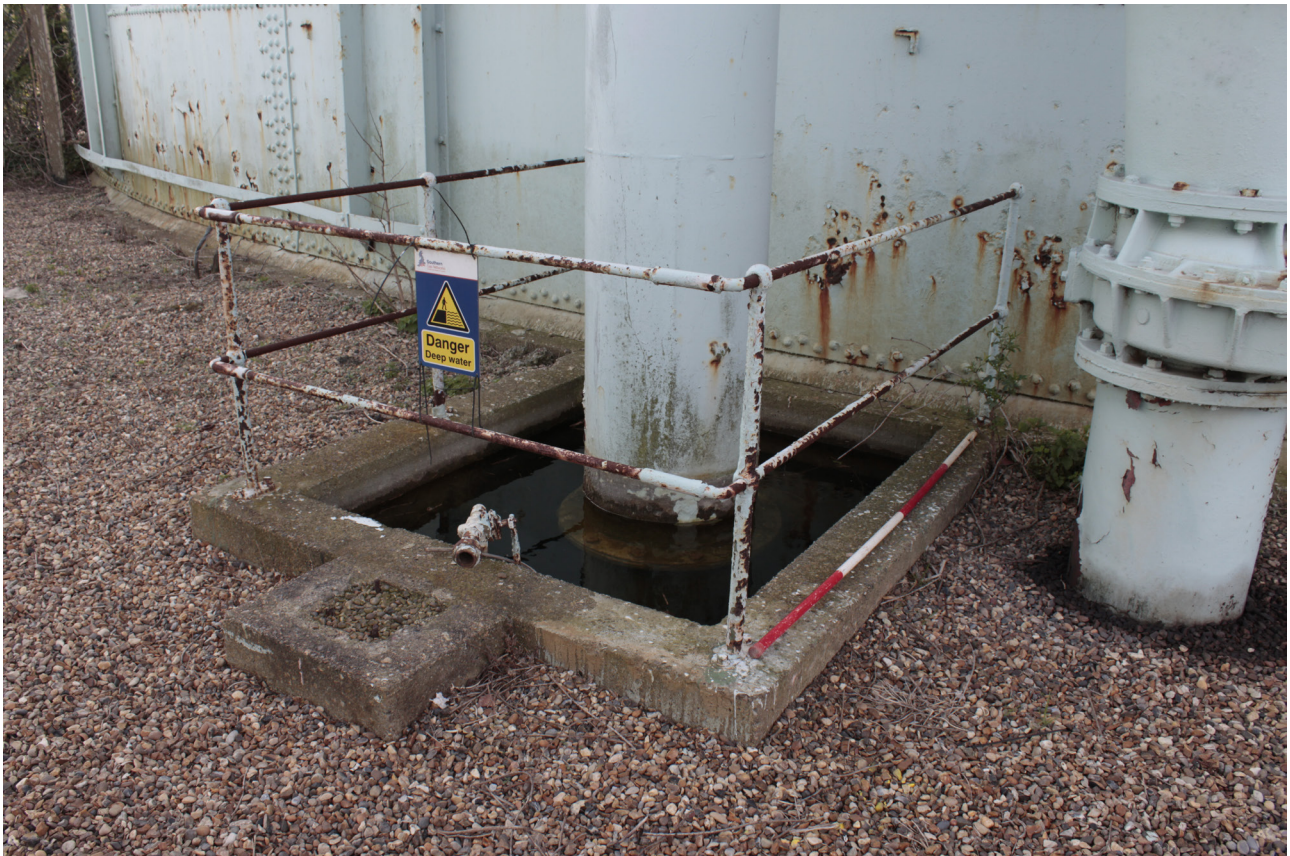
Plate 26: Gasholder No 5, detail of small compound for pipe on the north-east side from the north
