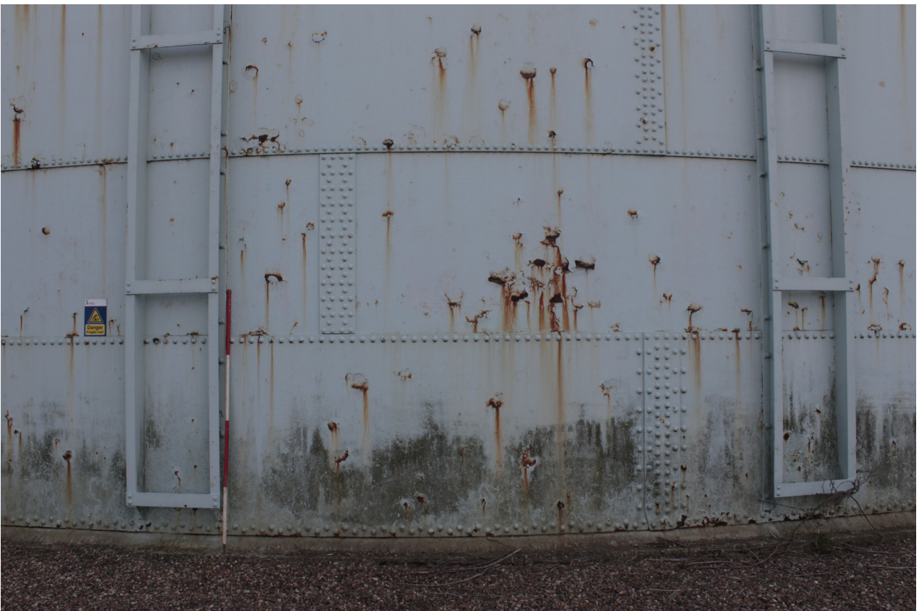
Plate 22: Gasholder No 5, detail of the steel construction and stanchions from the north
