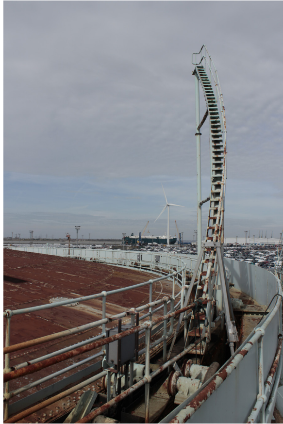
Plate 33: Gasholder No 5, general view of the top of the gasholder from the south
