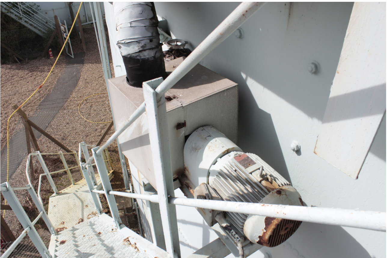
Plate 12: Gasholder No 4, detail of electric motor and pump at the top of the stair from the south-east
