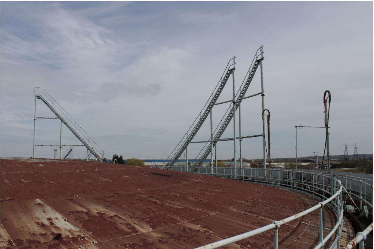
Plate 32: Gasholder No 5, general view of the top of the gasholder from the north
