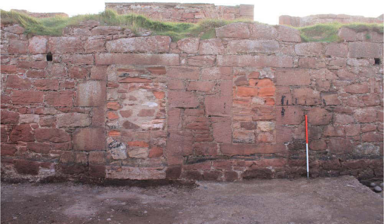
Plate 24: The Hospital building, south-east elevation, detail of the central blocked doorways from the north-west
