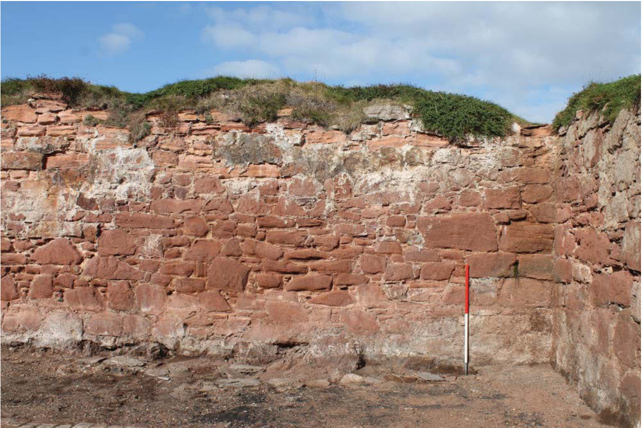
Plate 29: The Hospital building, north-east elevation, general view of the south-east side from the south-west
