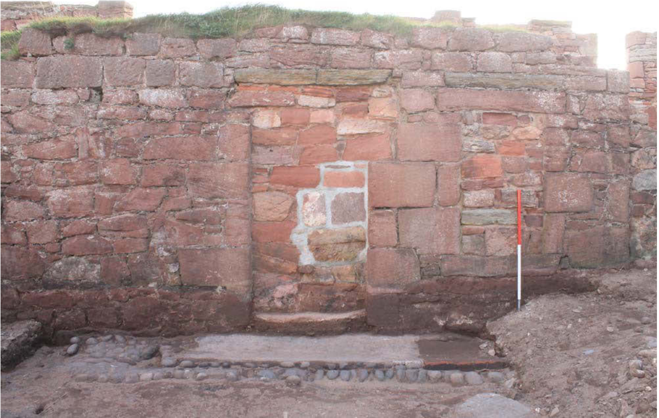
Plate 25: The Hospital building, south-east elevation, detail of blocked doorways to the south-west side, from the north-west
