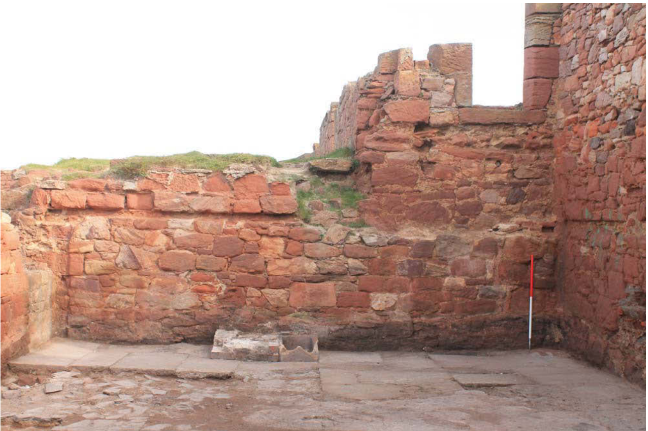
Plate 48: The Fumigation House, general view of the north-east wall from the south-west
