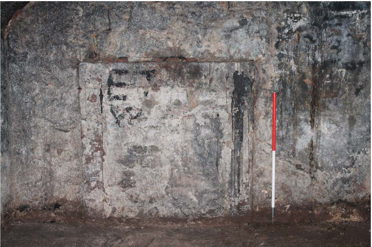
Plate 16: Vault 3, detail of the blocked fireplace in the south-west wall, from the north-east
