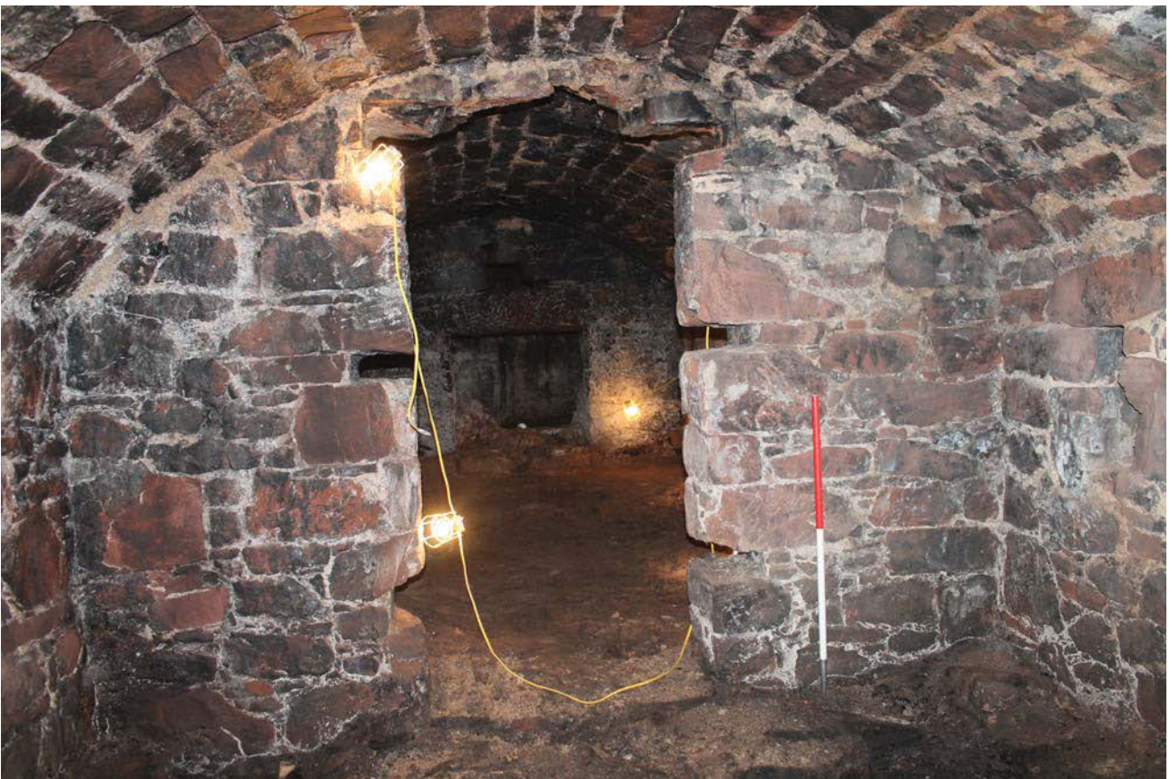
Plate 6: Vault 1, general view of the south-west wall showing doorway to Vault 2, from the north-east
