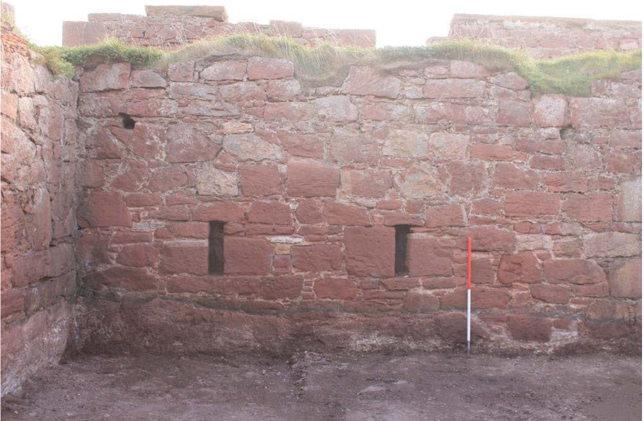
Plate 23: The Hospital building, south-east elevation, detail of the slit windows to the north-east side, from the north-west
