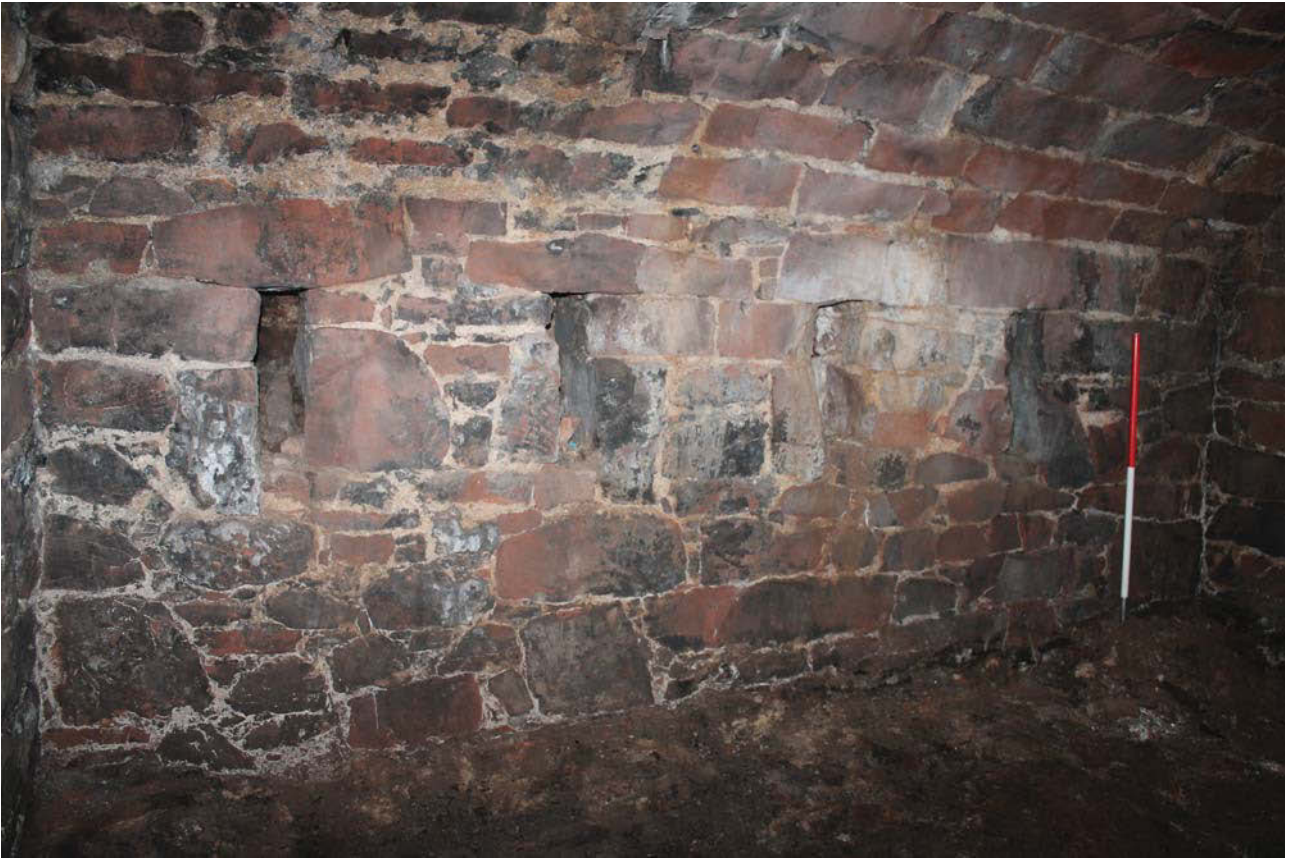
Plate 3: Vault 1, general view of the slit windows in the north-west wall from the south
