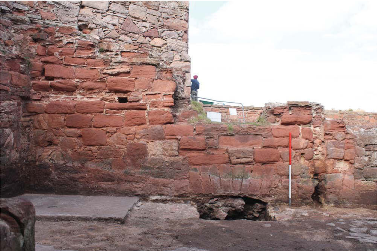
Plate 39: The Fumigation House, north-west elevation, general view to the south-west side from the south-east
