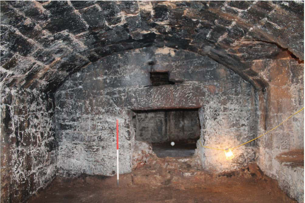
Plate 11: Vault 2, general view of the south-west wall showing the doorway to Vault 1, from the north-east
