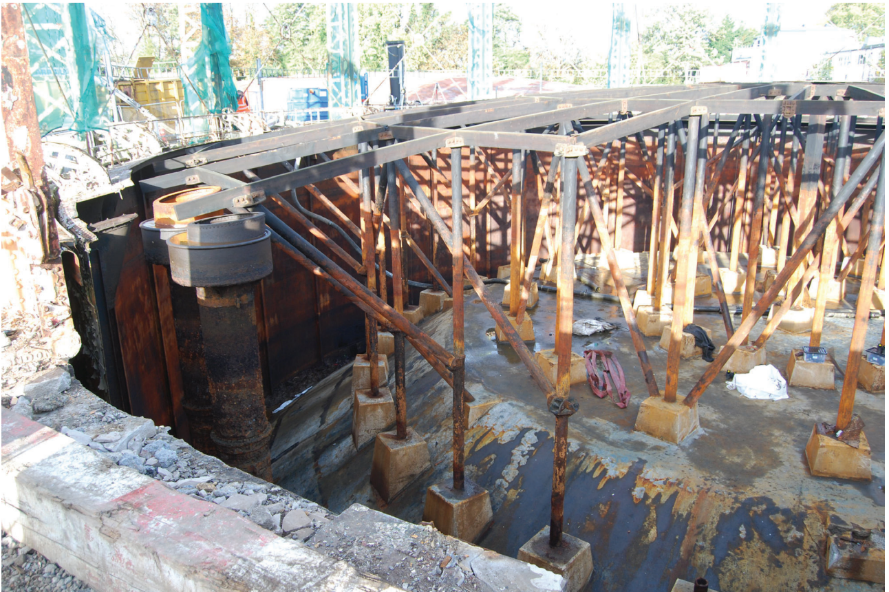
Plate 16: Gasholder No 5, detail of the dumping and crown framing support, from the SSE
