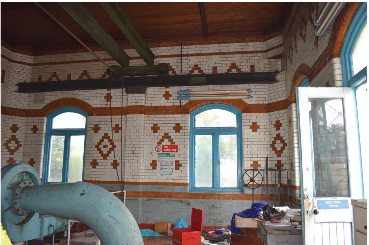
Plate 44: Building E, Booster House, general view of the interior from the north-west
