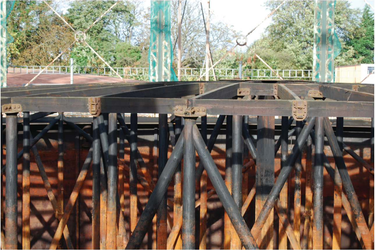
Plate 25: Gasholder No 5, close detail of the exposed timber crown framing, from the south
