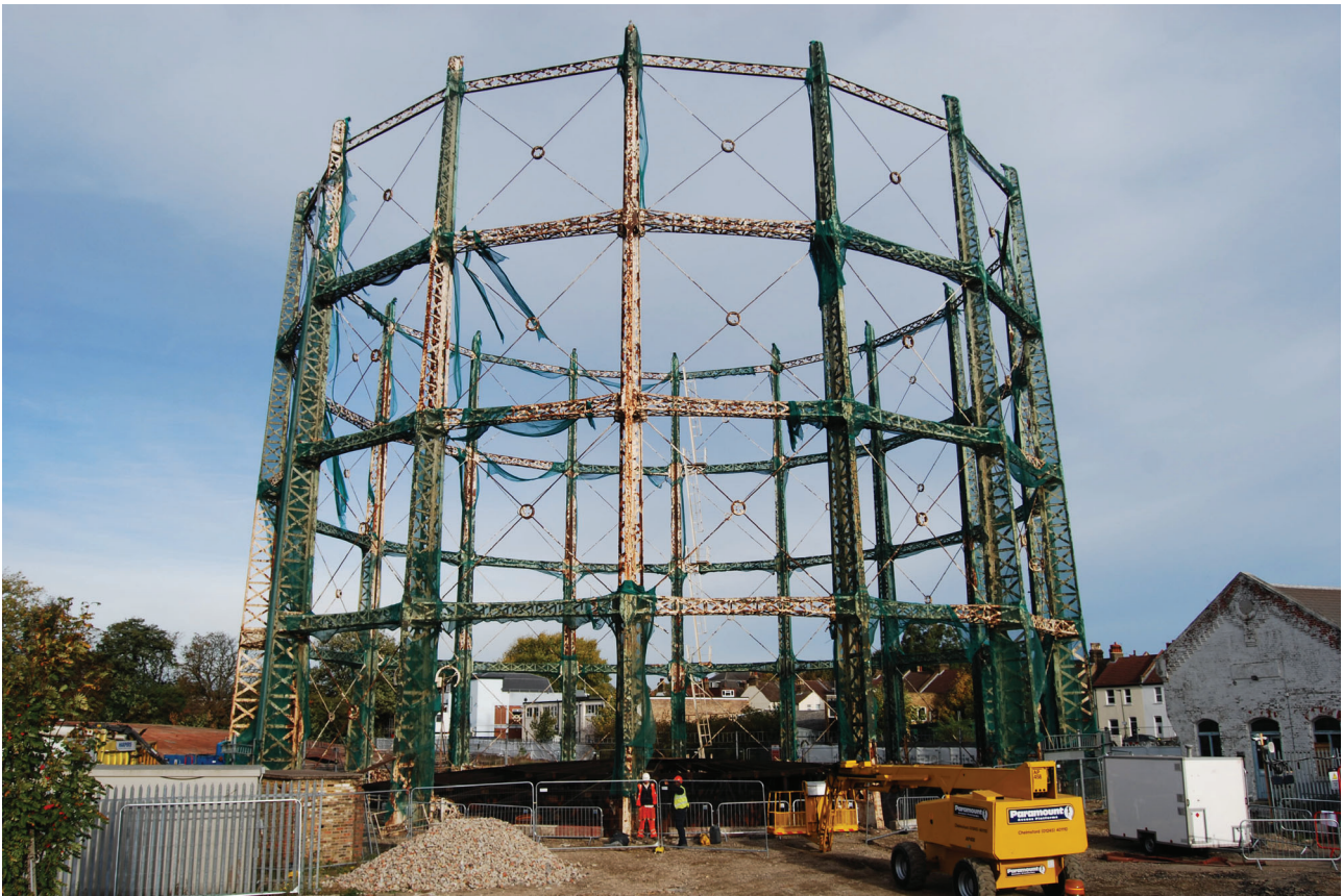
Plate 10: Gasholder No 5, general view of the gasholder after part-demolition, from the south
