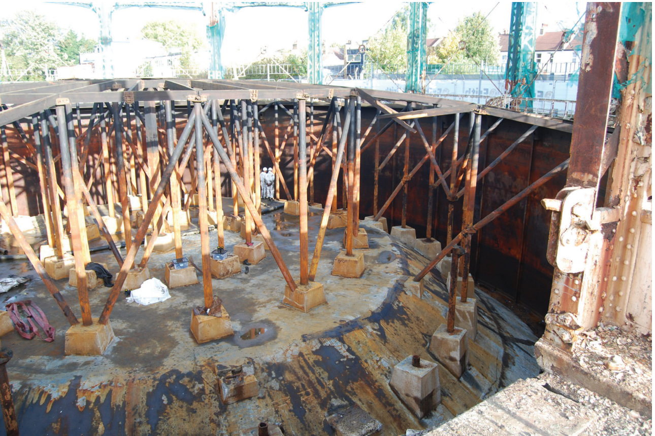
Plate 14: Gasholder No 5, detail of the dumping and crown framing support, from the SSW
