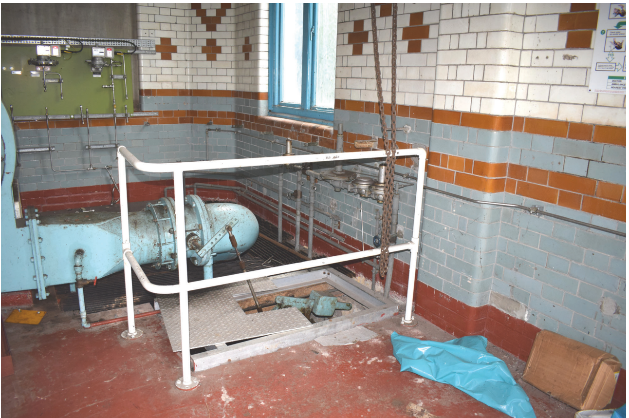
Plate 46: Building E, Booster House, general view of interior showing pipework from the south-west
