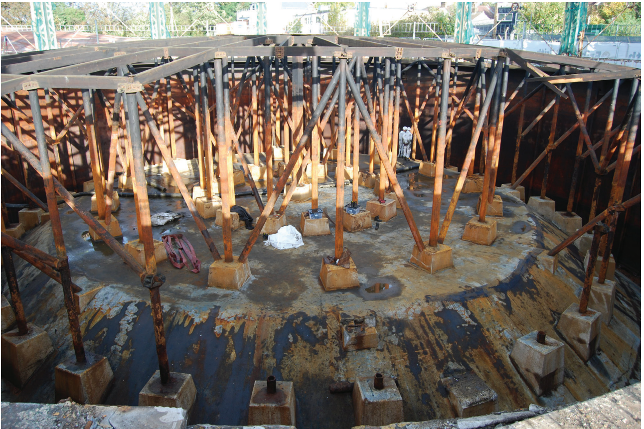
Plate 15: Gasholder No 5, detail of the dumping and crown framing support, from the south
