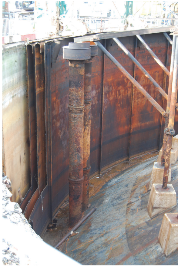
Plate 19: Gasholder No 5, detail of the inlet/outlet gas pipe adjacent to the inside of the exposed inner side of the lower lift, from the SSE
