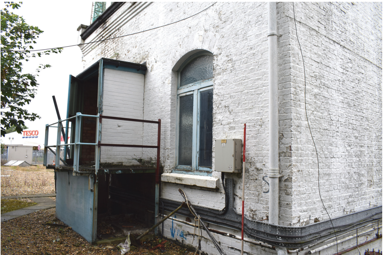
Plate 42: Building E, Booster House, general view of the south-east elevation from the east
