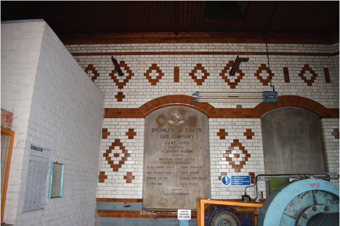
Plate 47: Building E, Booster House, general view of the interior north-east wall from the south-west
