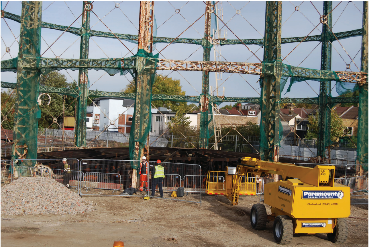
Plate 11: Gasholder No 5, general view of the gasholder after part-demolition, from the south
