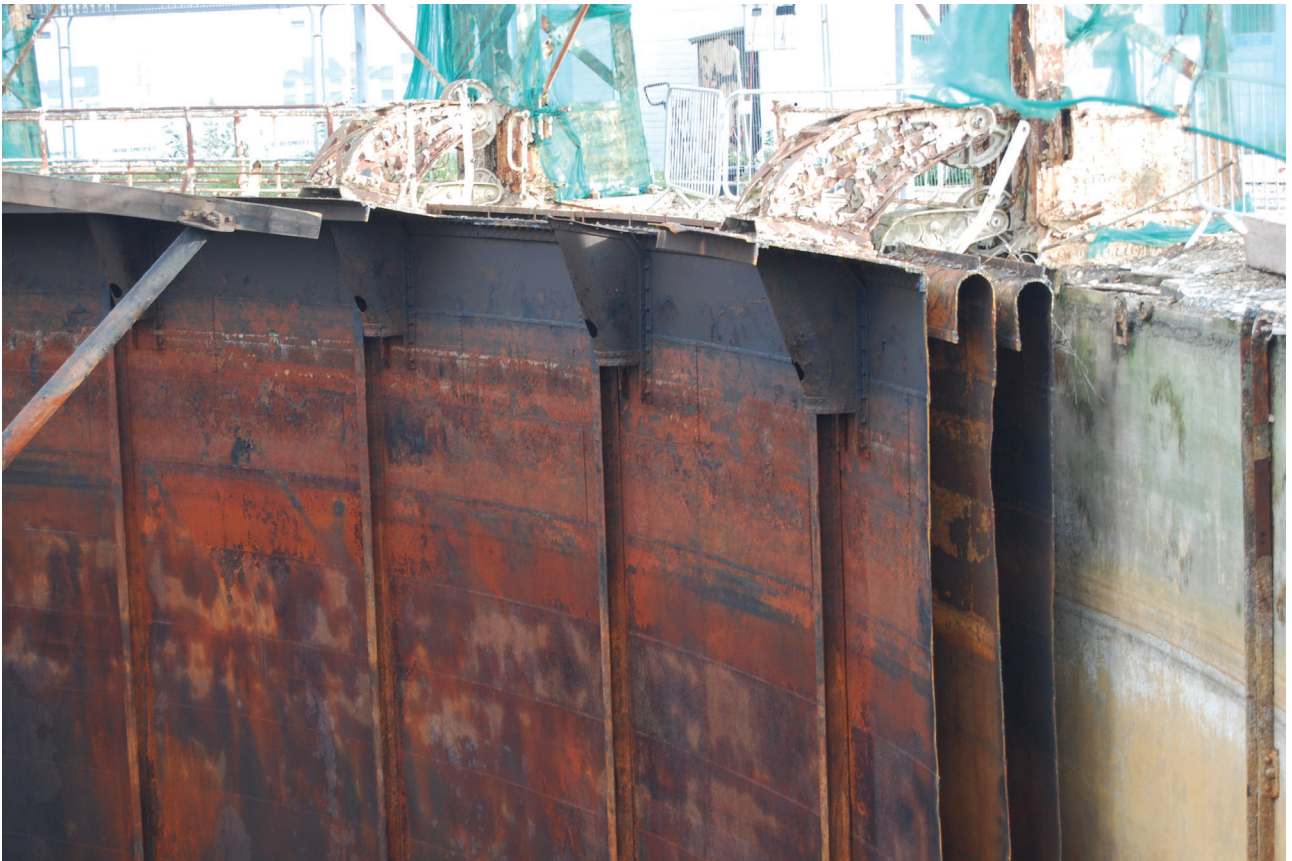
Plate 21: Gasholder No 5, detail of the exposed inner walls of the lower lift, from the SSW
