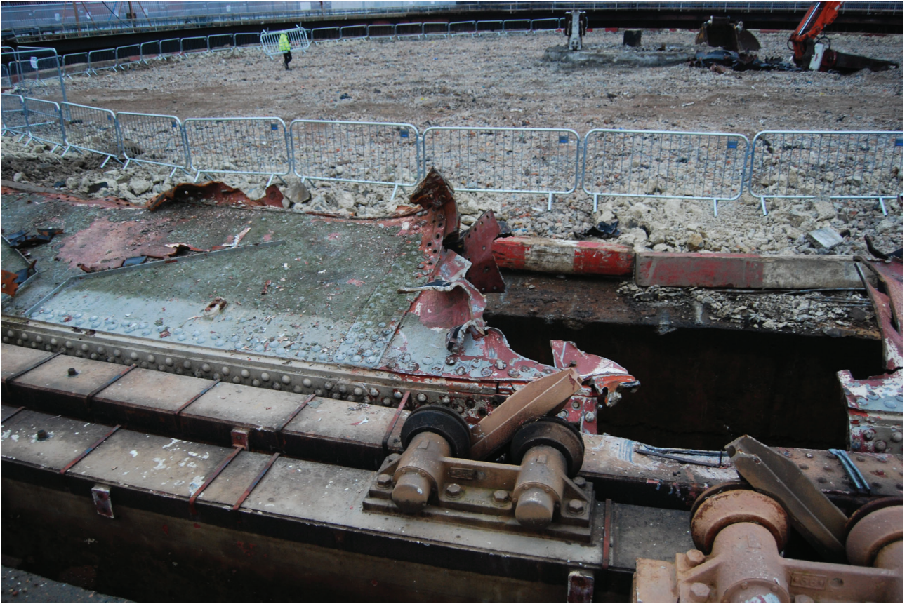
Plate 37: Gasholder No 4, detail of the broken-away lift and exposed tank after demolition, from the ENE
