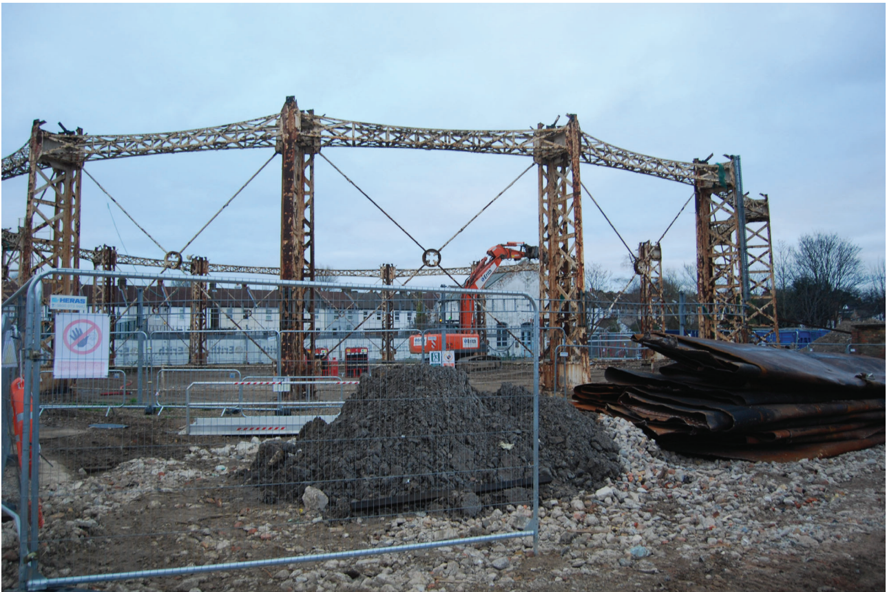
Plate 12: Gasholder No 5, general view of the gasholder after part-demolition, from the south-west
