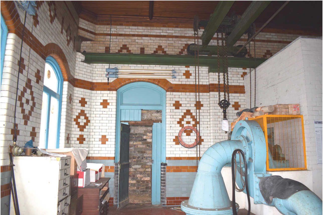
Plate 45: Building E, Booster House, general view of the interior from the south-east
