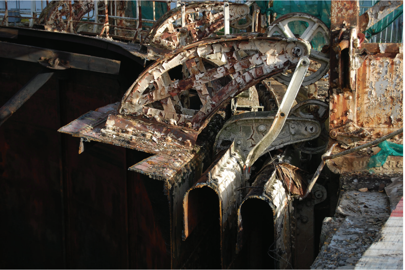
Plate 13: Gasholder No 5, detail of the guided rollers after part-demolition, from the south-west
