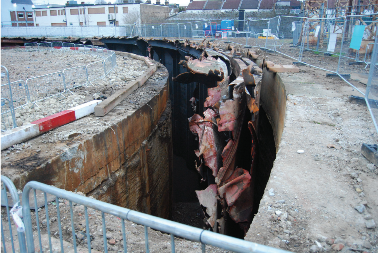
Plate 35: Gasholder No 4, detail of the broken-away lift and exposed tank after demolition, from the south
