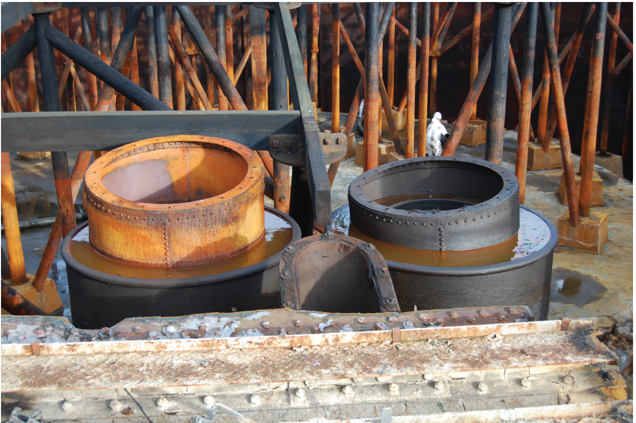
Plate 18: Gasholder No 5, close detail of the inlet/outlet gas pipe to the side of the tank, from the south
