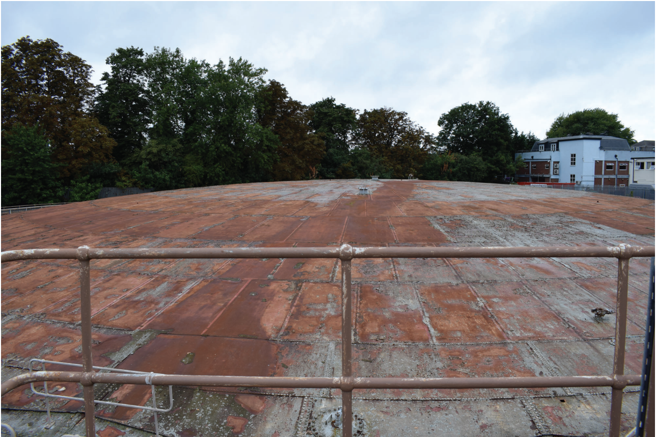
Plate 29: Gasholder No 4, general view of the crown of the gasholder from the south-east
