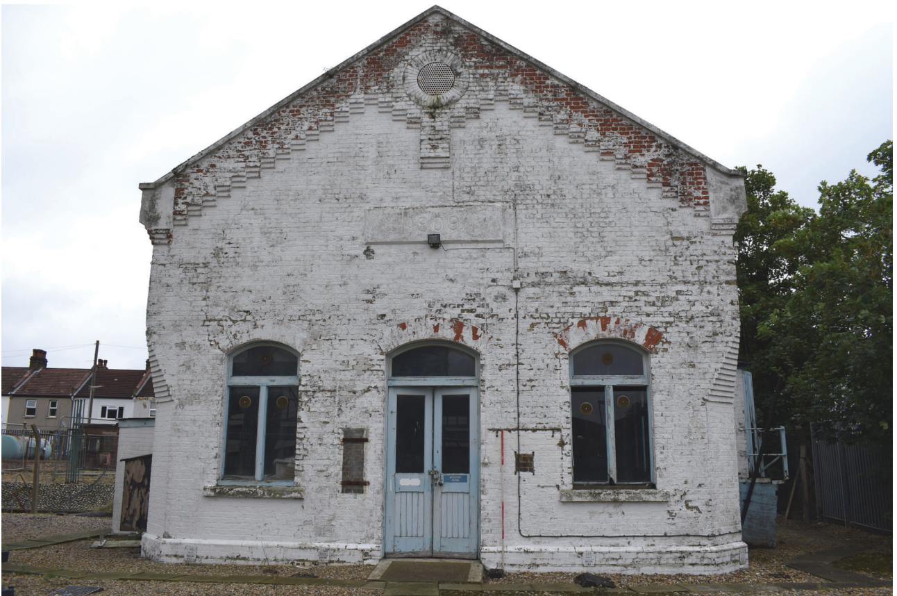
Plate 40: Building E, Booster House, general view of the south-west elevation from the south-west
