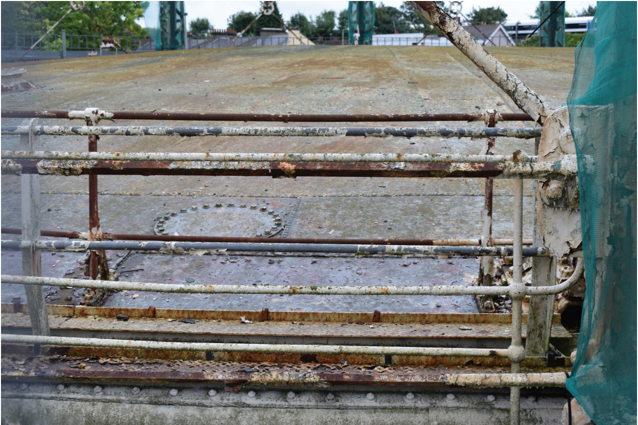
Plate 7: Gasholder No 5, detail of the riveted panel on the crown of the gasholder, from the north-west
