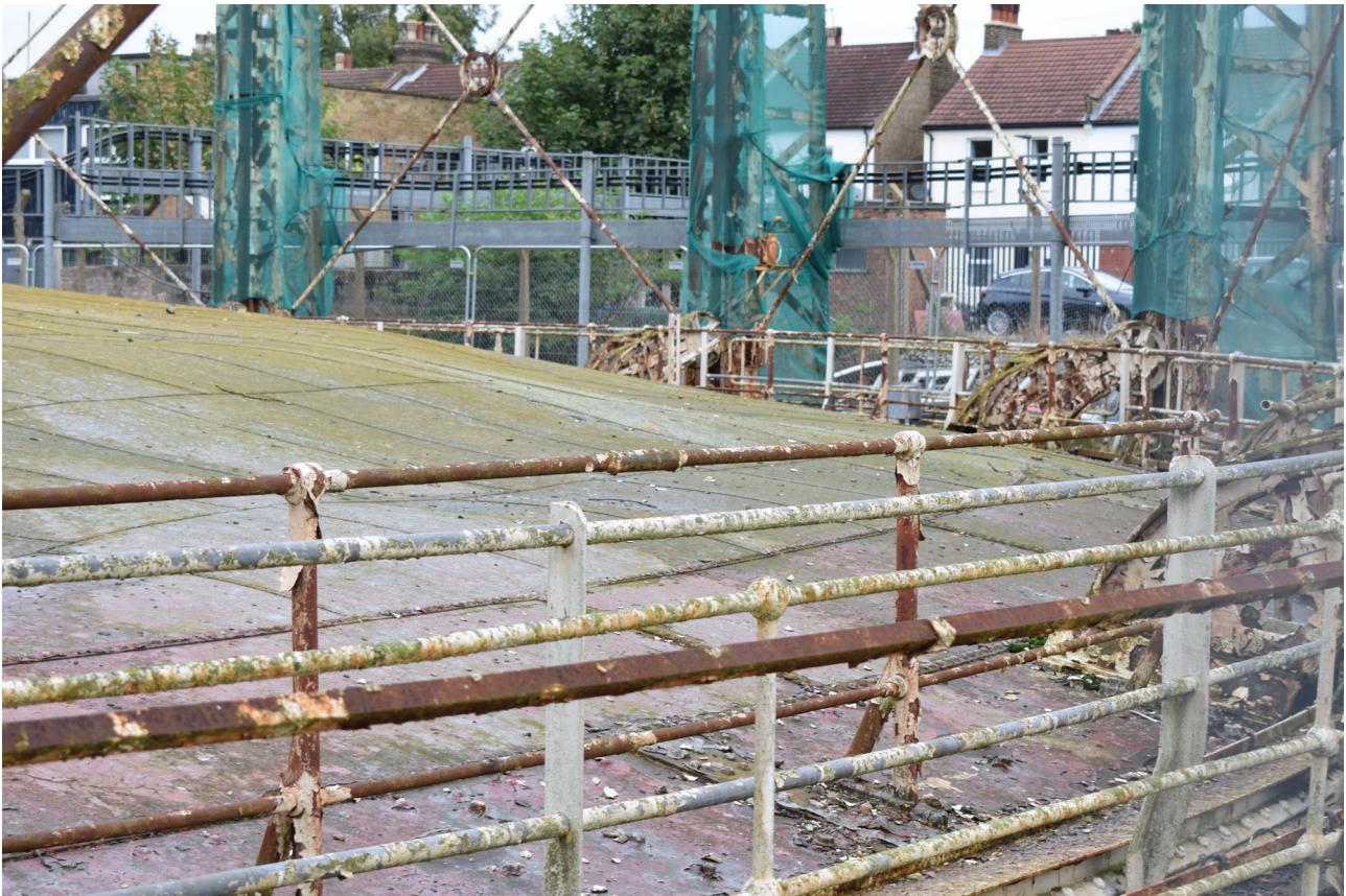
Plate 8: Gasholder No 5, detail of the hand rail to the south-east of the gasholder, from the south-east
