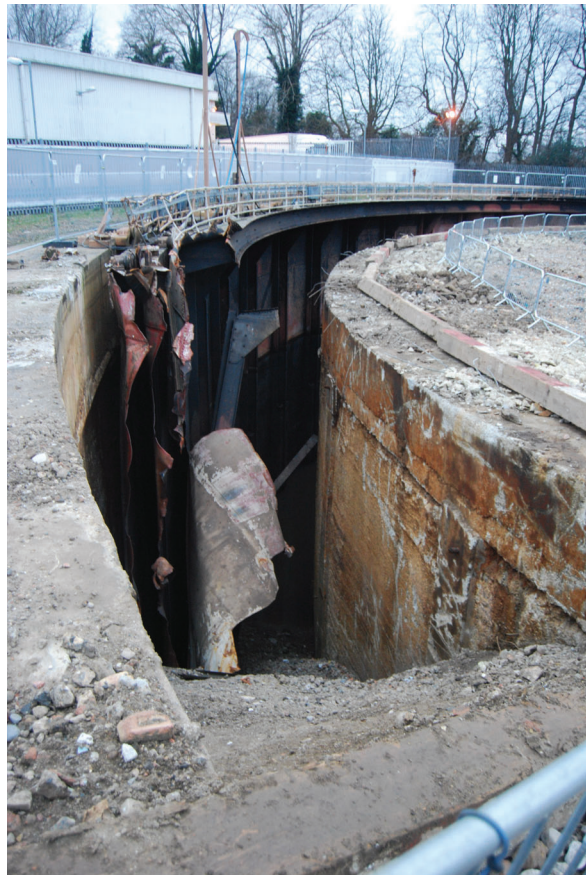
Plate 36: Gasholder No 4, detail of the broken-away lift and exposed tank after demolition, from the south-west
