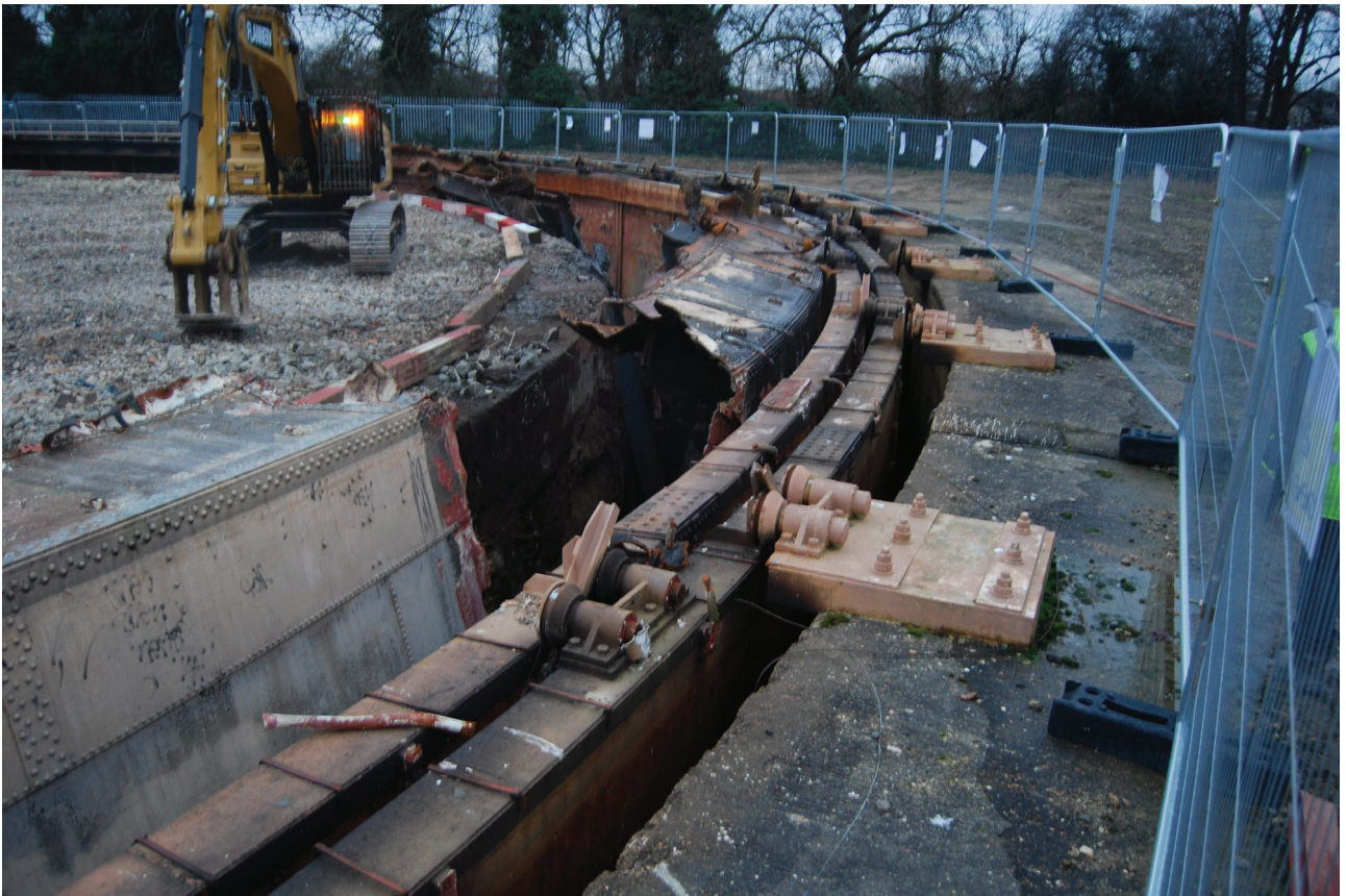
Plate 38: Gasholder No 4, detail of the broken-away lift and exposed tank after demolition (including guided rollers), from the south
