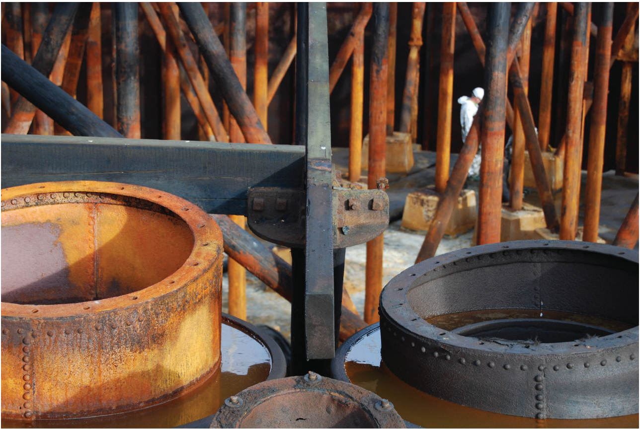
Plate 27: Gasholder No 5, close detail of the exposed timber crown framing, from the south
