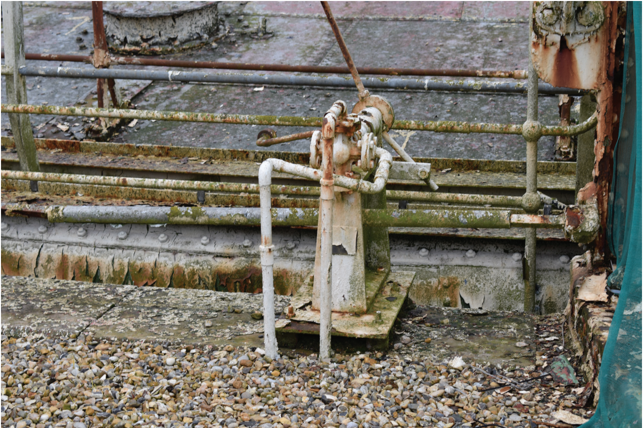
Plate 9: Gasholder No 5, detail of knock-off switch adjacent to the south-east side of the gasholder, from the south-east
