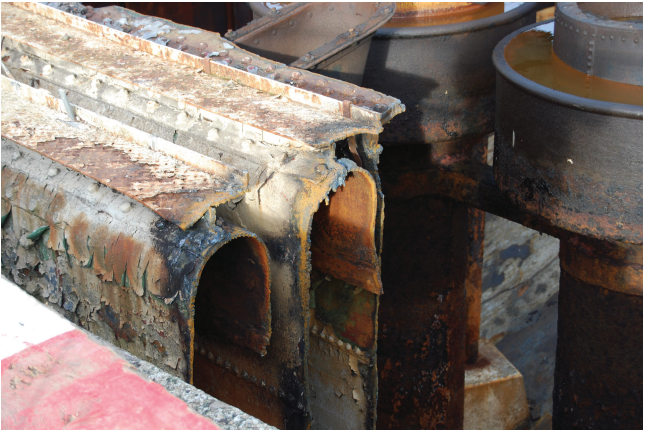
Plate 22: Gasholder No 5, close detail of the broken-away lifts from the SSE
