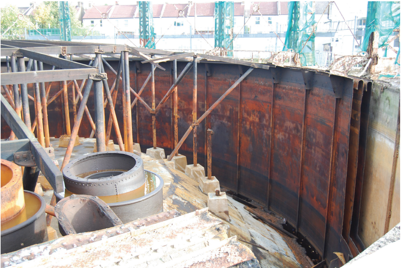
Plate 20: Gasholder No 5, detail of the exposed inner walls of the lower lift, from the SSW
