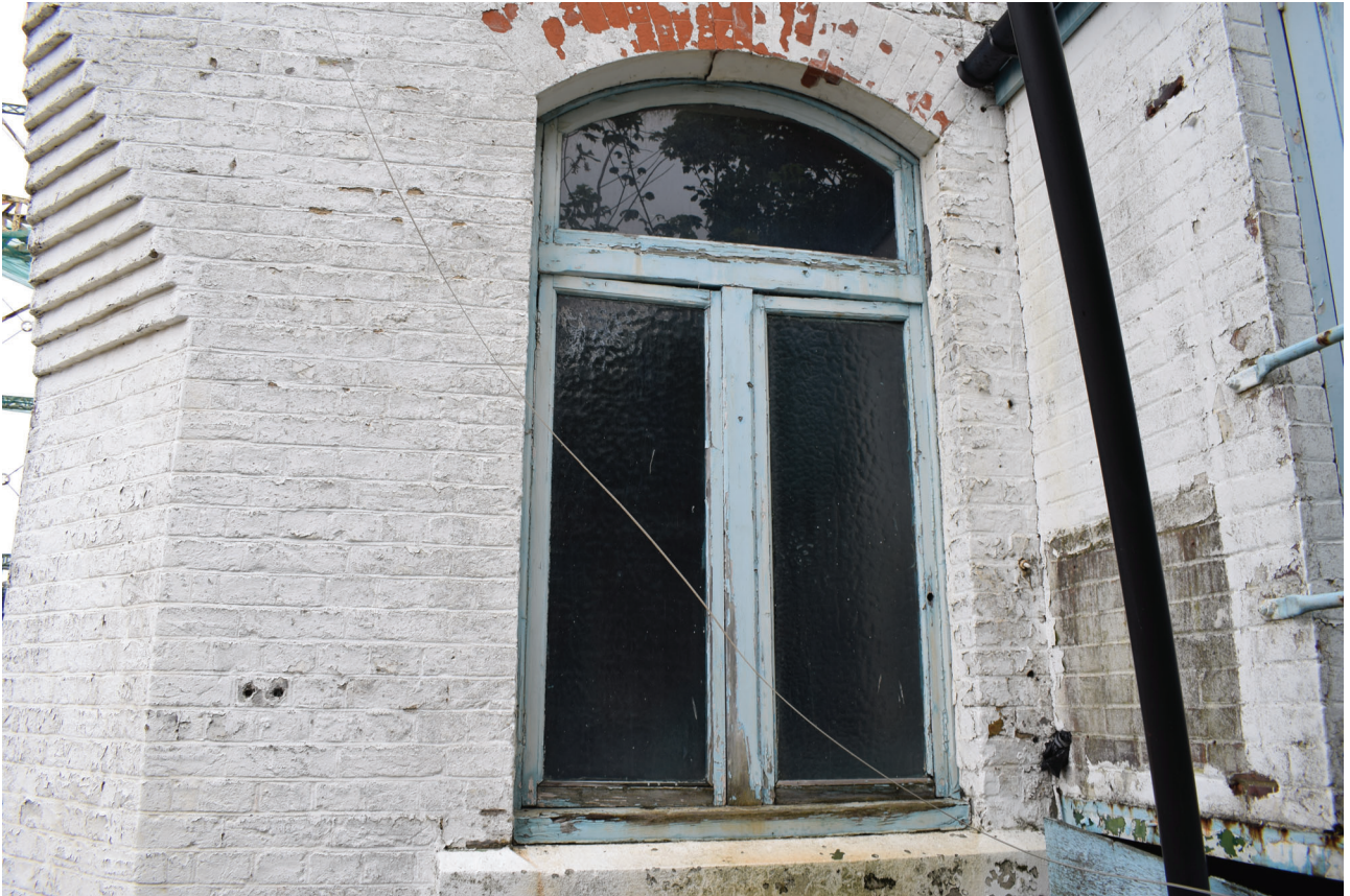
Plate 43: Building E, Booster House, detail of window to the south-west side of the south-east elevation, from the south-east
