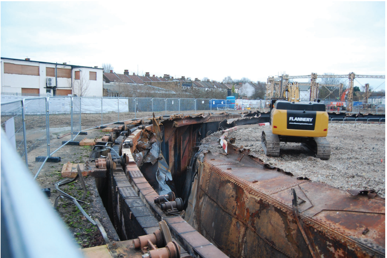
Plate 39: Gasholder No 4, detail of the broken-away lift and exposed tank after demolition (including guided rollers), from the north-west
