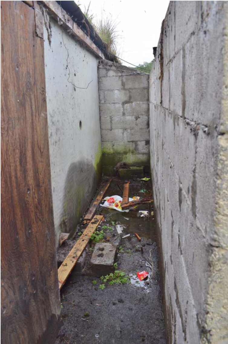
Plate 28: Image of interior of projecting concrete block fixture B4 on southeast exterior wall of B2, looking northeast
