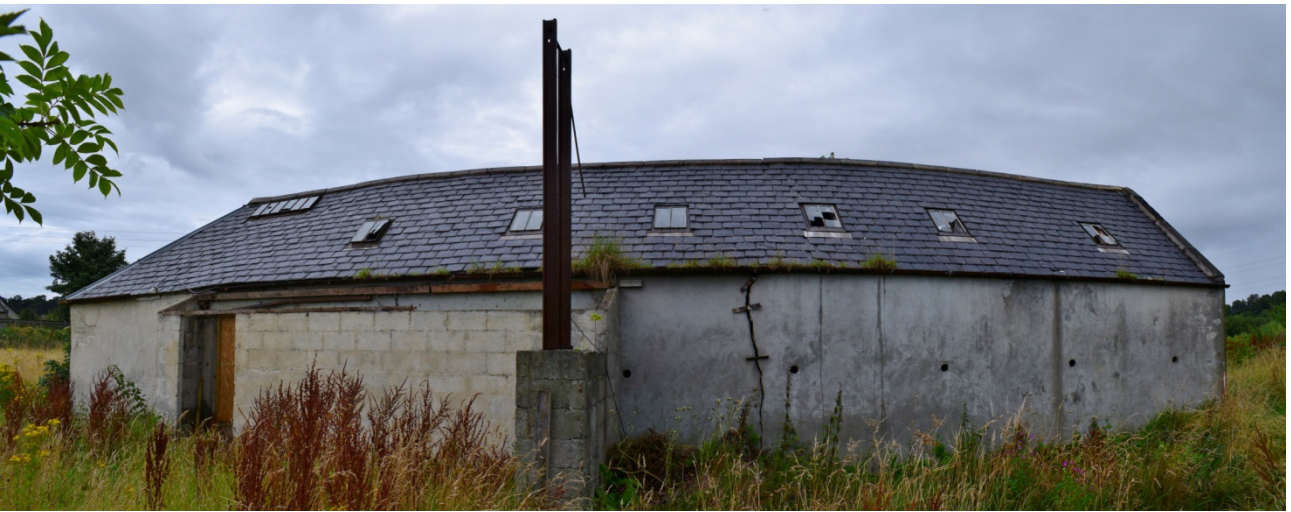
Plate 19: Image of south exterior wall of steading B2, showing B4 to the left
