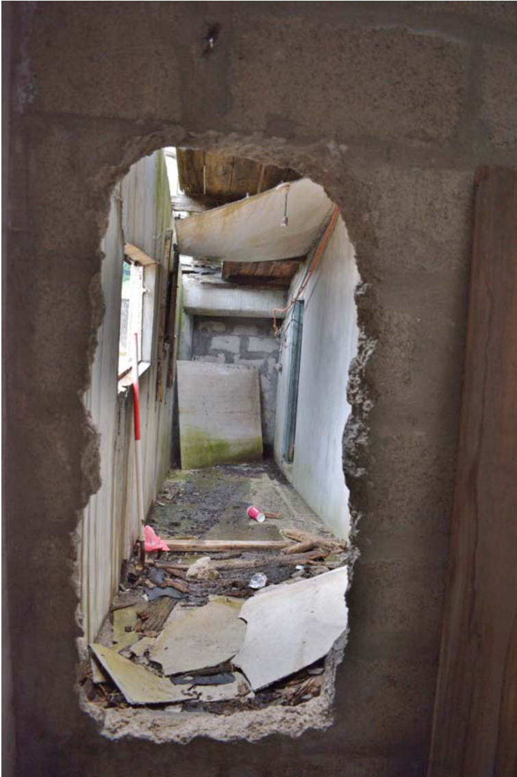
Plate 30: Close up of hole in northeast interior wall of A1, leading through to D
