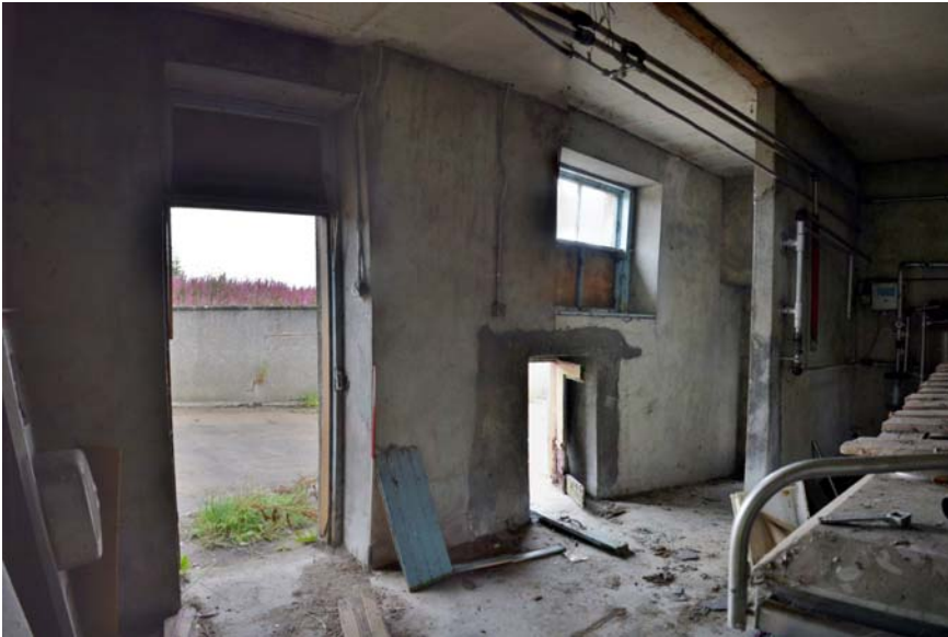
Plate 6: Northwest interior wall of pasteurisation room A1, concrete block partition visible to the right of image
