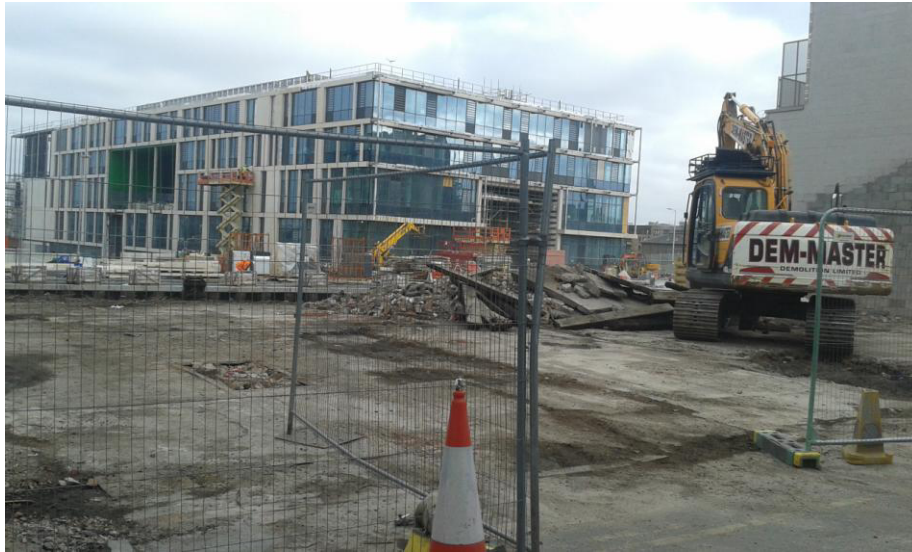
Plate 3 – General view of the Development area showing floor slab of former industrial building
