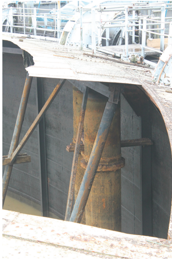
Plate 49: Bell Green, Sydenham, Gasholder No 8, detail view of the inlet/outlet pipe, from the south-west
