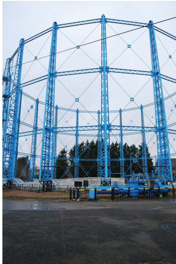
Plate 3: Bell Green, Sydenham, Gasholder No 7, general view of the gasholder frame from the east
