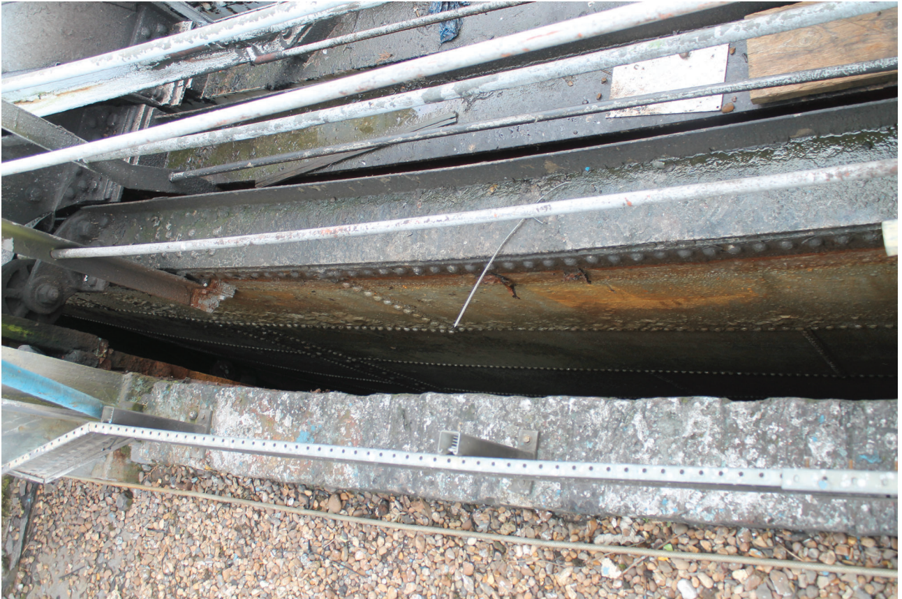
Plate 21: Bell Green, Sydenham, Gasholder No 7, general view of the tank wall, from the south
