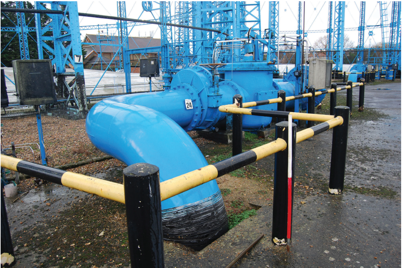
Plate 27: Bell Green, Sydenham, Gasholder No 7, general view of the pipework to the east of the gasholder from the south-east
