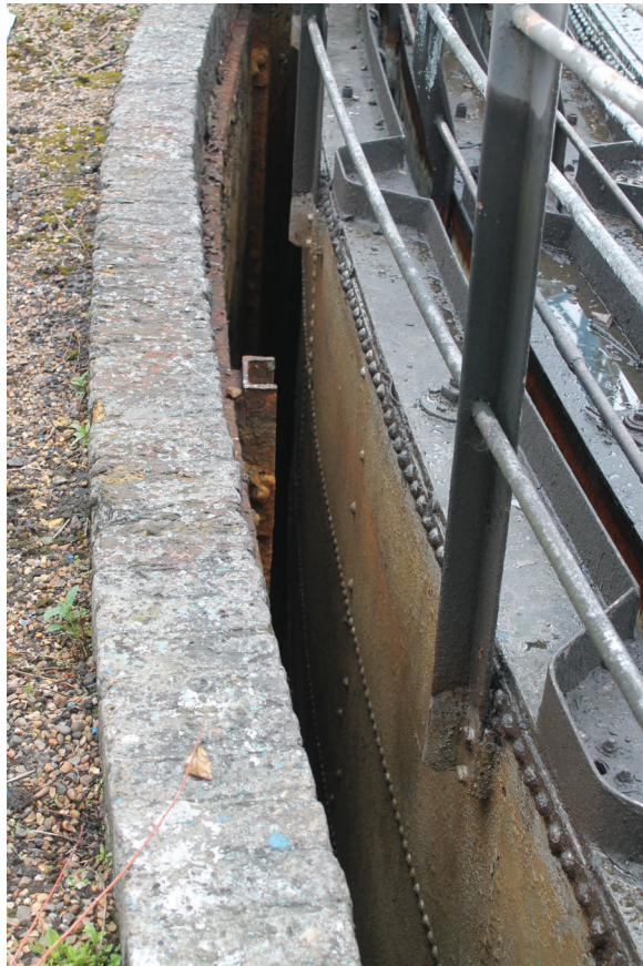
Plate 42: Bell Green, Sydenham, Gasholder No 8, general view of the bell outer lift wall, from the east
