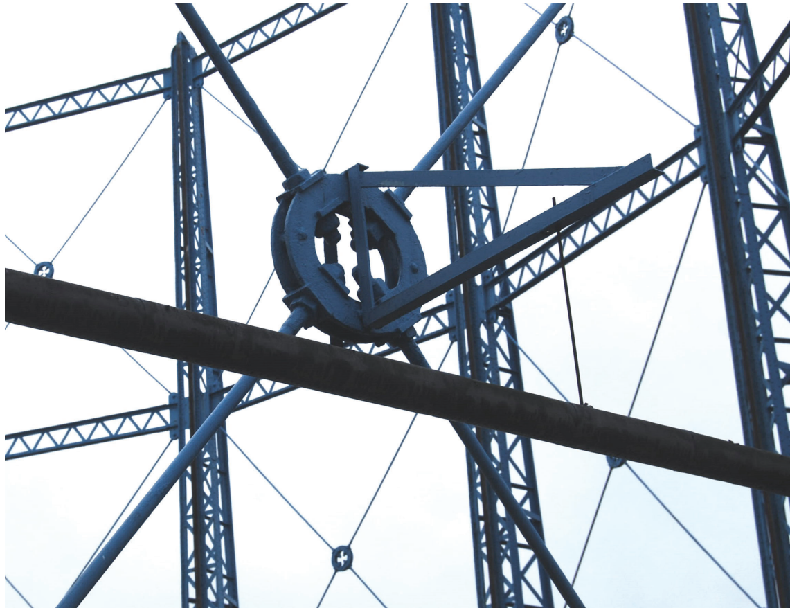
Plate 9: Bell Green, Sydenham, Gasholder No 7, detail of the diagonal bracing between No 13 and 14 standards from the NNE
