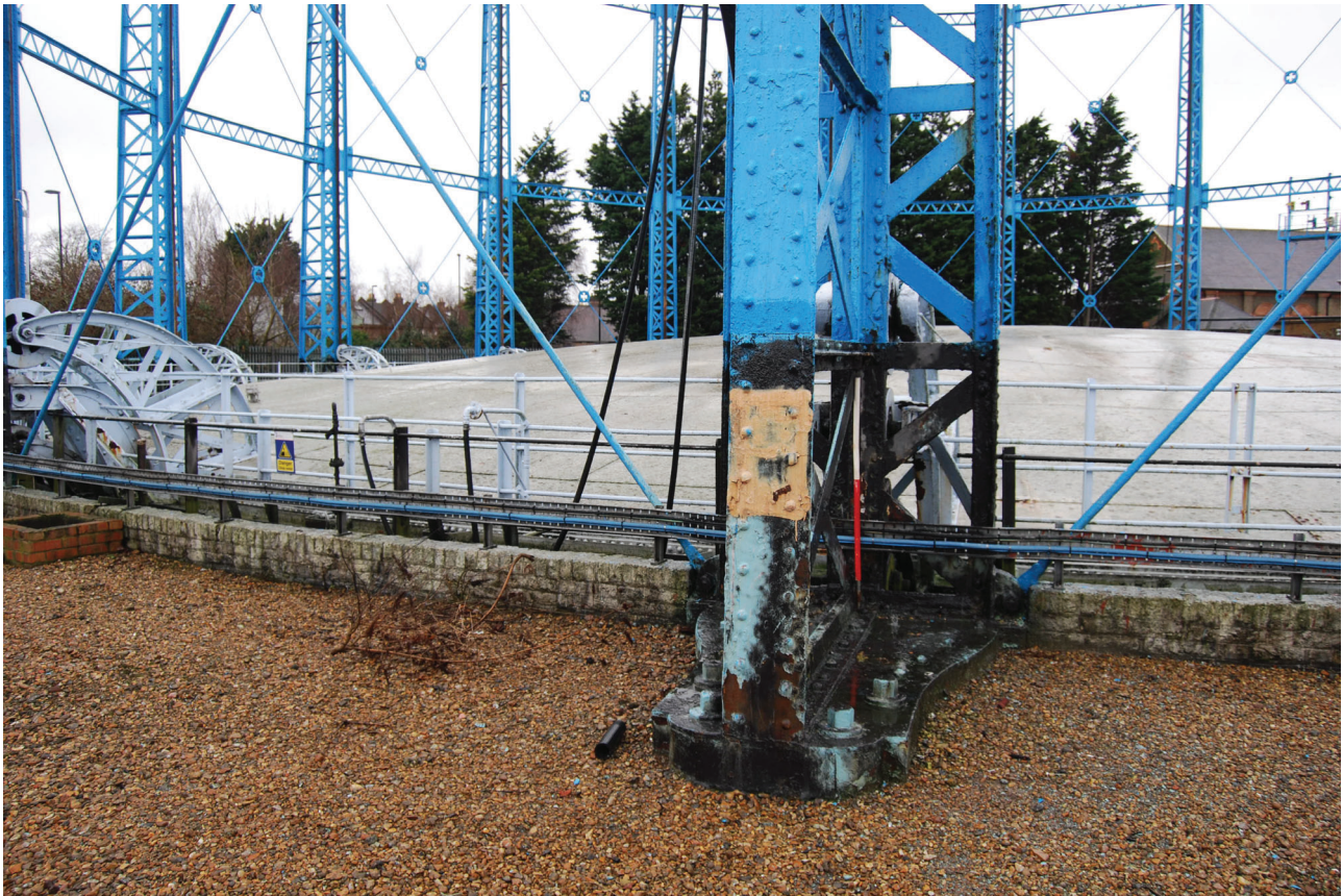
Plate 12: Bell Green, Sydenham, Gasholder No 7, detail of the base of No 2 standard from the east
