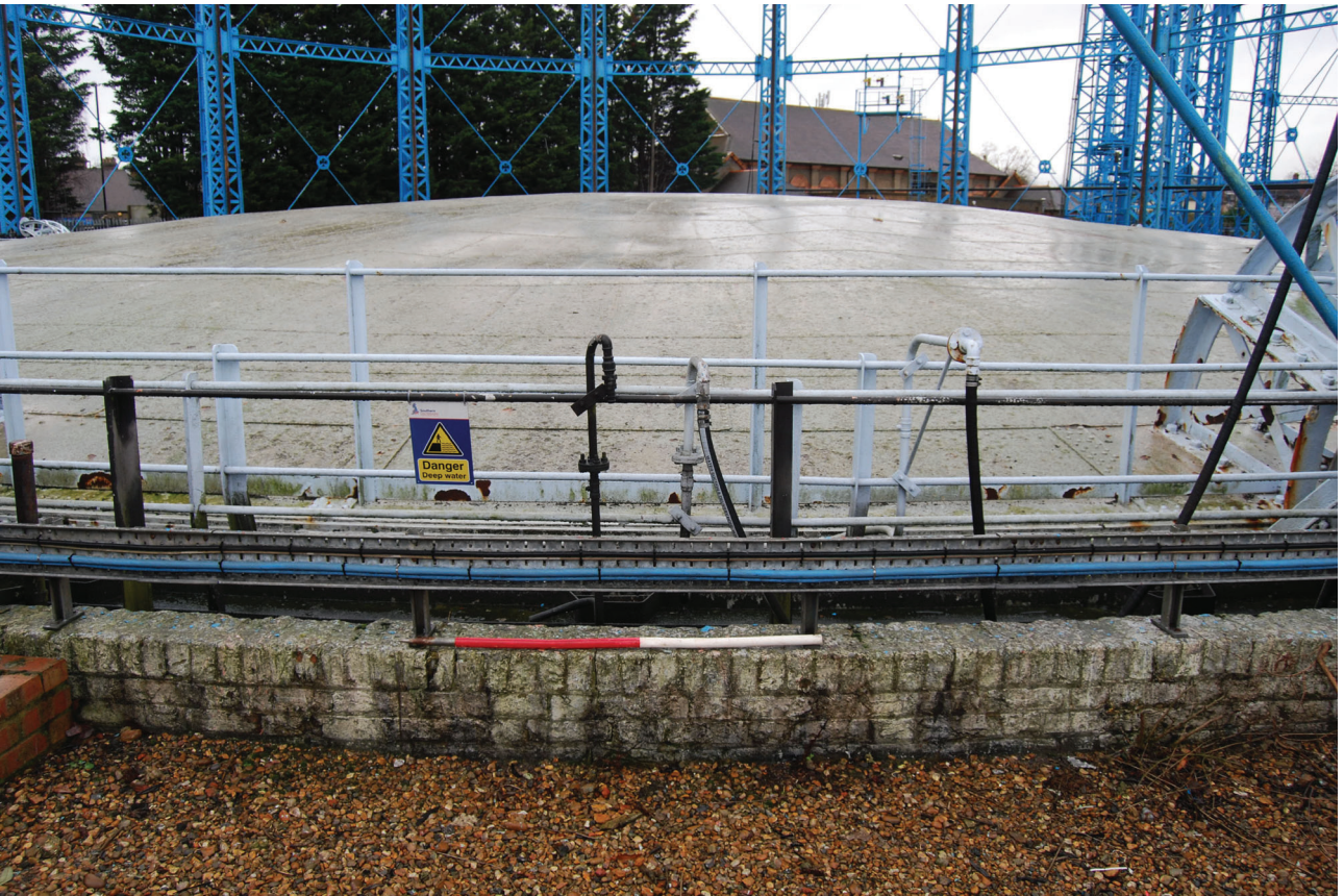
Plate 18: Bell Green, Sydenham, Gasholder No 7, general view of the crown of the gasholder from the south-east
