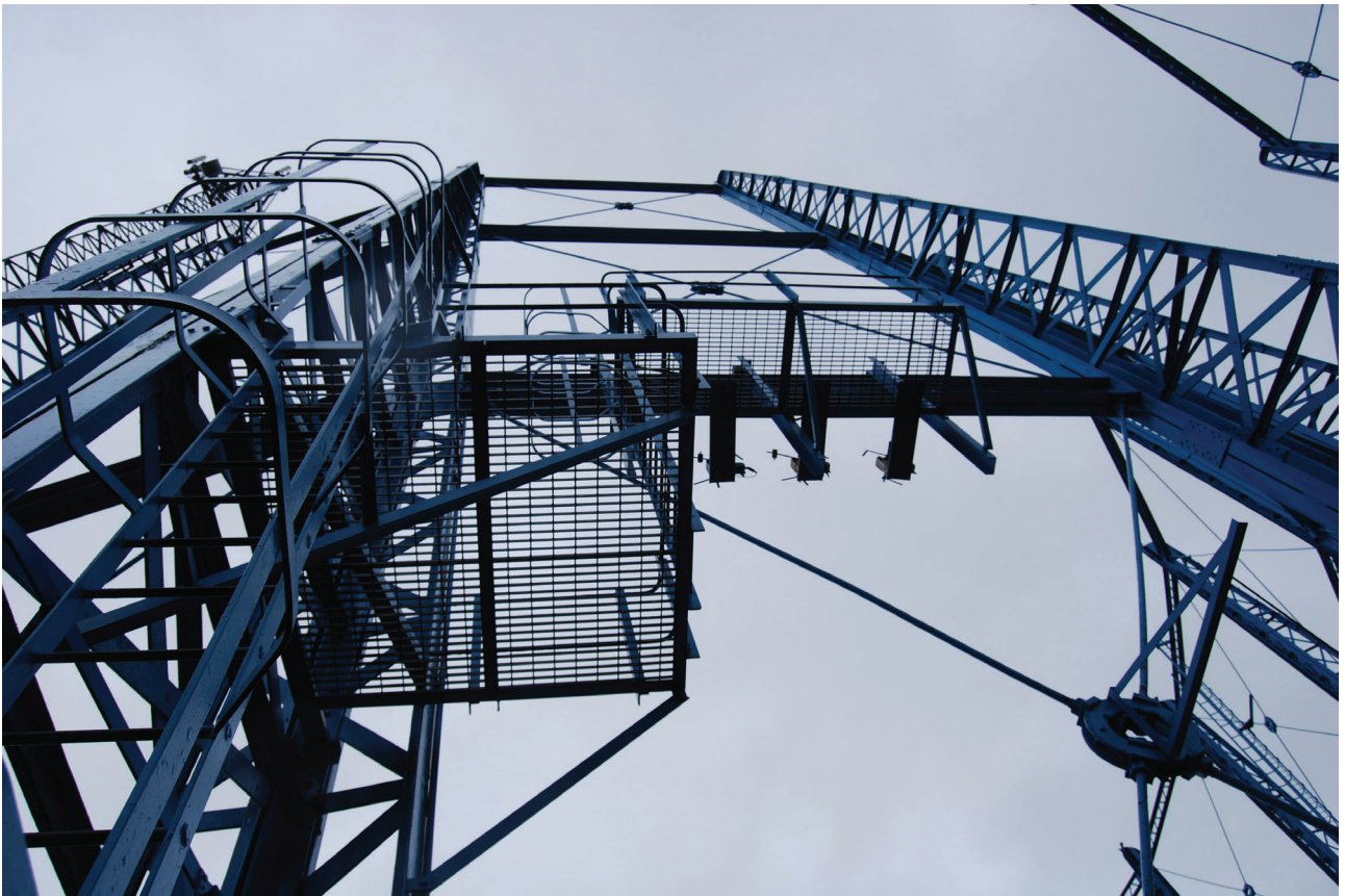
Plate 41: Bell Green, Sydenham, Gasholder No 8, general view looking up at the access ladders and gantries between No 4 and No 5 standards from the south-west
