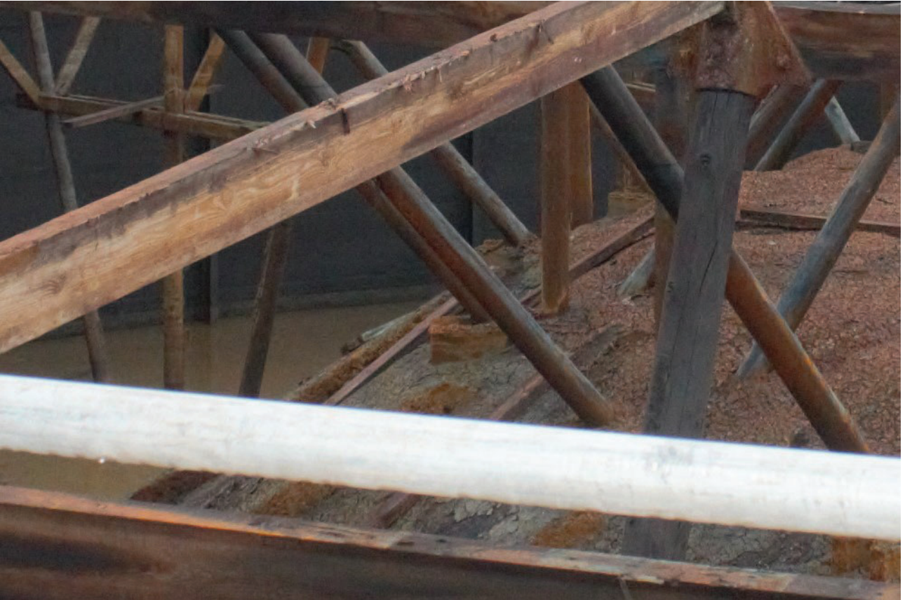
Plate 45: Bell Green, Sydenham, Gasholder No 8, detail view of the upright posts base within a concrete block, from the south-east
