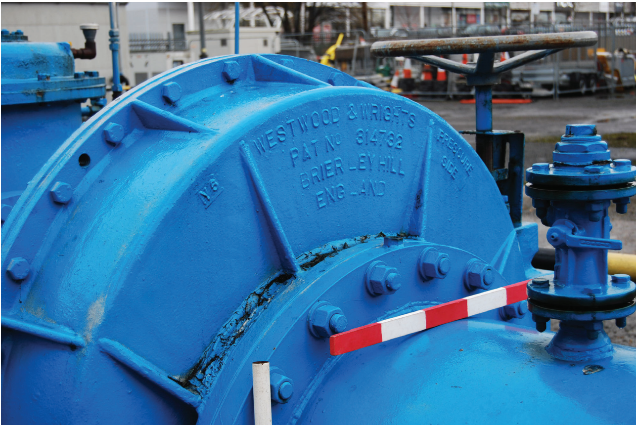
Plate 28: Bell Green, Sydenham, Gasholder No 7, close detail of the pipework to the east side of the gasholder, from the south-west
