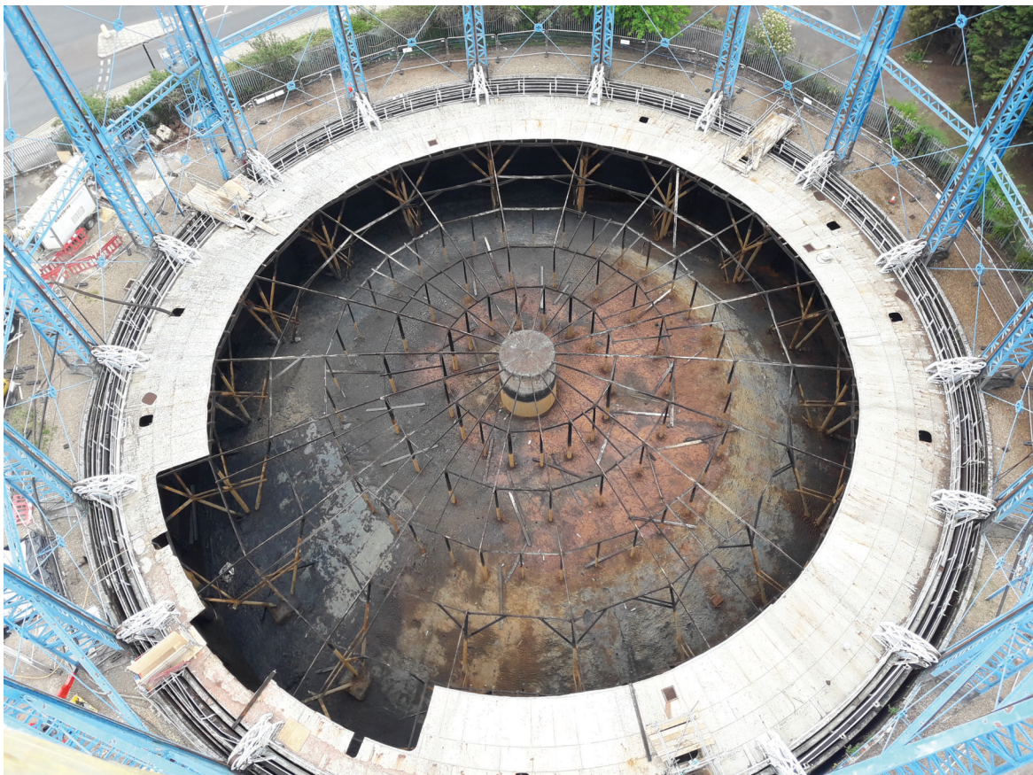
Plate 22: Bell Green, Sydenham, Gasholder No 7, general view of the crown rest frame, from the north © Keltbray
