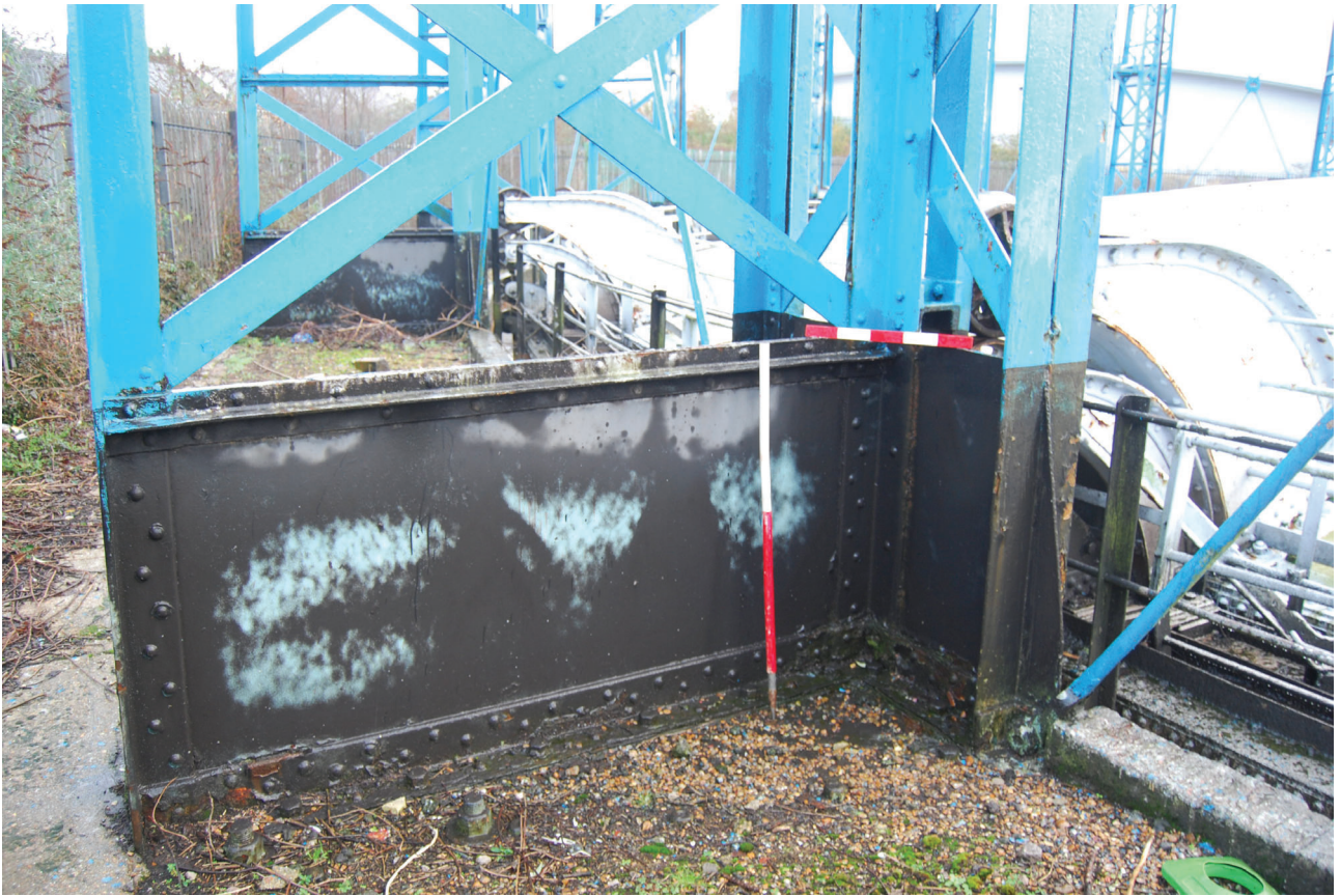
Plate 35: Bell Green, Sydenham, Gasholder No 8, detail of the foot of No 10 standard from the north
