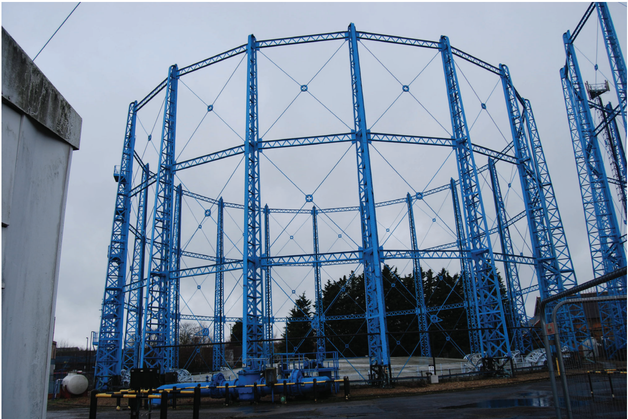
Plate 4: Bell Green, Sydenham, Gasholder No 7, general view of the gasholder frame from the ENE
