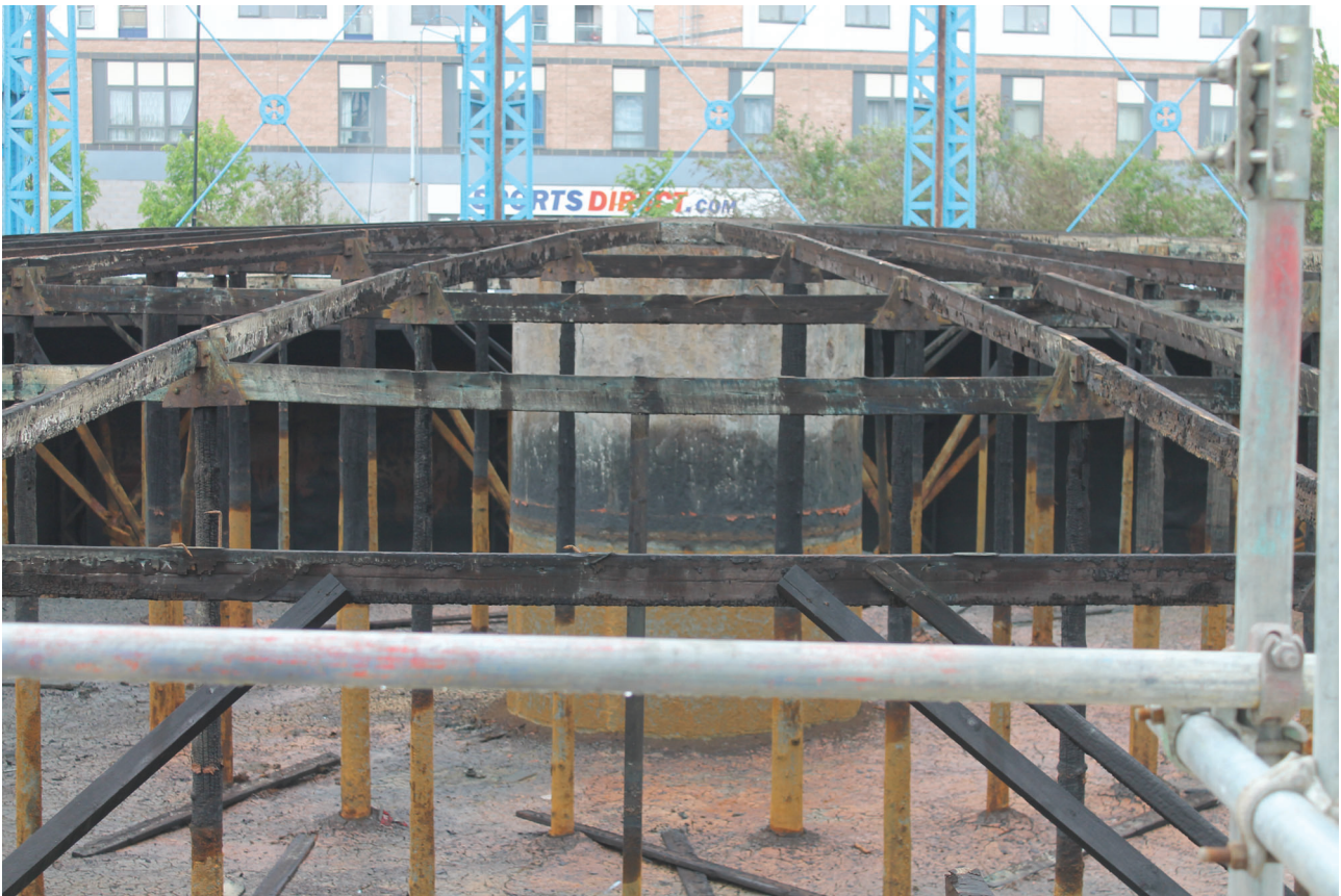
Plate 23: Bell Green, Sydenham, Gasholder No 7, general view of the central support post, from the north
