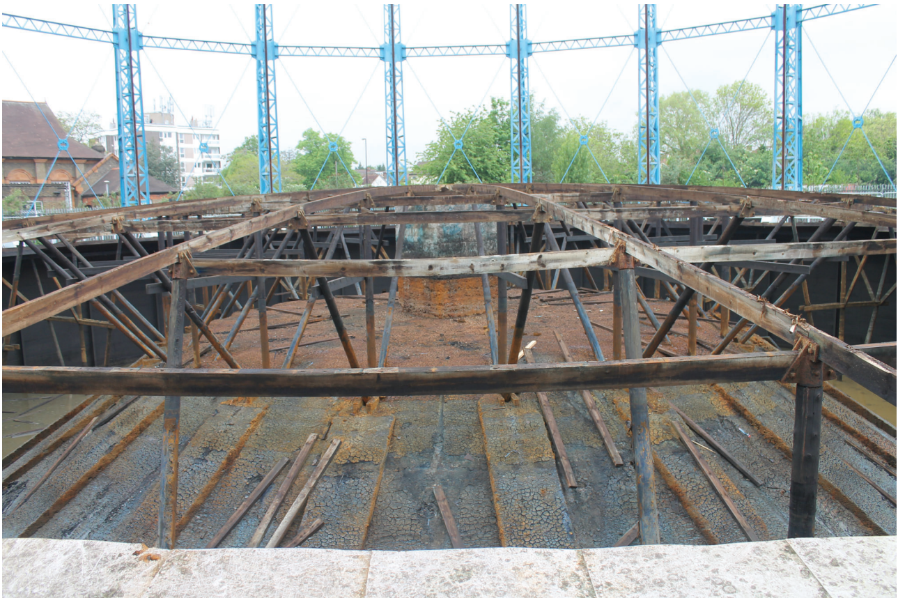
Plate 44: Bell Green, Sydenham, Gasholder No 8, general view of the dumping with raised linear, radial design
