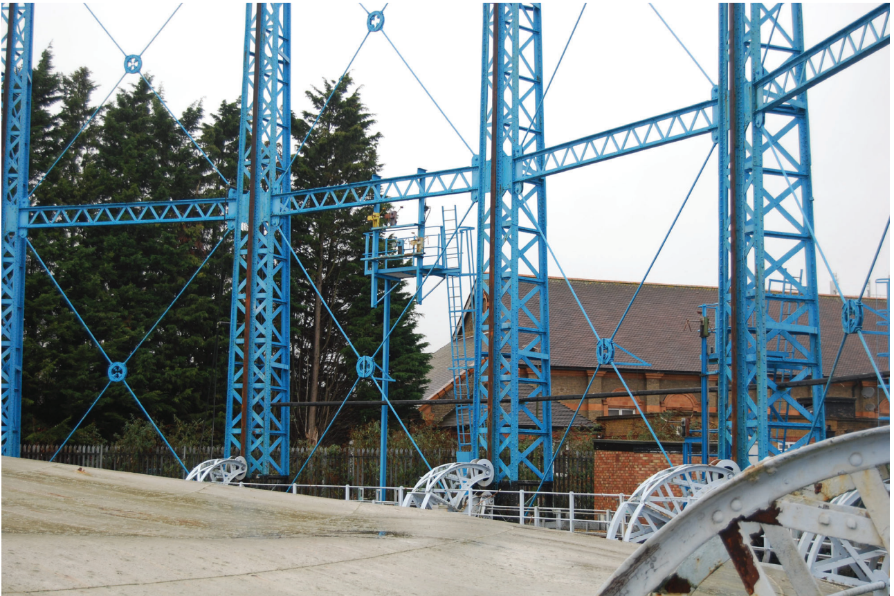
Plate 7: Bell Green, Sydenham, Gasholder No 7, general view of the gasholder frame from the south-east
