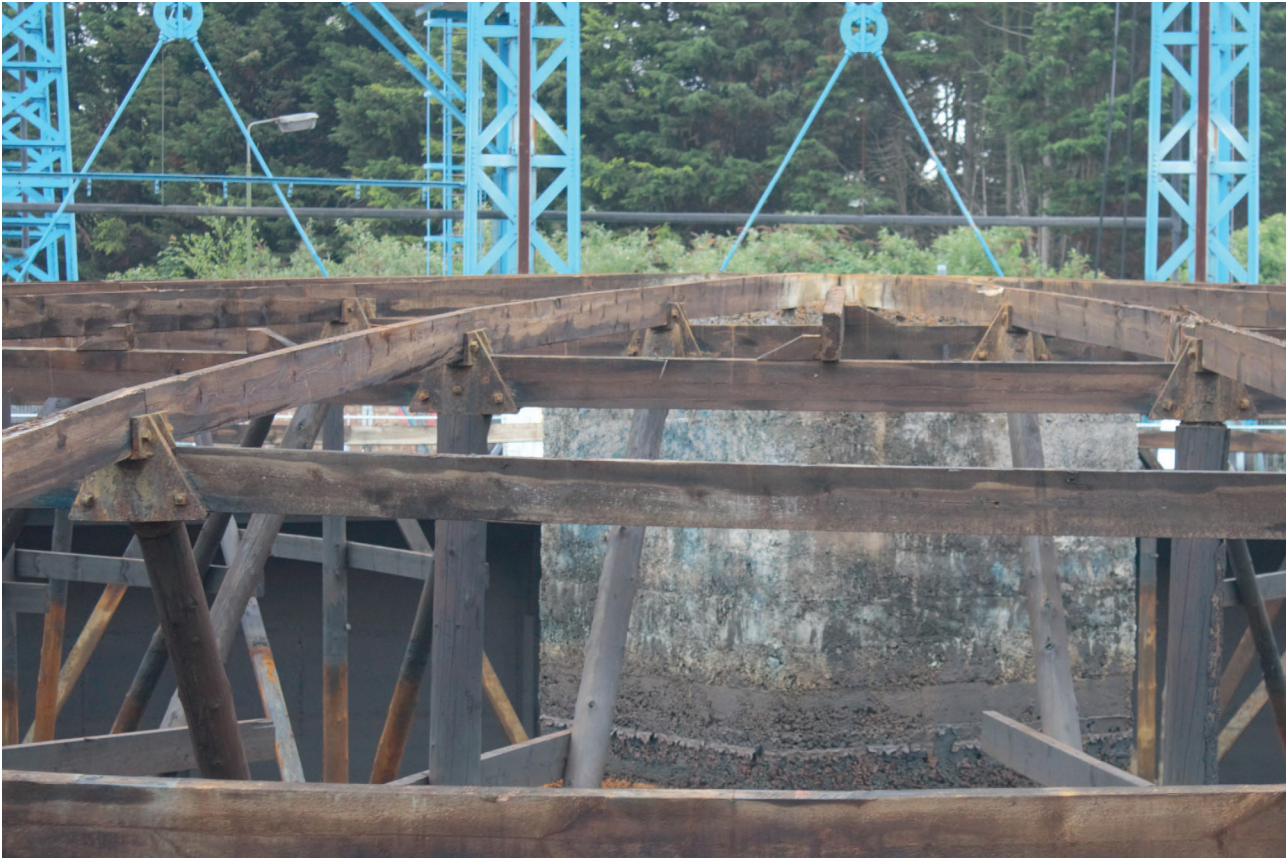
Plate 47: Bell Green, Sydenham, Gasholder No 8, detail of the metal fixtures attaching the upright poles to the dome frame, from the west
