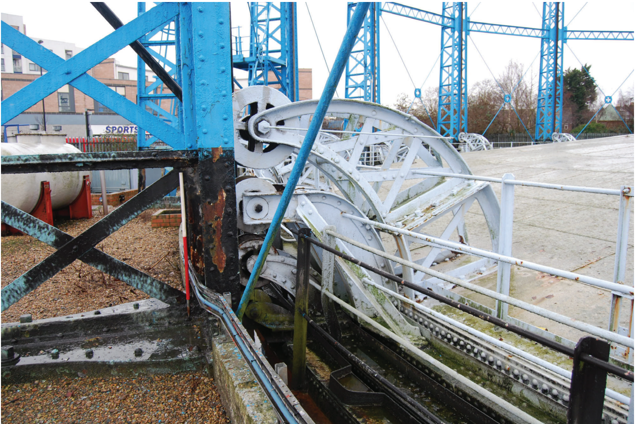
Plate 14: Bell Green, Sydenham, Gasholder No 7, detail of the guided rollers behind No 2 standard from the north-east
