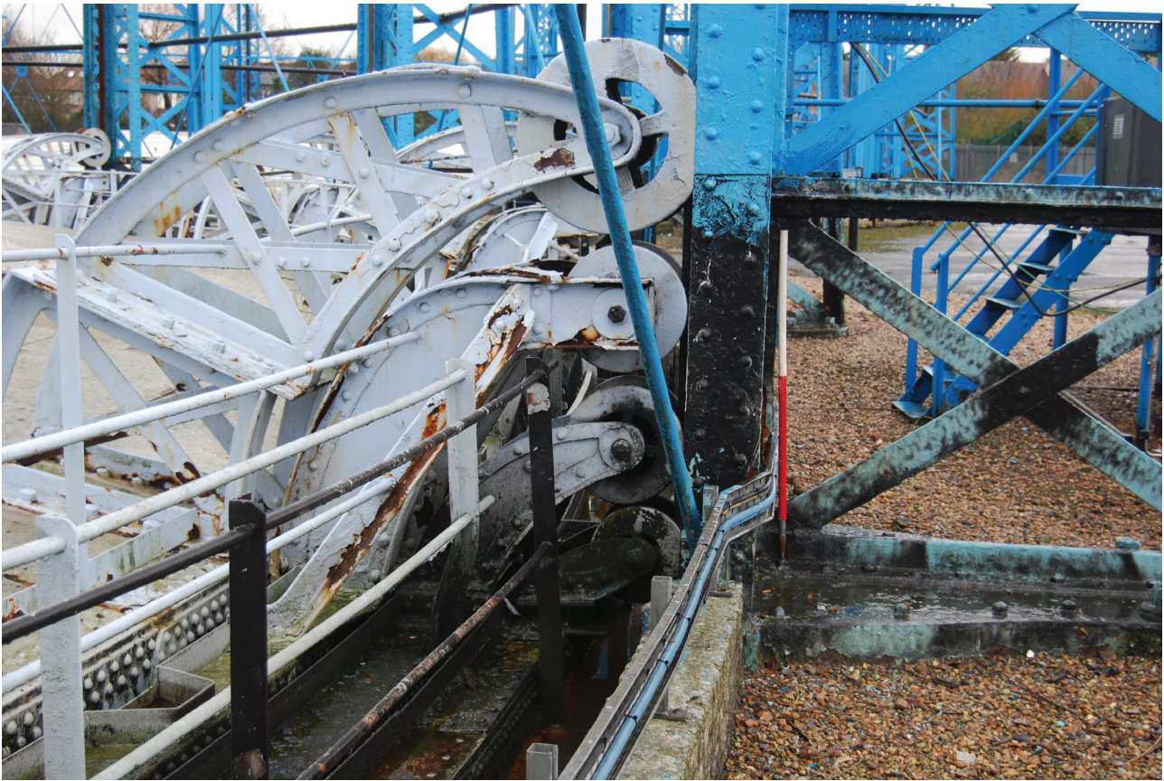
Plate 13: Bell Green, Sydenham, Gasholder No 7, detail of the guided rollers behind No 1 standard from the SSE
