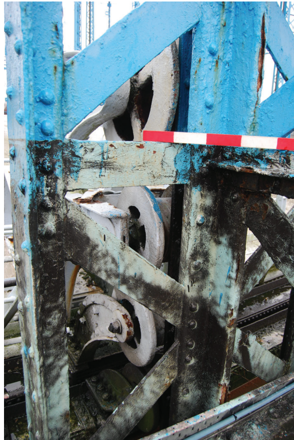
Plate 15: Bell Green, Sydenham, Gasholder No 7, detail of the guided rollers behind No 4 standard from the SSE
