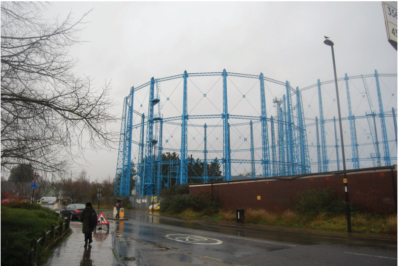
Plate 2: Bell Green, Sydenham, Gasholder No 7, general view of the gasholder frame from the south-east
