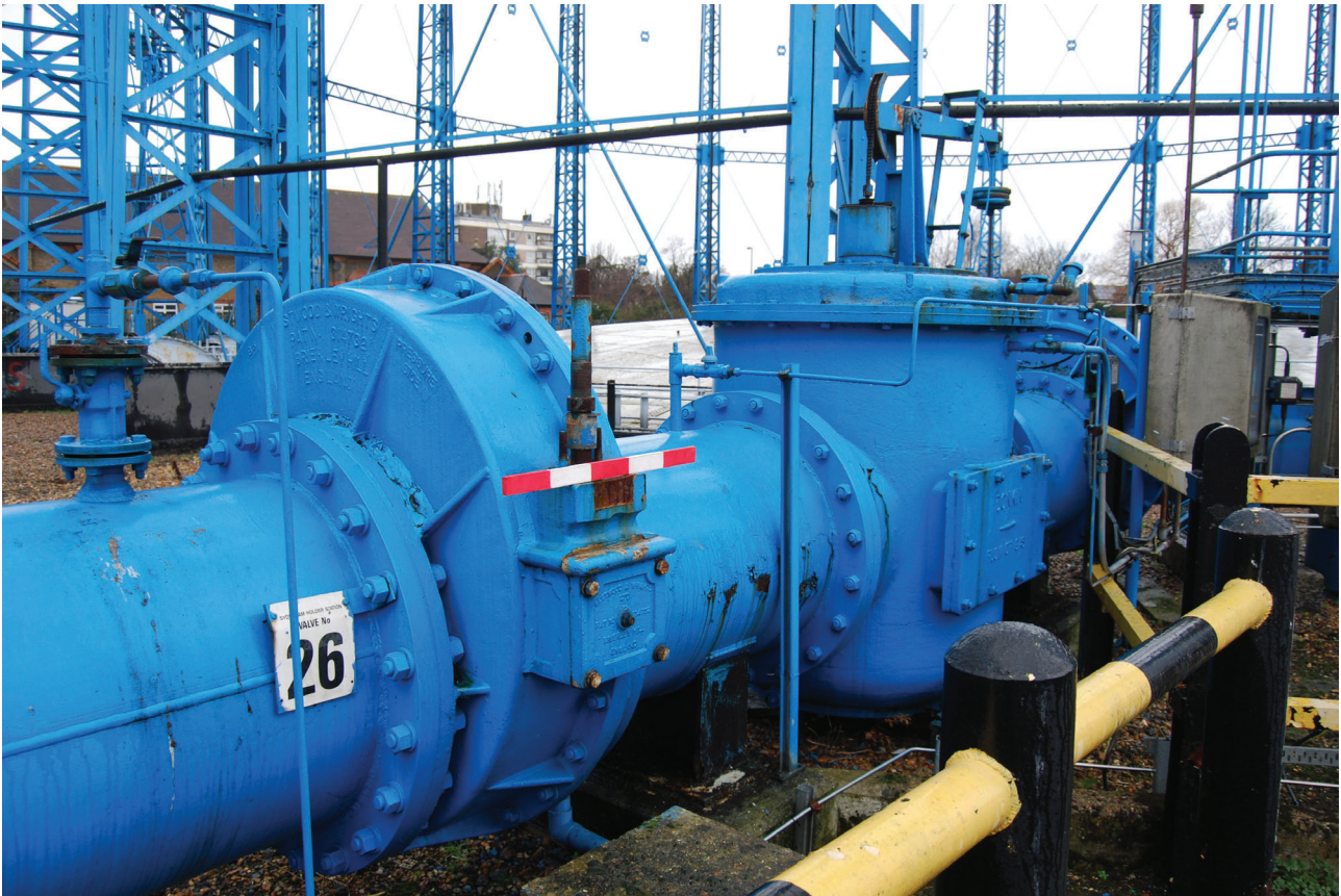
Plate 51: Bell Green, Sydenham, Gasholder No 8, general view of the pipework to the south-east of the gasholder from the south-east
