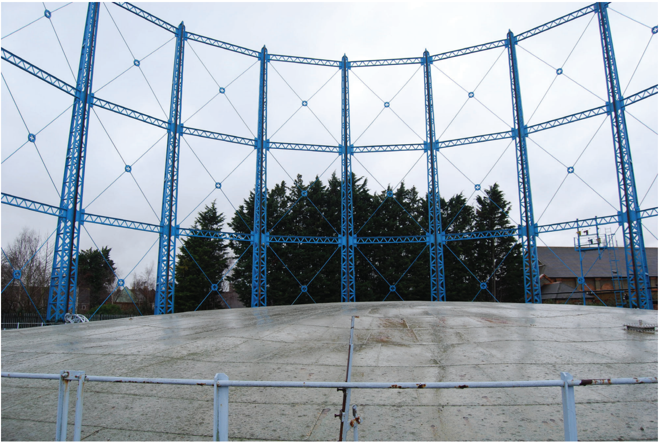
Plate 5: Bell Green, Sydenham, Gasholder No 7, general view of the gasholder frame from the ESE
