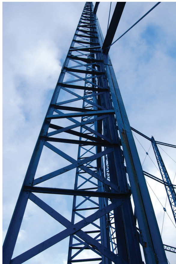
Plate 32: Bell Green, Sydenham, Gasholder No 8, general view of the gasholder frame from the SSW
