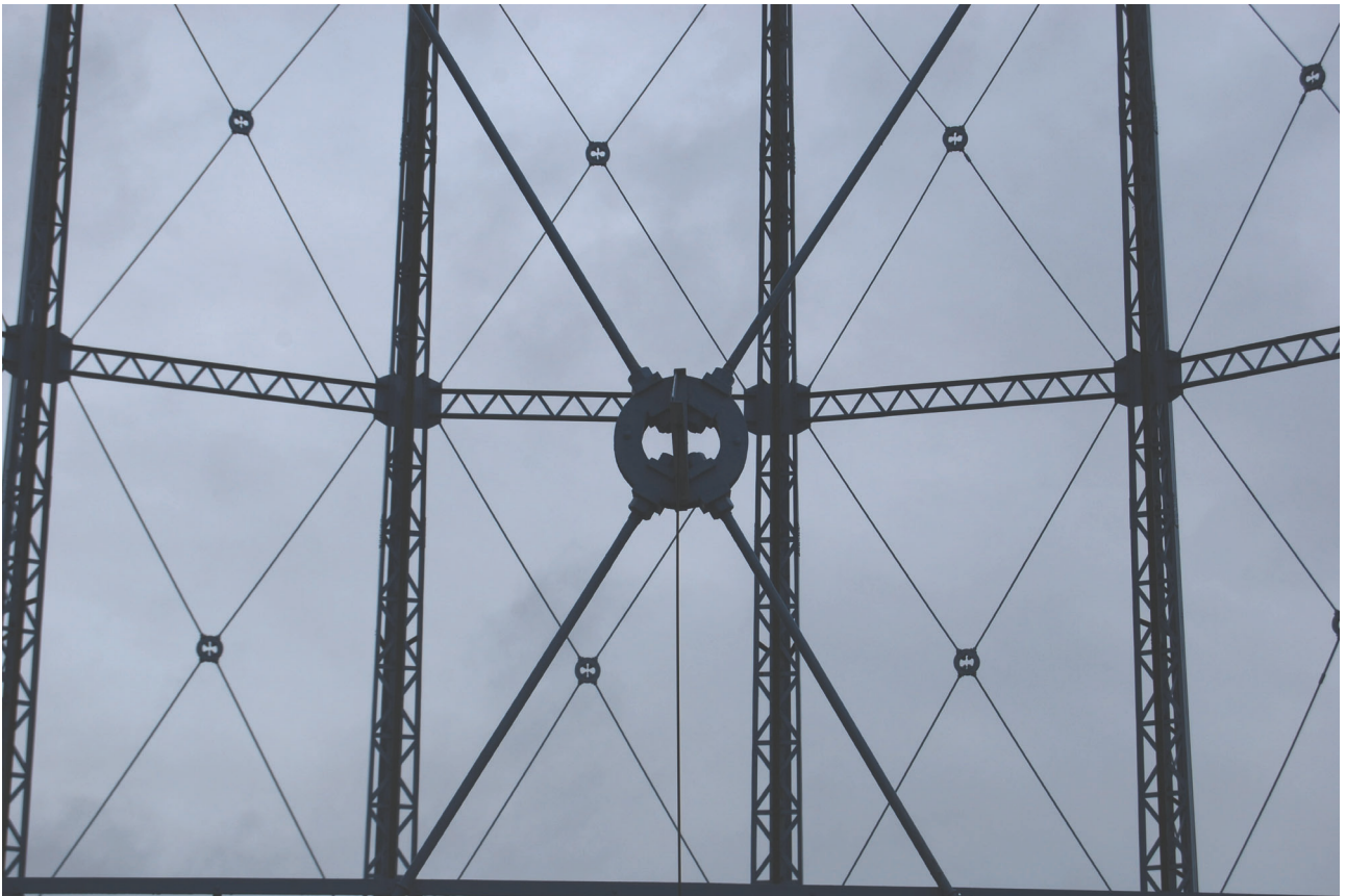
Plate 33: Bell Green, Sydenham, Gasholder No 8, detail of the diagonal bracing between the standards from the SSE
