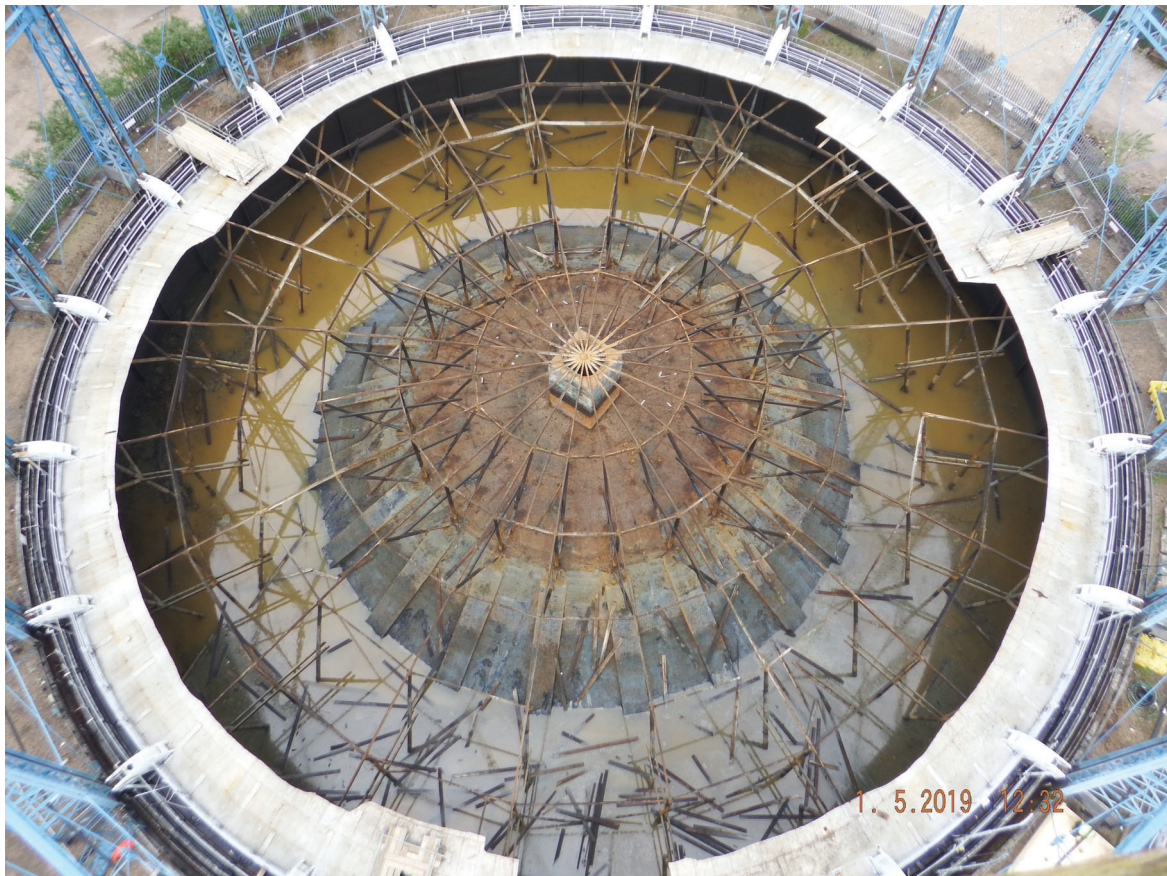
Plate 43: Bell Green, Sydenham, Gasholder No 8, general view of the dumping and crown rest frame, from the south © Keltbray
