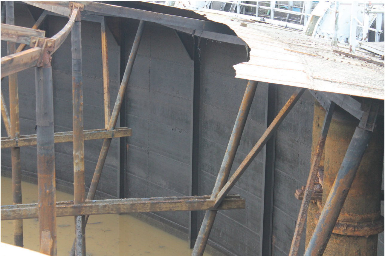
Plate 48: Bell Green, Sydenham, Gasholder No 8, detail view of the I-shape standards attached to the bell inner lift interior wall, from the SSW
