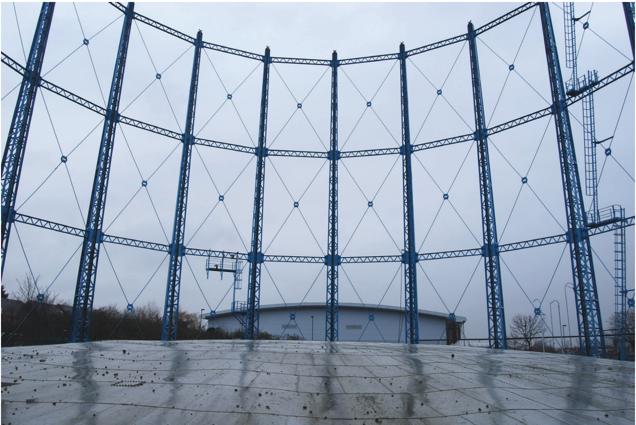
Plate 31: Bell Green, Sydenham, Gasholder No 8, general view of the gasholder frame from the south-west
