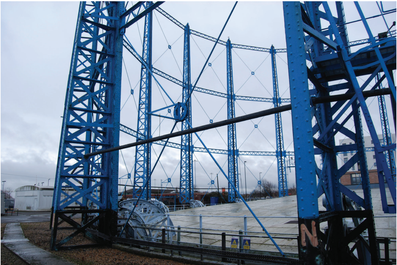
Plate 10: Bell Green, Sydenham, Gasholder No 7, detail of the diagonal bracing between the standards from the NNW
