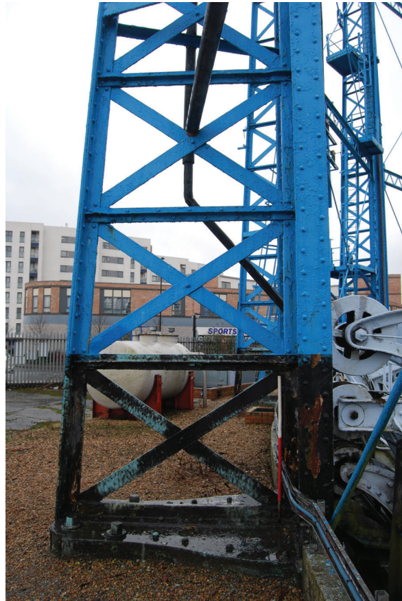
Plate 11: Bell Green, Sydenham, Gasholder No 7, detail of the base of No 2 standard from the NNE
