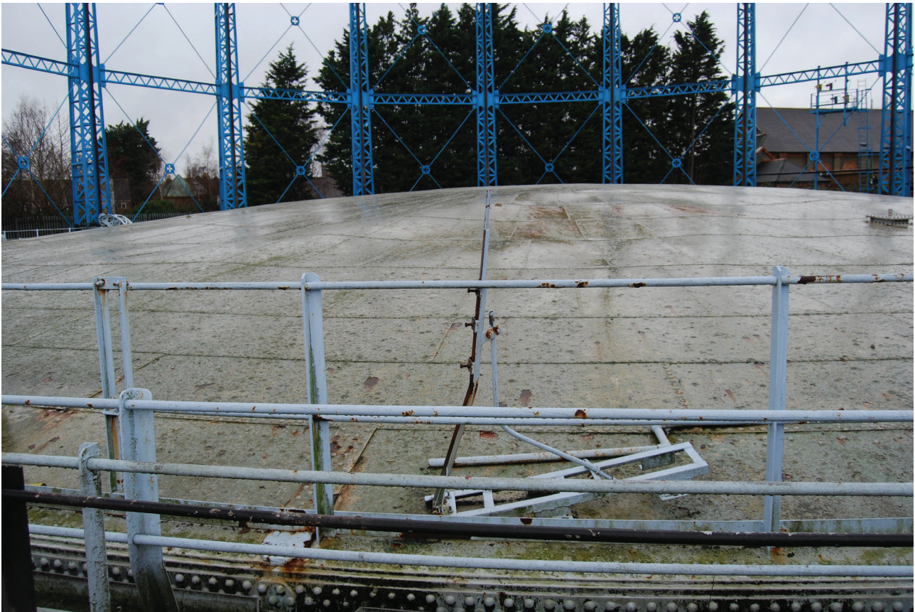
Plate 19: Bell Green, Sydenham, Gasholder No 7, general view of the crown of the gasholder from the ESE
