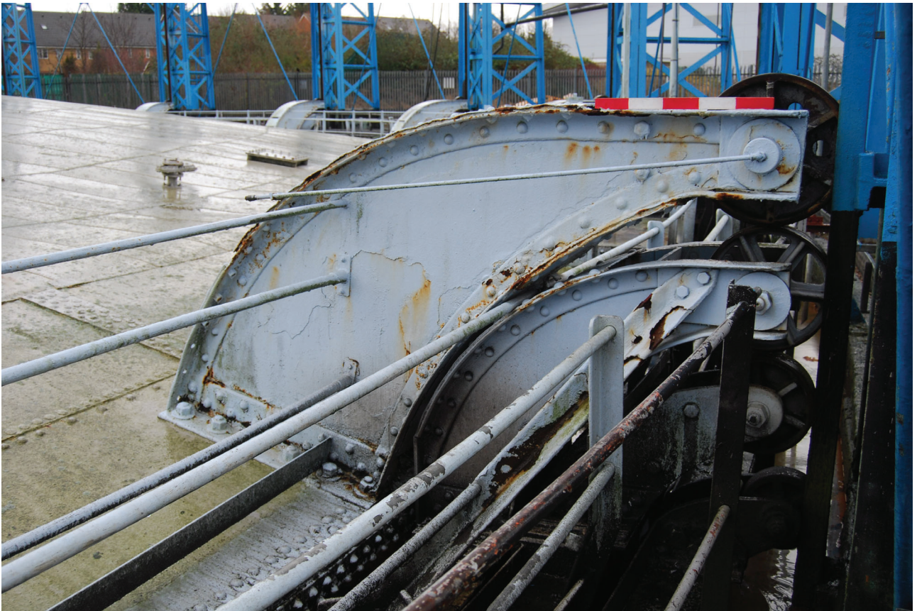
Plate 37: Bell Green, Sydenham, Gasholder No 8, detail of the guided rollers behind No 1 standard from the south-west
