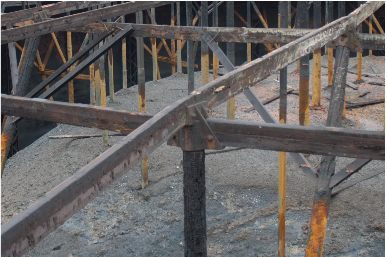
Plate 26: Bell Green, Sydenham, Gasholder No 7, detail view of the metal fixture attaching the uprights and dome timbers, from the east
