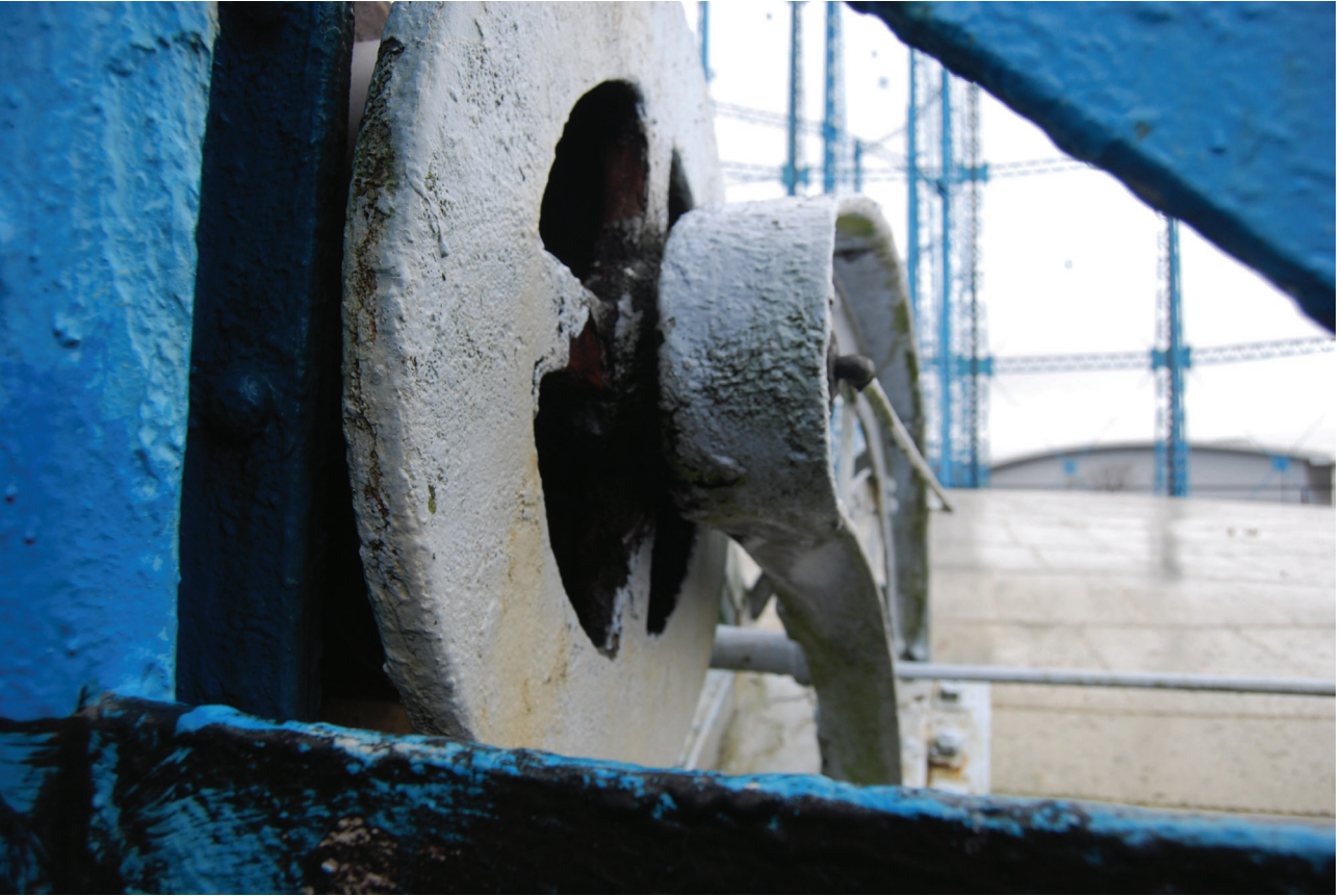
Plate 17: Bell Green, Sydenham, Gasholder No 7, close detail of the guided rollers behind No 7 standard from the SSE
