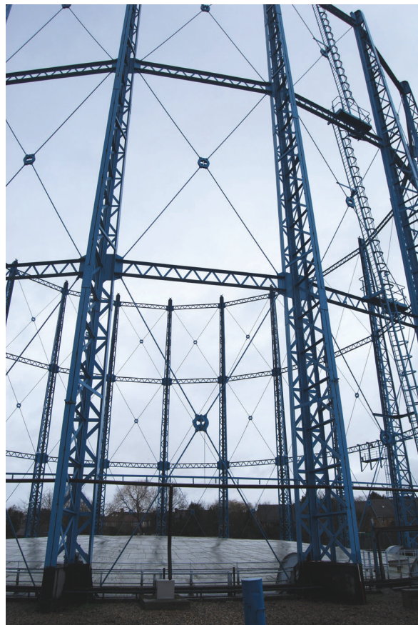
Plate 30: Bell Green, Sydenham, Gasholder No 8, general view of the gasholder frame from the SSE
