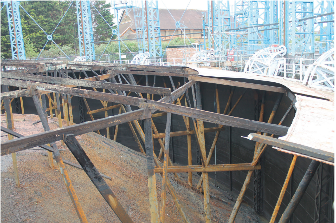
Plate 25: Bell Green, Sydenham, Gasholder No 7, general view of the outermost upright posts with metal support bracket, and lattice standards within the bell, from the south-east
