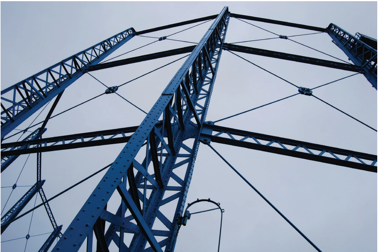
Plate 6: Bell Green, Sydenham, Gasholder No 7, general view of the gasholder frame from the south
