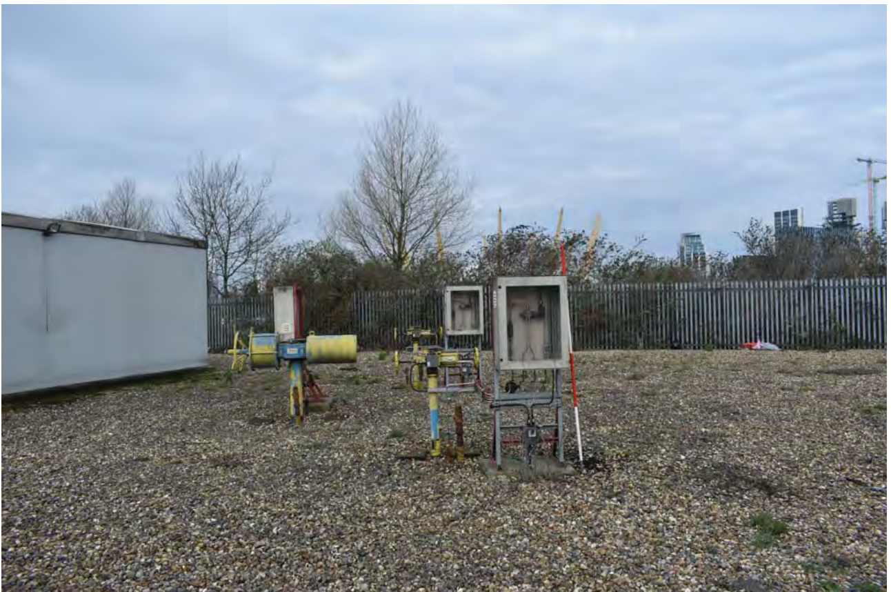
Plate 46: Features D, E & F and their associated pipework to the east of Building B, from the SSE
