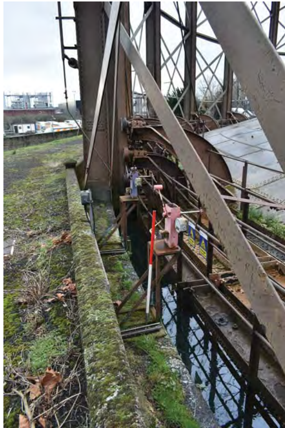
Plate 17: Gasholder No 1, detail of the knock-off switches (Q & R) between No 7 and No 8 standards from the north
