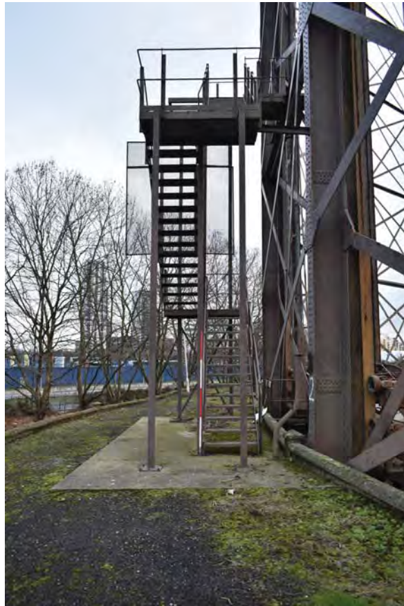
Plate 11: Gasholder No 1, detail of the stairs between No 2 and No 3 standards from the west
