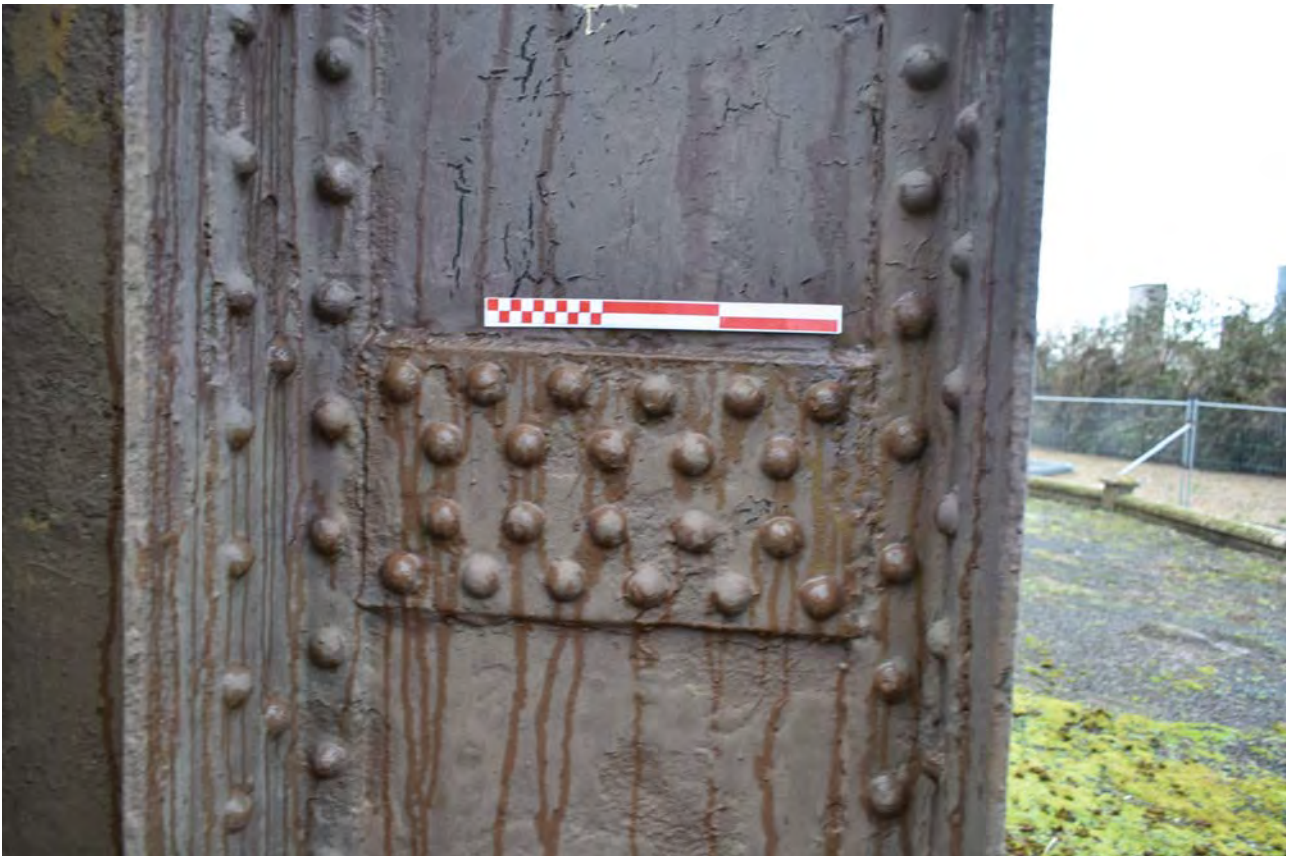
Plate 8: Gasholder No 1, close detail of the inner section of No 1 standard from the east
