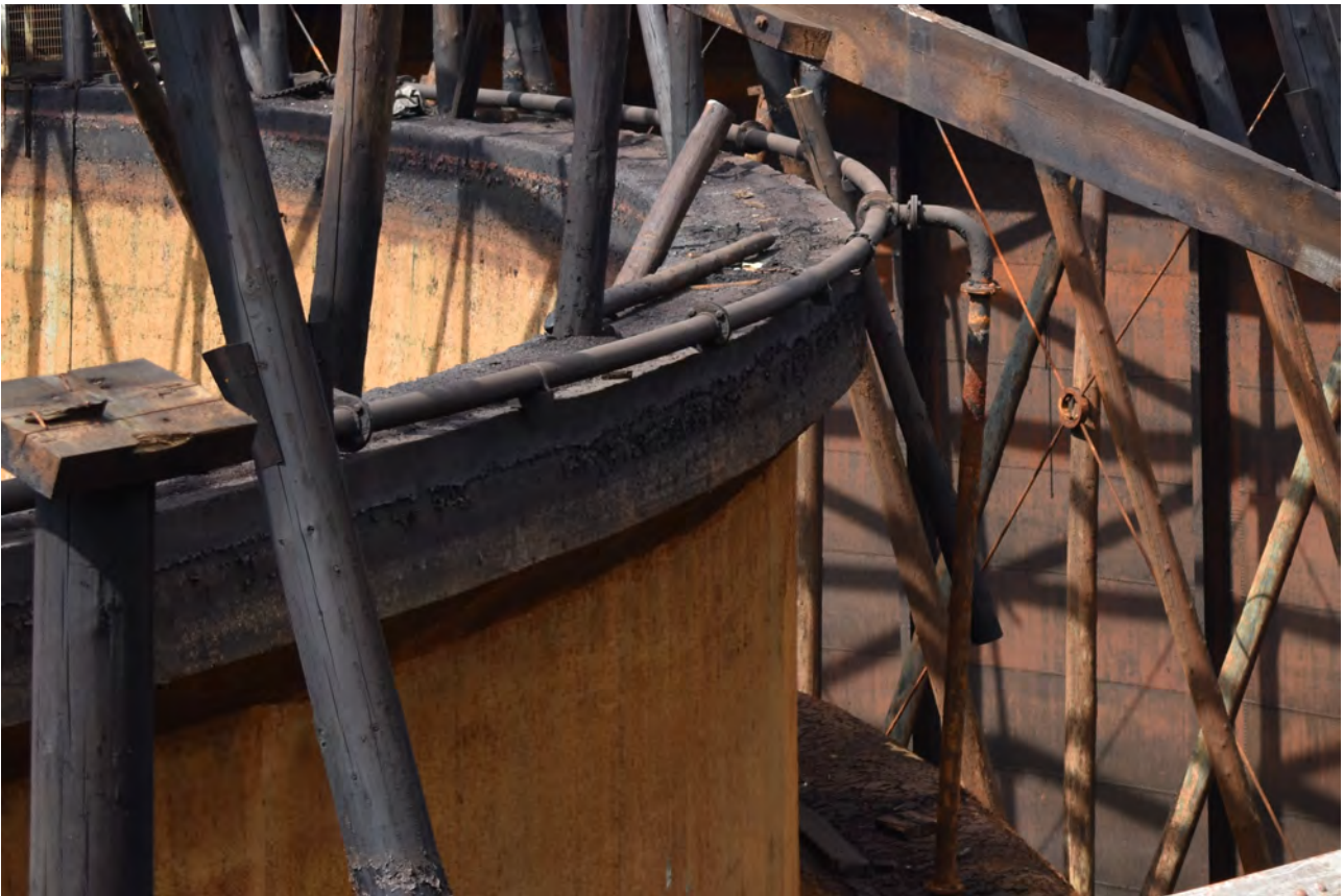
Plate 38: Gasholder No 1, general view of a pipe entering the tank from the north and running up and around the top of the wall in the tank, from the ENE
