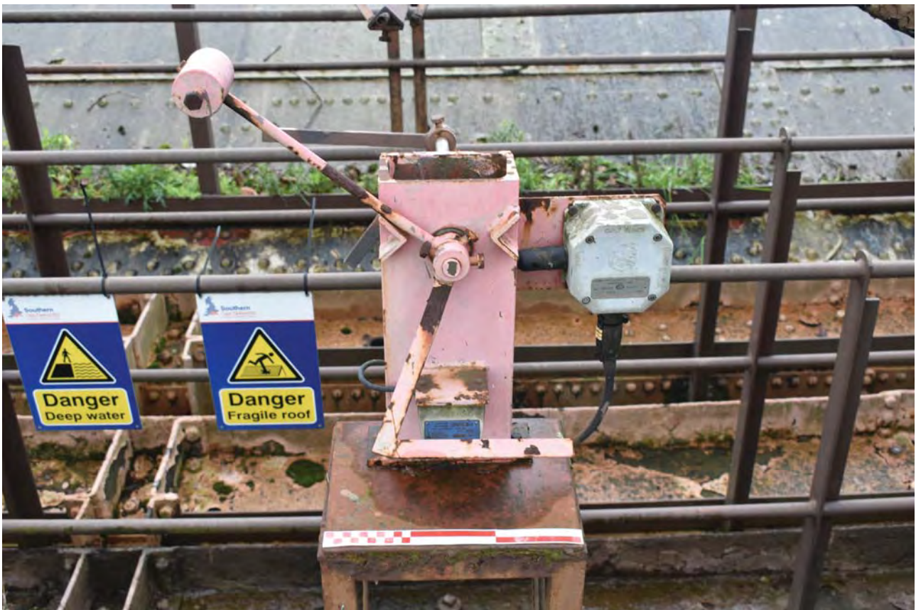
Plate 18: Gasholder No 1, detail of the northernmost knock-off switch (Q) between No 7 and No 8 standards from the north-east
