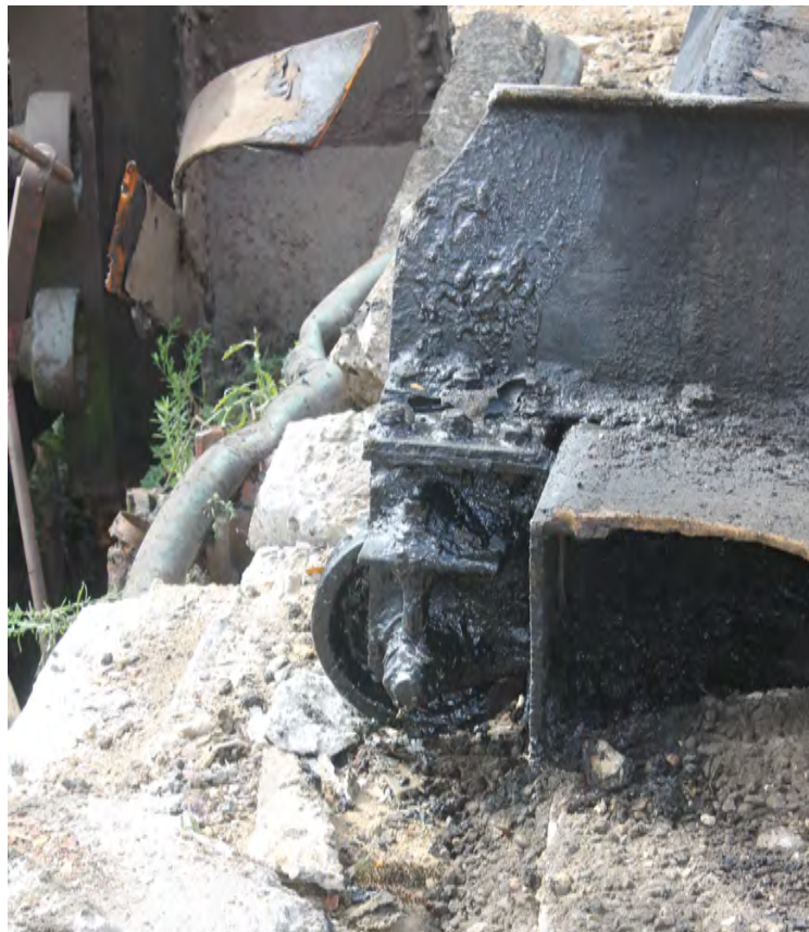
Plate 42: Gasholder No 1, detail of the cup-and-grip and roller wheel on the base of one of the lifts, not in situ
