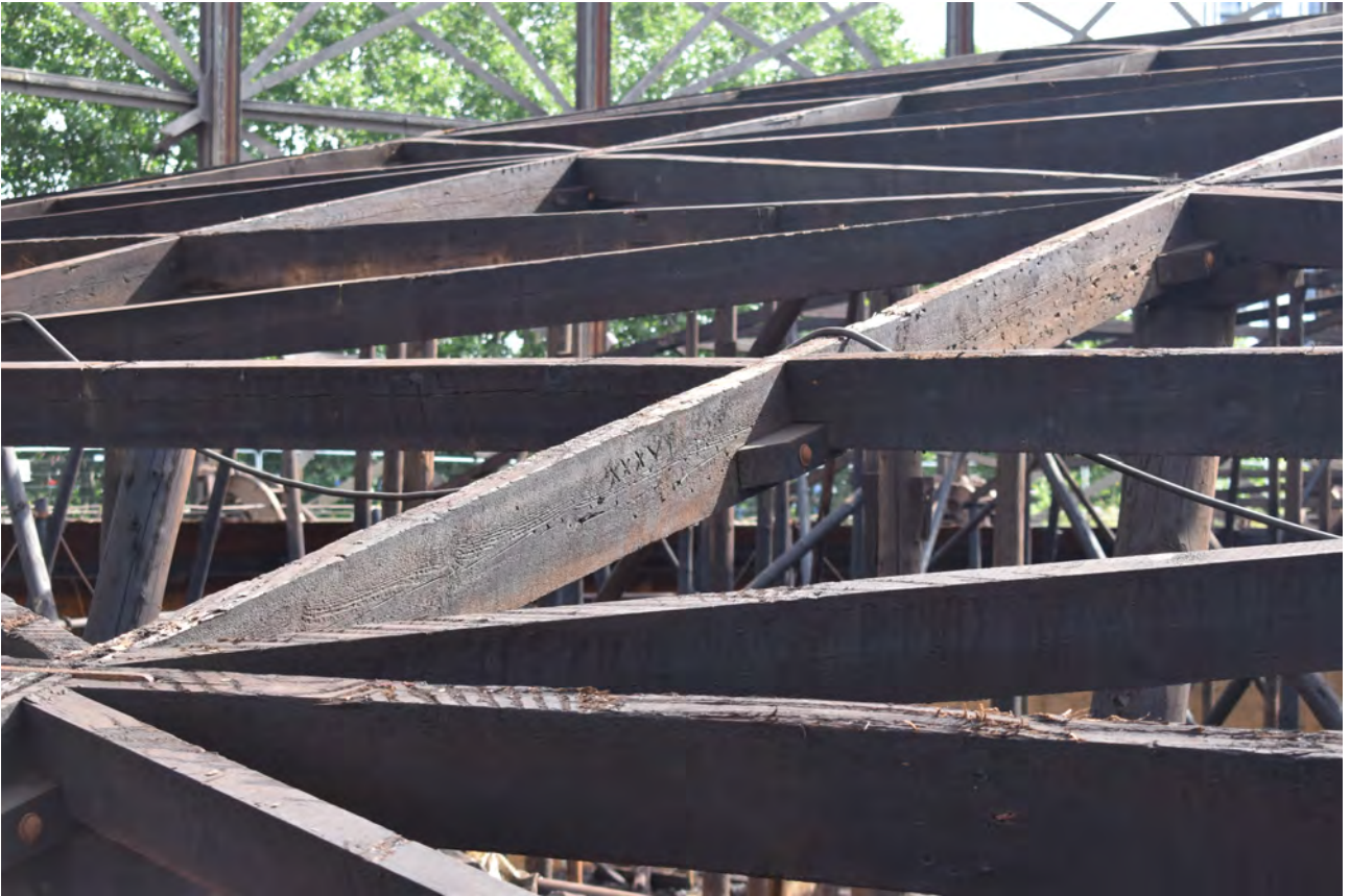
Plate 27: Gasholder No 1, detail of blocks nailed at the joints to increase stability, from the WSW
