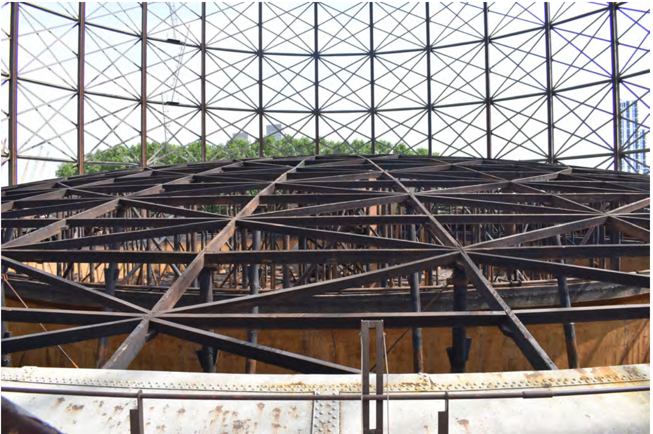
Plate 23: Gasholder No 1, general view of the timber support frame visible due to the crown removal, from the south-west
