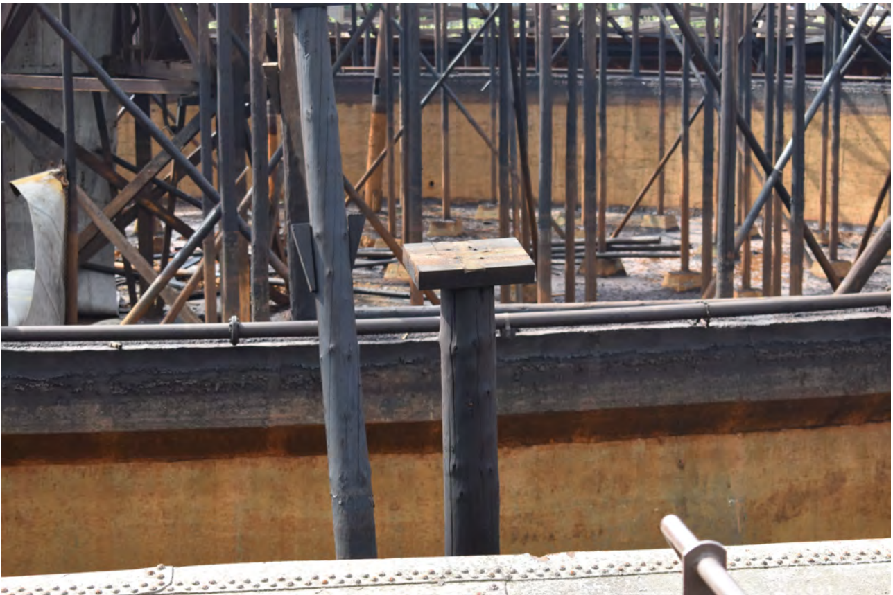
Plate 34: Gasholder No 1, detail view of a square block set on top of each upright to support the timber joint above, and blocks nailed to the side of the uprights for standing on during constructions, from the north
