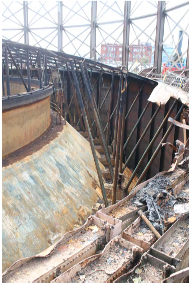
Plate 35: Gasholder No 1, general view of the platform halfway up the dumping which supports the outermost ring of uprights with three set in each concrete base at this level, from the north-east
