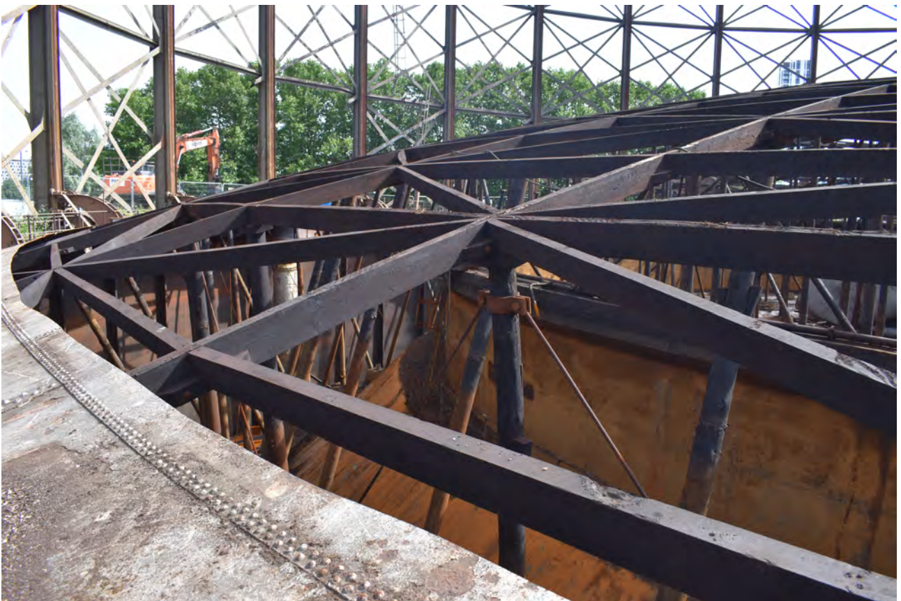
Plate 24: Gasholder No 1, general view of the timber support frame comprised of many short lengths of timber, from the WSW
