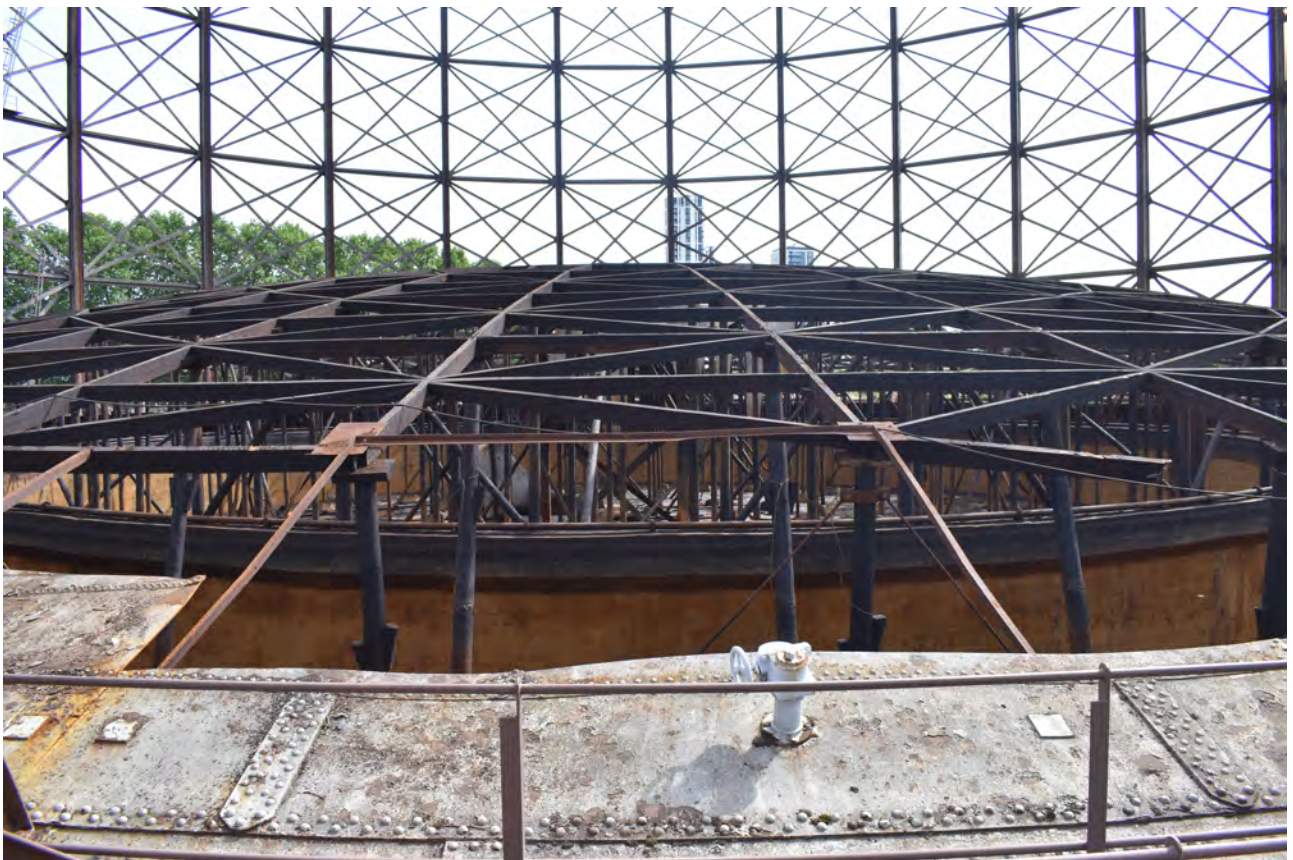
Plate 28: Gasholder No 1, detail of metal repair to the crown support frame between standards 21 and 22, from the south-west
