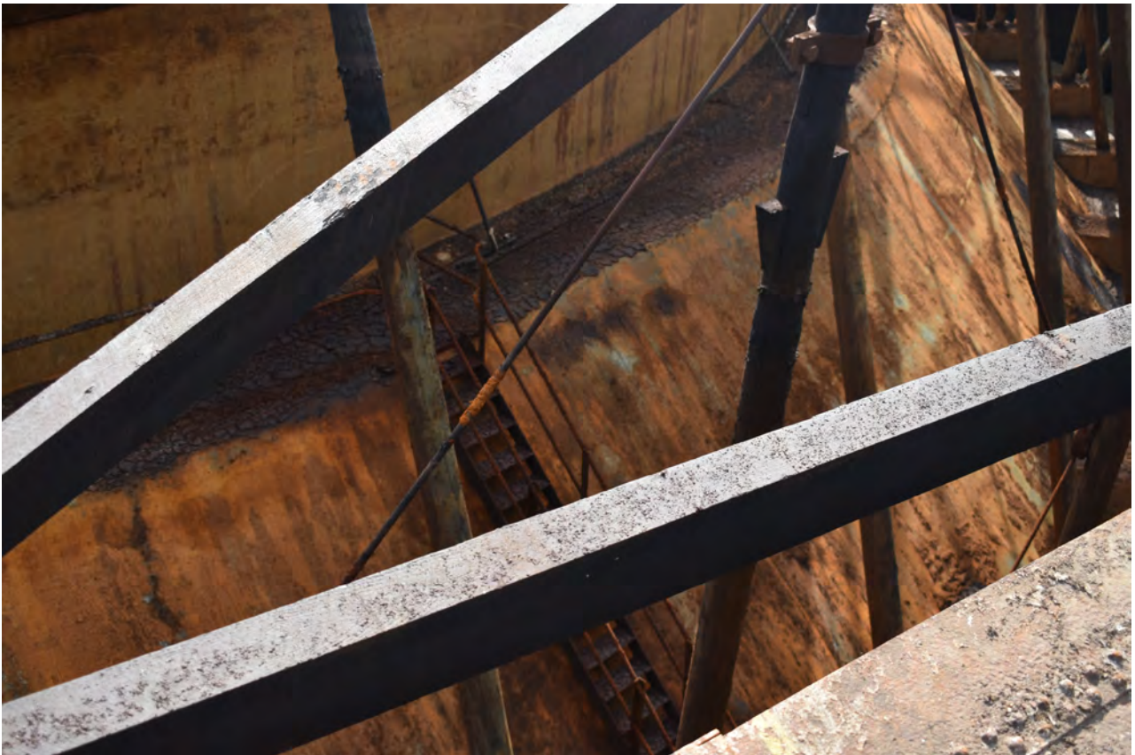
Plate 36: Gasholder No 1, general view of the steps leading up the west side of the dumping, from the WNW
