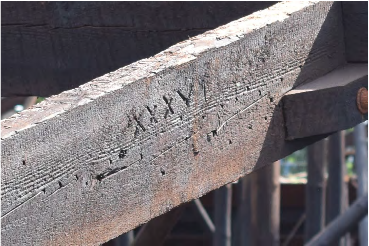
Plate 29: Gasholder No 1, detail of carved roman numeral (XXXVI) on spoke timber suggesting a numbering system was used during construction, from the WSW
