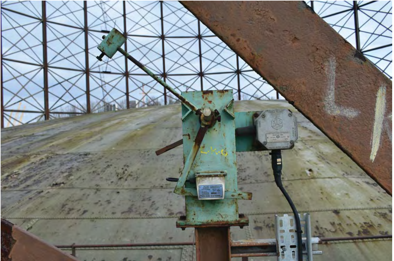
Plate 19: Gasholder No 1, detail of the knock-off switch (S) between No 19 and No 20 standards from the SSW
