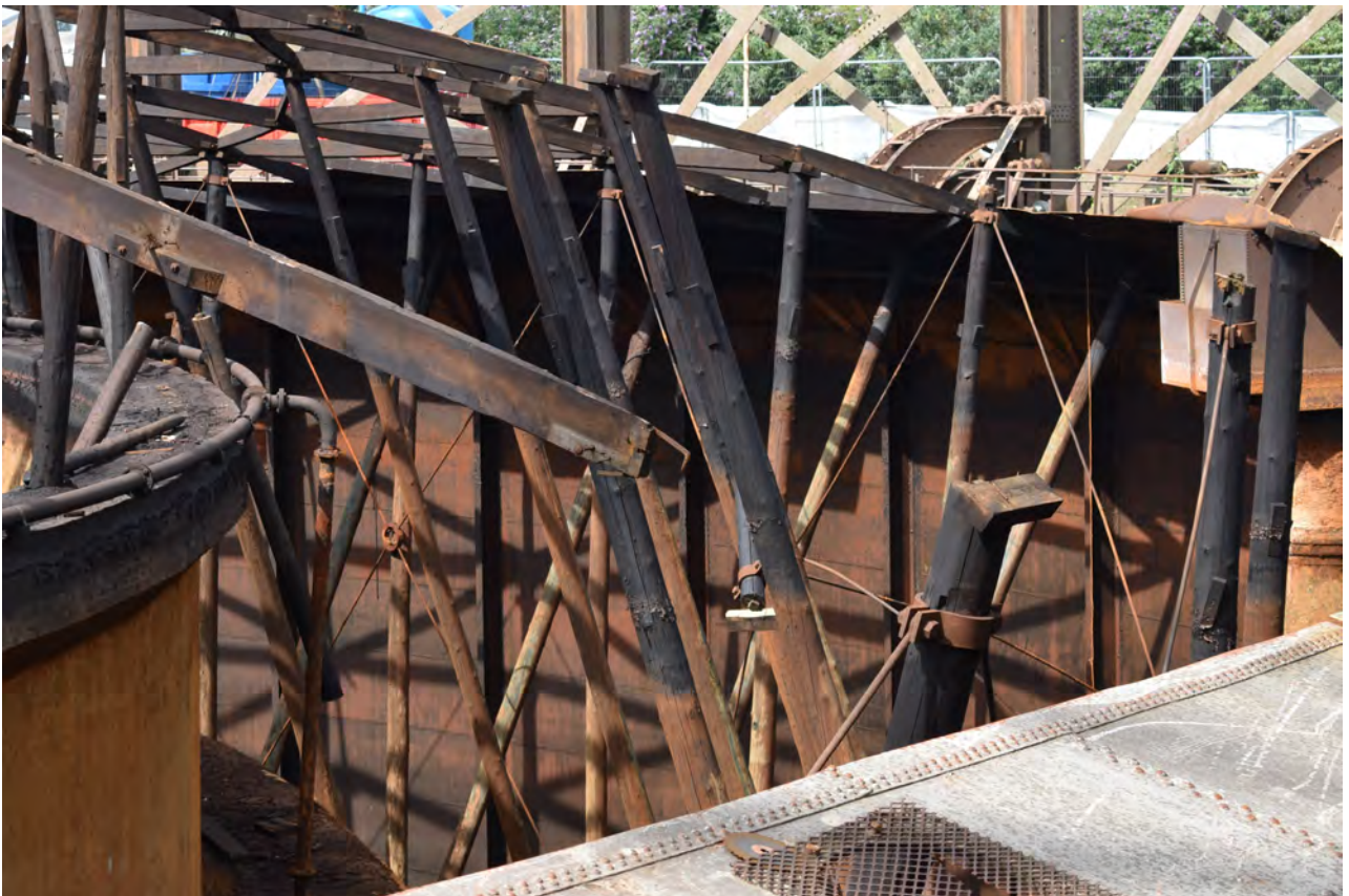
Plate 30: Gasholder No 1, general view of diagonal tie-bars secured with tension rings between the timber uprights of the outermost support ring, from the east
