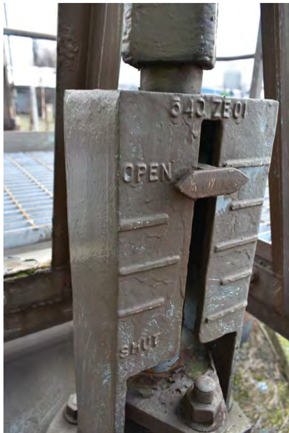
Plate 22: Gas Main, detail of the gauge from the north-west
