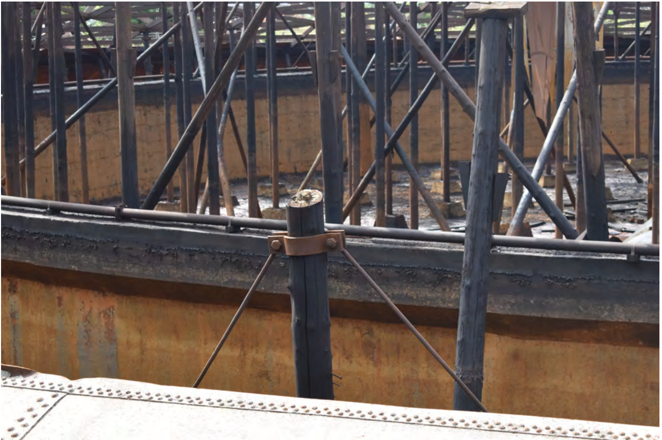
Plate 31: Gasholder No 1, general view of concrete block bases for uprights, from the north-east
