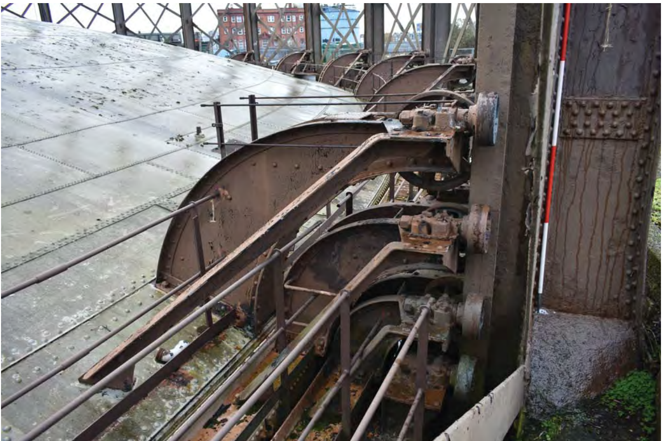
Plate 14: Gasholder No 1, detail of the guided rollers behind No 1 standard from the ENE
