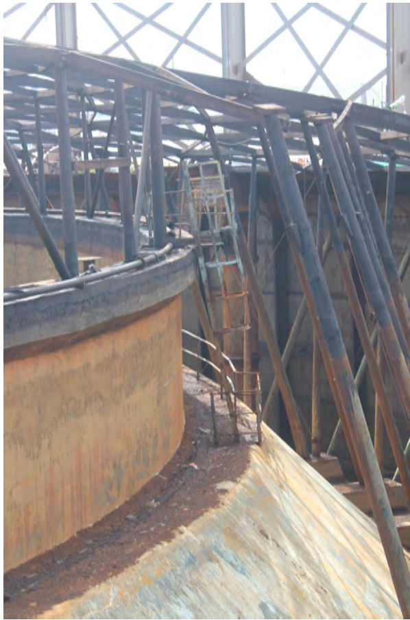
Plate 37: Gasholder No 1, general view of the ladder leading up the dumping wall, from the ENE
