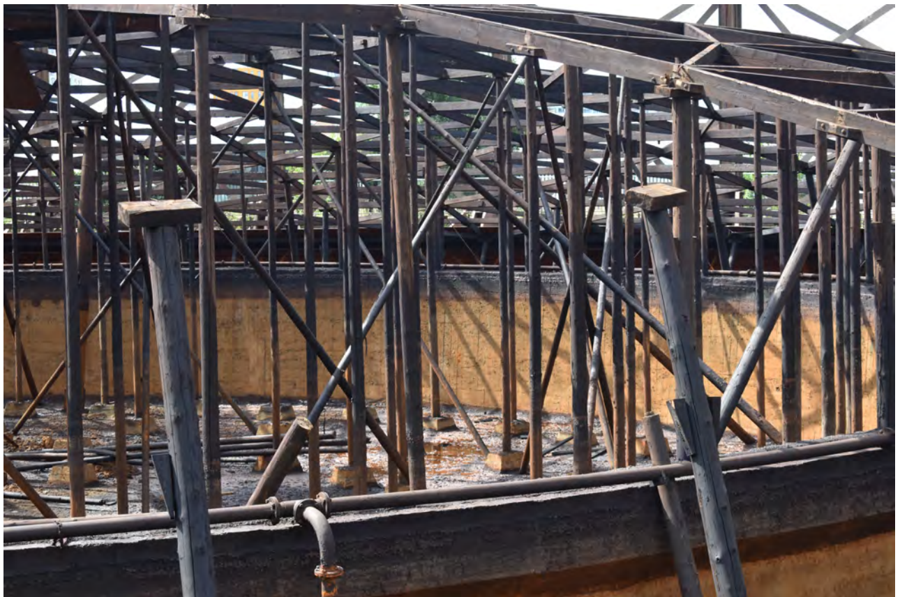
Plate 32: Gasholder No 1, general view of concrete block bases for uprights, from the north-east
