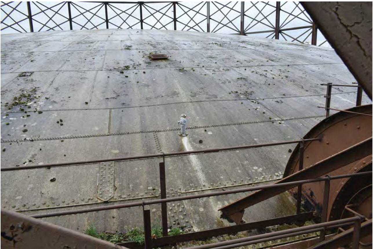
Plate 13: Gasholder No 1, general view of the crown of the gasholder from the north-east
