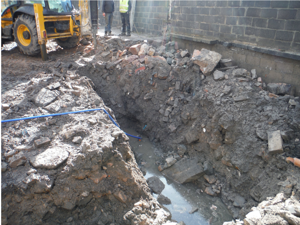
Plate 2: Flooded foundation trench showing made ground
