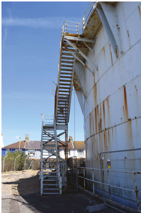
Plate 10: Park Road, Worthing, detail of the access stair to the west side of the gasholder, from the SSE
