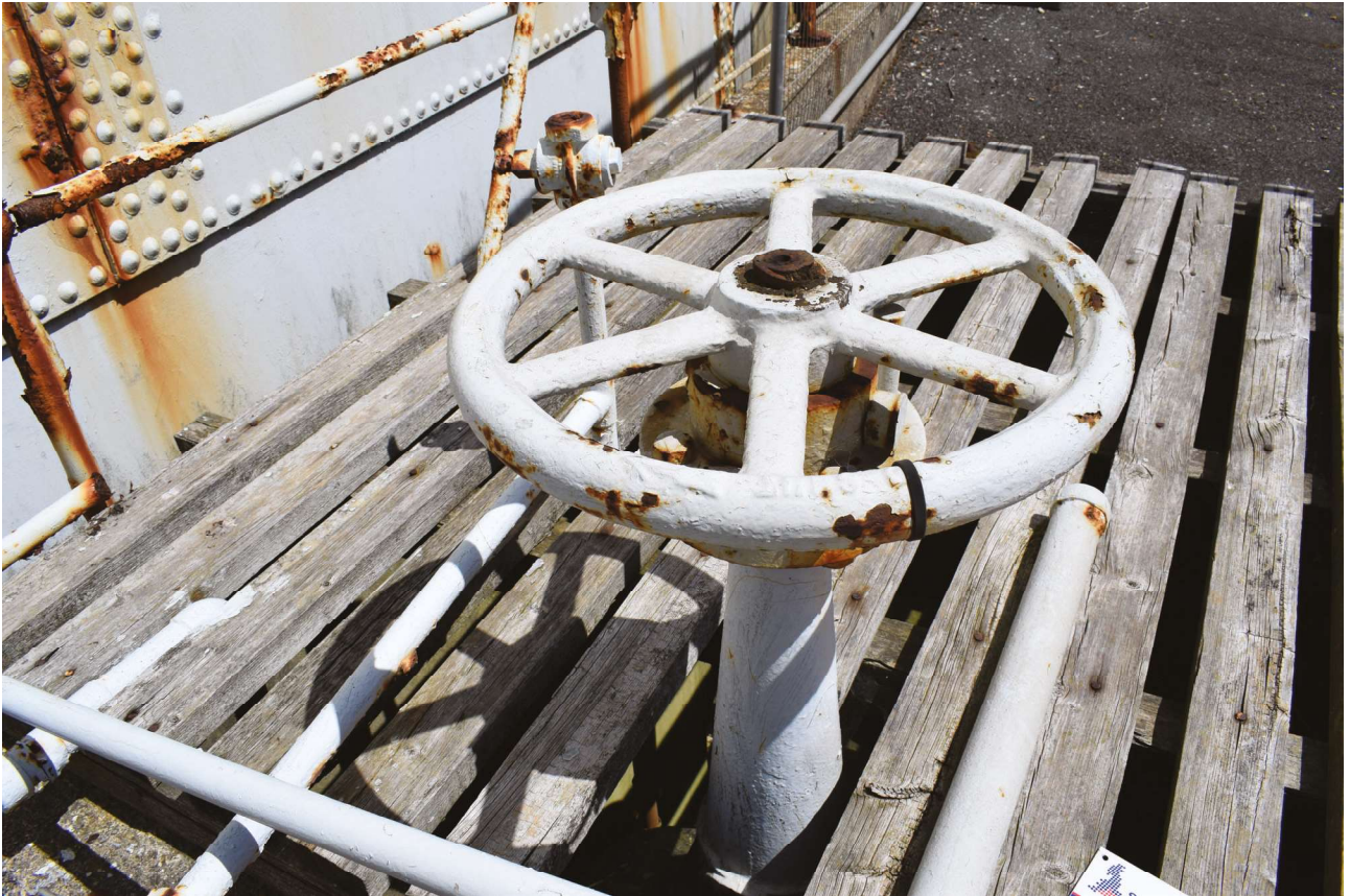
Plate 13: Park Road, Worthing, Structure 4, detail of the valve wheel, from the south-west
