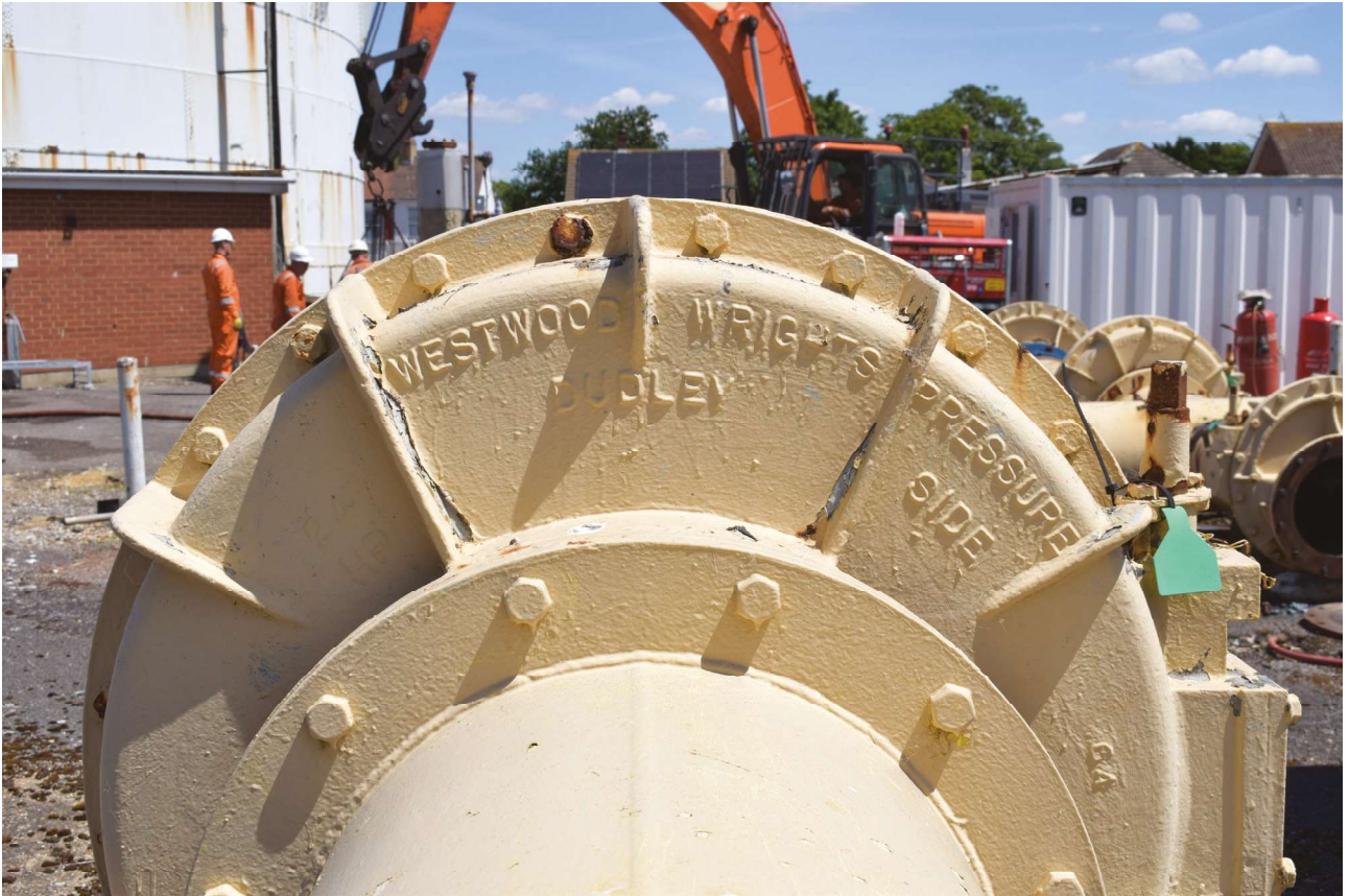
Plate 29: Park Road, Worthing, Structure 8, detail of the pipework showing the manufacturer's mark, from the ENE
