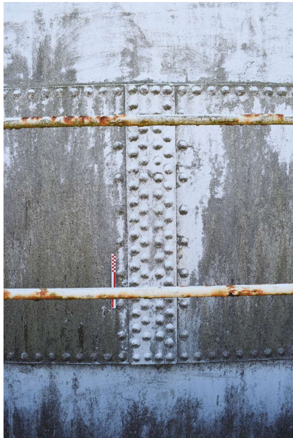
Plate 6: Park Road, Worthing, detail of riveted plate on the north-east side of the gasholder, from the north-east
