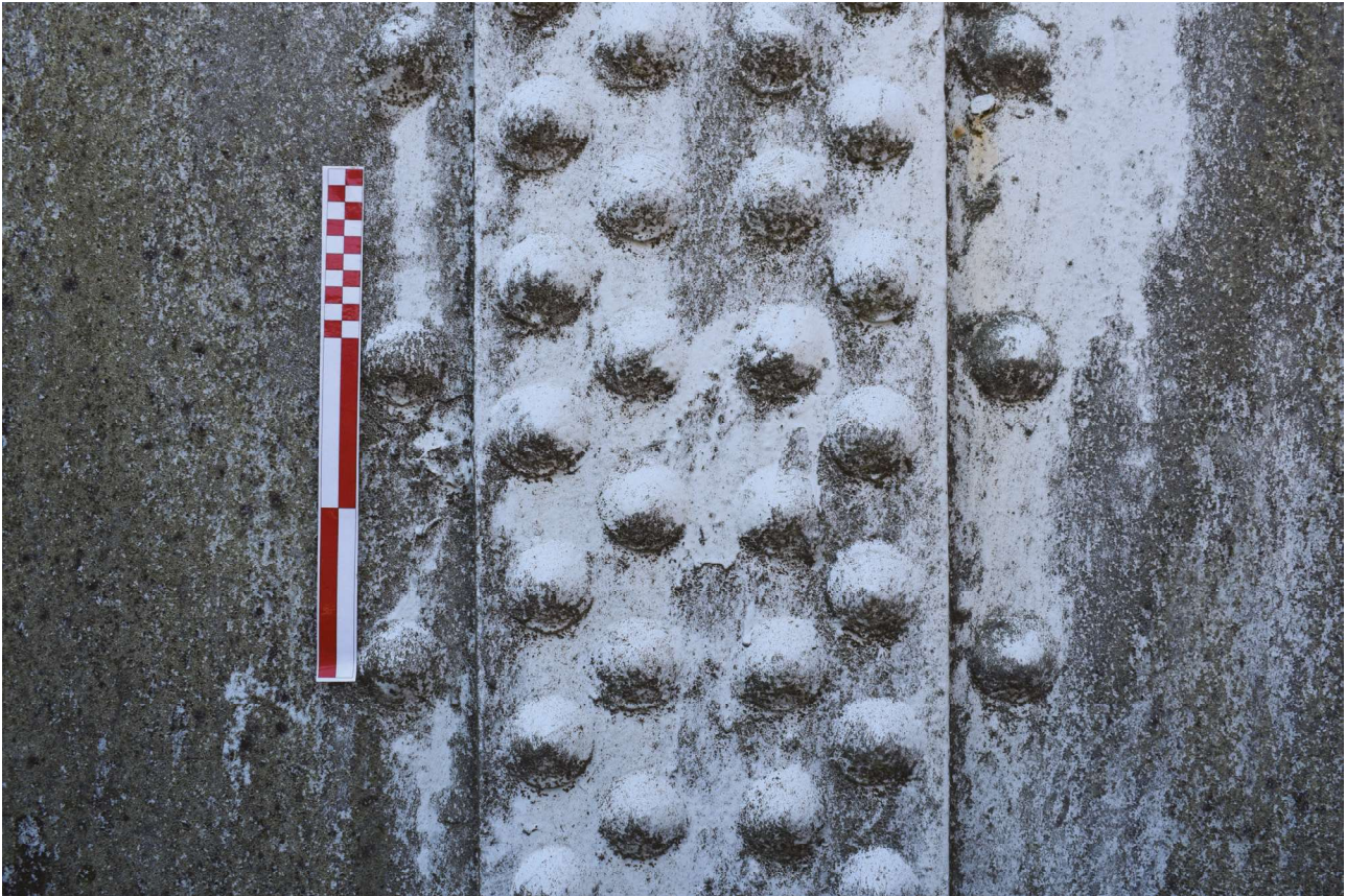
Plate 7: Park Road, Worthing, close detail of riveted plate on the north-east side of the gasholder, from the north-east
