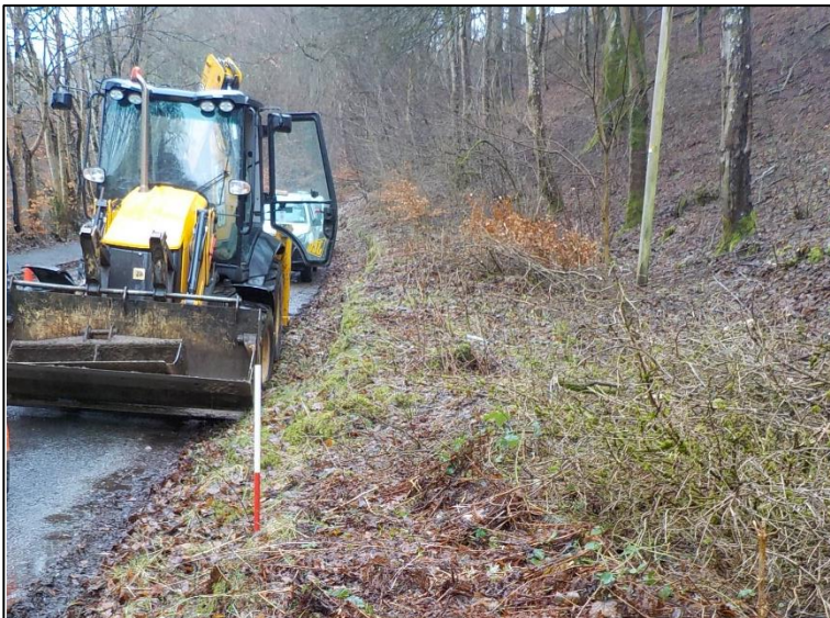
Plate 5: Pre-condition of degraded boundary wall
