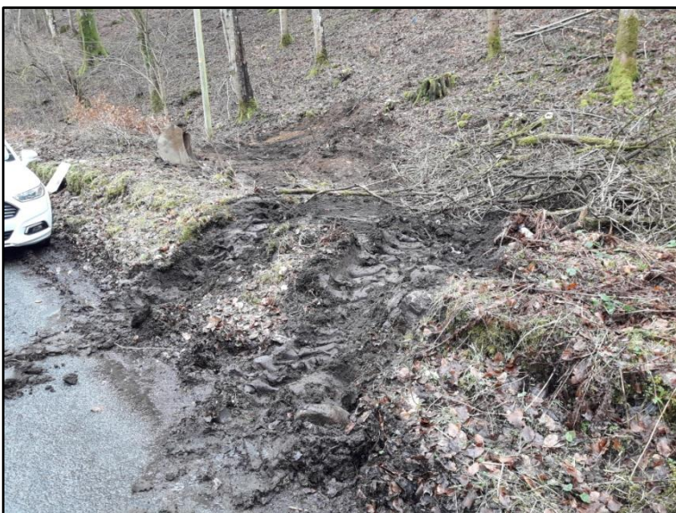
Plate 6: Post-condition of degraded boundary wall
