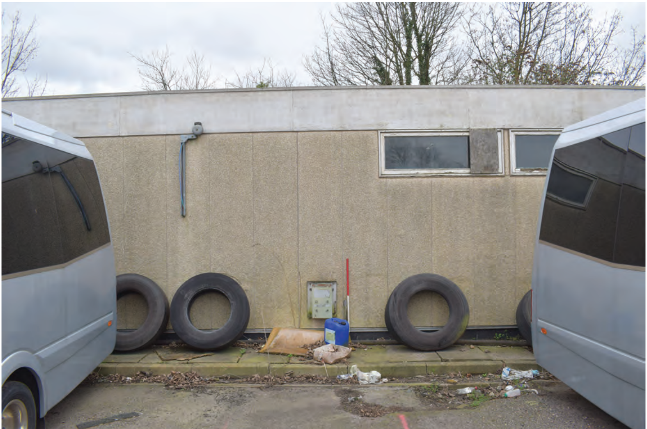
Plate 158: Structure V, detail view of exterior NNW wall showing pebbledash cladding, entrance and high windows, from the NNW
