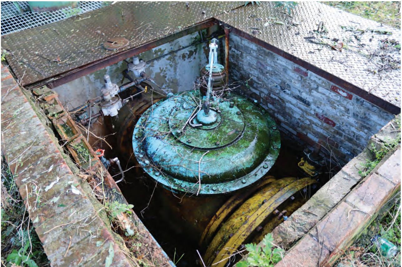
Plate 94: Gasholder No 2, general view of the brick-lined valve pit associated with the gas inlet pipe, from the north
