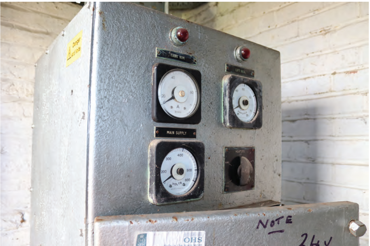
Plate 62: Gasholder No 1, detail view of gauges for the anti-freeze system in the tank rim and lift seal, from the north-west
