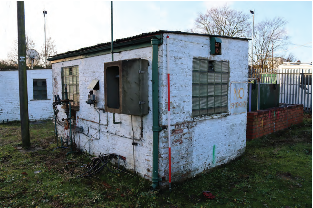
Plate 127: Structure H, general view of the exterior north and east walls showing glass block windows and instrumentation, from the north-east
