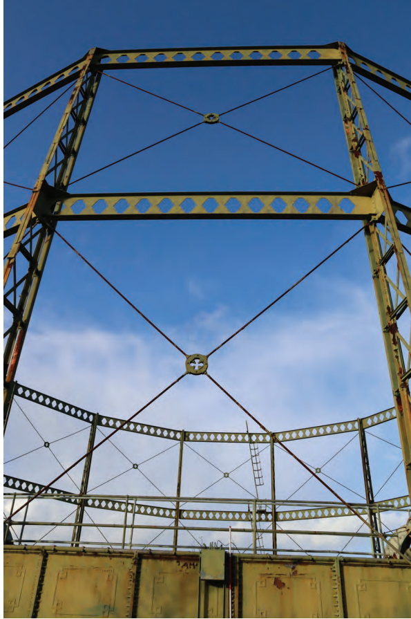
Plate 17: Gasholder No 1, detail view of the guide frame between standards 7 and 8 showing tie-bars and castellated girders, from the SSE
