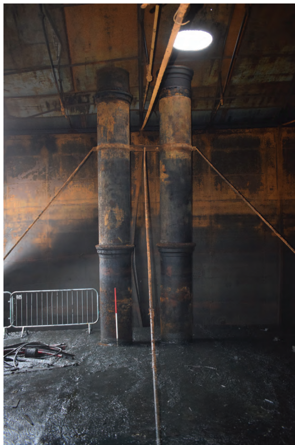
Plate 56: Gasholder No 1, detail view of gas inlet and outlet pipe within the tank, from the SSE
