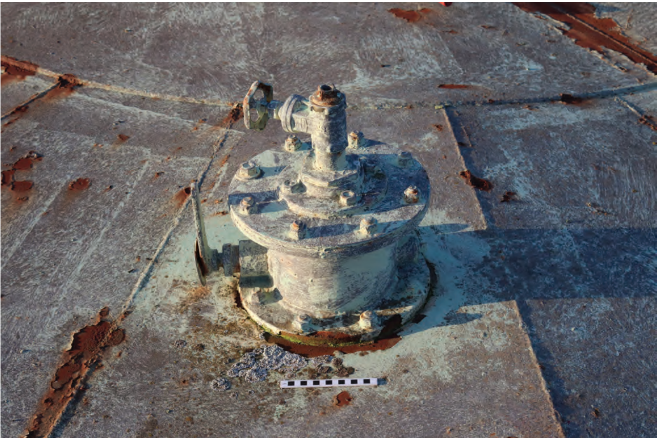
Plate 40: Gasholder No 1, detail view of crown vent just south-east of the centre of the crown, from the south-east
