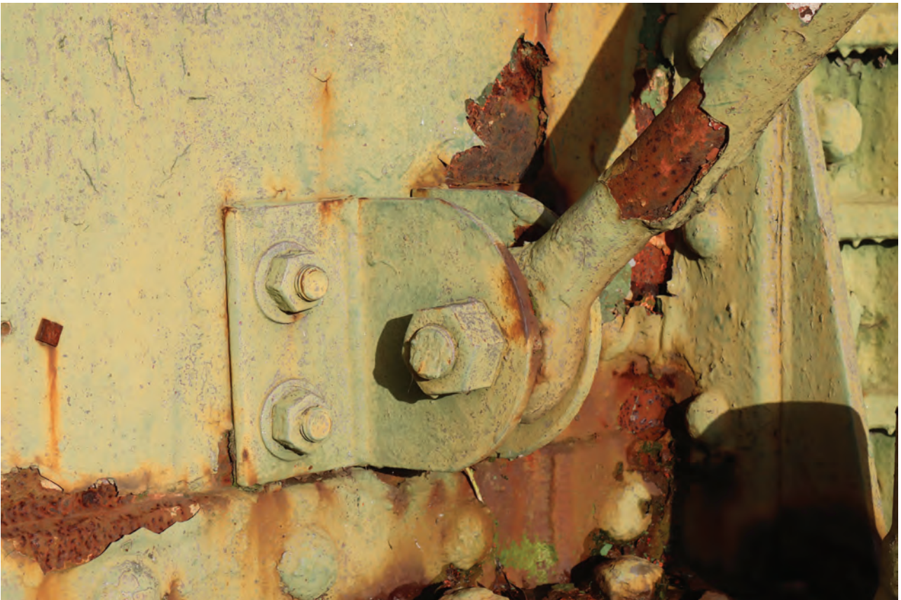
Plate 20: Gasholder No 1, detail view of steel fixture bolted to tie-base and standard 12, from the south-west
