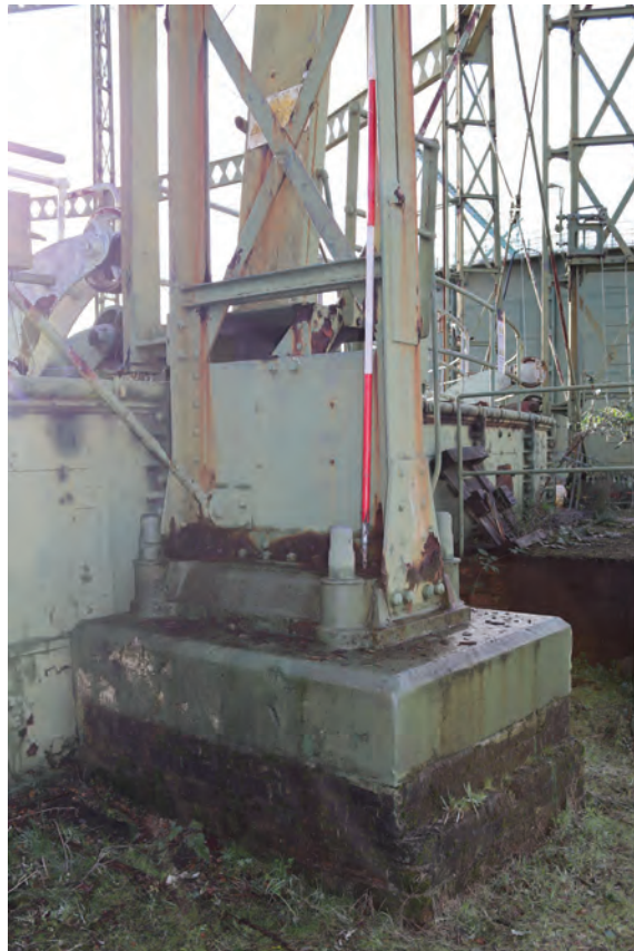
Plate 12: Gasholder No 1, detail view of the base of standard 1, from the north-east
