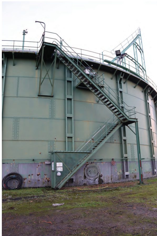
Plate 78: Gasholder No 2, general view of the access stair on the north side of the holder, from the NNE
