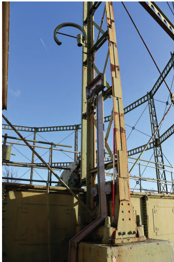
Plate 64: Gasholder No 1, detail view of the north side of standard 12 showing swan neck with missing hose and missing electrical controls below, from the WNW
