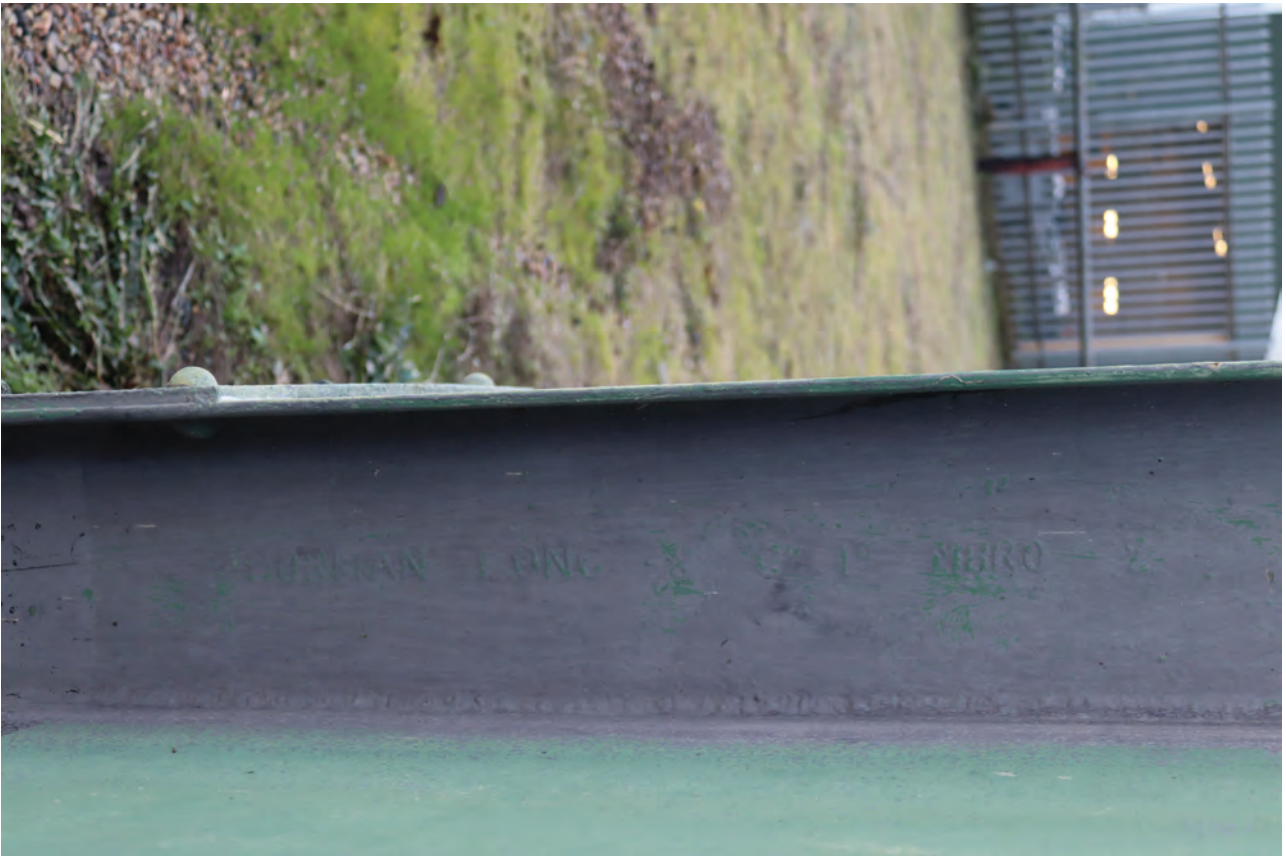
Plate 75: Gasholder No 2, detail view of maker's mark 'DORMAN LONG & CO' on the vertical braces, from the north
