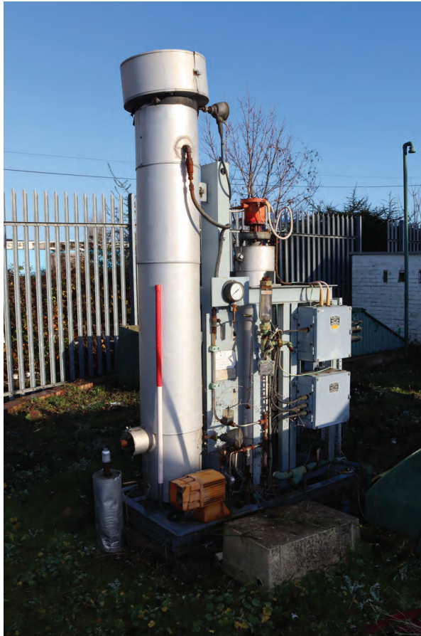
Plate 133: Structure K, general view of the fogger system, from the south-west
