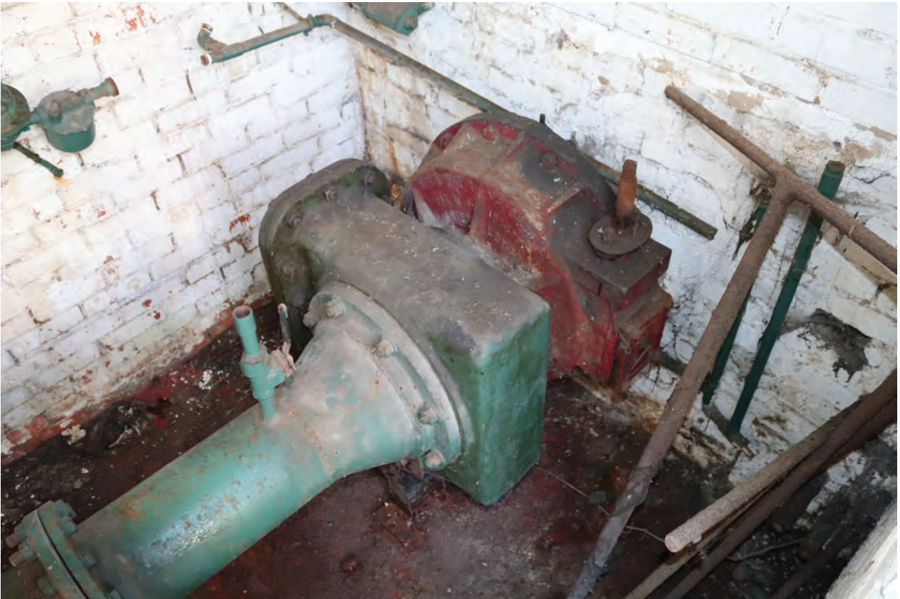
Plate 145: Structure N, detail view of the west end of the volumetric governor pipework with valve, possible filter and manual hand crank apparatus, from the NNE
