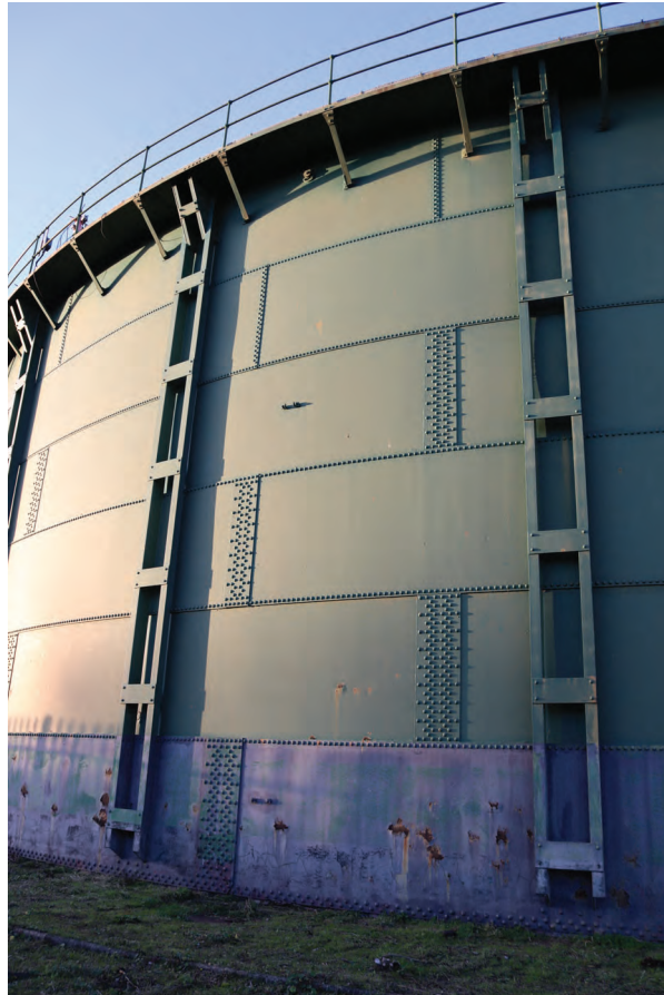
Plate 105: Gasholder No 2, general view of the SSE side of the holder showing fixtures for possible previous overflow pipe, from the south-east
