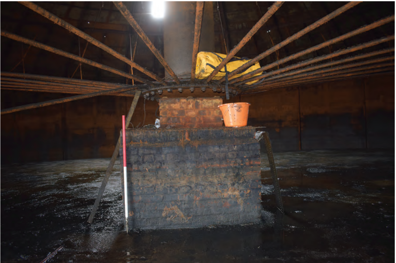
Plate 46: Gasholder No 1, detail view of the brick support block on the dumpling, from the WSW
