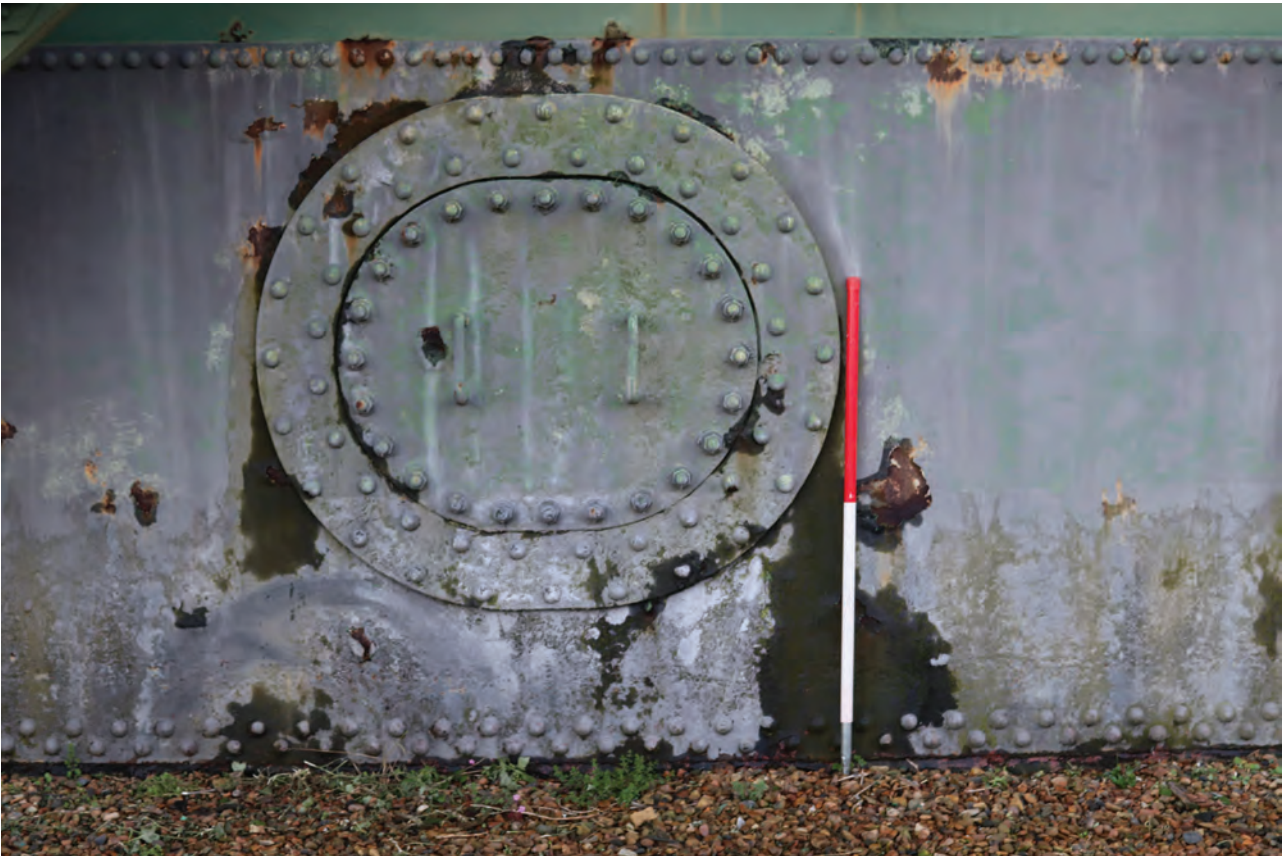
Plate 77: Gasholder No 2, detail view of cotter plate on the north side of the structure, from the north
