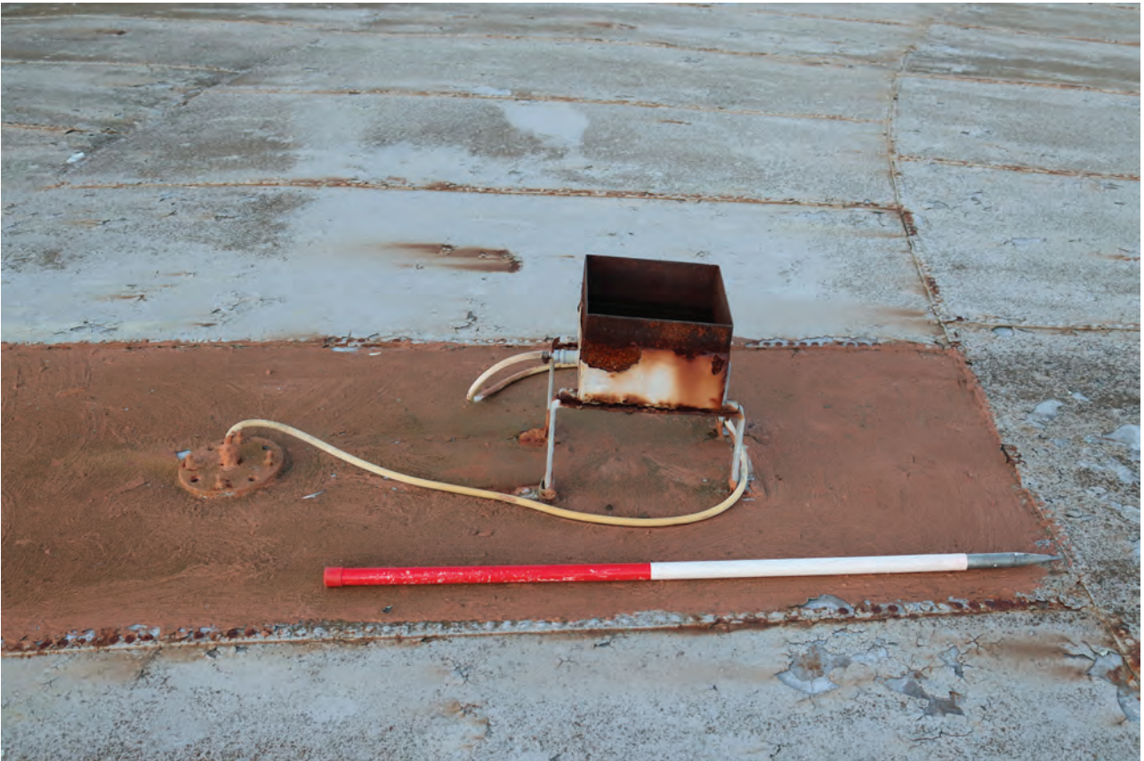
Plate 89 Gasholder No 2, detail view of the glycol pot on the west side of the crown situated within an area of non-slip paint, from the south
