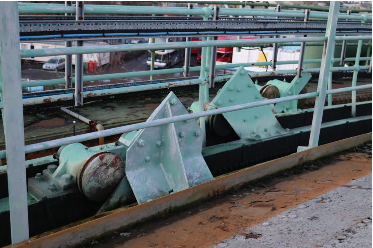
Plate 80: Gasholder No 2, detail view of the different directional guide rails and guide roller pairs, from the south-east
