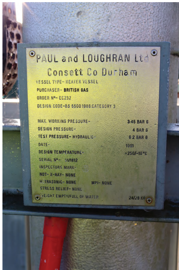
Plate 134: Structure K, detail view of Paul & Loughran Ltd specification on the fogger system, from the north
