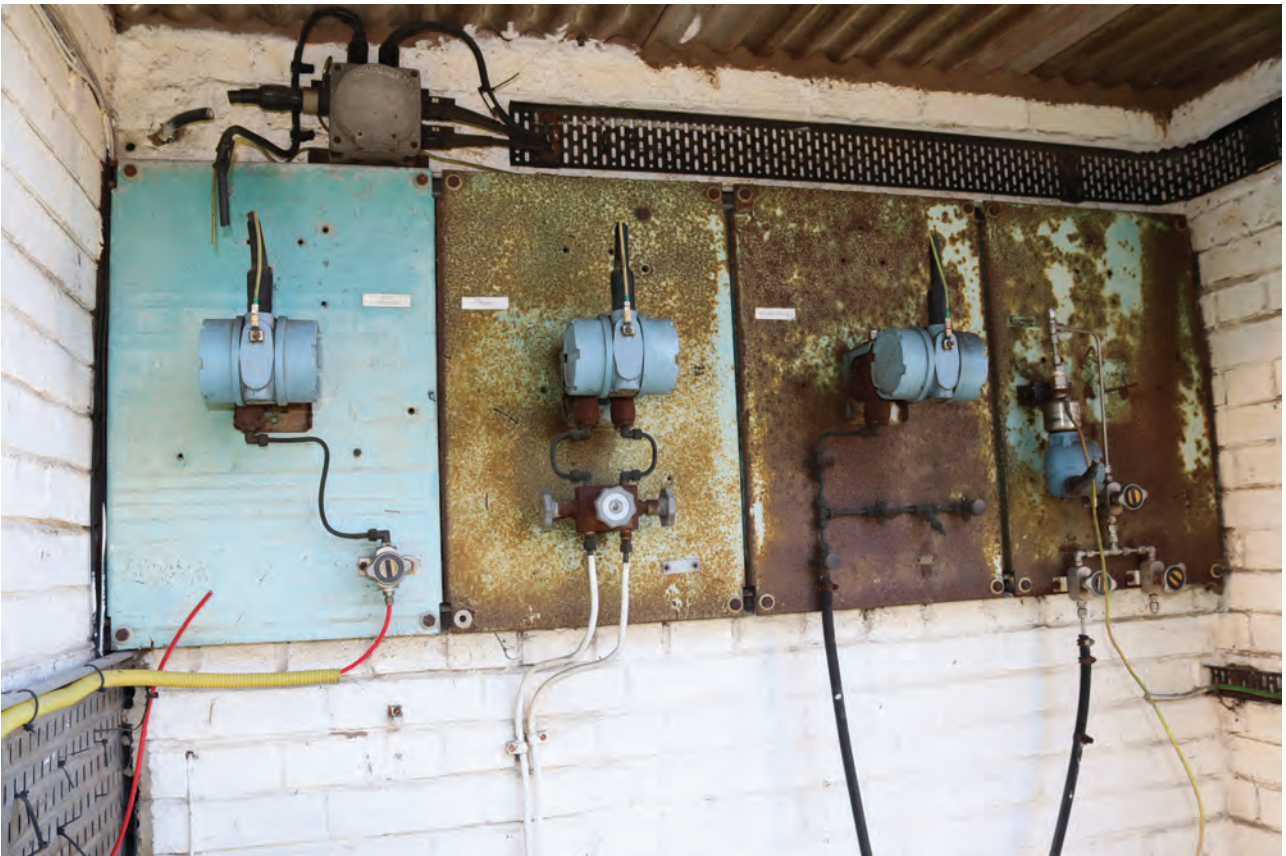
Plate 114: Structure B, detail view of pressure monitoring devices within the shelter at the east end of the building, from the ESE
