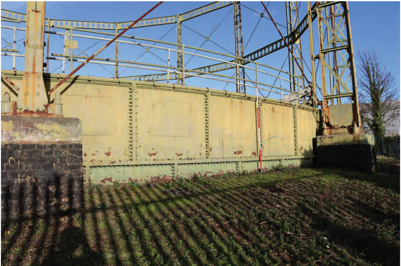
Plate 22: Gasholder No 1, general view of the panelled tank exterior between standards 8 and 9, from the WSW
