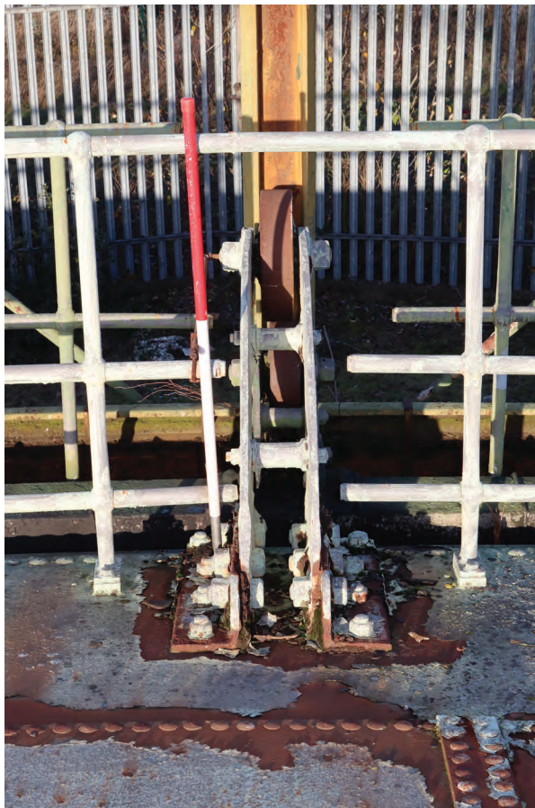
Plate 36: Gasholder No 1, detail view of top guide roller at standard 2 showing bolted bar construction, from the south
