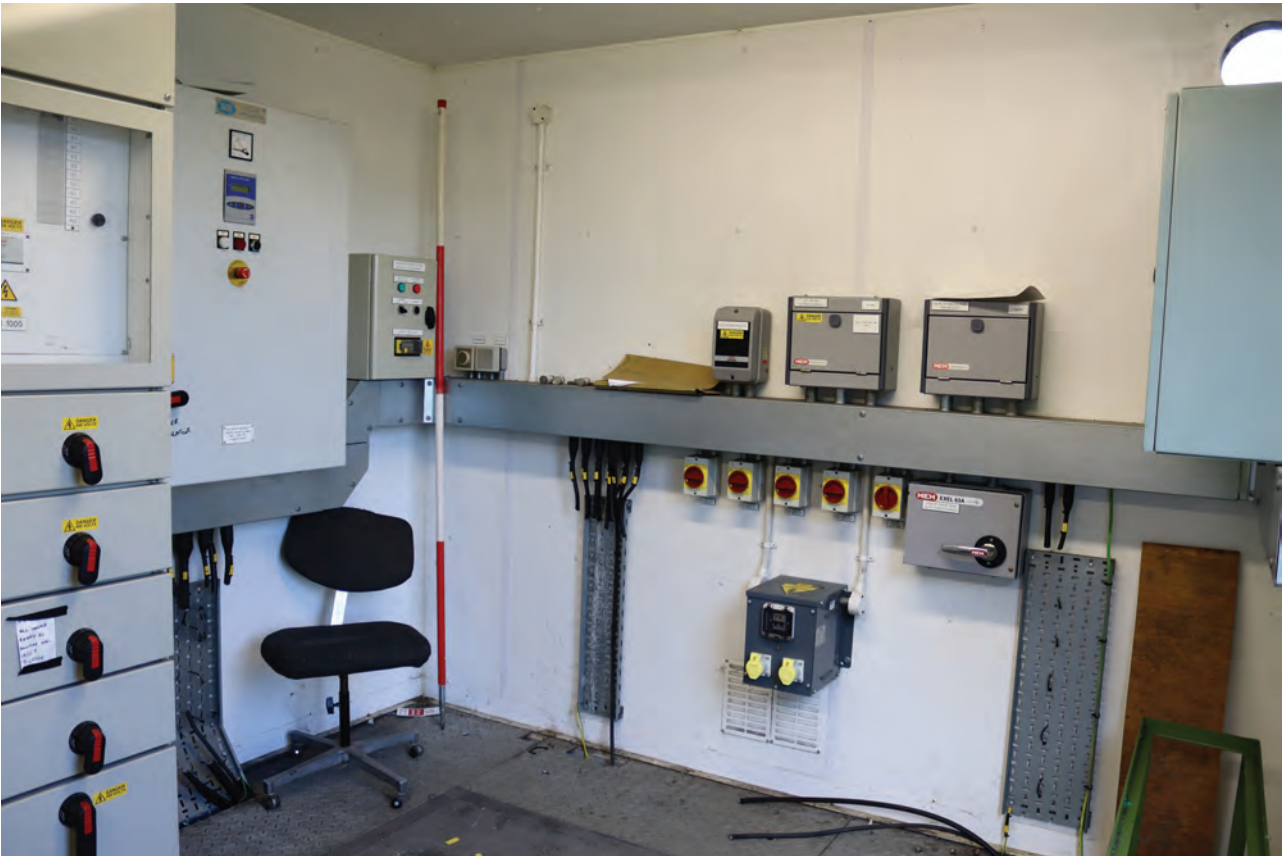
Plate 109: Gasholder No 2 & Structure A, general view of the interior north side showing electrical panels, from the east
