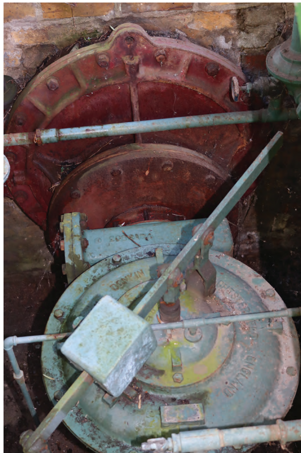
Plate 138: Structure M, detail view of Bryan Donkin weighted diaphragm valve within the grid/district pit, from the WSW
