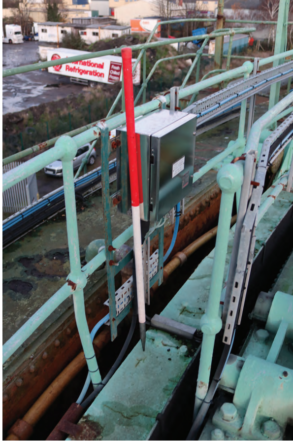
Plate 103: Gasholder No 2, detail view of radial box 1 on the north side of the holder related to the bottom cup-and-grip, from the south-west
