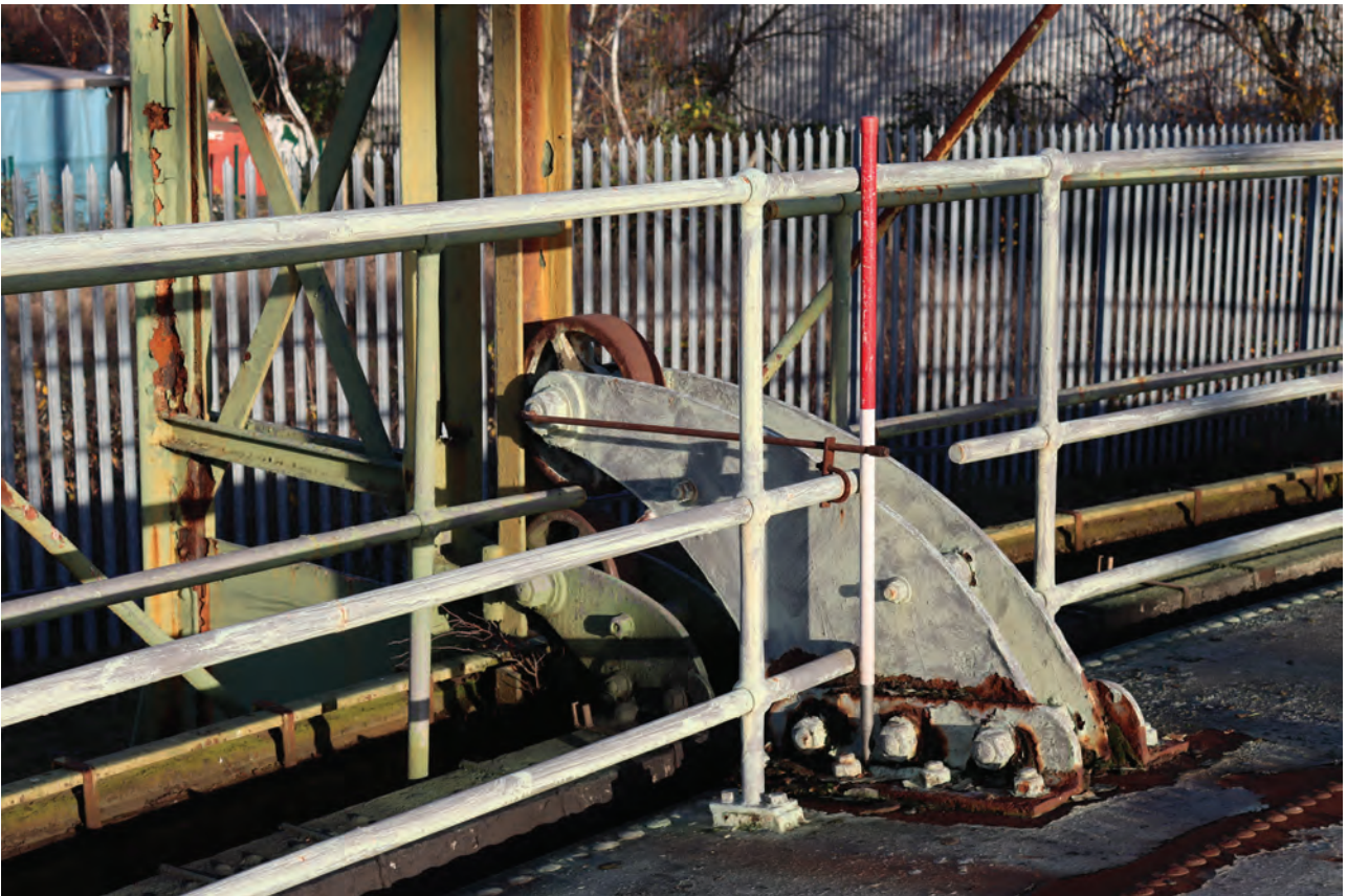
Plate 34: Gasholder No 1, detail view of guide rollers and carriages at standard 23, from the WSW
