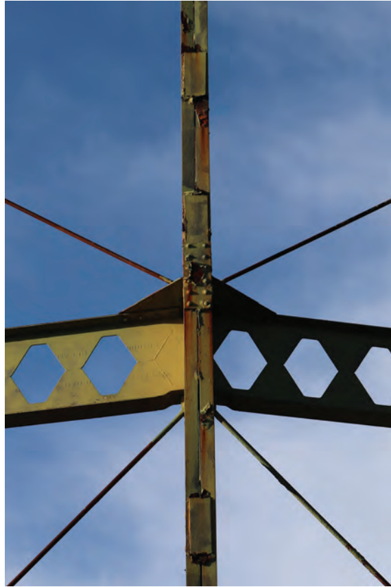
Plate 15: Gasholder No 1, detail view of the south-east side of standard 6 showing welded flange plates and central bolted flange plate, from the ESE
