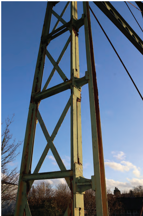
Plate 14: Gasholder No 1, detail view of the lattice work on standard 5, from the NNW
