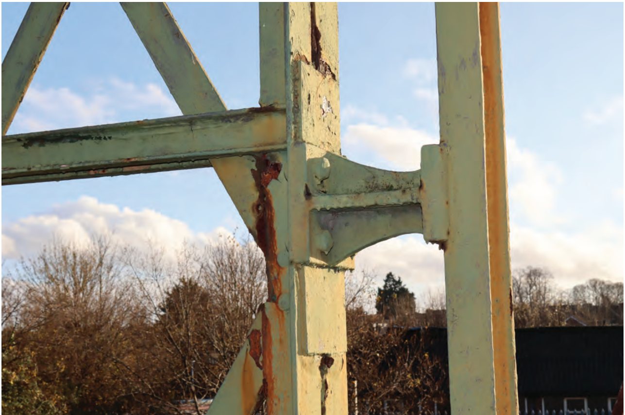
Plate 16: Gasholder No 1, detail view of bracket bolted to standard 5 and welded to a vertical guide rail, from the NNW
