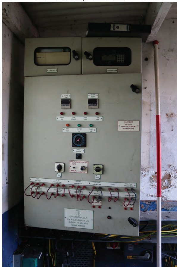
Plate 128: Structure H, detail view of E.V. controller in the electrical services room, from the north
