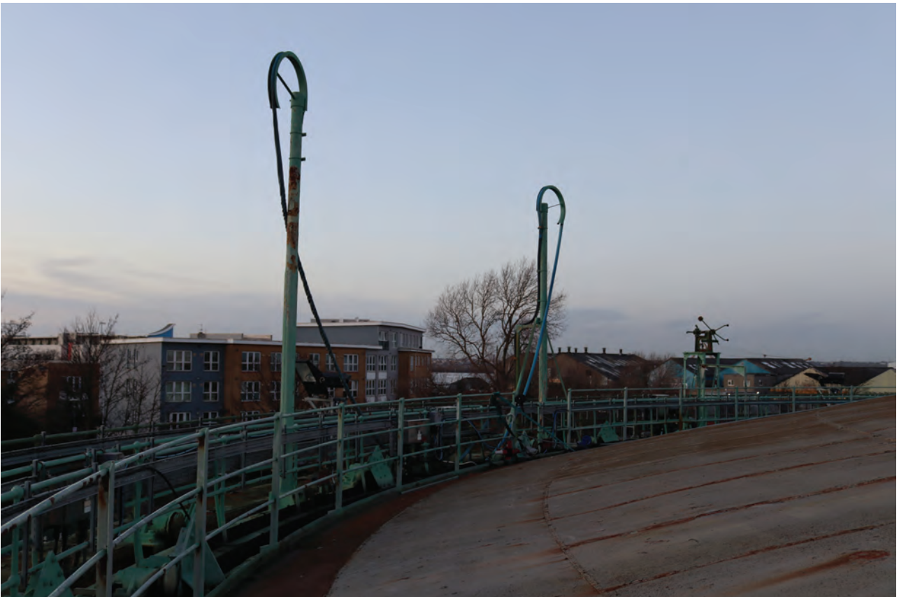
Plate 102: Gasholder No 2, detail view of swan necks on the west side of the holder, from the south-east
