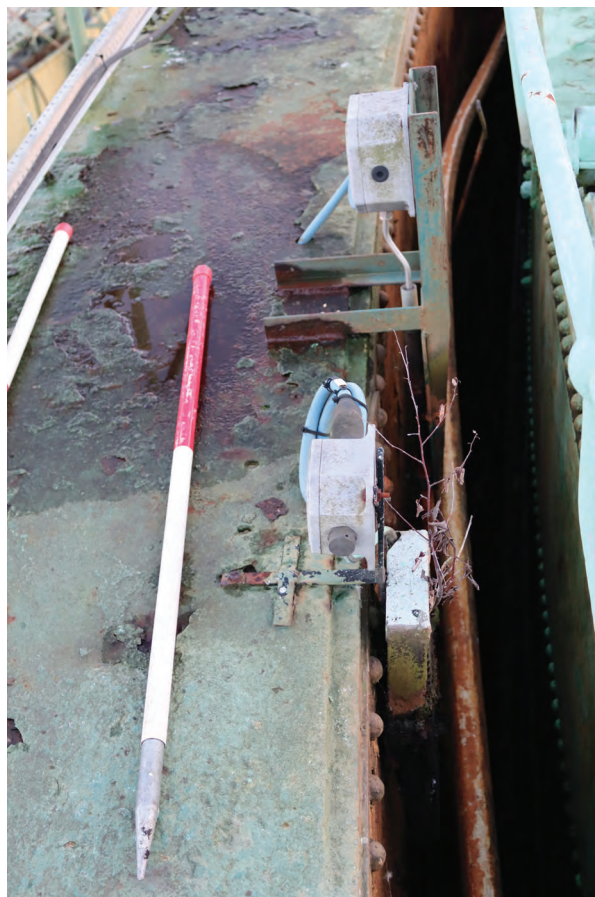
Plate 100: Gasholder No 2, detail view of possible tank water temperature monitoring device, from the north-west
