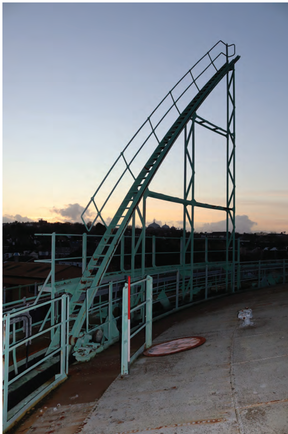
Plate 82: Gasholder No 2, general view of the guide rail and stair structure on the south side of the holder with access onto the crown, from the ENE
