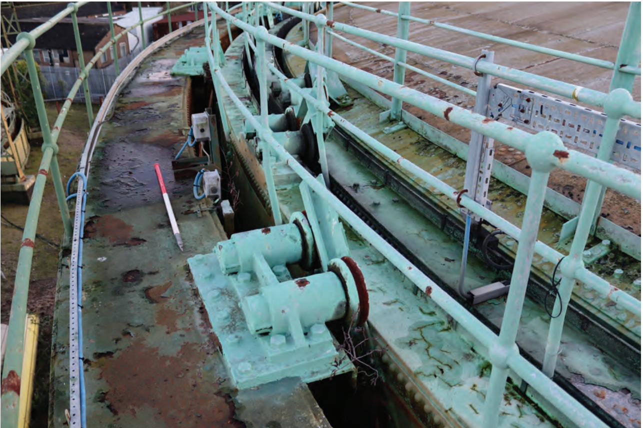
Plate 79: Gasholder No 2, general view of the lift tops showing pairs of tangential rollers, from the NNW
