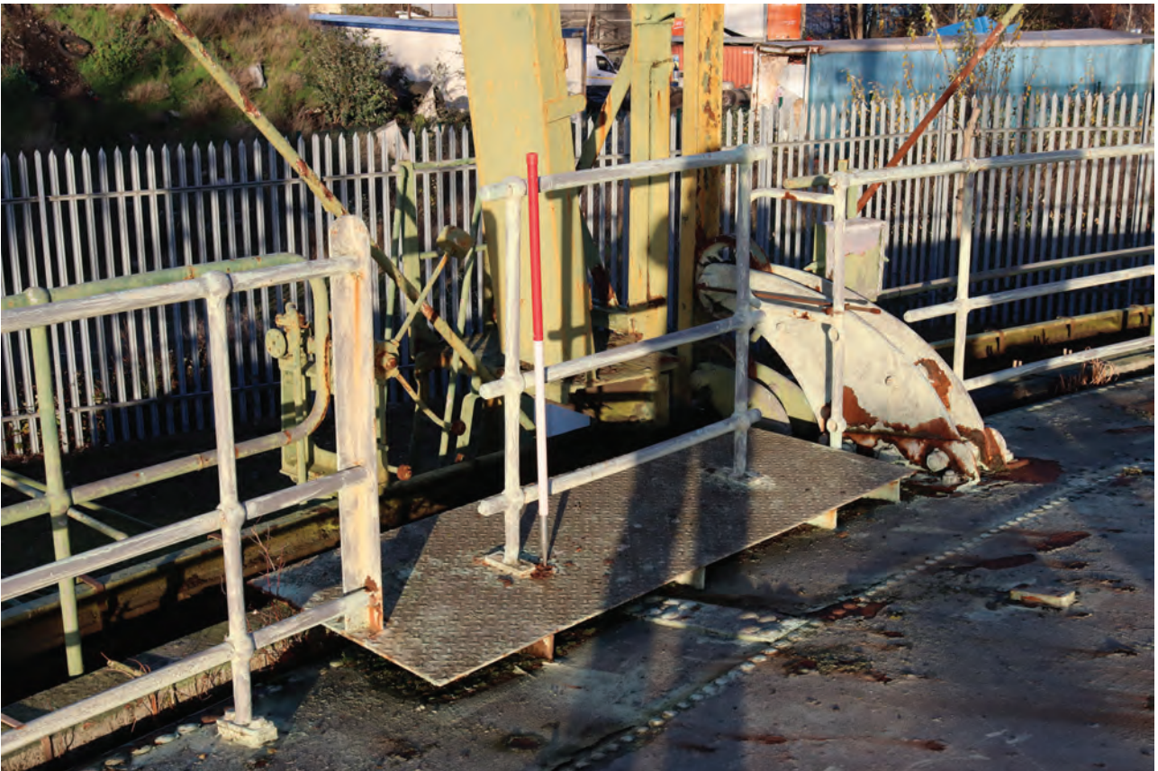
Plate 44: Gasholder No 1, detail view of access platform onto the NNW side of the crown, from the south-west
