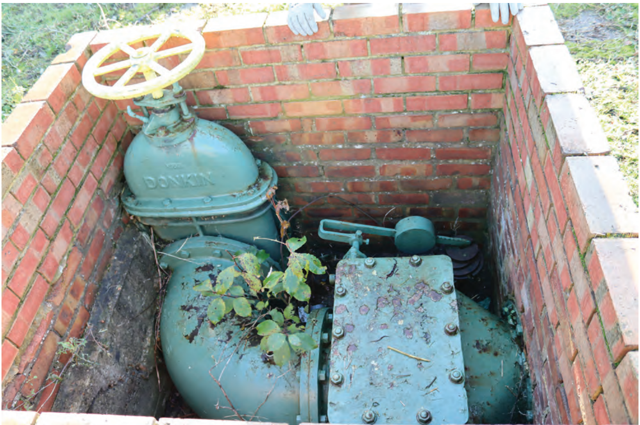
Plate 122: Structure F, detail view of brick-lined valve pit containing gate valve and # valve, from the north
