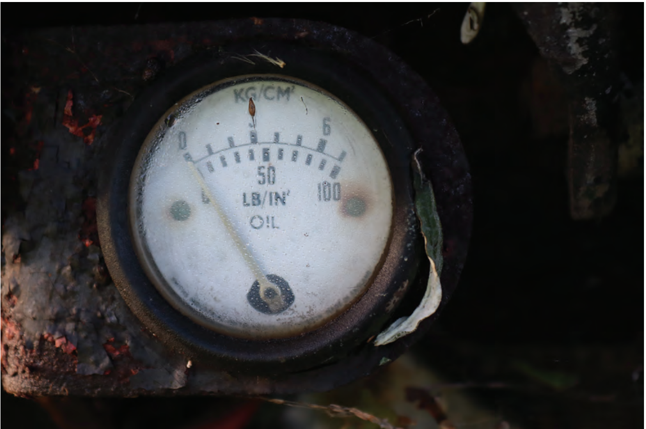
Plate 124: Structure G, detail view of oil gauge on the standby generator, from the west
