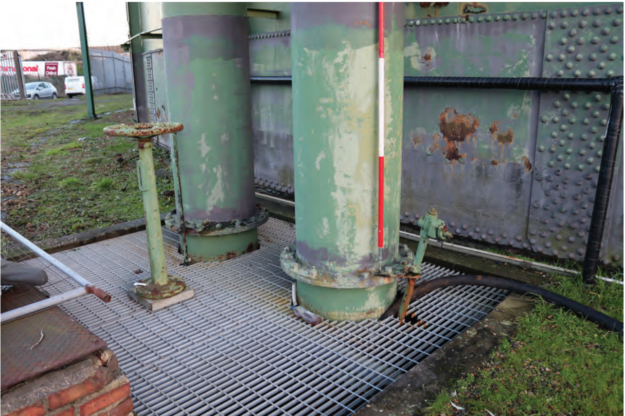
Plate 92: Gasholder No 2, detail view of the base of the gas inlet pipe set within a pit with pipe vents and manual valve control wheel, from the west
