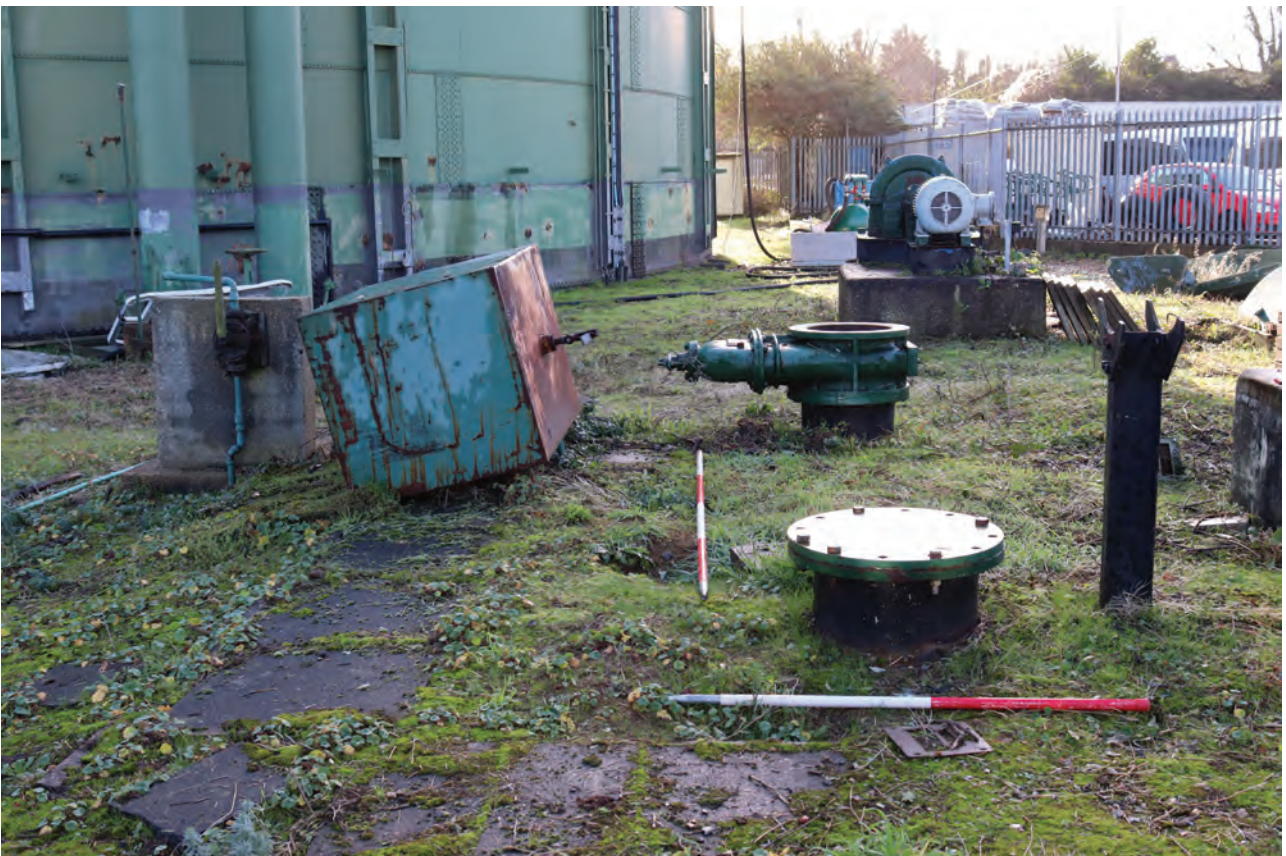
Plate 148: Structure Q, general view of two blanked pipe sections, from the north
