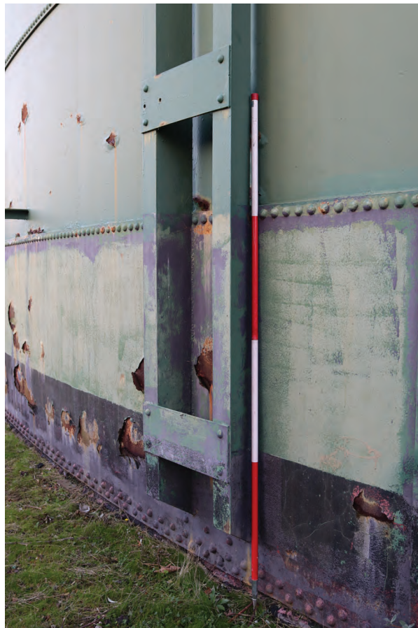
Plate 74: Gasholder No 2, detail view of the base of a vertical brace welded to the tank, from the south-west
