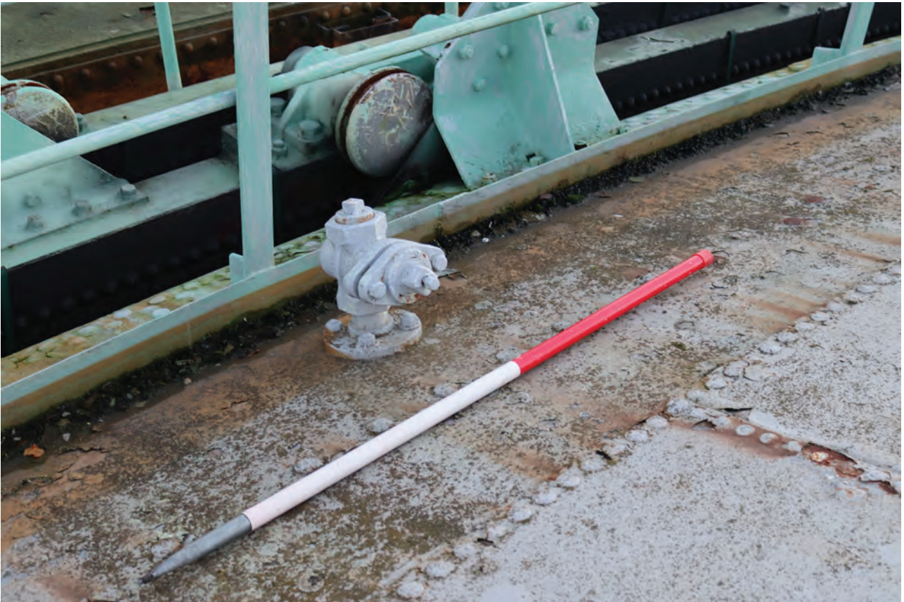
Plate 87: Gasholder No 2, detail view of crown vent on the south-east side, from the north
