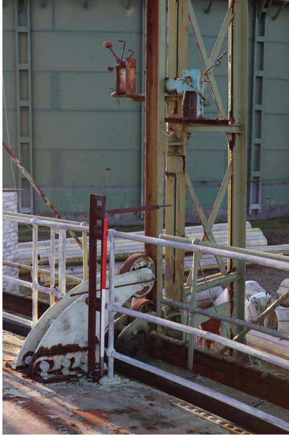
Plate 59: Gasholder No 1, detail view of knock-off switches and associated striker plate at standard 13, from the ENE
