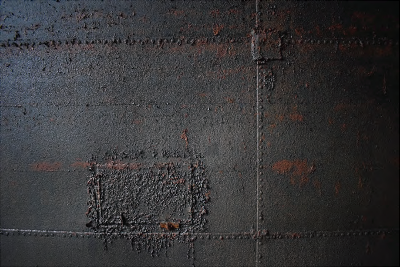
Plate 31: Gasholder No 1, detail view of welded repair patches on the top lift wall interior, from the south
