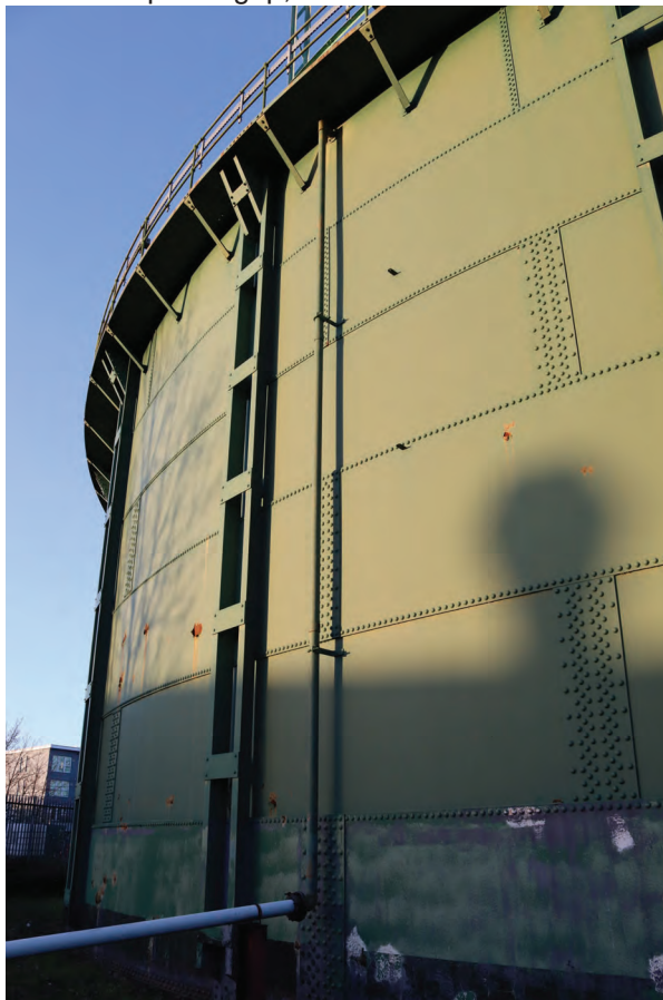
Plate 104: Gasholder No 2, detail view of overflow pipe on the south-west side of the holder, from the south-east
