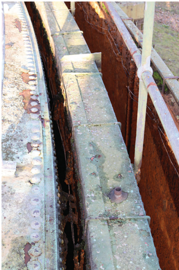
Plate 60: Gasholder No 1, detail view of heating elements clipped to the lower lift and tank wall between standards 5 and 6, from the SSW
