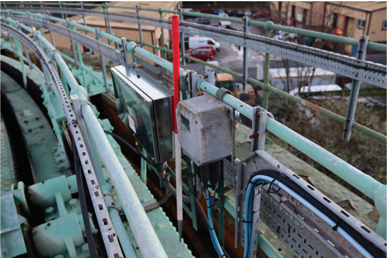
Plate 98: Gasholder No 2, detail view of the bottom lift antifreeze distribution board, from the north
