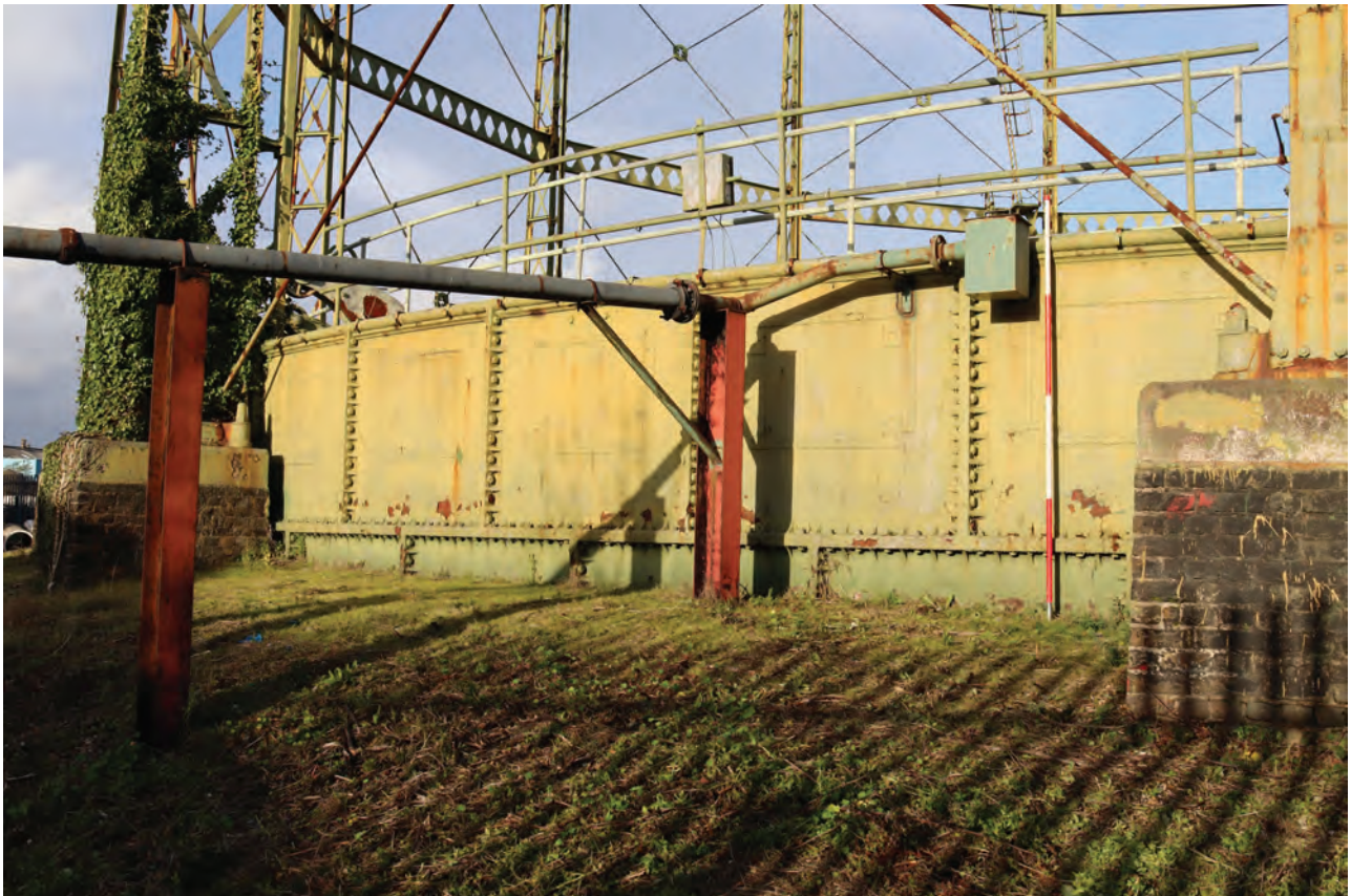
Plate 66: Gasholder No 1, detail view of overflow pipe leaving the gasholder between standards 9 and 10, from the SSE
