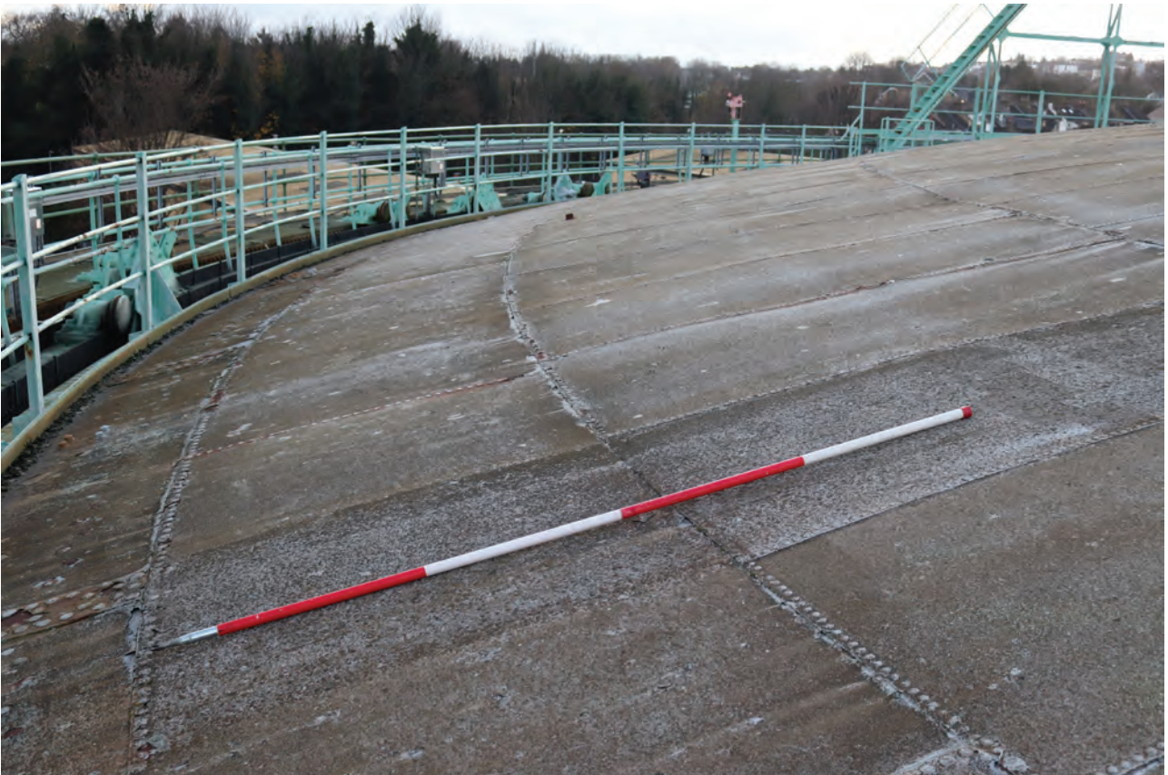
Plate 84: Gasholder No 2, general view of the domed crown constructed of riveted steel sheets, from the NNE
