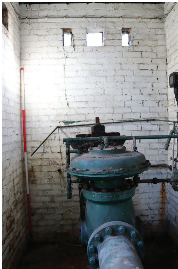
Plate 142: Structure N, general view of the volumetric governor and governor house east end, from the west
