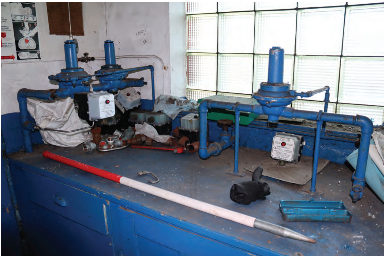
Plate 130: Structure H, general view of instrumentation in the instrument room, from the south-east
