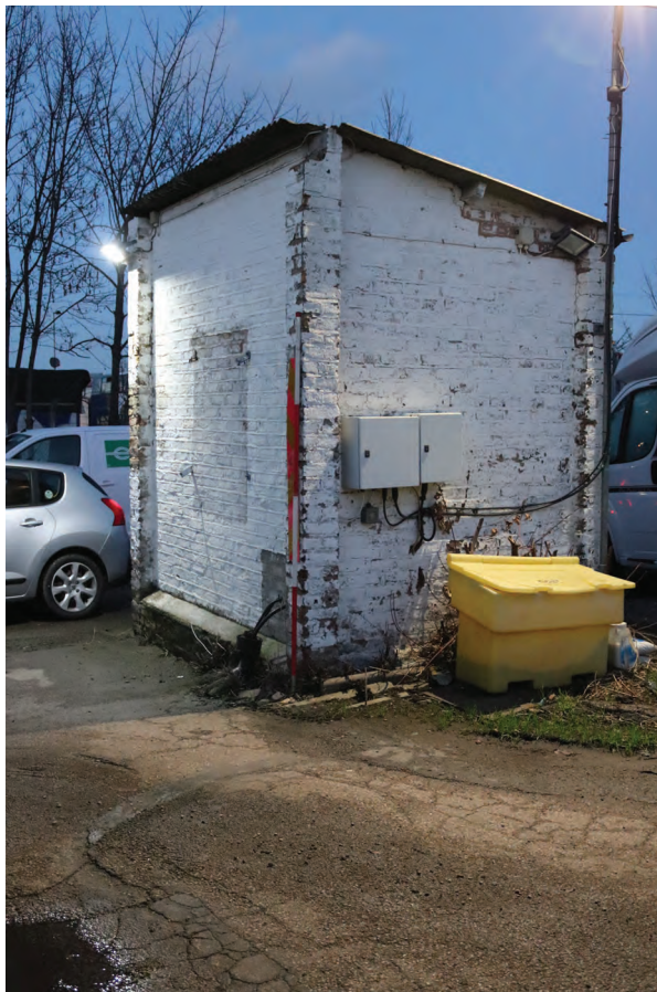
Plate 154: Structure T, general view of the exterior SSE and WSW walls showing exterior electrical panels, from the south-west
