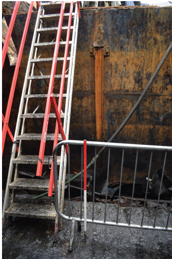
Plate 37: Gasholder No 1, detail view of guide rail bolted to the tank wall, from the south-east
