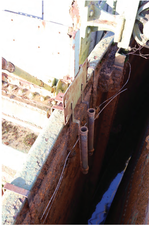
Plate 63: Gasholder No 1, detail view of tank float switch on the south side of standard 12, from the SSE
