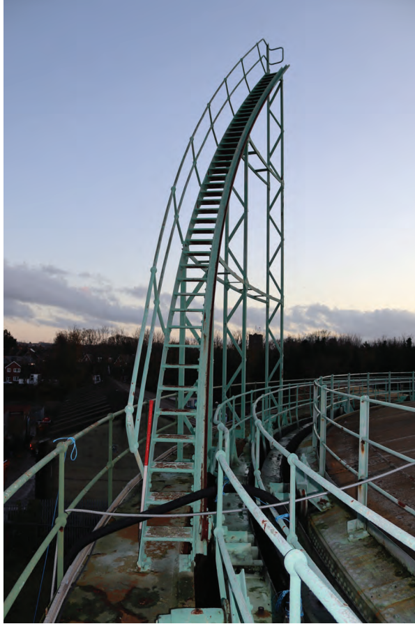
Plate 81: Gasholder No 2, detail view of guide rail and stair structure on the east side of the holder, from the north
