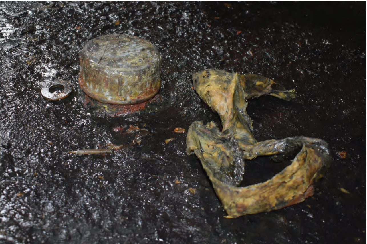
Plate 28: Gasholder No 1, detail view of metal cap with removed bitumen-soaked cloth, from the south
