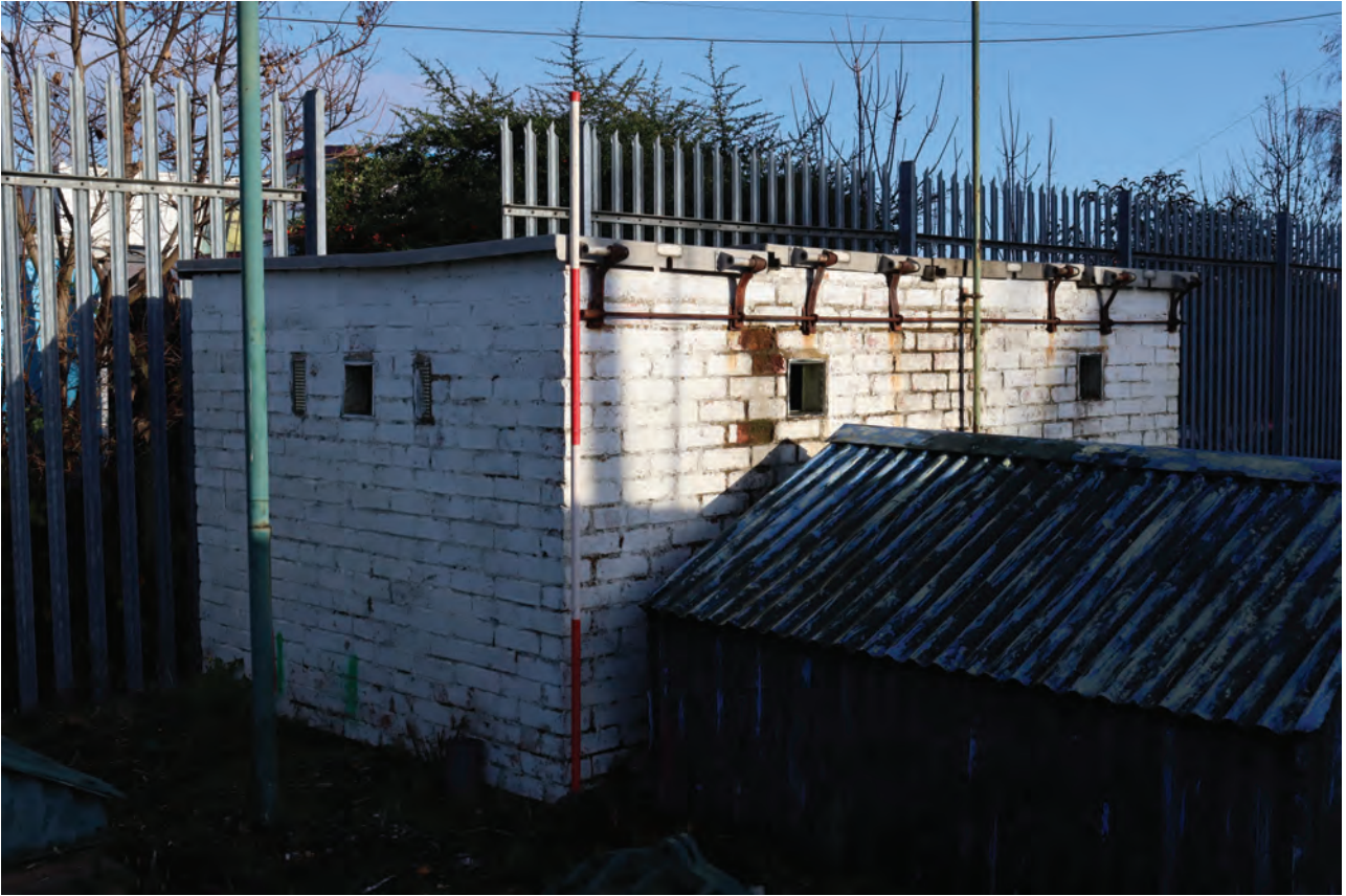
Plate 139: Structure N, general view of the WSW and SSE walls, from the south-west
