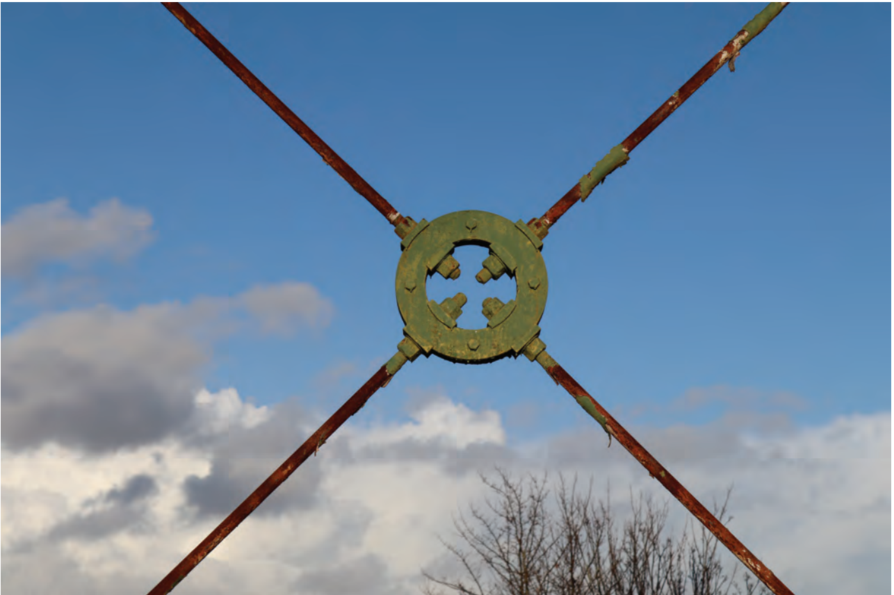
Plate 19: Gasholder No 1, detail view of tension ring between standards 2 and 3, from the SSW
