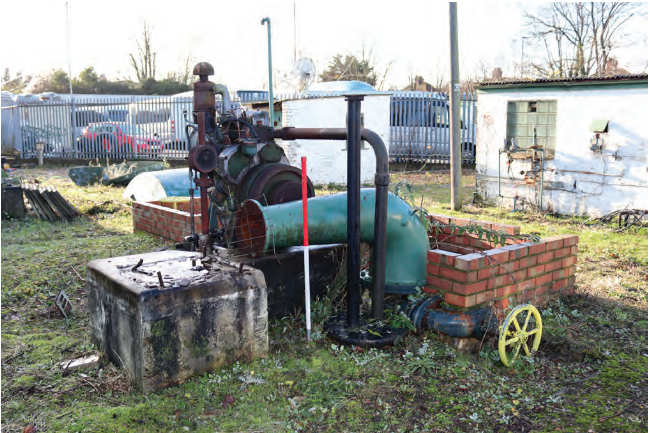
Plate 123: Structure G, general view of standby generator and valve pit showing yellow manual valve control wheel, from the north-east
