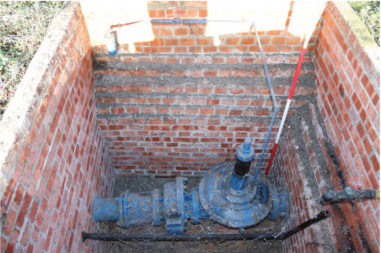
Plate 119: Structure D, general view of brick-lined pit with pipe and valve, from the south
