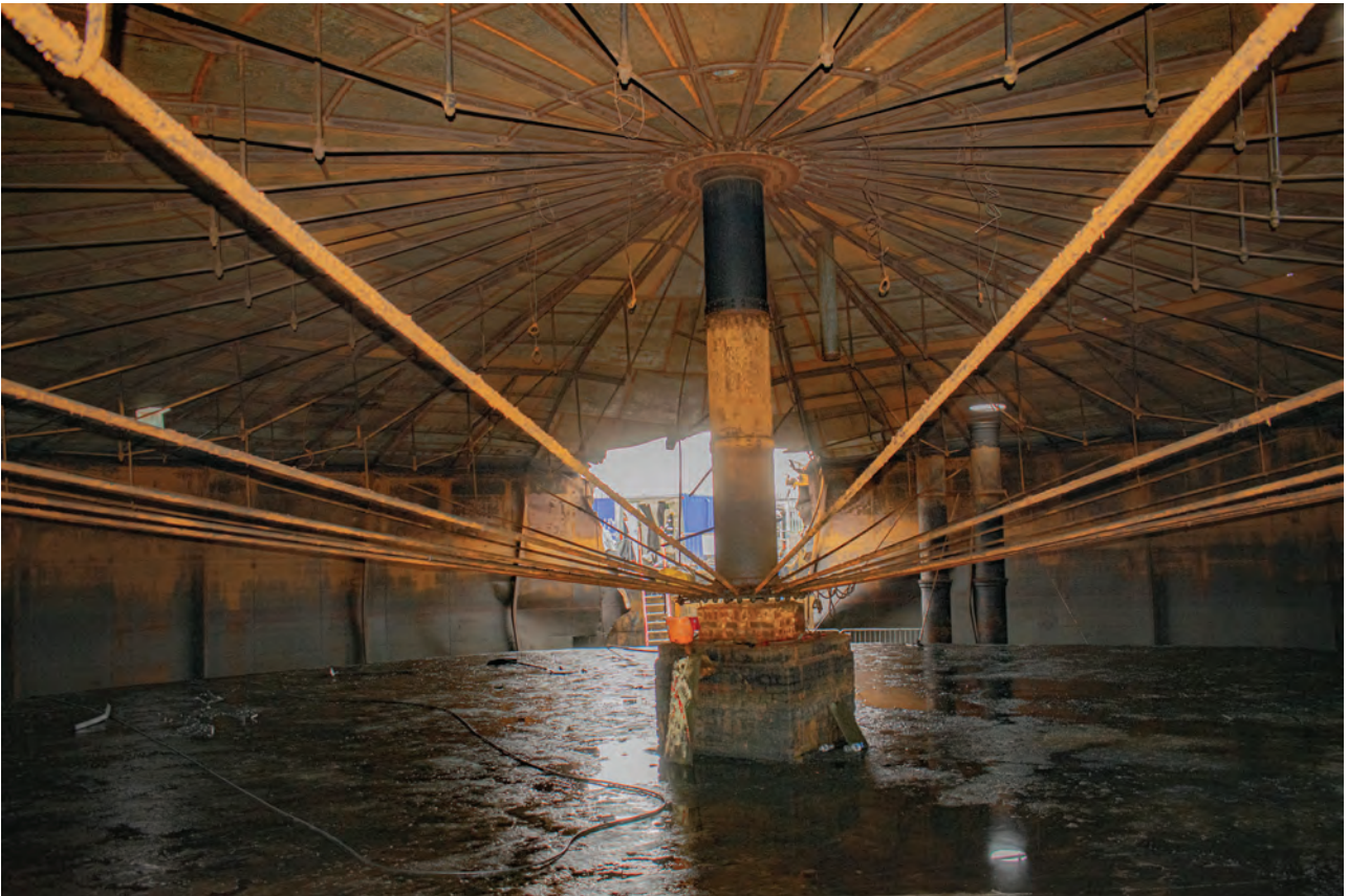
Plate 45: Gasholder No 1, general view of the crown truss frame, from the south-east
