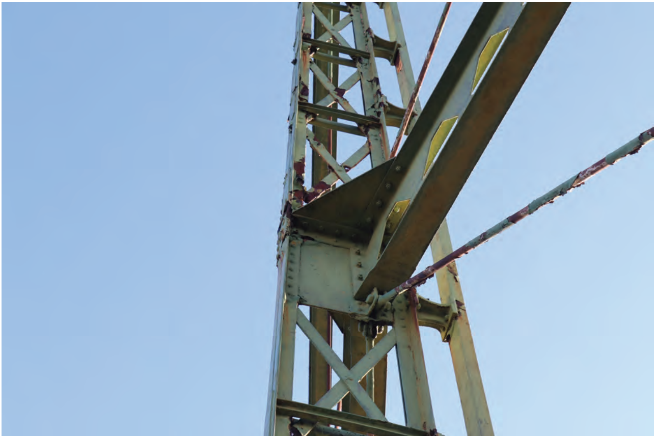
Plate 18: Gasholder No 1, detail view of girder bolted to standard 3 and gusset plate above, from the NNW
