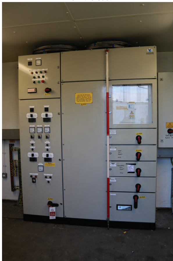
Plate 110: Gasholder No 2 & Structure A, detail view of monitoring and control device relating to the anti-freeze system and top-up pump of Gasholder No 2, from the north-east
