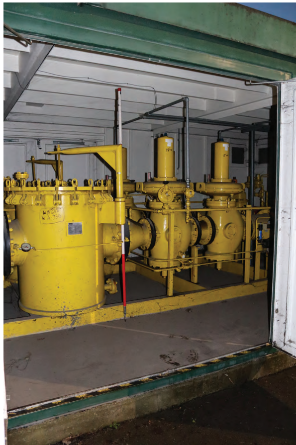
Plate 156: Structure U, general view of the district governor including filter and pressure reducing valves, from the south-east
