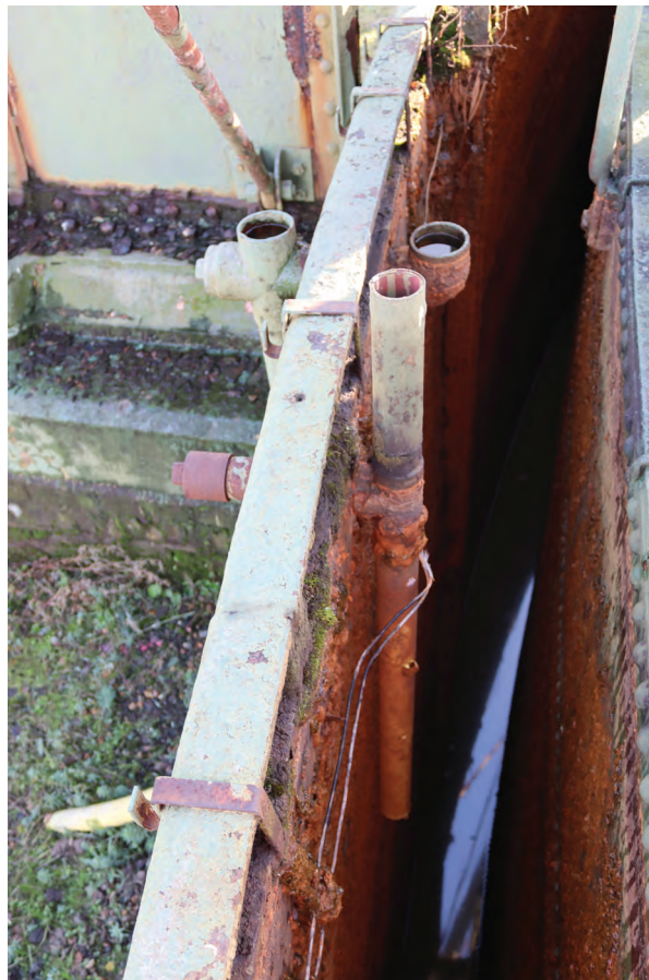
Plate 68: Gasholder No 1, detail view of previous overflow pipe to the north of standard 5, from the north
