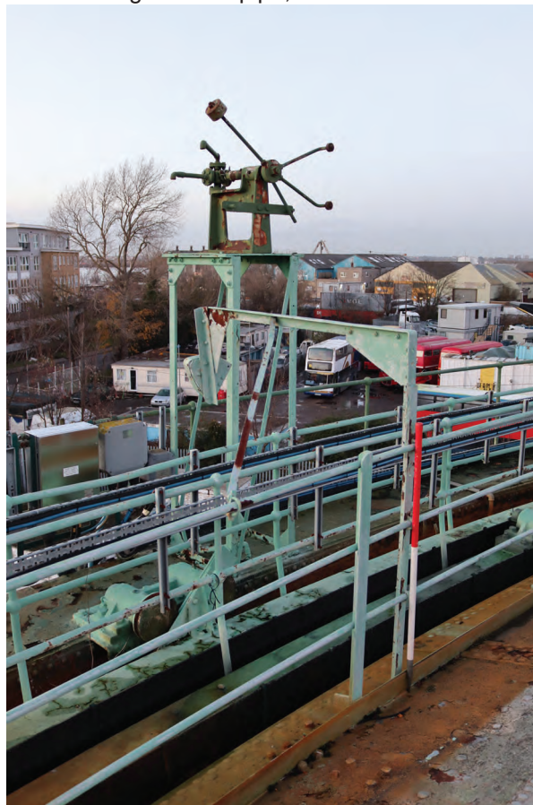
Plate 96: Gasholder No 2, detail view of gasmatic knock-off switch and associated striker arm on the north-west side of the holder, from the SSW
