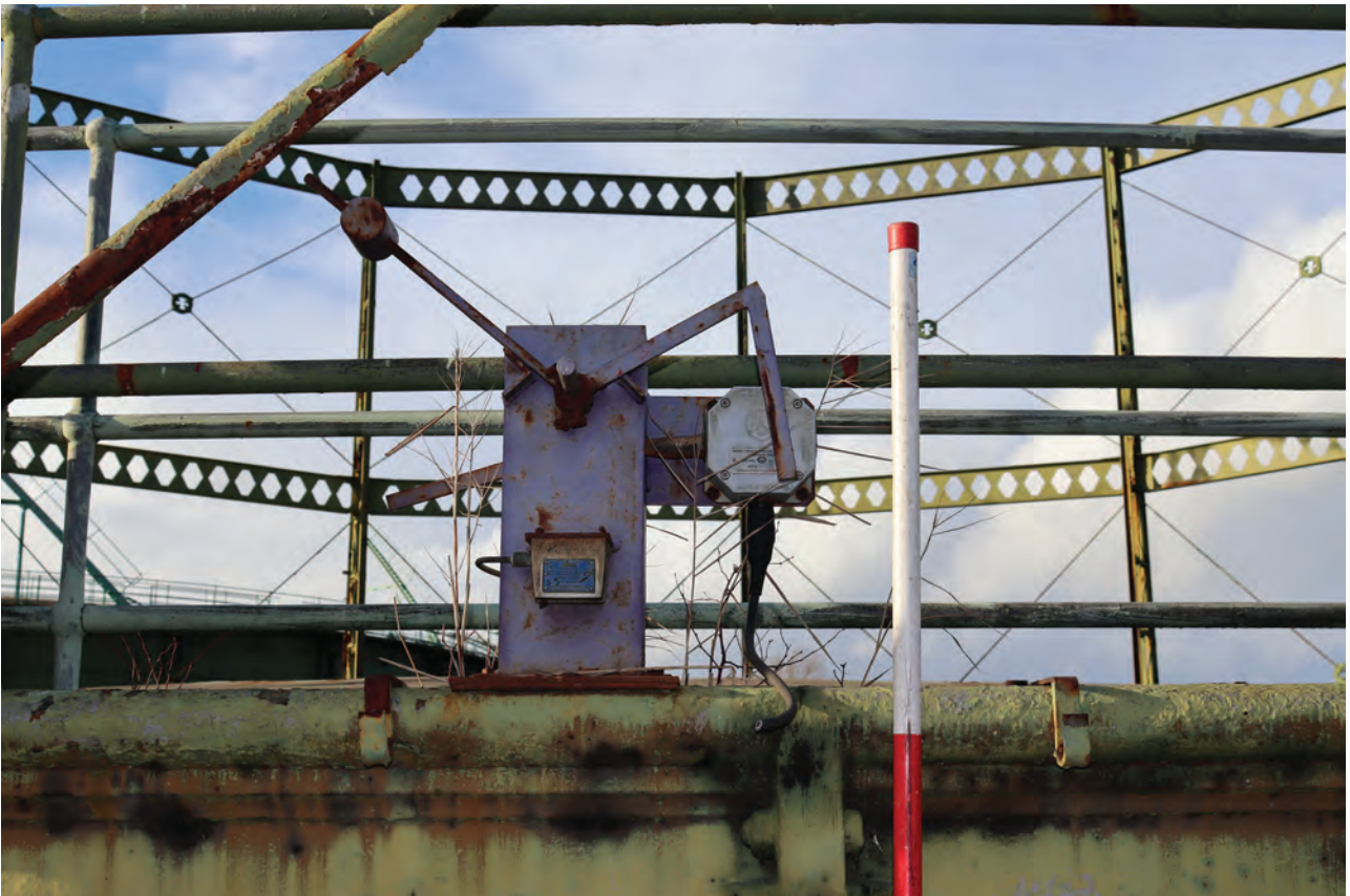
Plate 58: Gasholder No 1, detail view of knock-off switch attached to the tank to the north of standard 6, from the ESE
