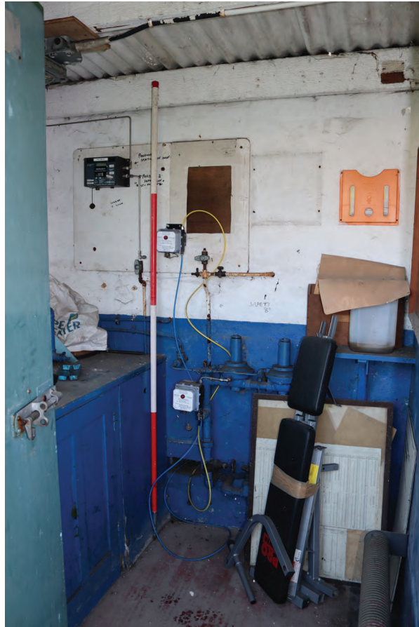
Plate 129: Structure H, general view of instrumentation in the instrument room, from the WSW
