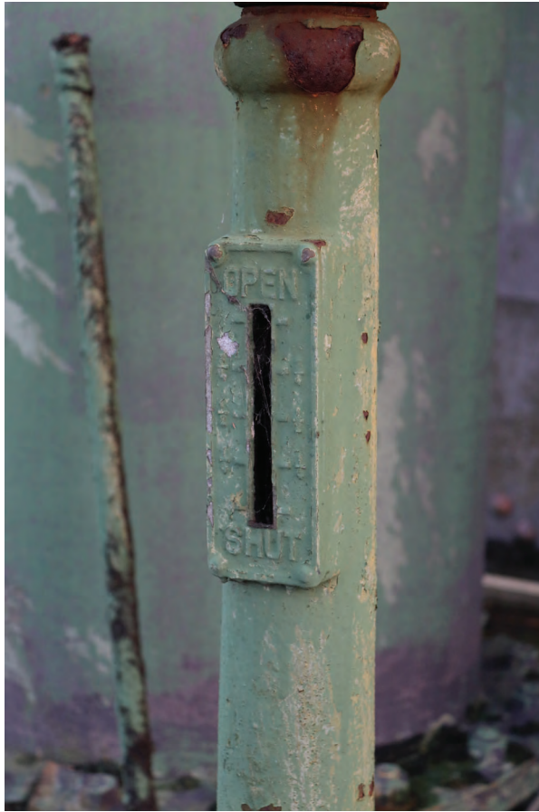
Plate 93: Gasholder No 2, detail view of the open/shut manual valve control wheel at the gas outlet, from the NNW
