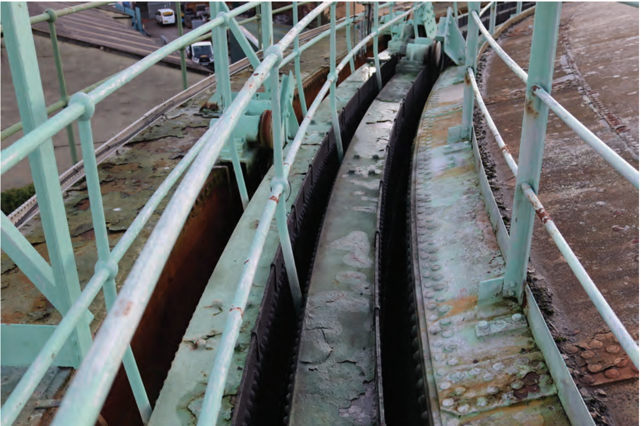
Plate 83: Gasholder No 2, general view of the lift tops showing square grips, from the NNE
