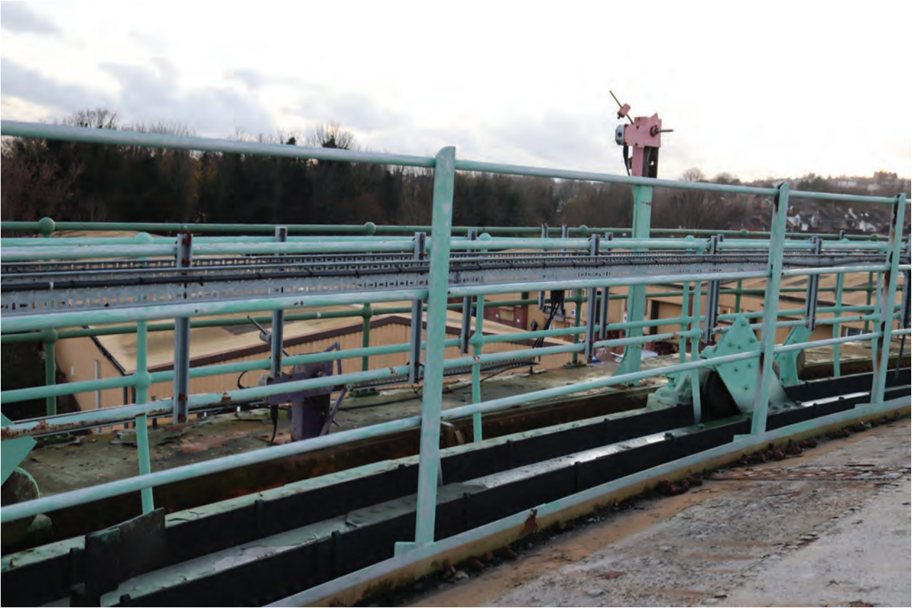
Plate 97: Gasholder No 2, general view of the knock-off switches on the south side of the holder, from the north-east
