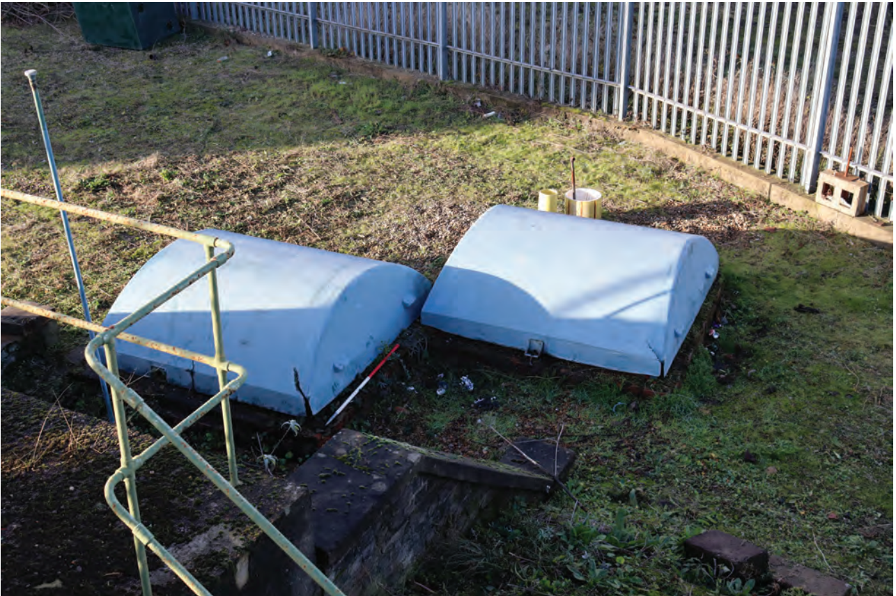
Plate 55: Gasholder No 1, detail view of valve pits related to the inlet and outlet pipes, from the south-east
