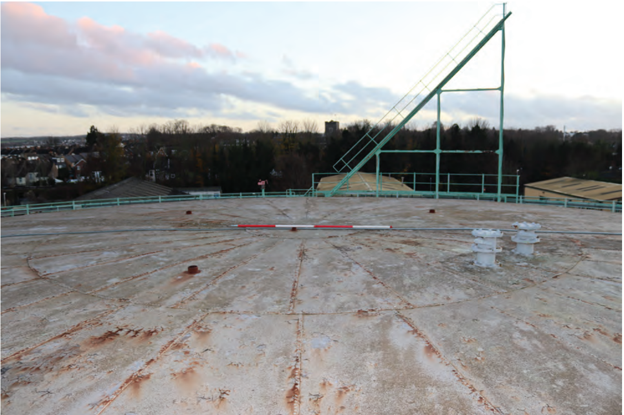
Plate 85: Gasholder No 2, general view of the centre of the crown, from the north
