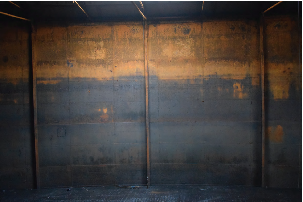
Plate 30: Gasholder No 1, detail view of the top lift wall interior showing riveted sheet and rigid stanchion design, from the north-east
