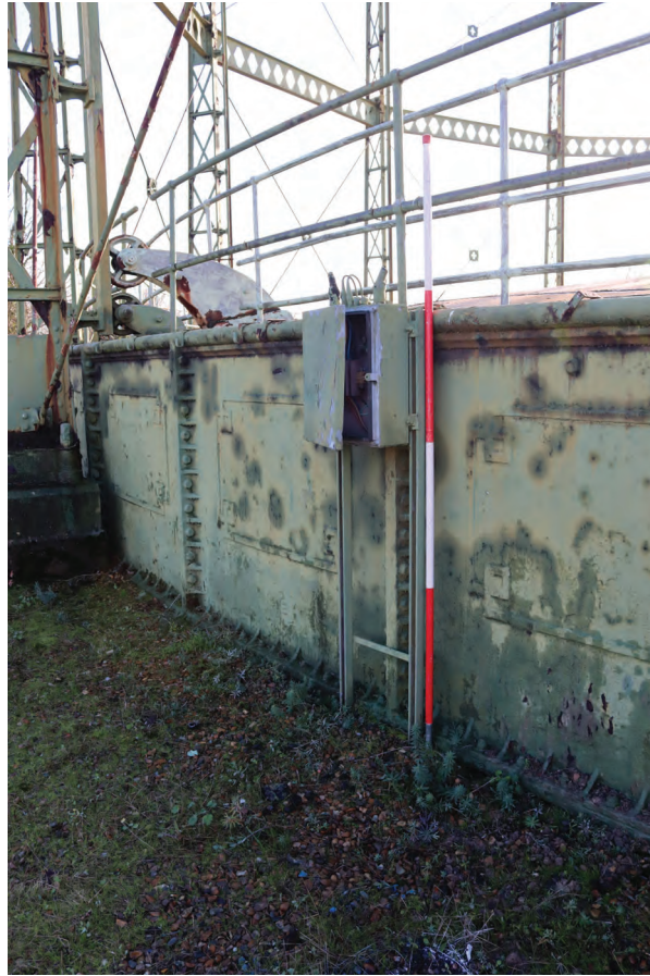
Plate 65: Gasholder No 1, detail view of blanked electronic box between standards 2 and 3 related to automated gasholder running procedures, from the NNW
