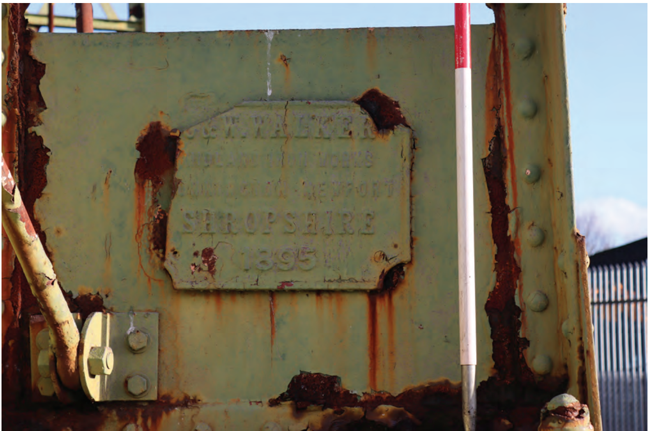
Plate 10: Gasholder No 1, maker's plate on the west side of standard 9 identifying C & Walker as the builders in 1895, from the WNW
