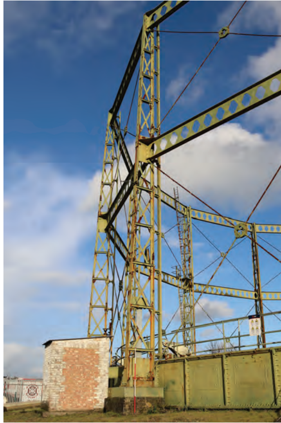
Plate 11: Gasholder No 1, general view of the south side of standard 12, from the SSW
