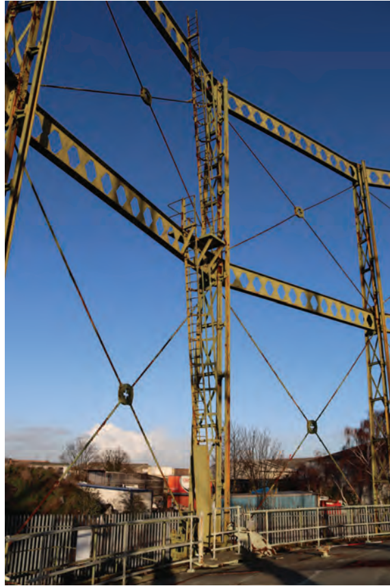
Plate 21: Gasholder No 1, general view of two middle and upper ladder on the exterior north side of the guide frame, from the south-west
