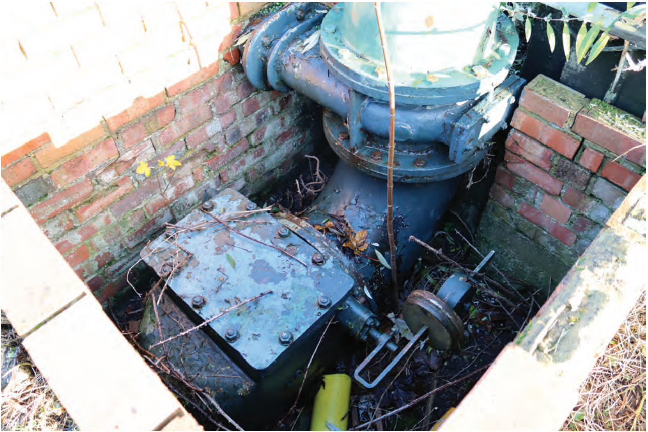
Plate 125: Structure G, detail view of valve pit and valve, from the south-west
