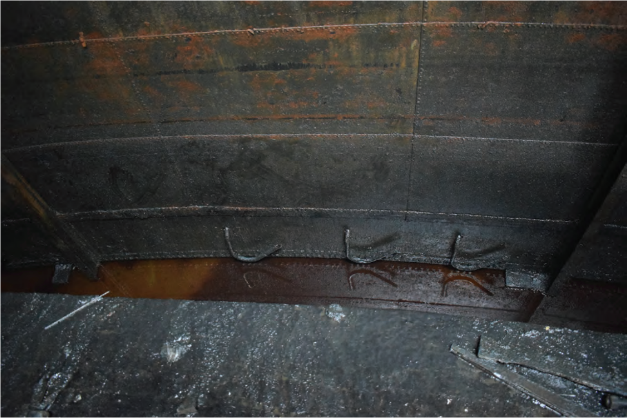
Plate 33: Gasholder No 1, detail view of grip overflow pipes situated at the base of the top lift wall interior, from the north
