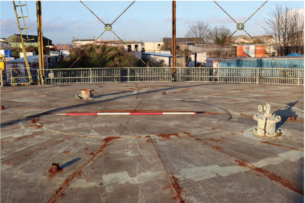
Plate 39: Gasholder No 1, general view of the centre of the crown showing semi-circular iron sheet, crown vents and purge points, from the south
