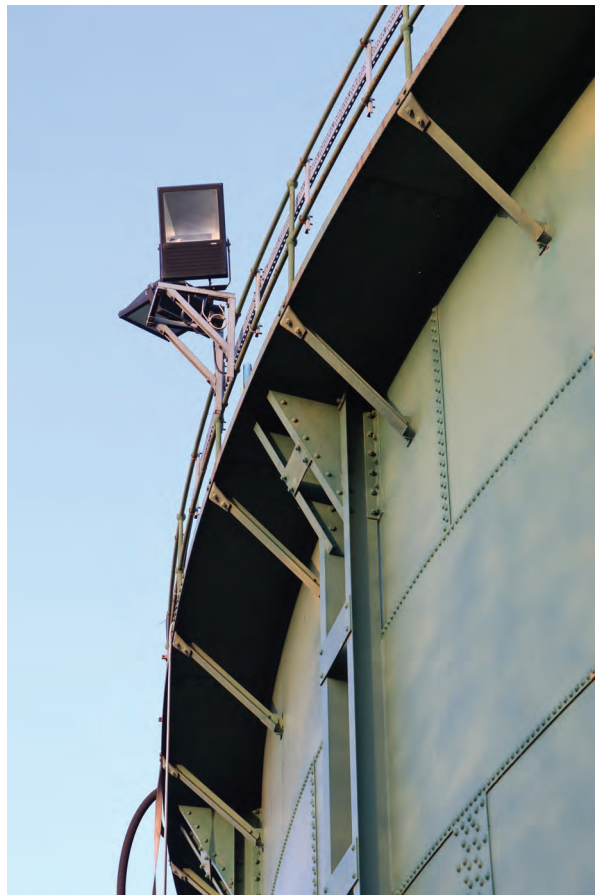
Plate 76: Gasholder No 2, detail view of triangular top to the vertical braces and floodlight on the west side of the holder, from the south
