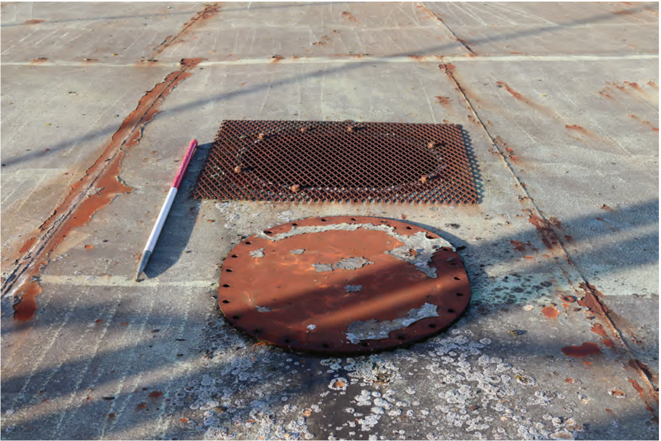
Plate 43: Gasholder No 1, detail view of removed cotter plate and aeration grate added on the SSE of the crown, from the SSE
