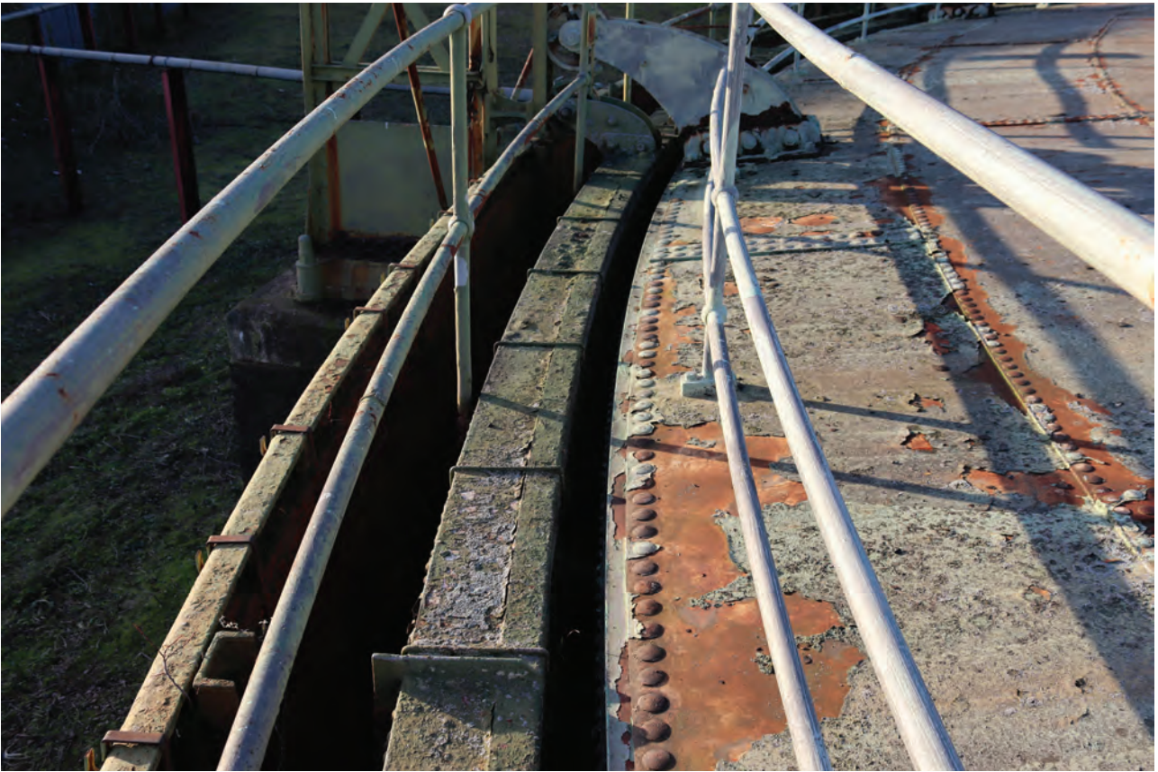
Plate 29: Gasholder No 1, general view of the top of the tank showing lower lift with square grip and top curb of the bell between standards 8 and 9, from the east
