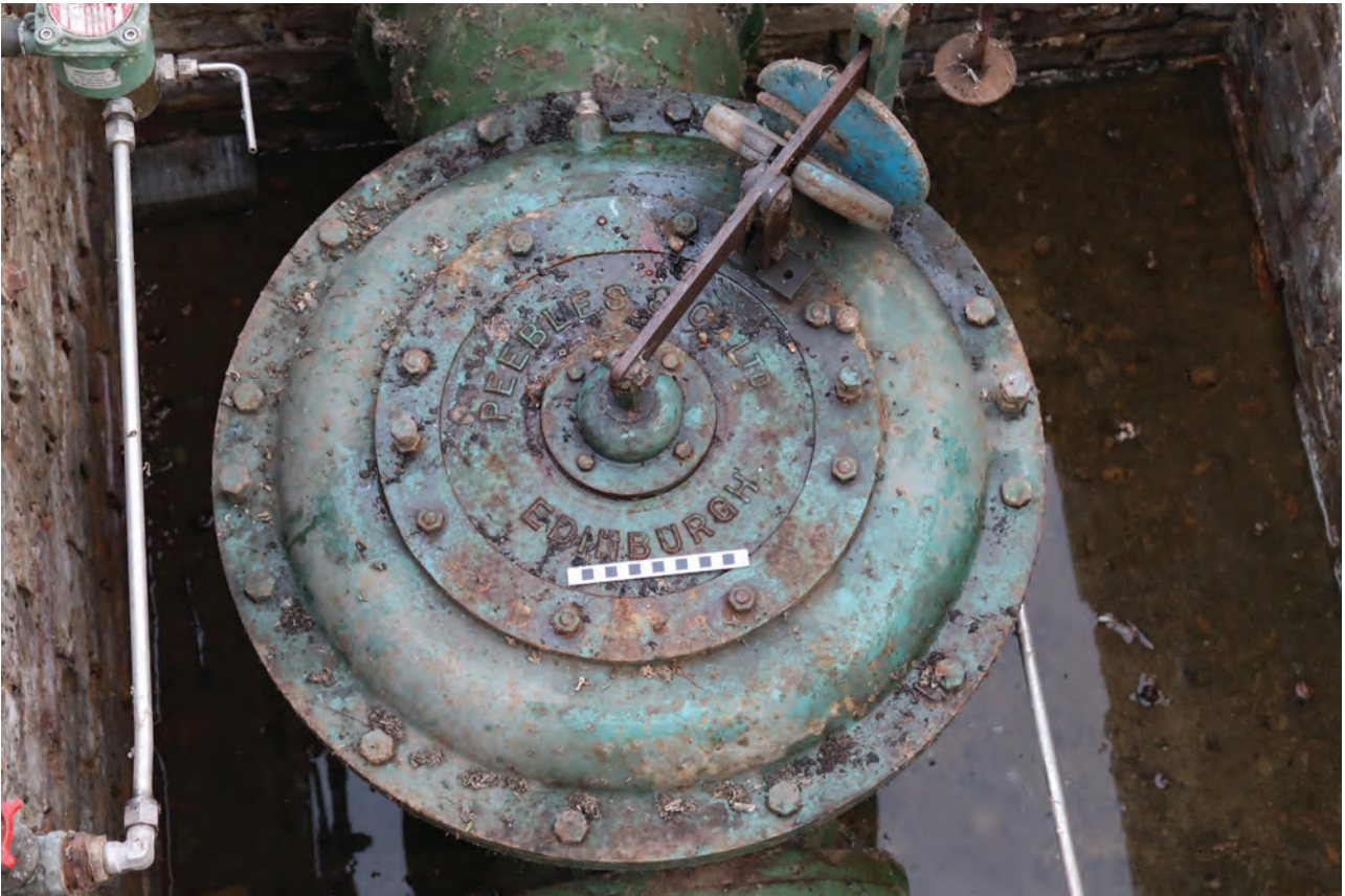
Plate 95: Gasholder No 2, detail view of the weighted diaphragm valve made by Peebles & Co associated with the gas outlet pipe, from the south-west
