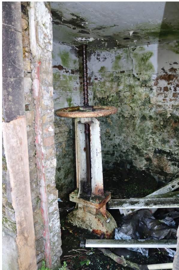
Plate 54: Gasholder No 1, detail view of northernmost inlet/outlet valve control, from the north-west
