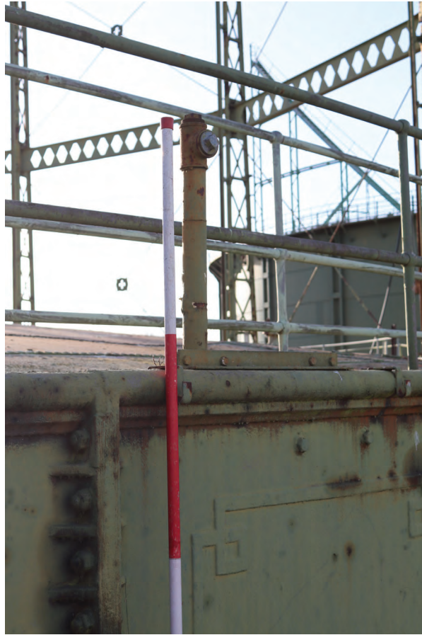
Plate 69: Gasholder No 1, detail view of pipe used for oil, from the north
