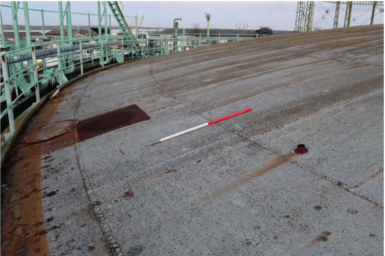
Plate 90: Gasholder No 2, general view of the north-west side of the crown showing removed cotter plate and purge point added during decommissioning works to aerate the bell, from the west
