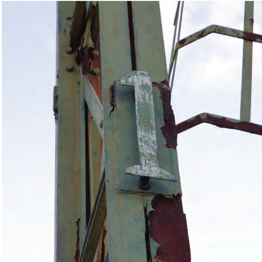
Plate 9: Gasholder No 1, detail view of welded, steel sign on standard 1 identifying the structure as Gasholder No 1, from the NNW
