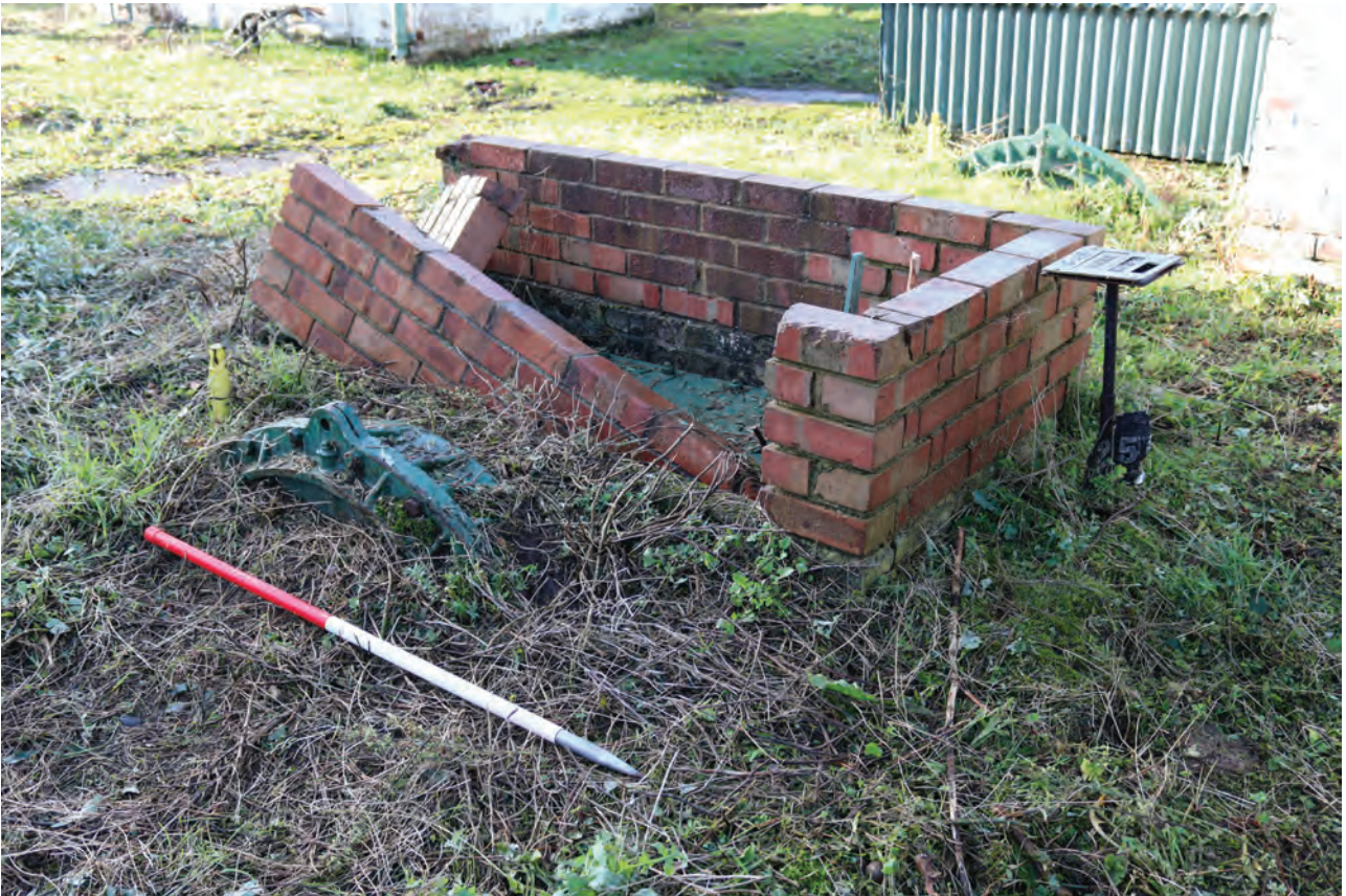
Plate 147: Structure P, general view of valve pit with collapsed brick wall surround, from the north-east
