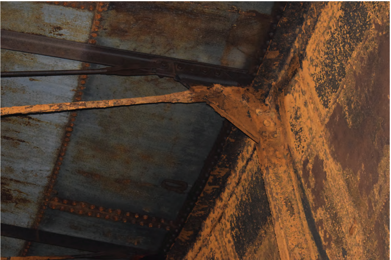
Plate 48: Gasholder No 1, detail view of triangular fixture at the top of the top lift wall interior, from the north
