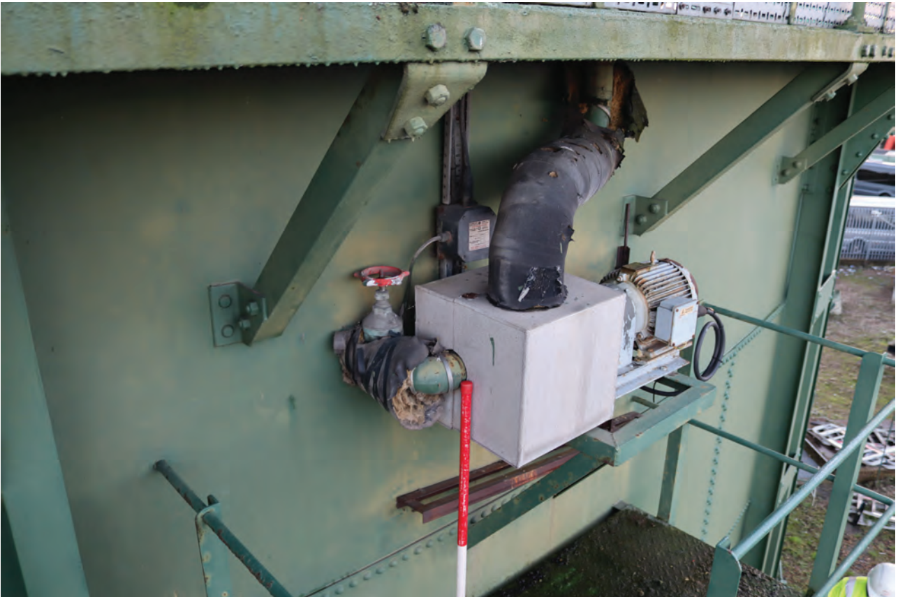
Plate 99: Gasholder No 2, detail view of heating motor, from the north-east
