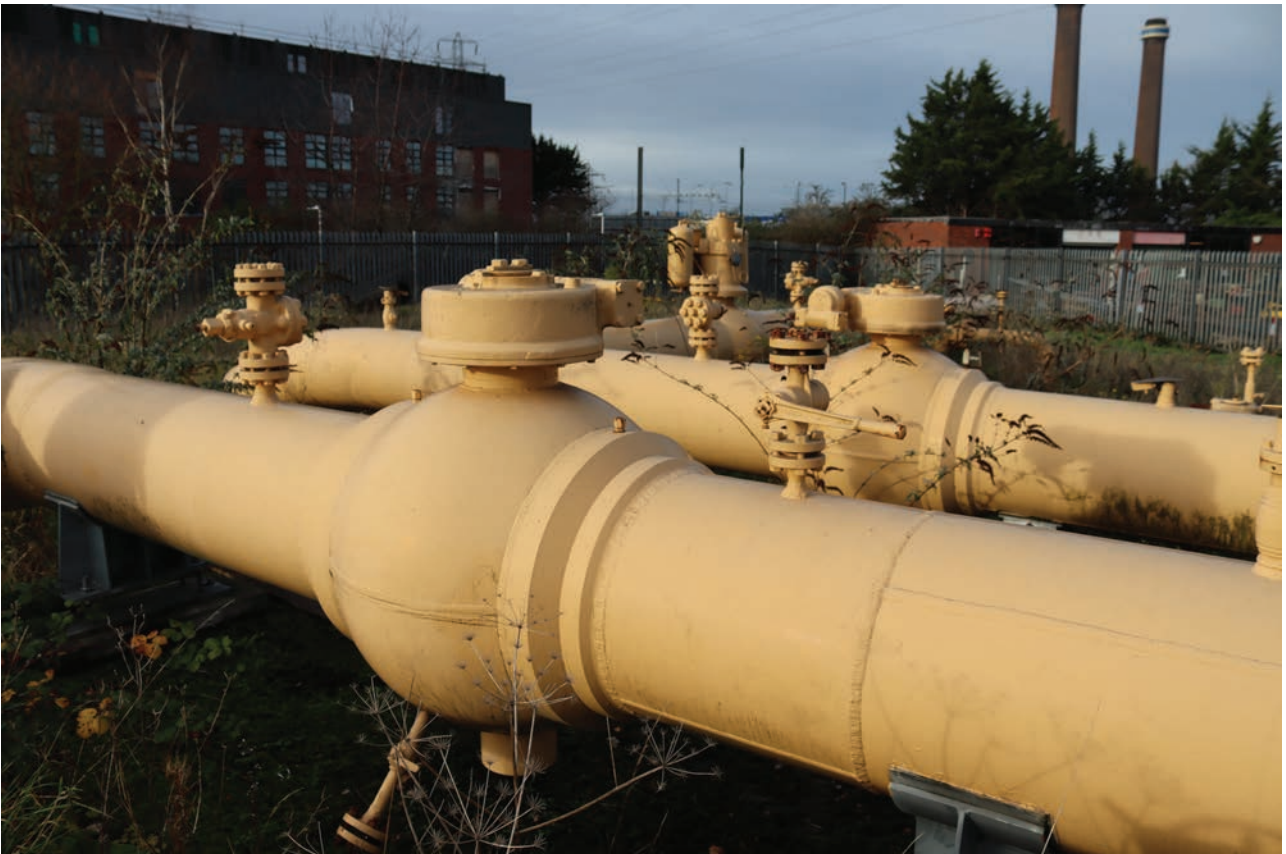
Plate 194: Pipework, detail view of Cameron ball valve, from the north-west
