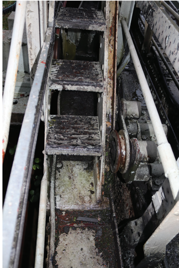
Plate 45: Gasholder No 4, detail view of the tangential rollers gripping the guide rail on the interior of the stair structure, from the SSW
