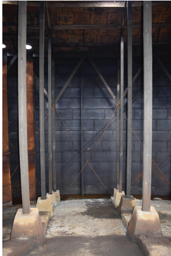
Plate 25: Gasholder No 4, general view of the iron bar and timber plank cross-bracing between vertical posts of ring 7, from the ENE
