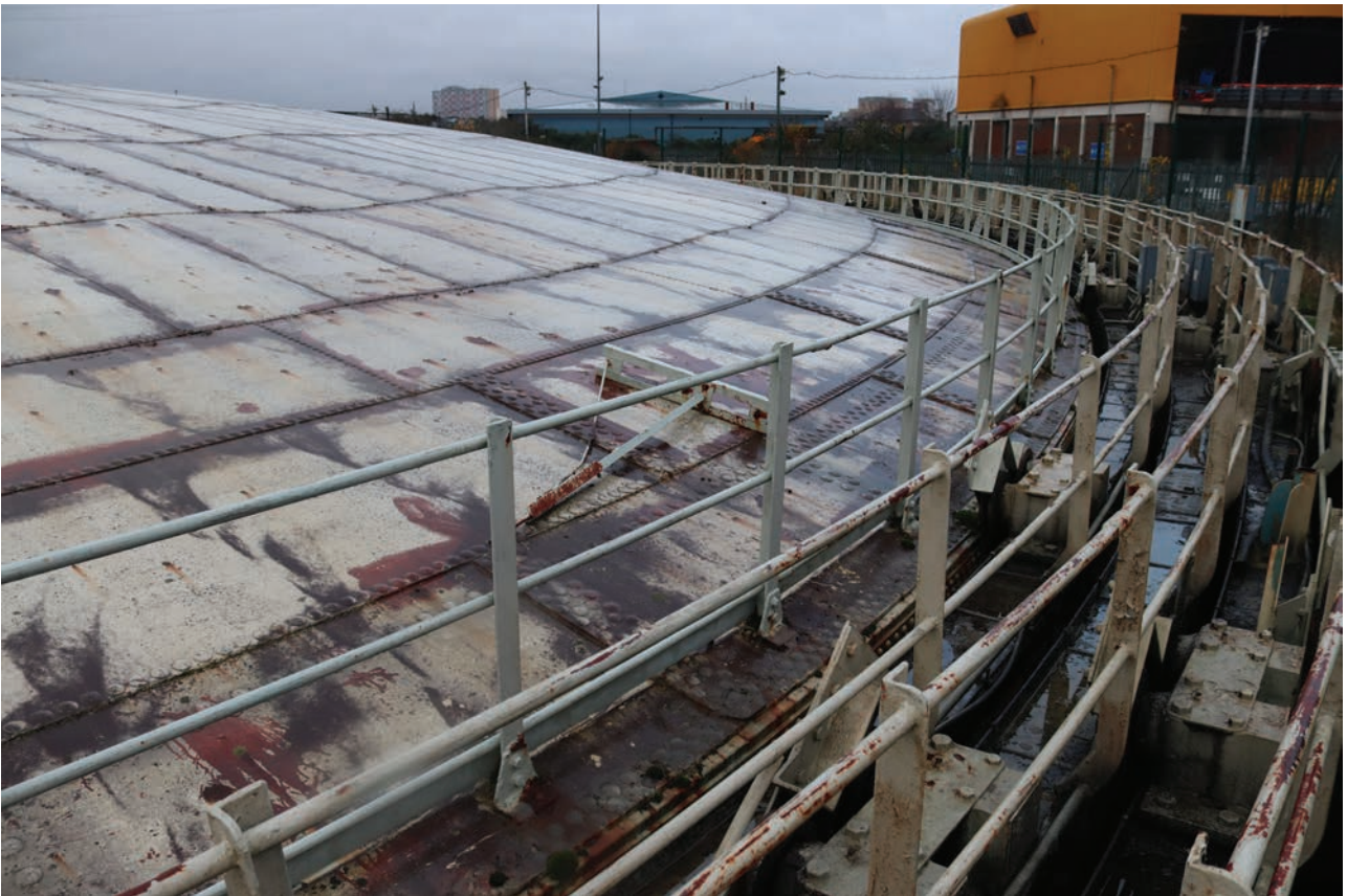
Plate 62: Gasholder No 4, detail view of displaced striker arm on the south-east side of the holder, from the SW
