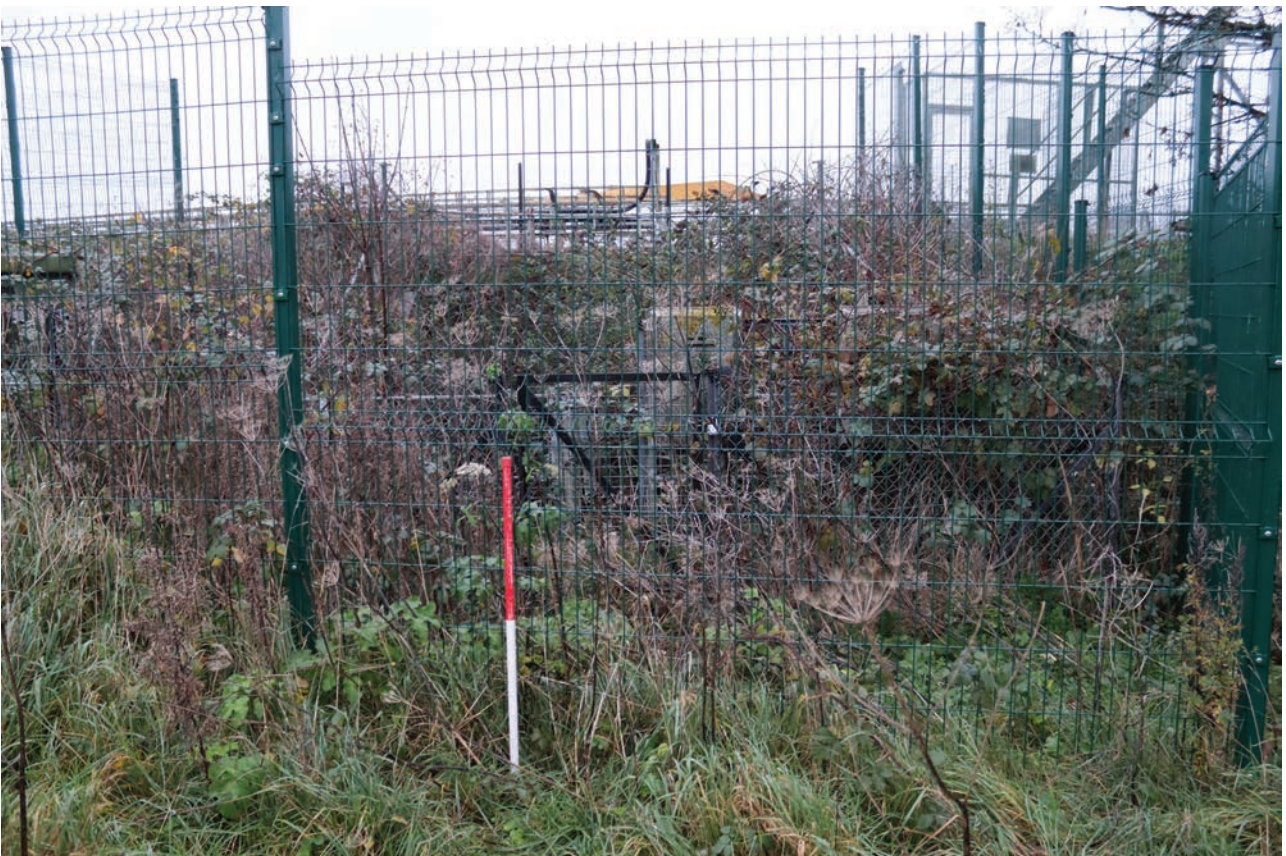
Plate 56: Gasholder No 4, general view of overgrown gas inlet and outlet fenced area, from the west
