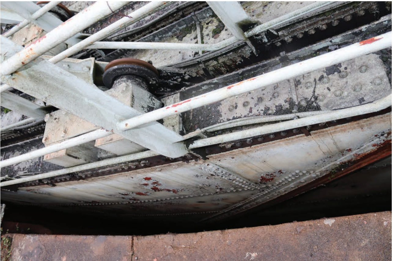
Plate 36: Gasholder No 4, detail view of the outer wall of the bottom lift showing riveted steel sheet construction and helical guide rail, from the NNW
