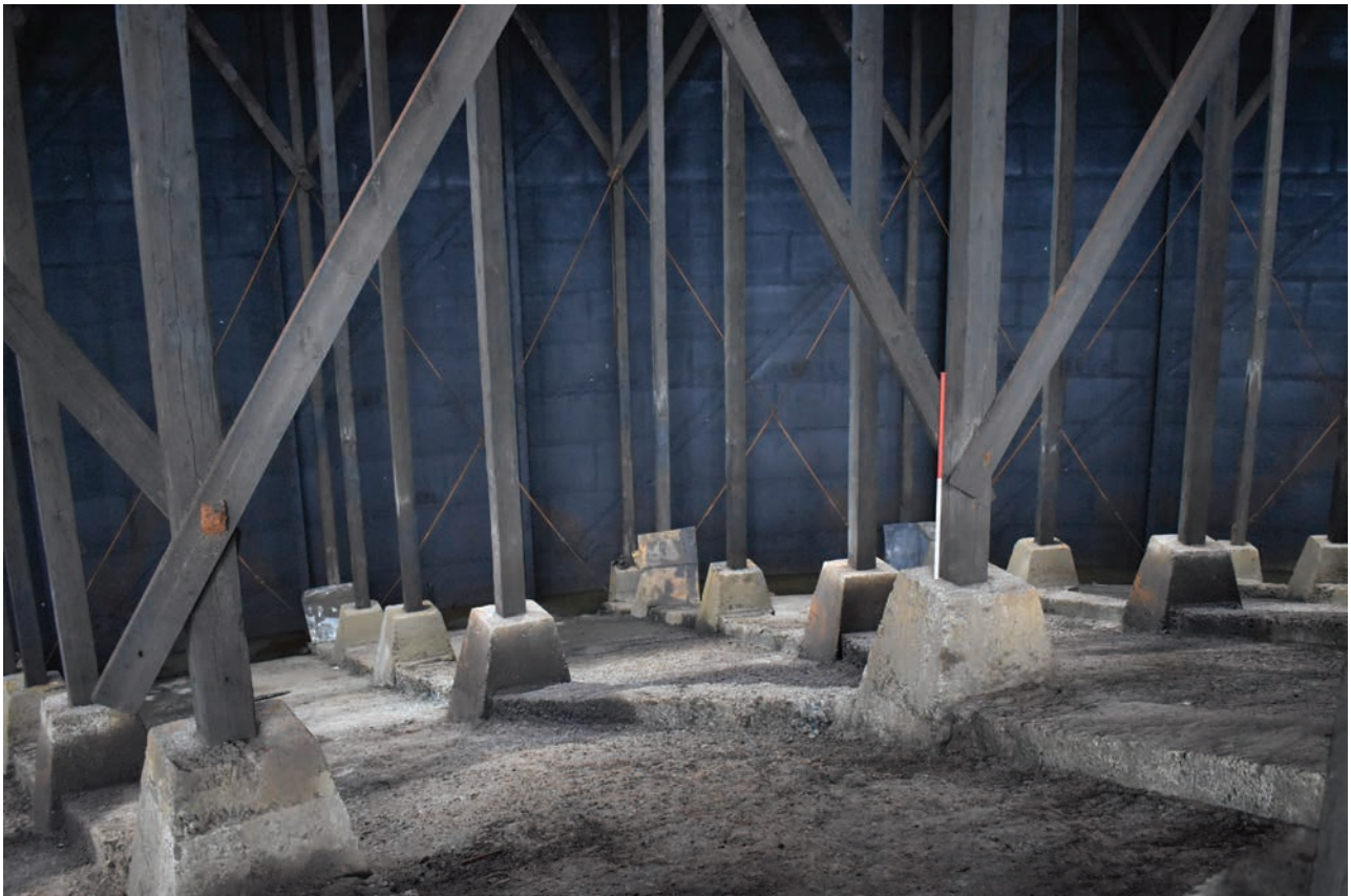
Plate 28: Gasholder No 4, general view of the lines of concrete connecting the concrete block bases of the vertical posts of rings 2–7, from the NNW
