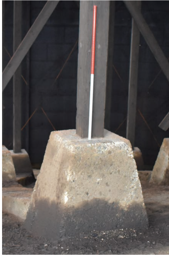
Plate 27: Gasholder No 4, detail view of concrete block base of ring 2, from the WNW
