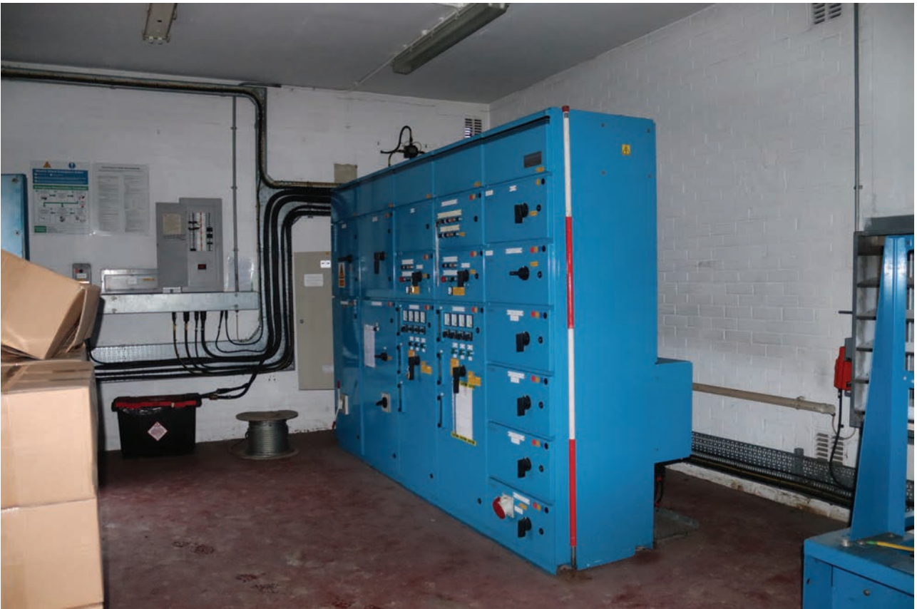
Plate 176: Structure 4, general view of the instrumentation panels within the Switch Room, from the SSE
