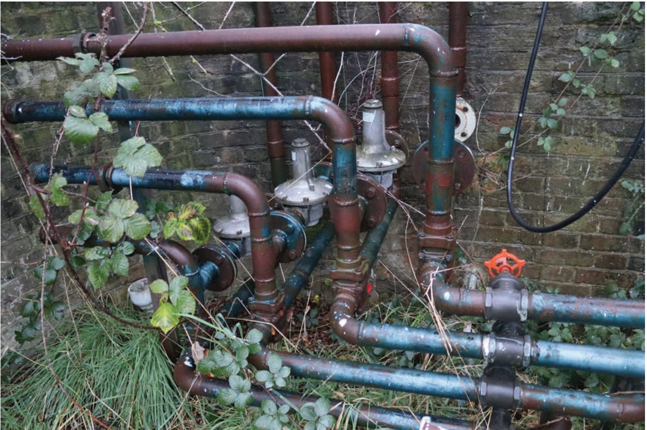
Plate 135: Gasholder No 5, detail view of pipework with small diaphragms, from the SSE
