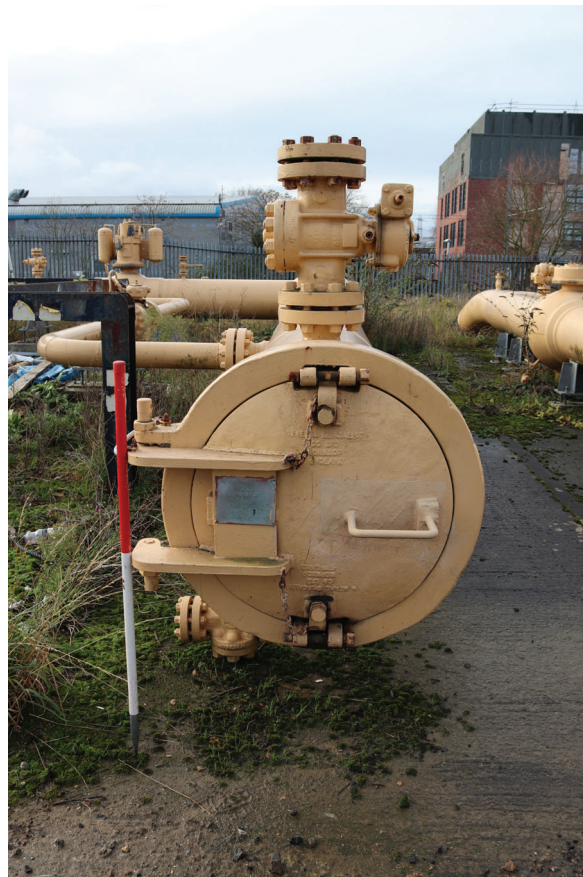
Plate 192: Pipework, detail view of entrance for intelligent pig, from the ENE
