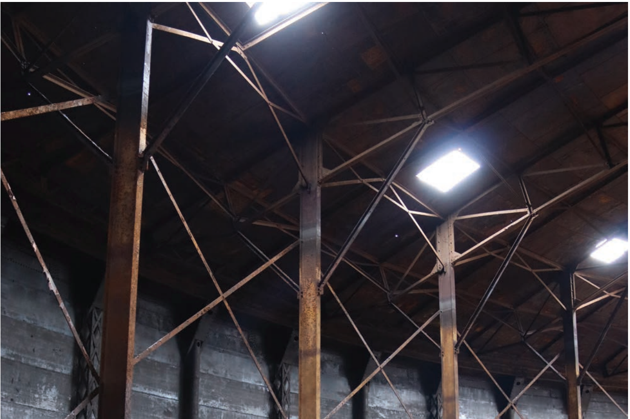
Plate 92: Gasholder No 5, detail view of the trussed ring at the outer edge of the crown rest frame, from the south-west
