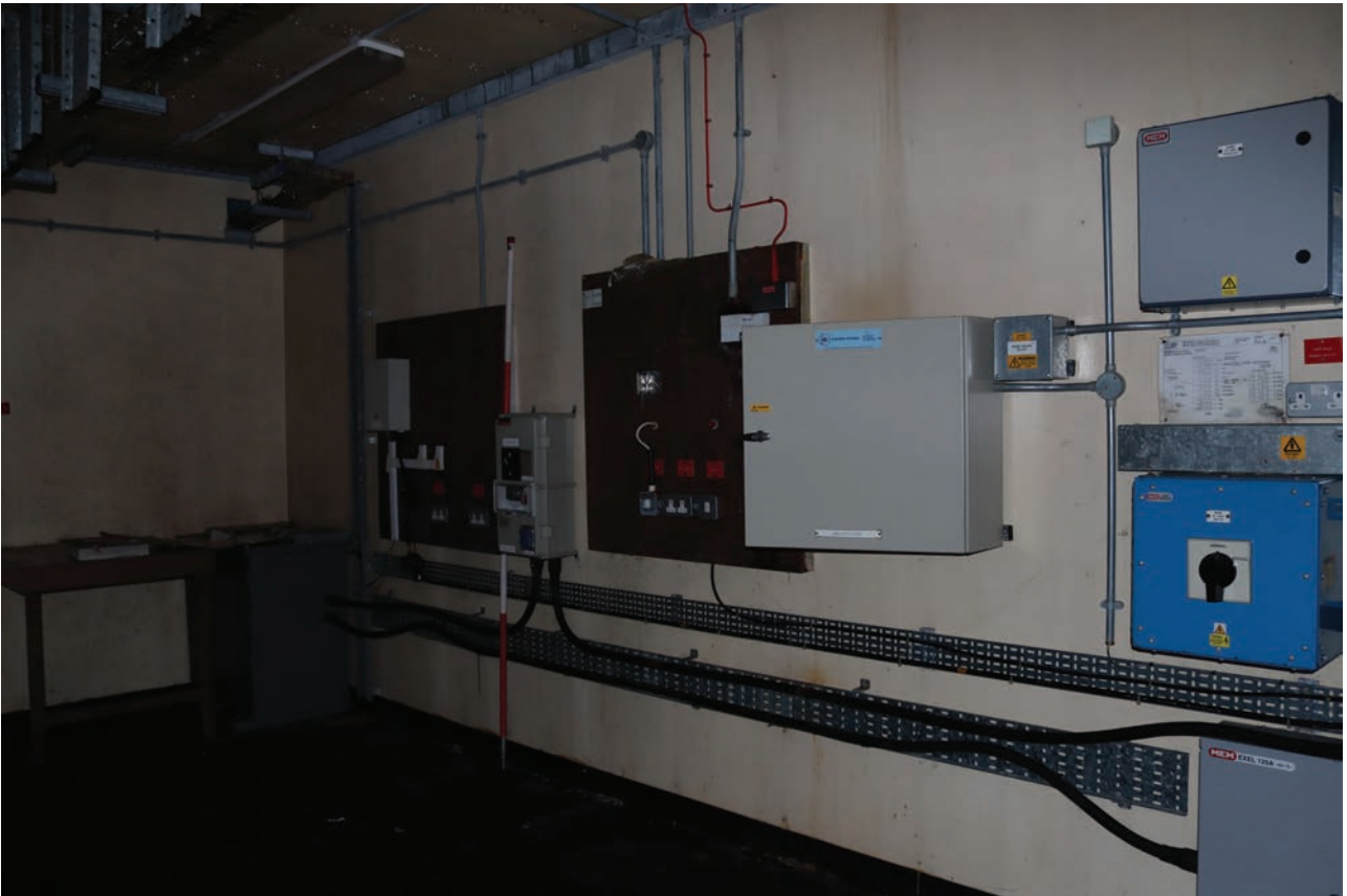
Plate 183: Structure 8, general view of Electrical Building interior showing electrical control panels, from the WNW
