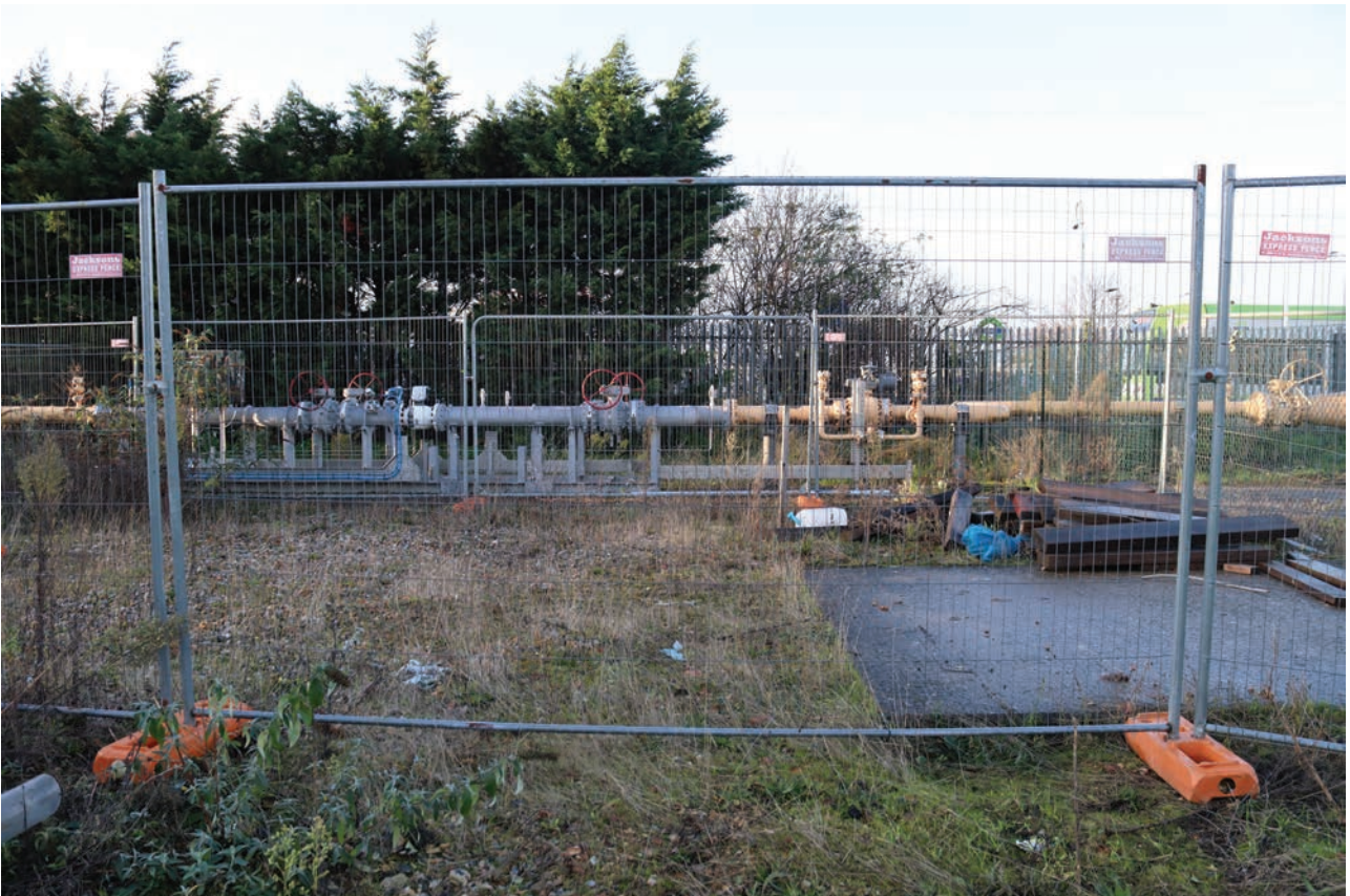
Plate 198: Pipework, general view of above ground pipework on the south-west boundary of the site, from the north-east
