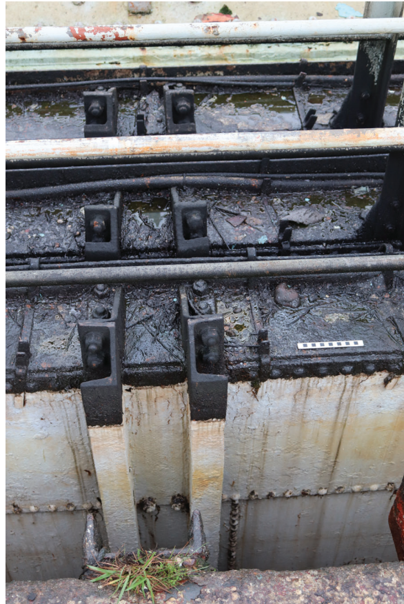
Plate 113: Gasholder No 5, detail view of stanchions bolted to the lift tops to give rigidity to the lifts, from the south-east
