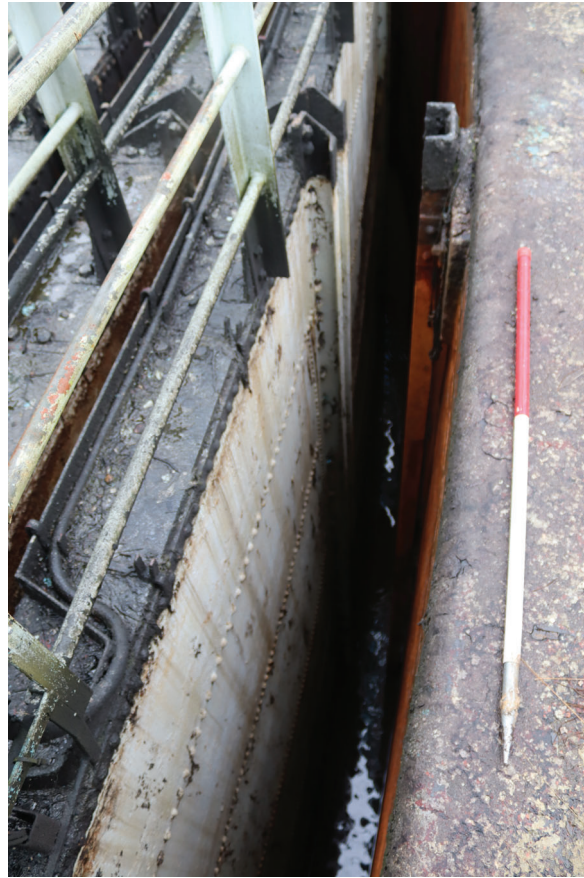
Plate 111: Gasholder No 5, detail view of the external wall of the bottom lift constructed of riveted steel sheets, from the east
