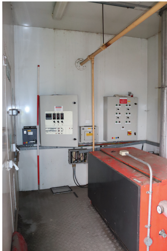
Plate 166: Structure 2, detail view of the heat monitoring panels within the Boiler House, from the south-east
