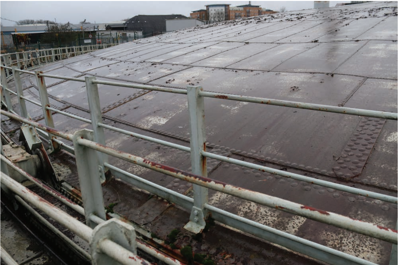
Plate 49: Gasholder No 4, detail view of the crown showing riveted, steel sheets with larger rivets and additional plates covering joints at the top curb, from the north
