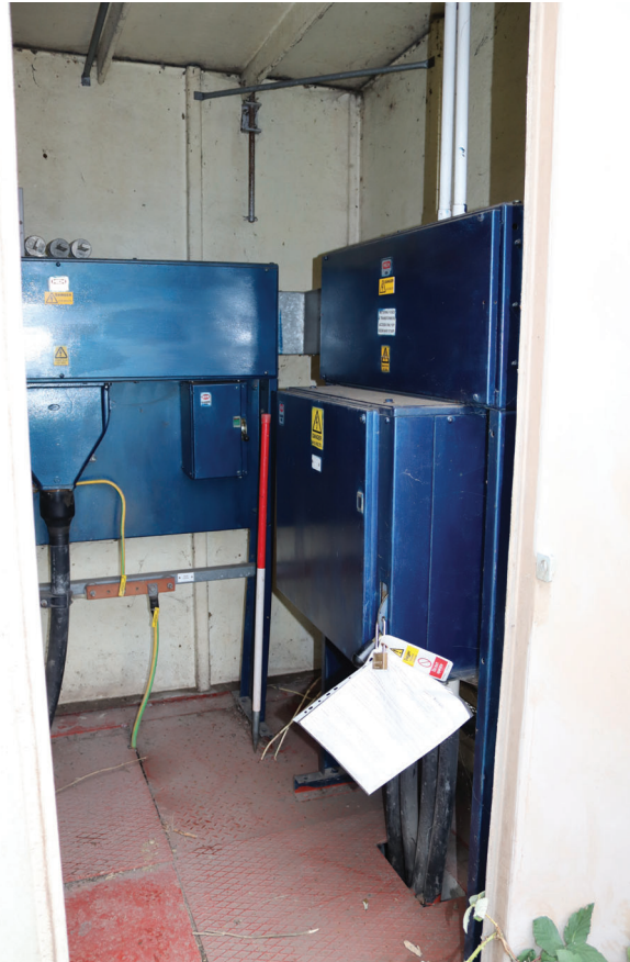
Plate 179: Structure 5, general view of the interior of the Electrical Room, from the ESE
