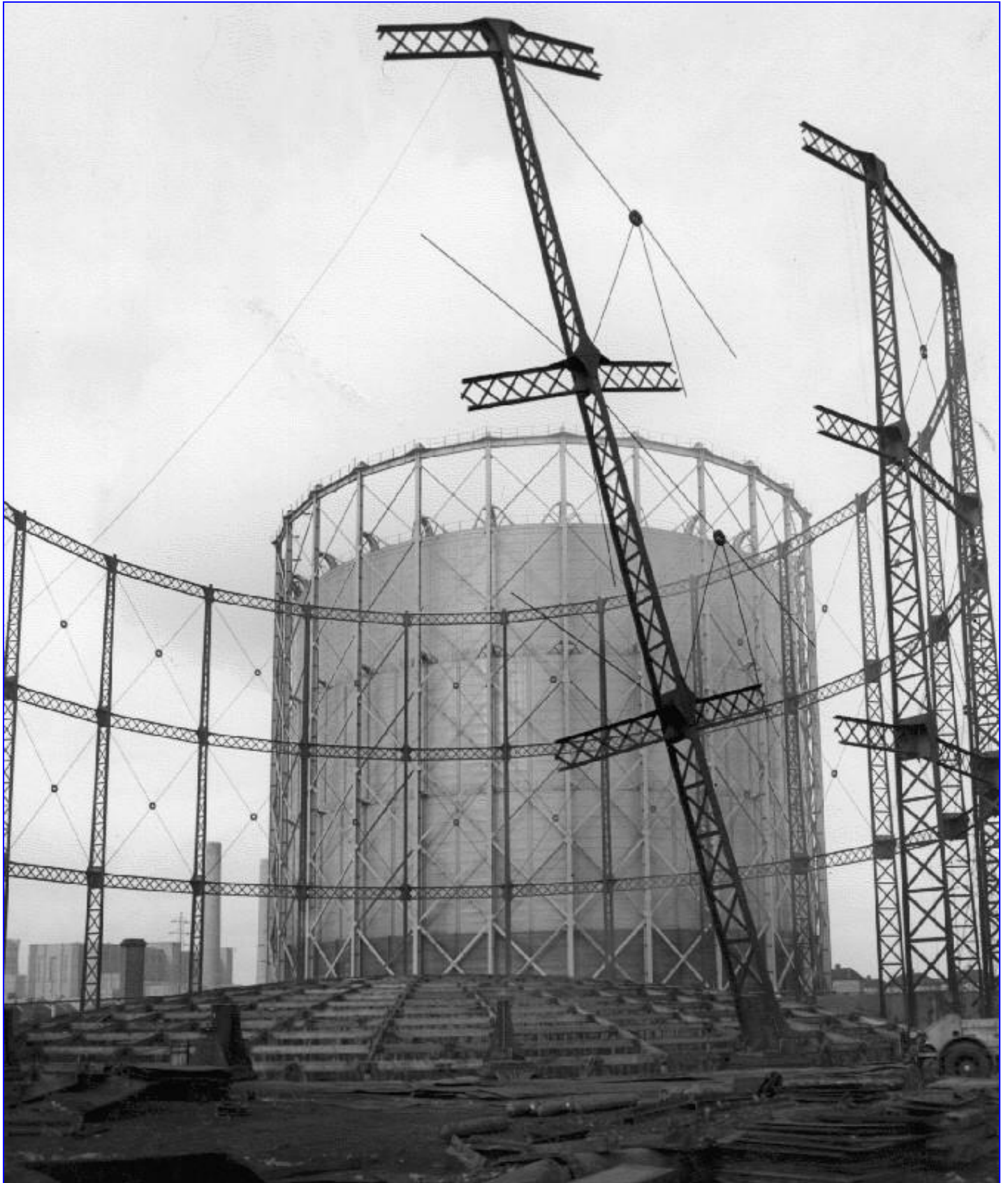
Figure 23: Archive photograph showing the dismantling of the 1890s guide frame of Gasholder No 4, ca. 1954 (NGA Ref: SE/SEG/ES/CRG/E/F/3); Gasholder No 5 is in the background
