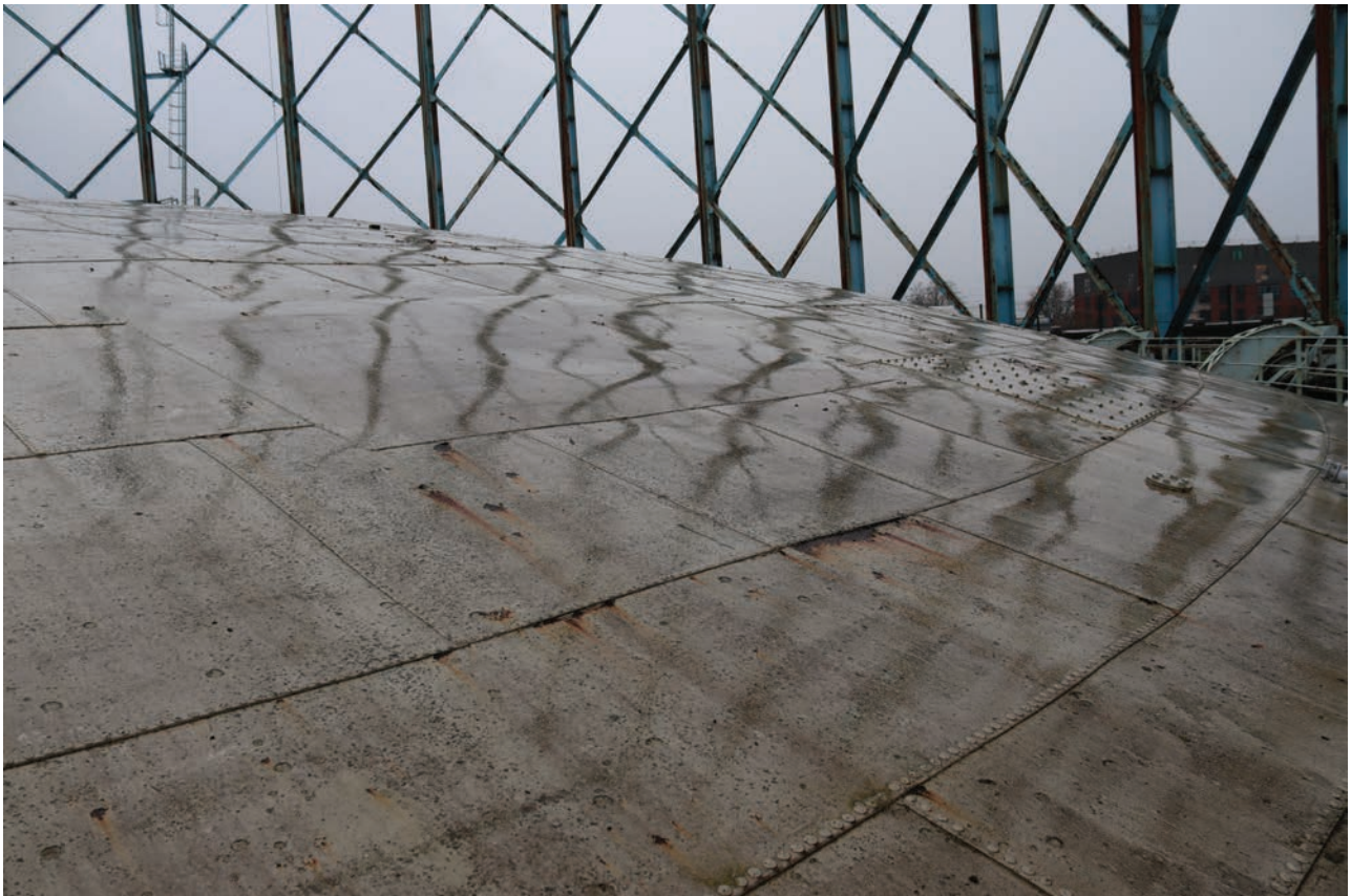
Plate 132: Gasholder No 5, detail view of different sheet repairs, from the east
