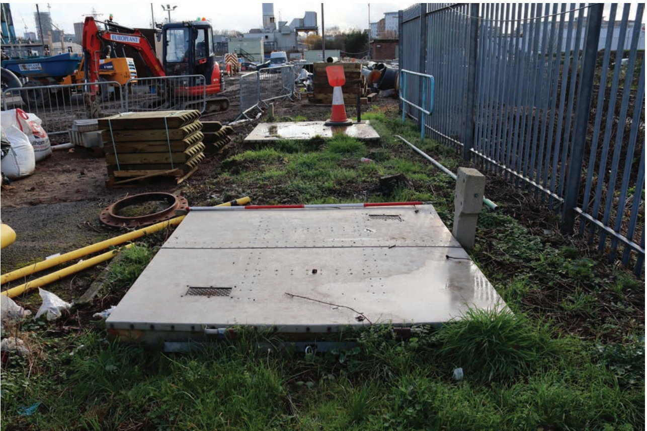
Plate 210: Valve pits, detail view of steel rain covers, from the north-west
