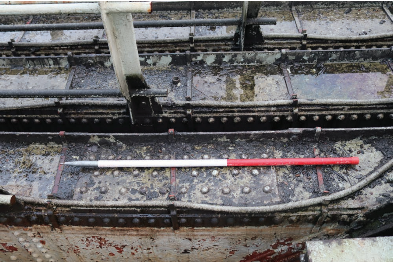
Plate 48: Gasholder No 4, detail view of the lift tops showing riveted plates, rubber tubing clipped into place and decommissioning vent points, from the south-west
