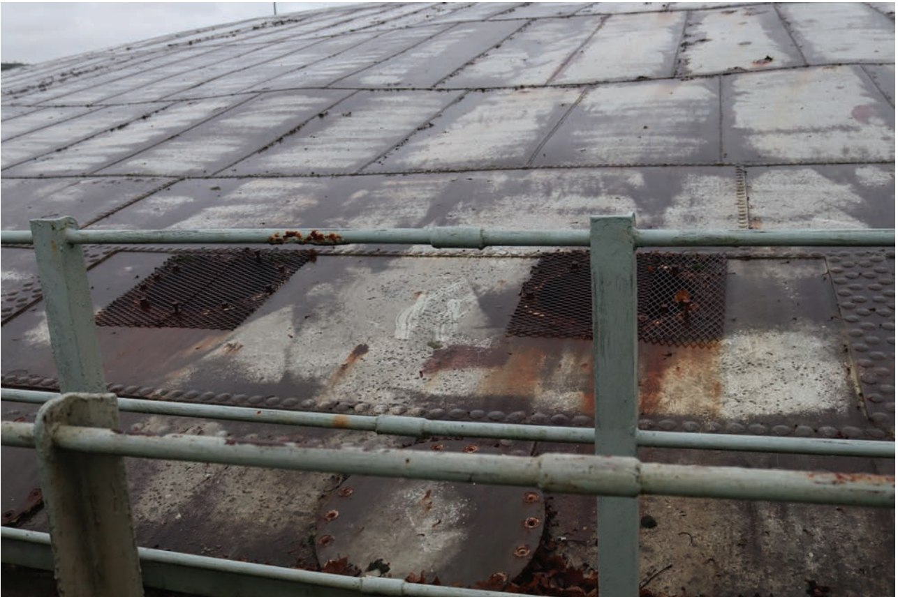
Plate 55: Gasholder No 4, detail view of the two removed cotter plates presumed to be inspection points for the gas inlet and outlet pipes, from the WSW
