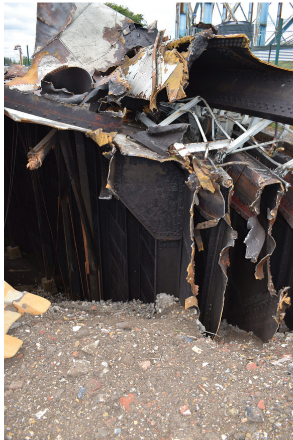
Plate 40: Gasholder No 4, detail view of bracket topping stanchion on the crown lift wall interior, from the east
