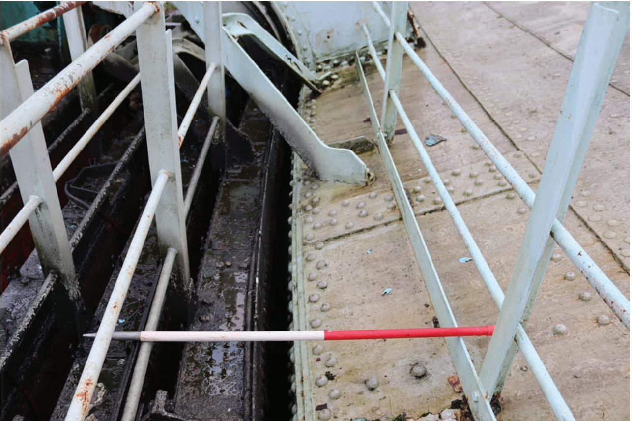
Plate 125: Gasholder No 5, detail view of larger rivets and additional sheeting over joints at the curb, from the NNW
