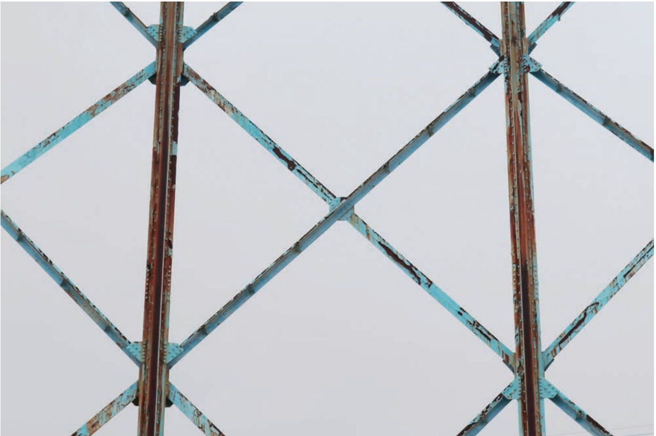
Plate 103: Gasholder No 5, detail view of diagonal struts attached to the interior side of standards 6 and 7 via gusset plates, from the ENE
