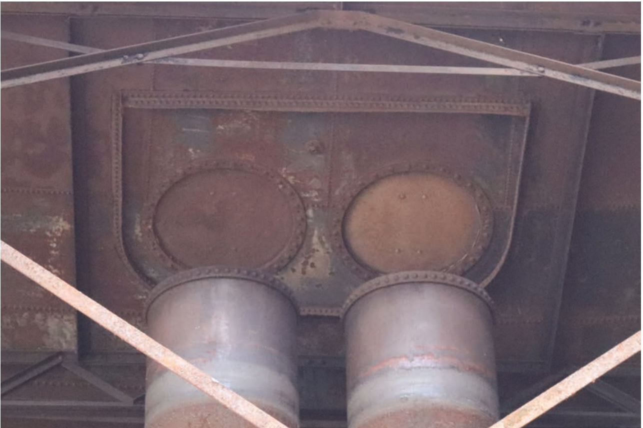
Plate 137: Gasholder No 5, detail view of inspection cotter plates and D-shaped surrounding support above the gas inlet and outlet pipes, from the north
