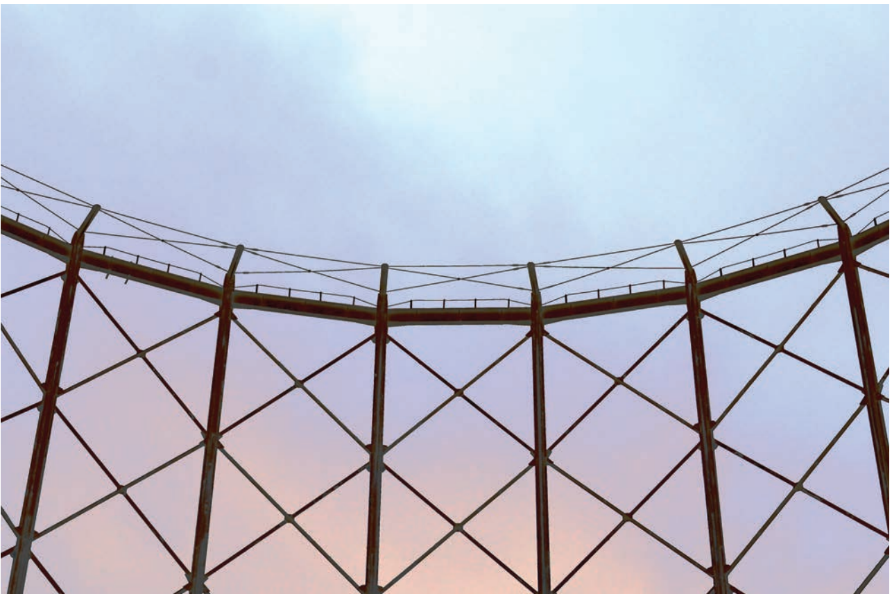
Plate 106: Gasholder No 5, detail view of cross tie bars to steady the top of the frame in high wind, from the north
