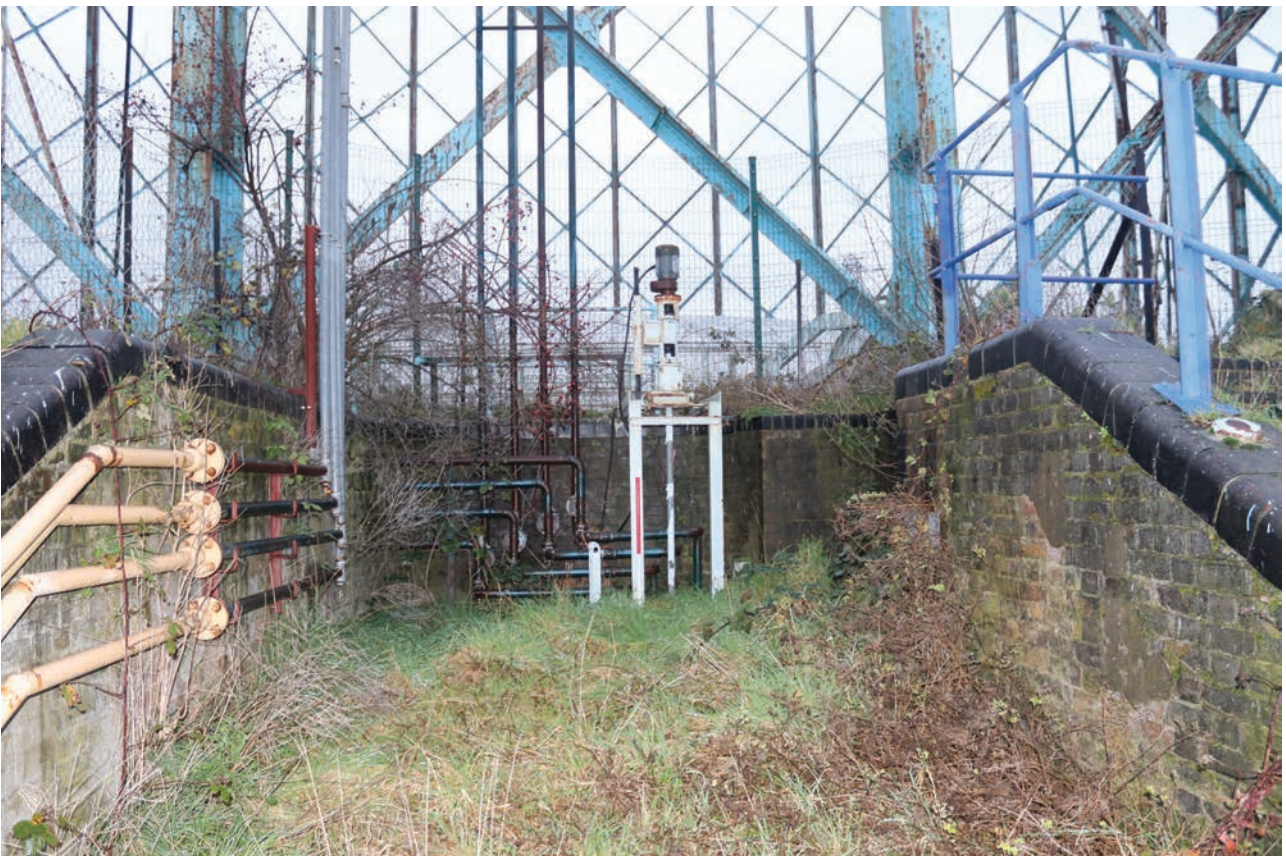
Plate 134: Gasholder No 5, detail view of horseshoe-shaped brick-walled area of pipework to the south of the holder, from the south
