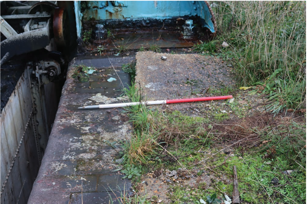
Plate 79: Gasholder No 5, detail view of blue brick tank wall cap and surrounding damaged hardcore, from the SSE
