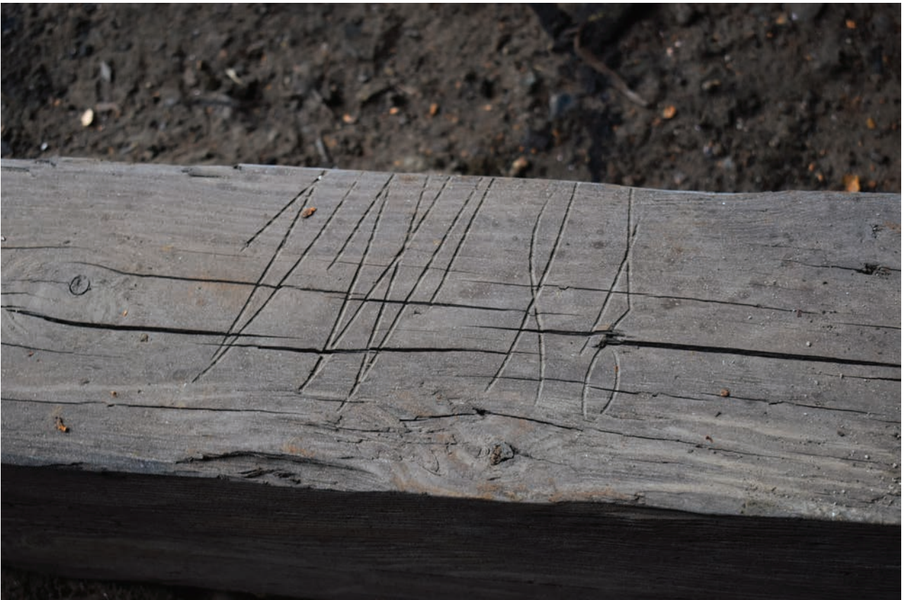
Plate 34: Gasholder No 4, detail view of possible initials and date carved into a displaced timber of the crown rest frame, not in situ
