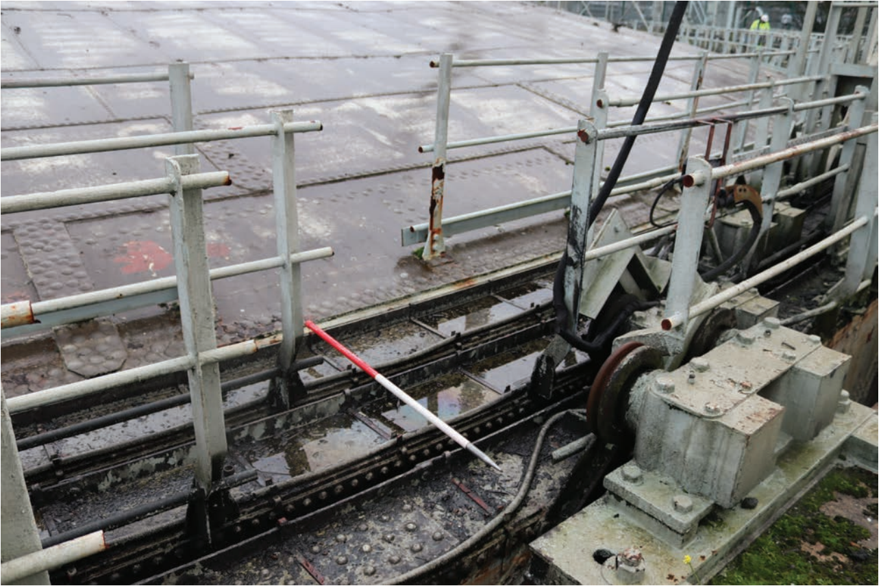
Plate 47: Gasholder No 4, detail view of handrails cut during decommissioning works for clear access onto the crown, from the north-west
