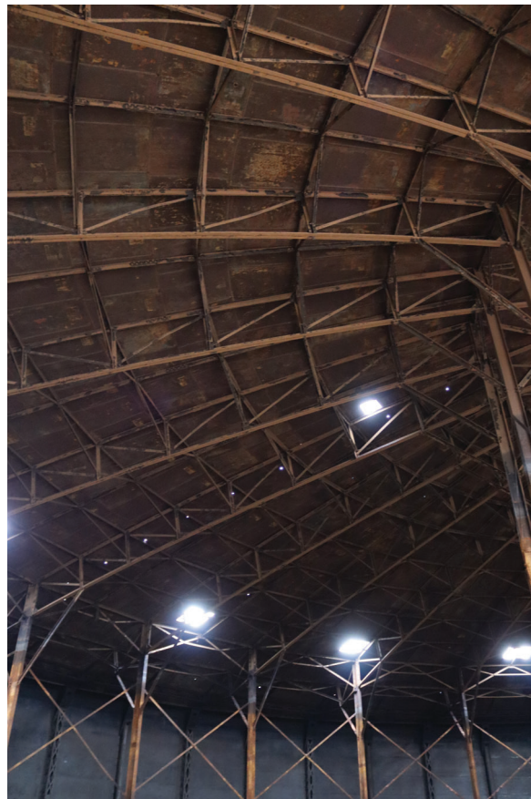
Plate 90: Gasholder No 5, general view of trussed beams supporting the dome crown rest frame, from the south-east
