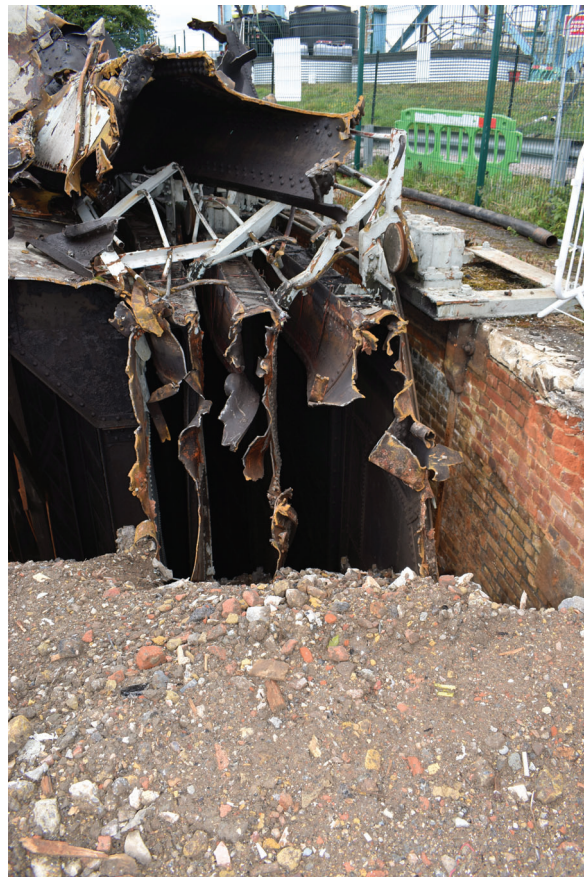
Plate 42: Gasholder No 4, detail view of square grips in section during demolition, from the east
