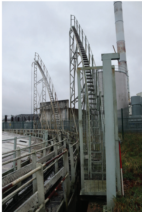
Plate 46: Gasholder No 4, detail view of the padlocked grated gate at the base of the outermost guide rail and stair structure with gap in the handrail of the bottom lift allowing access onto the bottom lift, from the NNW
