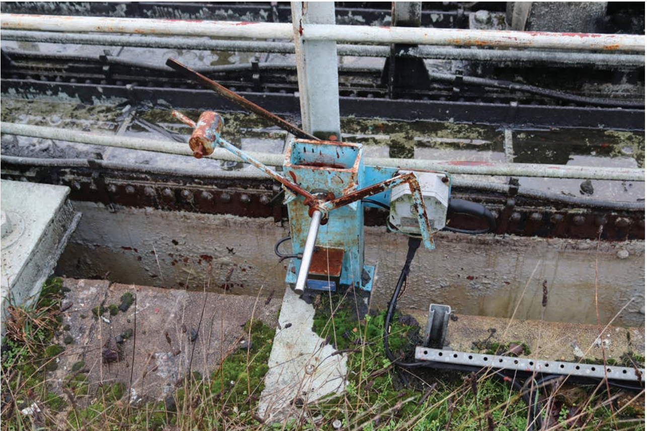
Plate 59: Gasholder No 4, detail view of high knock-off switch located on the south-east side of the holder, from the SSE
