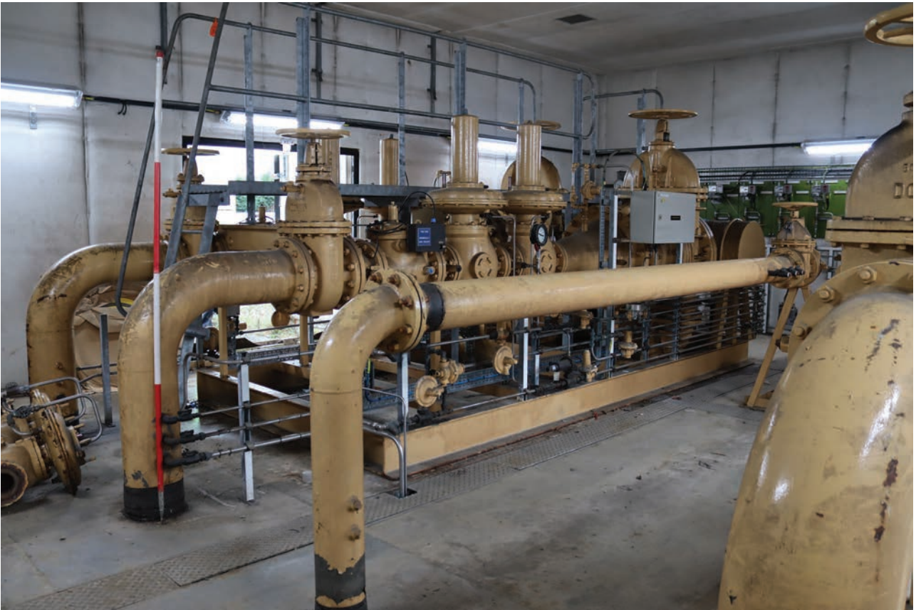
Plate 159: Structure 1, general view of equipment within the District Governor House, from the NNE
