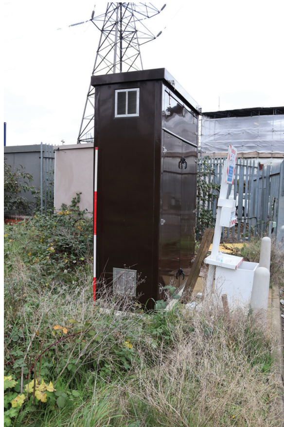
Plate 180: Structure 6, general view of the exterior of the Electrical Room, from the south
