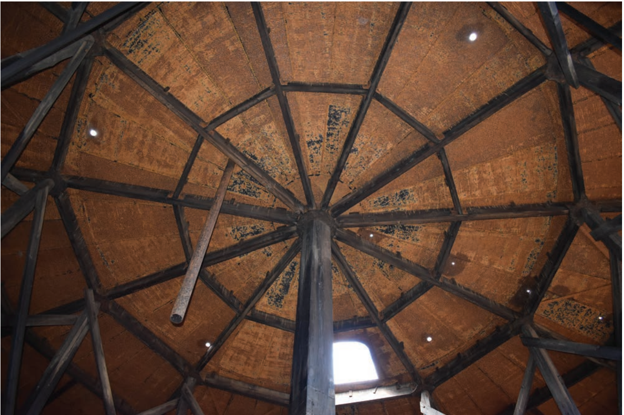
Plate 53: Gasholder No 4, detail view of the pipe beneath the crown vent just south-east of the centre of the crown, from the NNE
