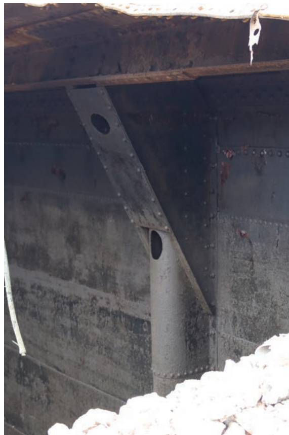
Plate 116: Gasholder No 5, detail view of the triangular-shaped bracket supporting the top curb of the bell, from the south
