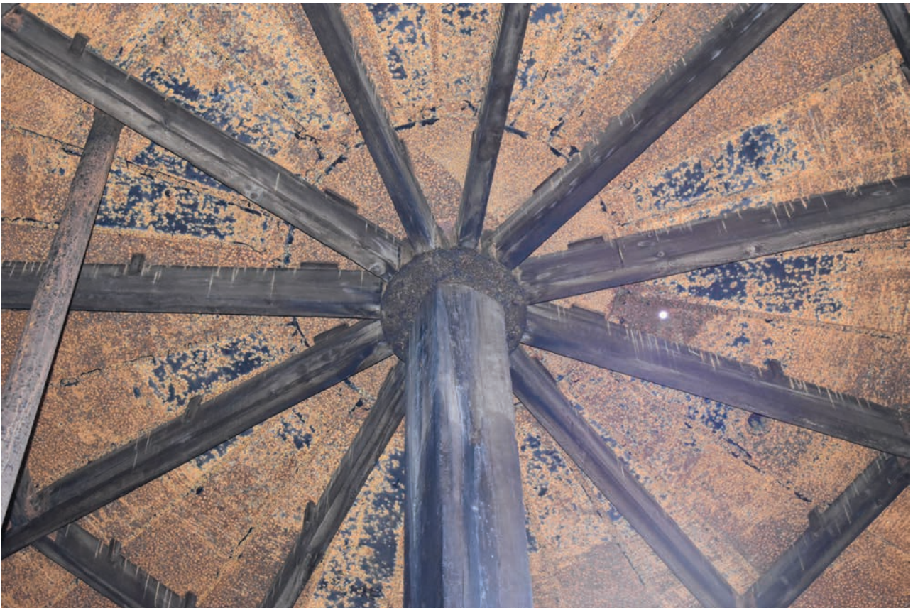
Plate 30: Gasholder No 4, detail view of central vertical post, cylindrical fixture and eleven timber spokes of the crown support frame, from the NNE
