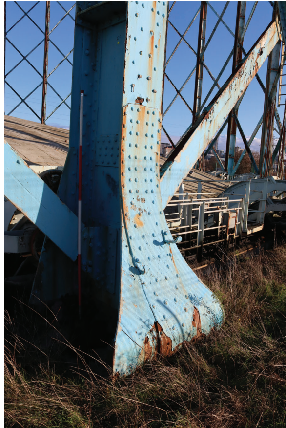
Plate 99: Gasholder No 5, detail view of the riveted rectangular plate on the exterior side of standard 5, from the NW
