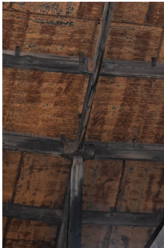
Plate 32: Gasholder No 4, detail view of timber chocks supporting the crown, from the WNW
