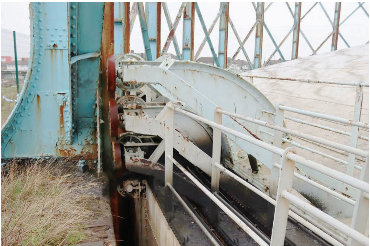
Plate 108: Gasholder No 5, detail view of the four guide rollers and carriages attached to the lifts at each standard, from the east
