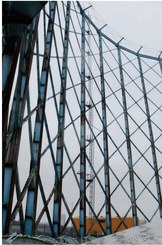
Plate 107: Gasholder No 5, detail view of set of ladders situated between standards 18 and 19, from the WNW
