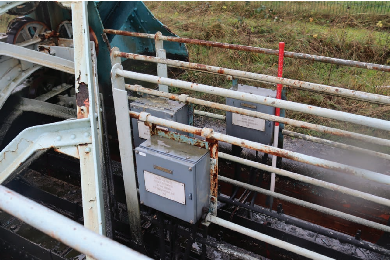
Plate 145: Gasholder No 5, detail view of electrical boxes related to automated systems situated between standards 9 and 10, from the east
