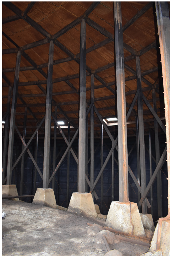
Plate 22: Gasholder No 4, general view of the crown support frame, from the WNW
