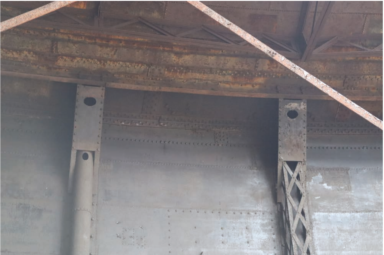
Plate 117: Gasholder No 5, detail view of the steel sheet riveted to the crown and triangular brackets adding rigidity to the top curb, from the south-west
