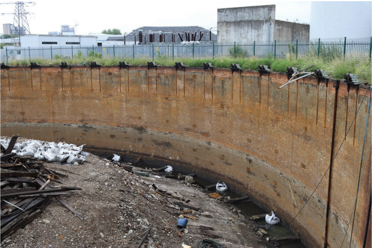
Plate 18: Gasholder No 4, general view of the tank during demolition, from the north-west
