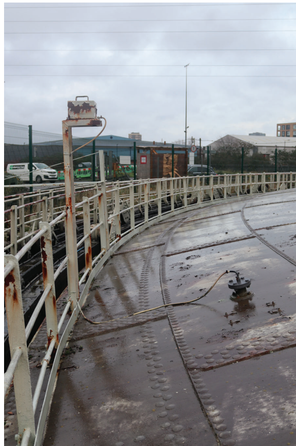
Plate 54: Gasholder No 4, detail view of the glycol pot on the north-west side of the holder and the rubber hose entering the bell, from the south-west
