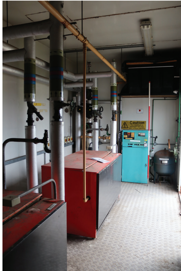
Plate 165: Structure 2, general view of the equipment within the Boiler House, from the north-west
