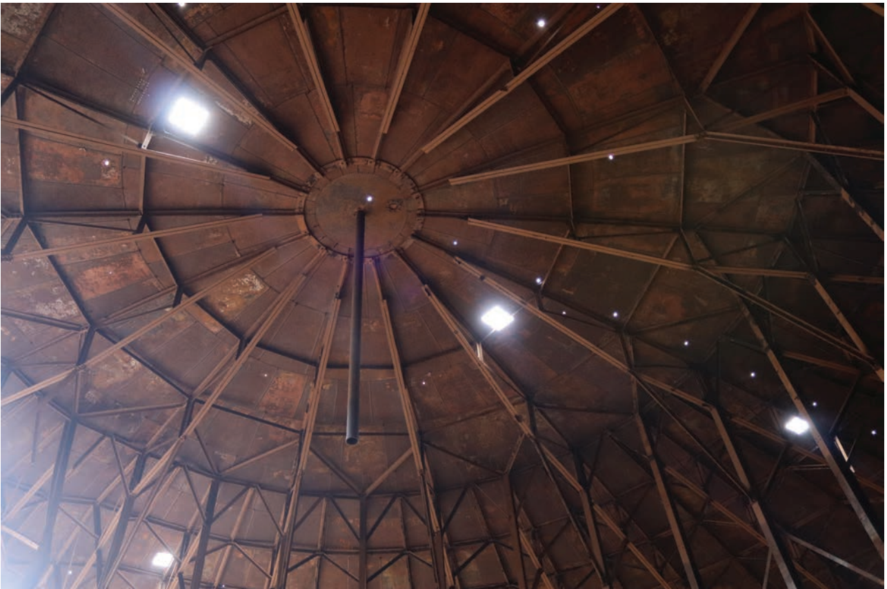
Plate 128: Gasholder No 5, detail view of pipe within the bell connected to the central crown vent on the exterior, from the north
