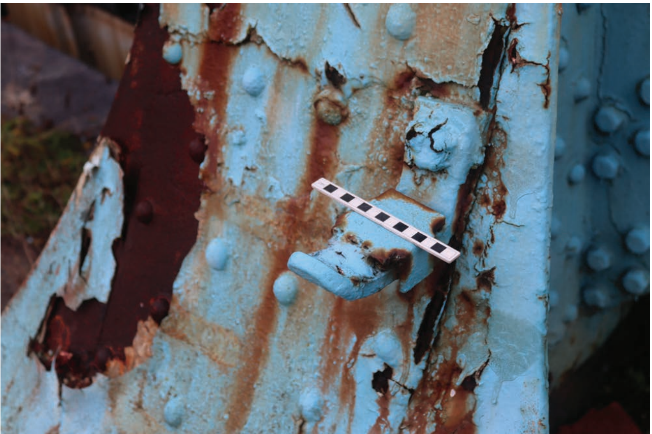
Plate 152: Gasholder No 5, detail view of disused hook on the exterior of many of the standards, from the ESE
