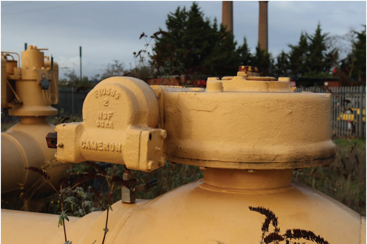
Plate 195: Pipework, detail view of Cameron maker's mark on the ball valve, from the south-east
