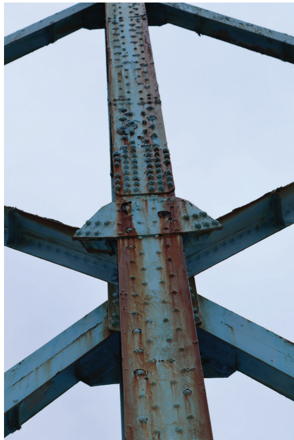
Plate 100: Gasholder No 5, detail view of bolted flange plate and riveted gusset plate on the exterior side of standard 12, from the NNW
