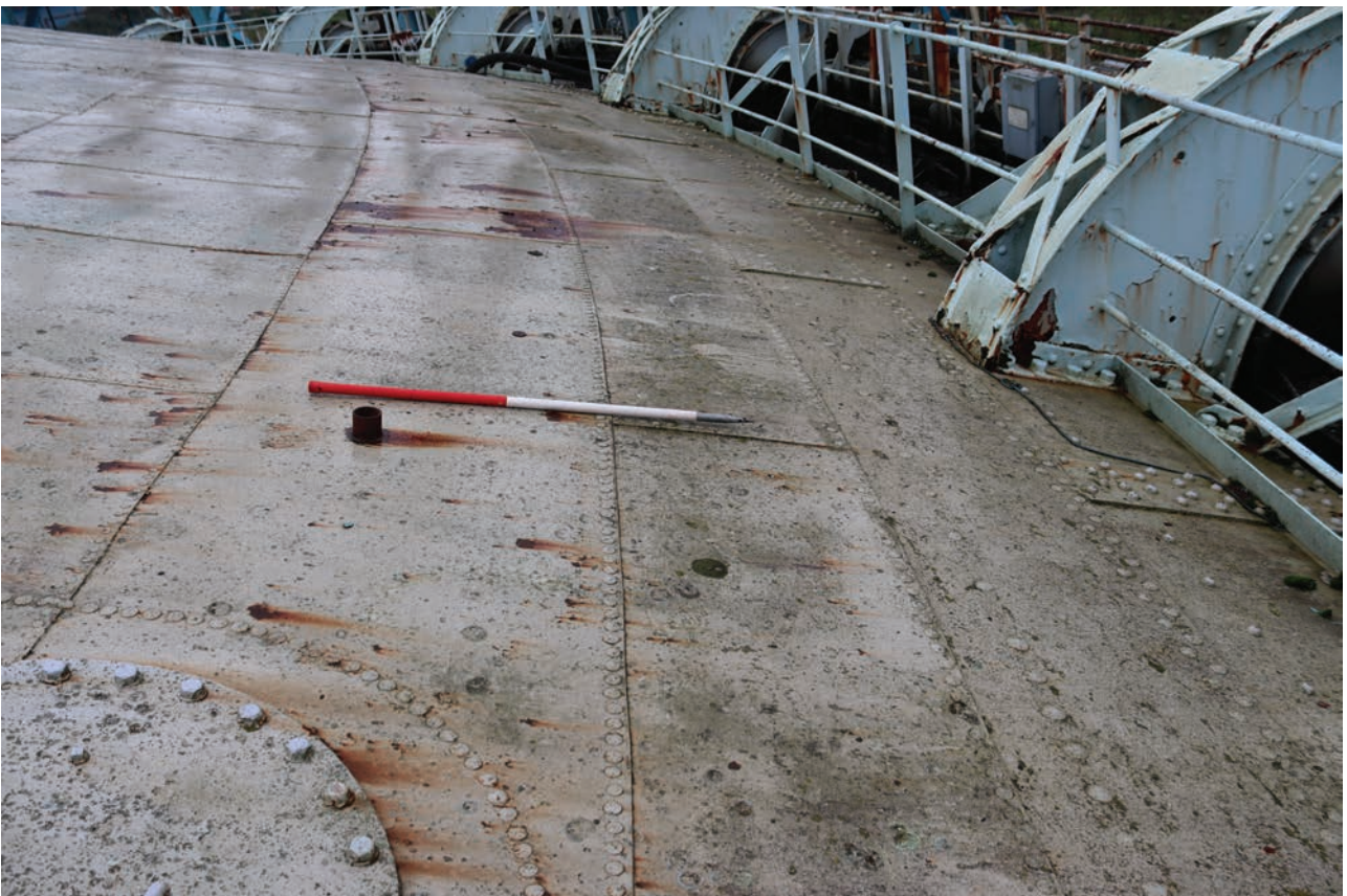
Plate 124: Gasholder No 5, detail view of rectangular riveted sheets of the crown, from the west
