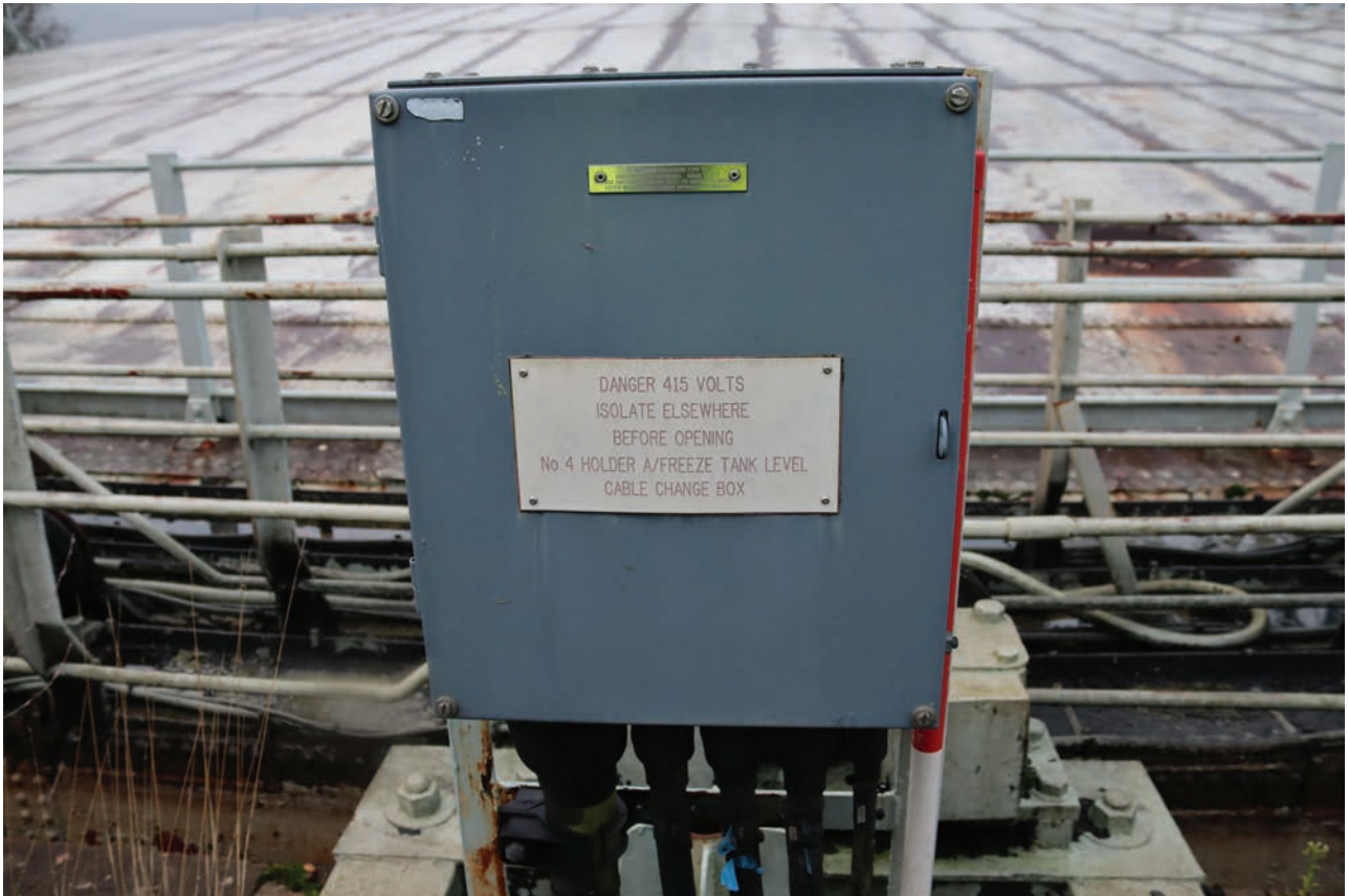
Plate 65: Gasholder No 4, detail view of the anti-freeze tank level cable change box, from the south-east
