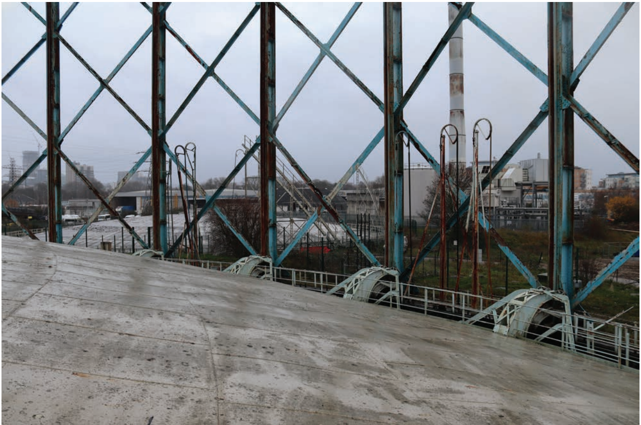
Plate 144: Gasholder No 5, general view of swan neck fixtures between standards 1 and 2, and 27 and 28, from the NNW
