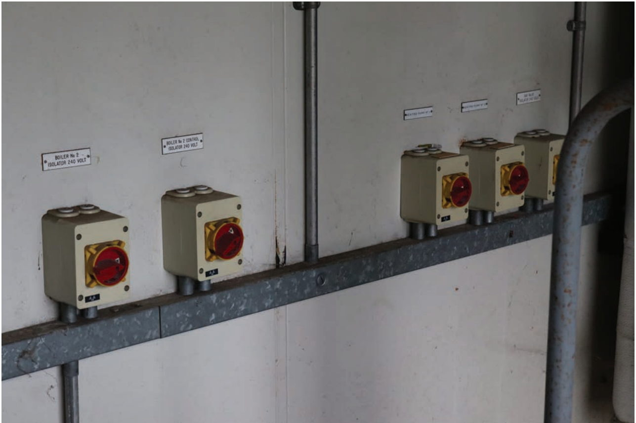
Plate 167: Structure 2, detail view of switches controlling heat pumps within the Boiler House, from the west
