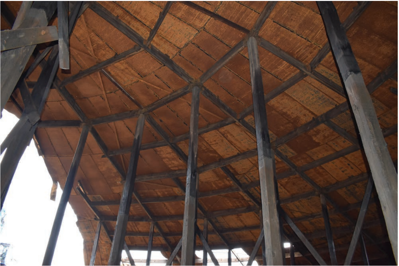
Plate 31: Gasholder No 4, detail view of additional spoke and iron cross-bracing in the timber dome of the crown support frame, from the south-west
