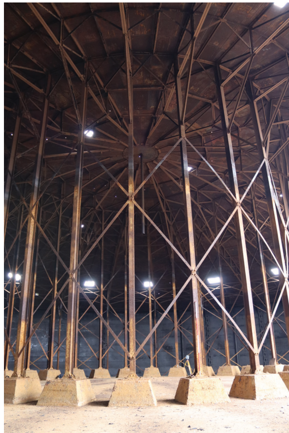
Plate 84: Gasholder No 5, general view of crown rest frame inner ring of steel supports with bracing latticework, from the SSE
