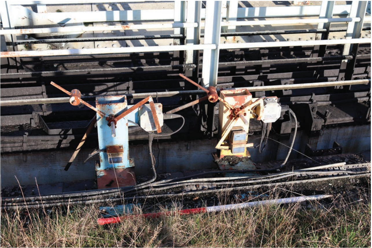
Plate 139: Gasholder No 5, detail view of high and sunstock knock-off switches bolted to the top of the tank, from the SSW
