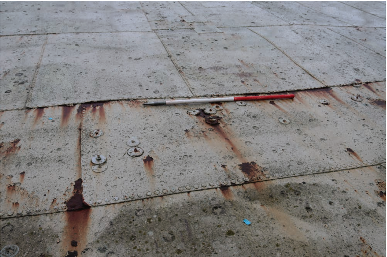
Plate 133: Gasholder No 5, detail view of small bolted circle repairs, from the SSW
