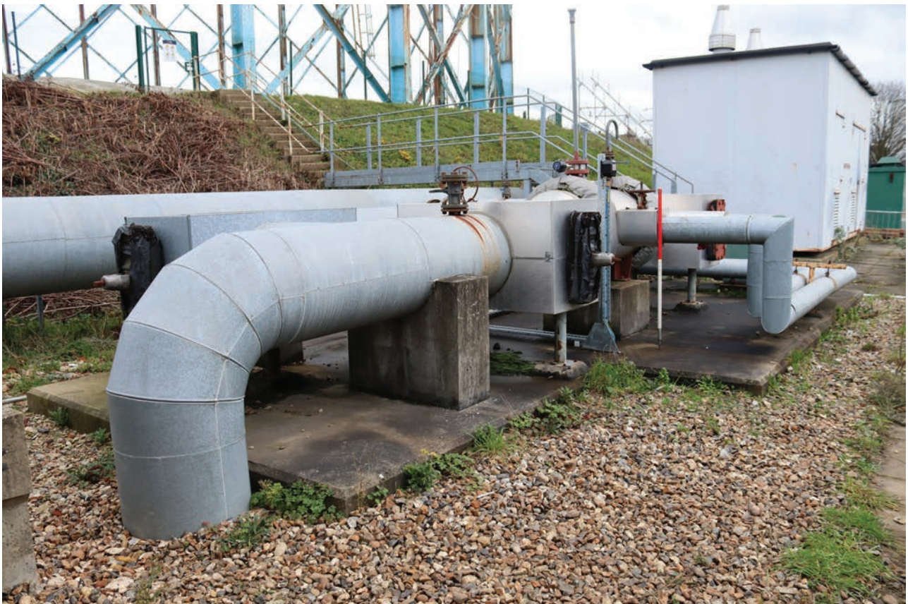
Plate 168: Structures 1 & 2, general view of pipework between the District Governor House and the Boiler House, from the WNW
