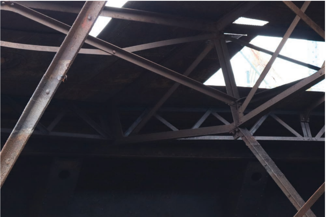
Plate 91: Gasholder No 5, general view of the multi-directional trussing of the crown support frame, from the north-east
