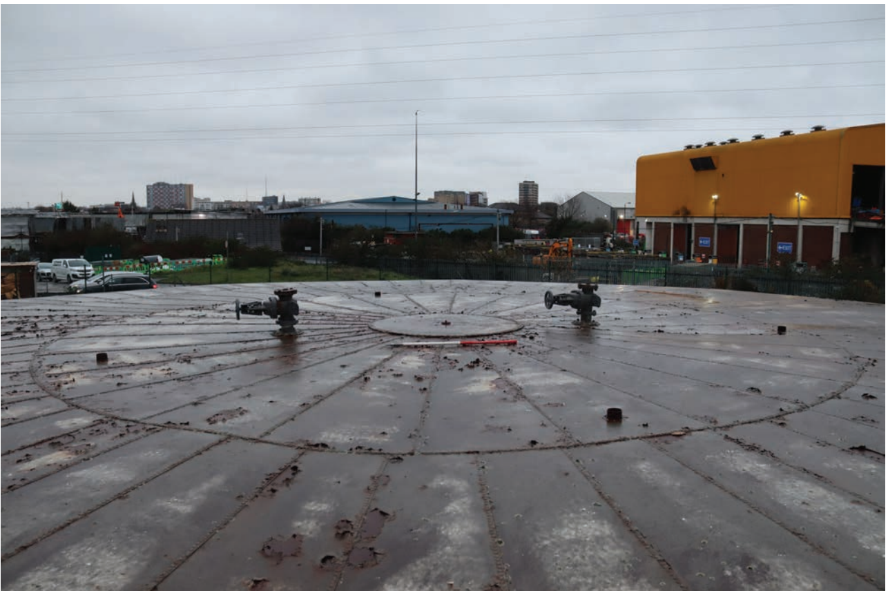
Plate 50: Gasholder No 4, general view of the top of the crown showing central circular steel sheet, crown vents and purge points, from the SSW
