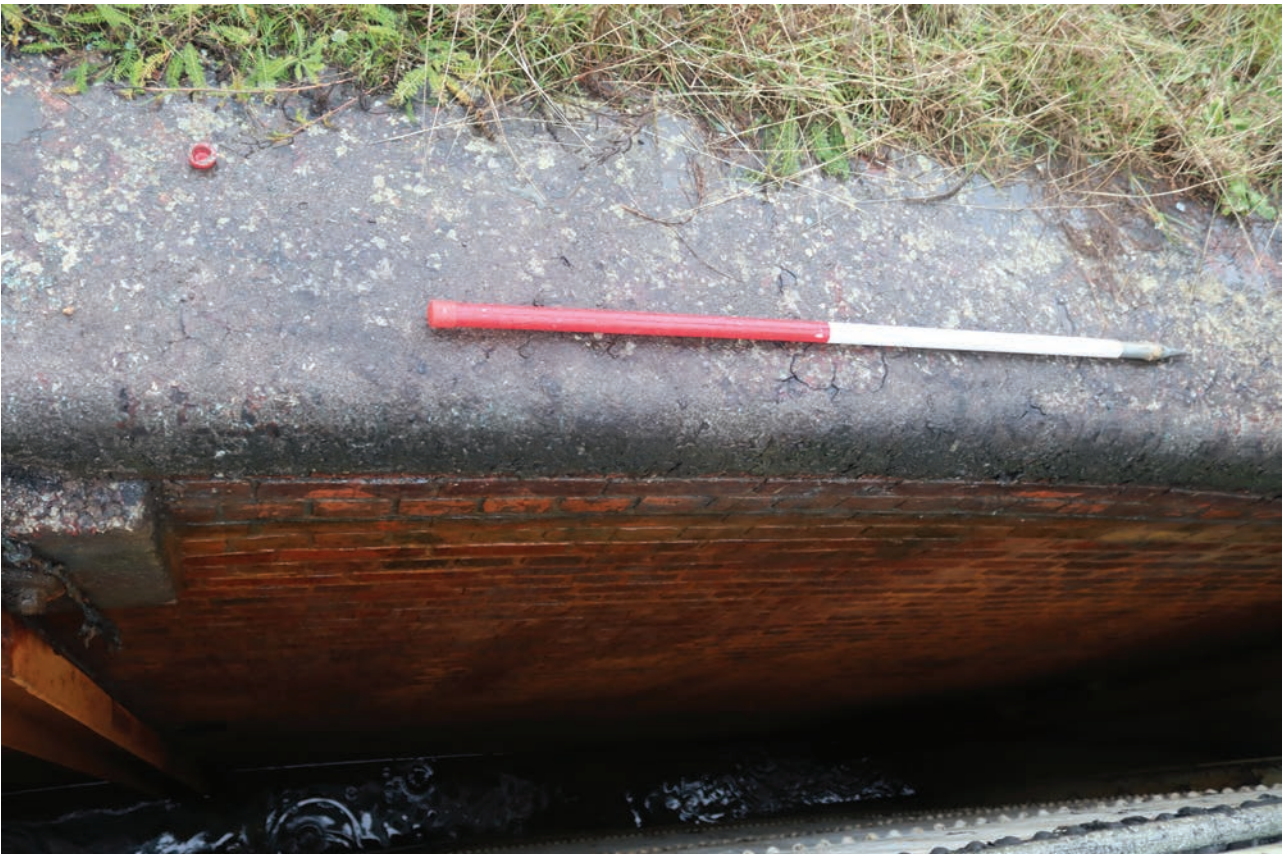
Plate 78: Gasholder No 5, detail view of the red brick tank wall, from the south
