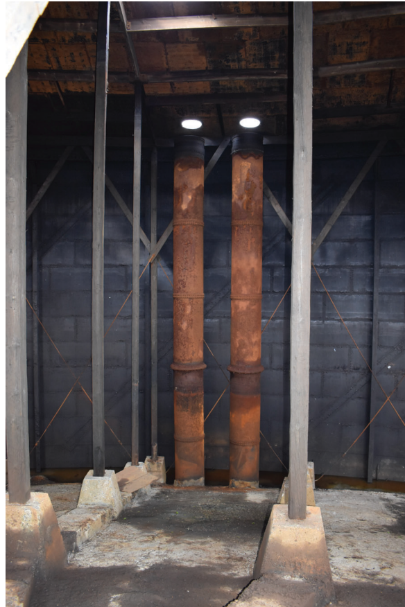
Plate 57: Gasholder No 4, detail view of the gas inlet and outlet pipes, from the ENE
