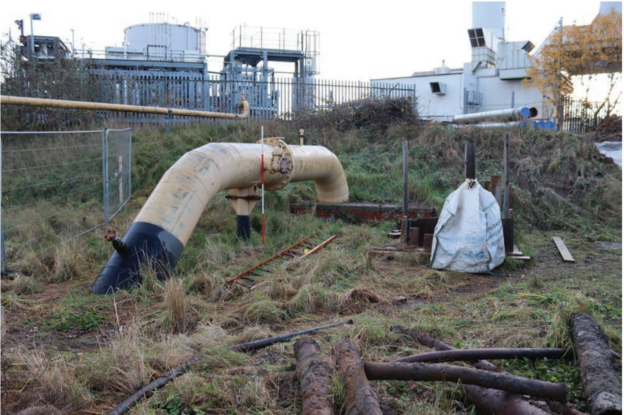
Plate 199: Pipework, detail view of above ground pipework to the south of structure 4, from the WNW
