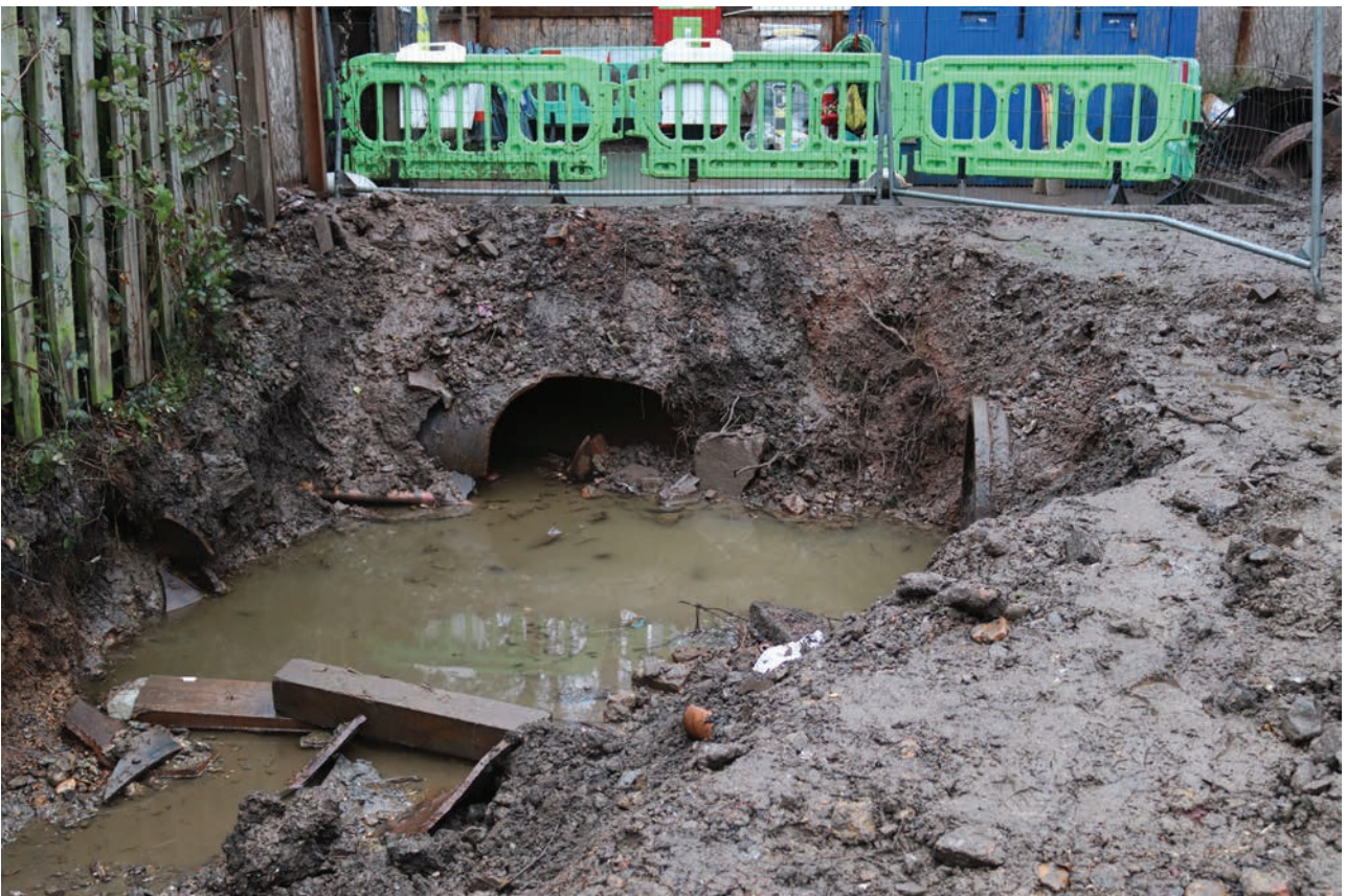
Plate 202: Pipework, section of below ground pipework being replaced outside the survey boundary, from the south-east
