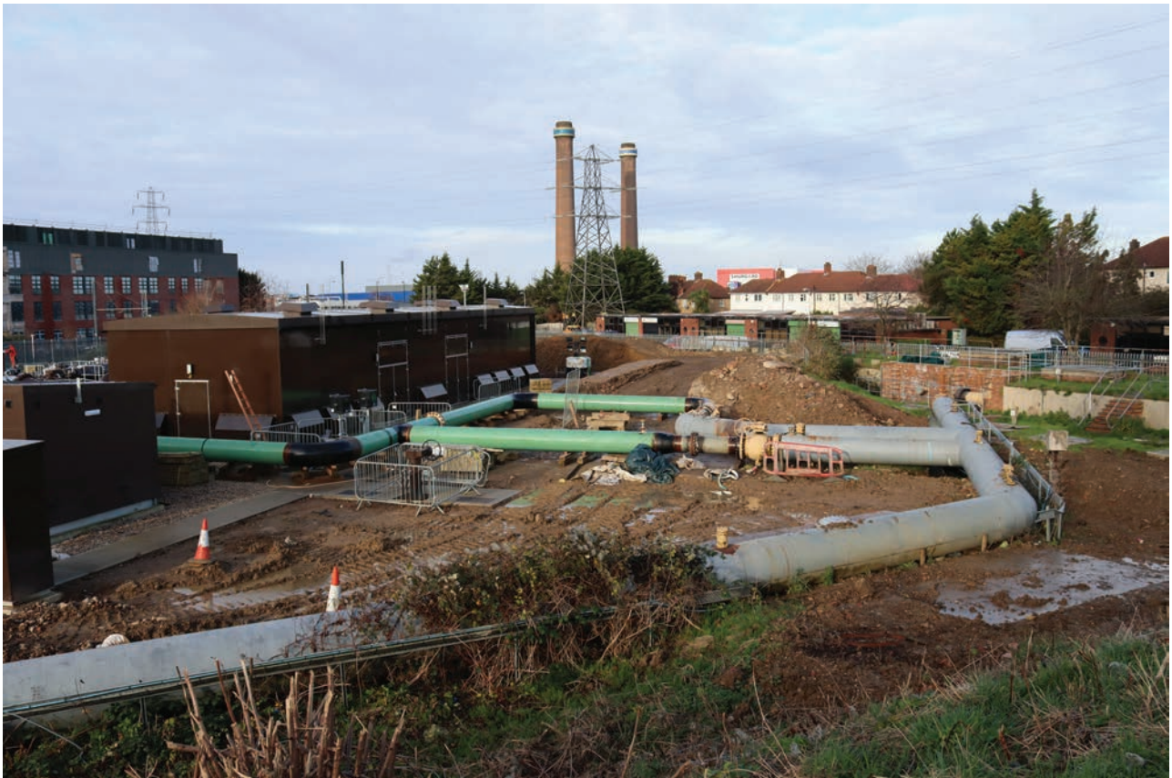
Plate 190: Pipework, general view of old grey pipework meeting new green pipework to the north of the high-pressure works, from the east
