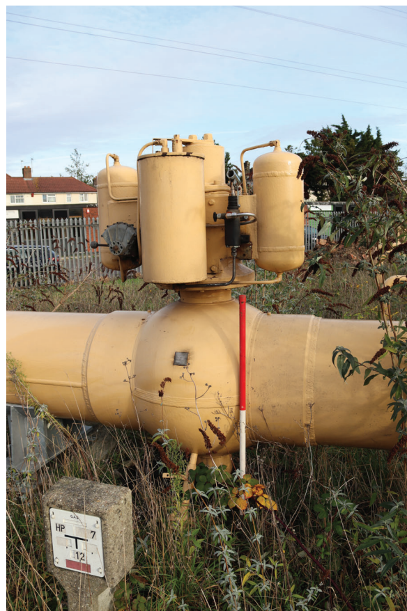
Plate 196: Pipework, detail view of air operated valve, from the WSW
