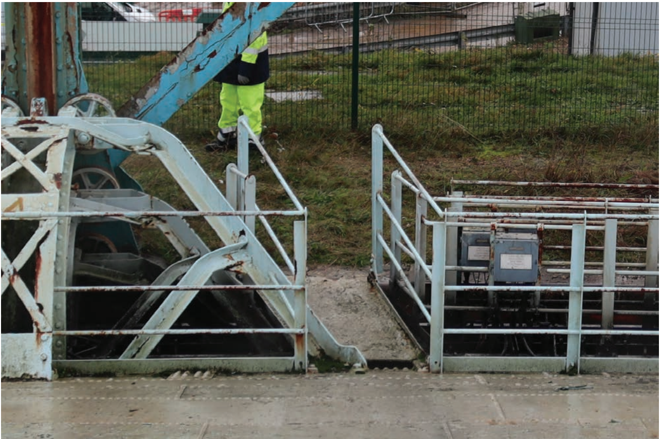
Plate 122: Gasholder No 5, detail view of platform access onto the crown between standards 4 and 5, from the NNE
