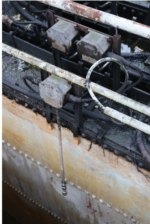
Plate 143: Gasholder No 5, detail view of float switch monitoring the tank water level, from the south-east
