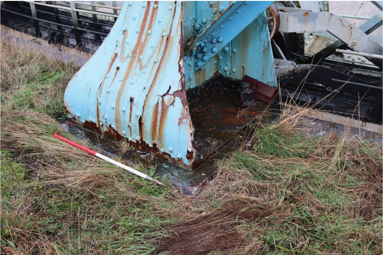
Plate 97: Gasholder No 5, detail view of concrete foundation that standard 8 is bolted to at the base, from the south-west
