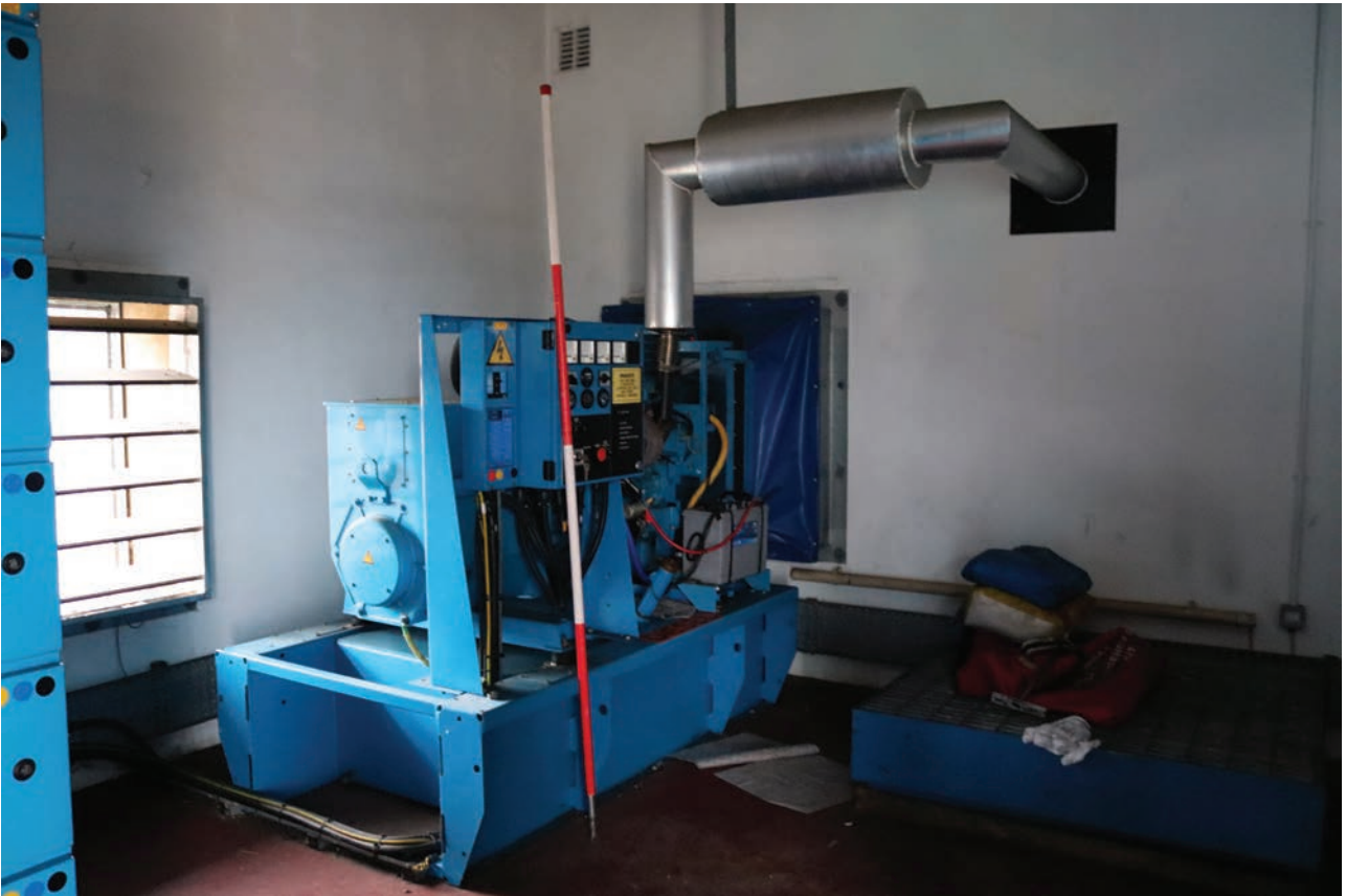
Plate 175: Structure 4, detail view of the booster motor within the Switch Room, from the WNW
