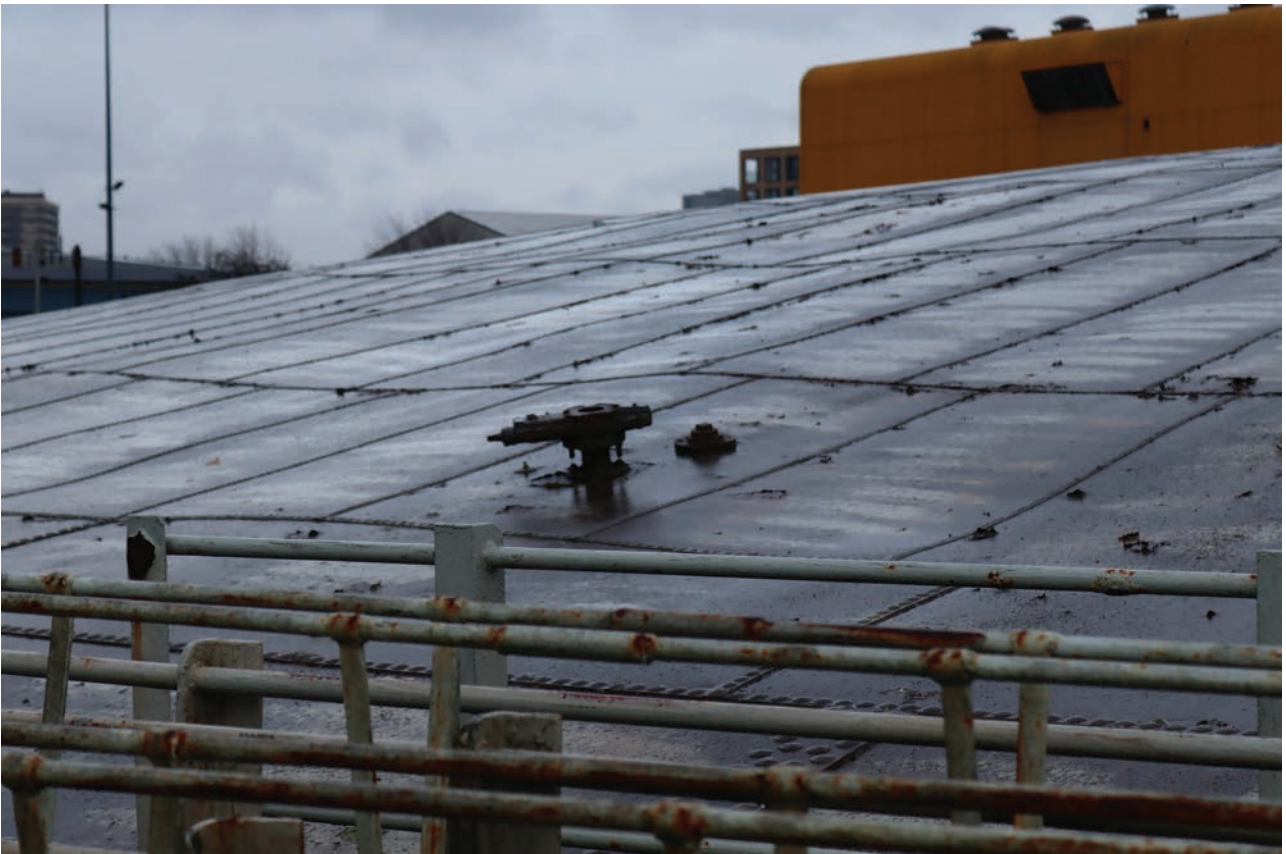
Plate 52: Gasholder No 4, detail view of the crown vent on the north-west side of the holder, from the WSW
