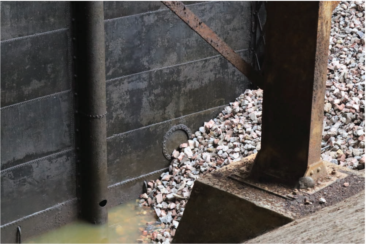
Plate 119: Gasholder No 5, detail view of cotter plate and water regulating grip pipe at the base of the top lift wall interior, from the WSW
