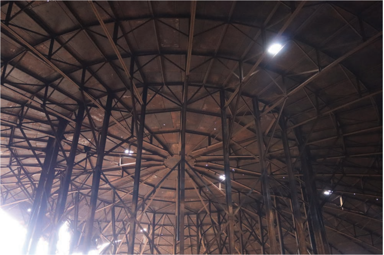
Plate 89: Gasholder No 5, general view of the centre of the crown rest frame dome with ring and spoke design, from the NNW
