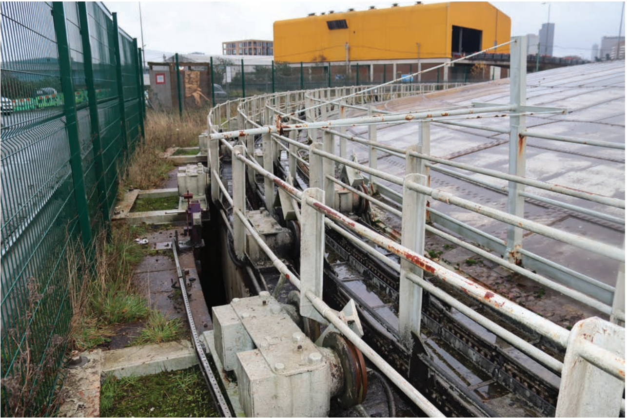
Plate 61: Gasholder No 4, detail view of striker arm with no associated knock-off switch located on the north-west side of the holder, from the west
