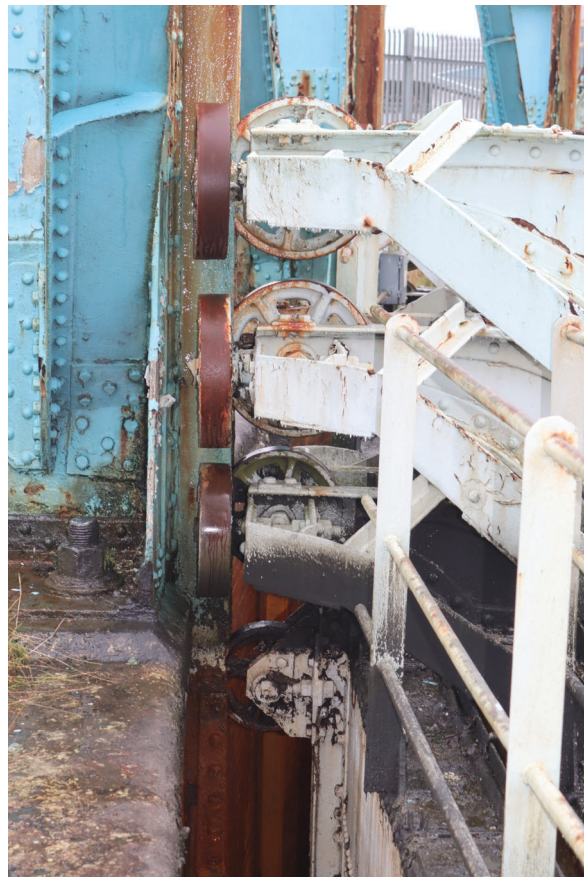
Plate 110: Gasholder No 5, detail view of single or triple roller sets on the west side of standard 13, from the WSW
