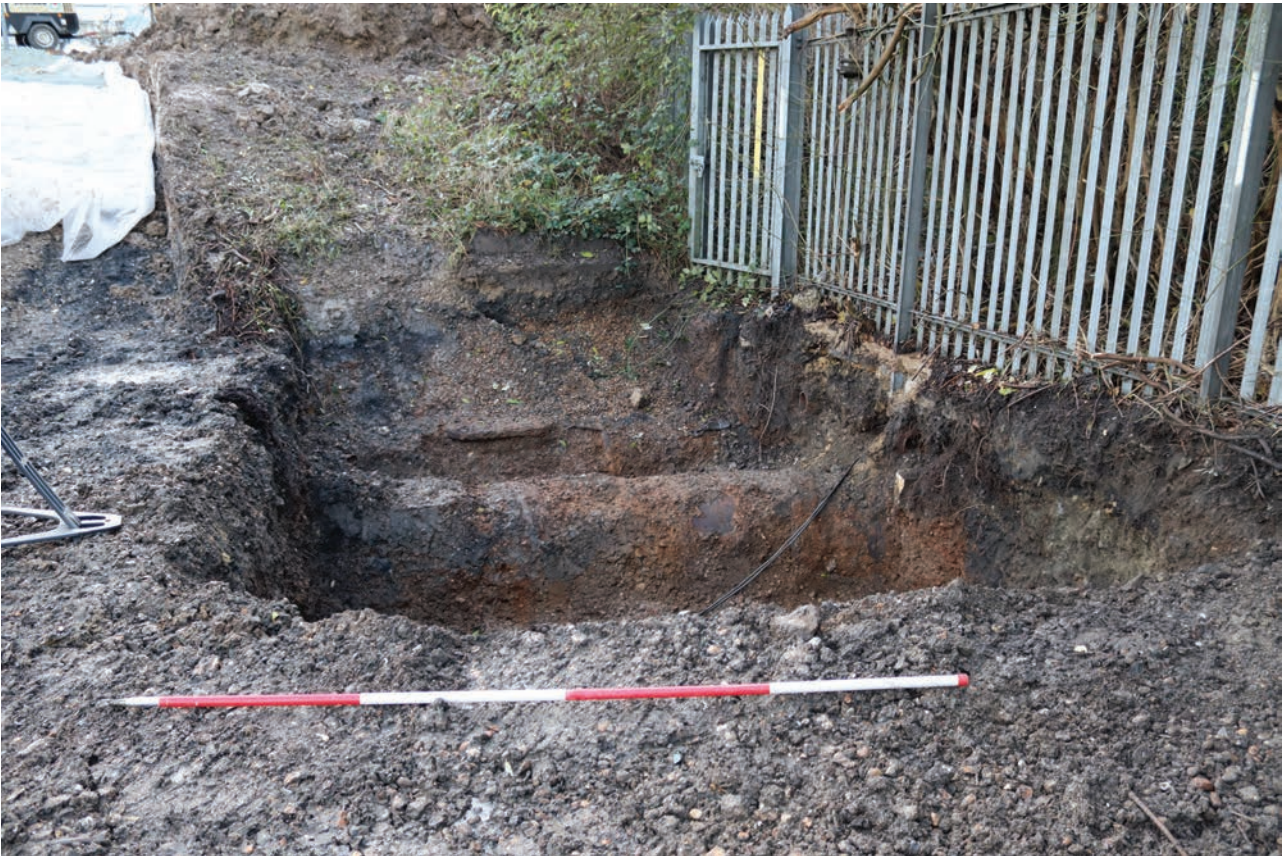
Plate 201: Pipework, section of below ground pipework being replaced during the survey works, from the north-west
