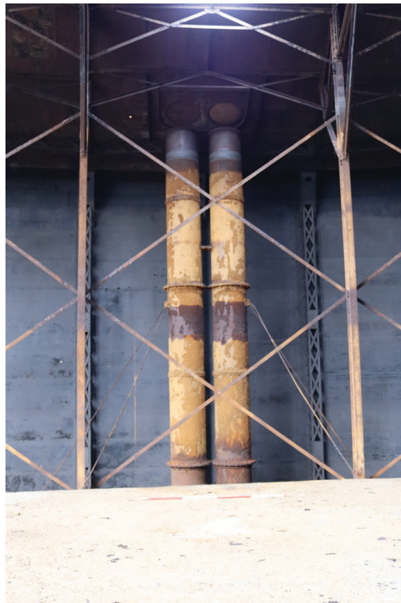
Plate 136: Gasholder No 5, general view of the gas inlet and outlet pipes within the bell with supporting struts, from the north
