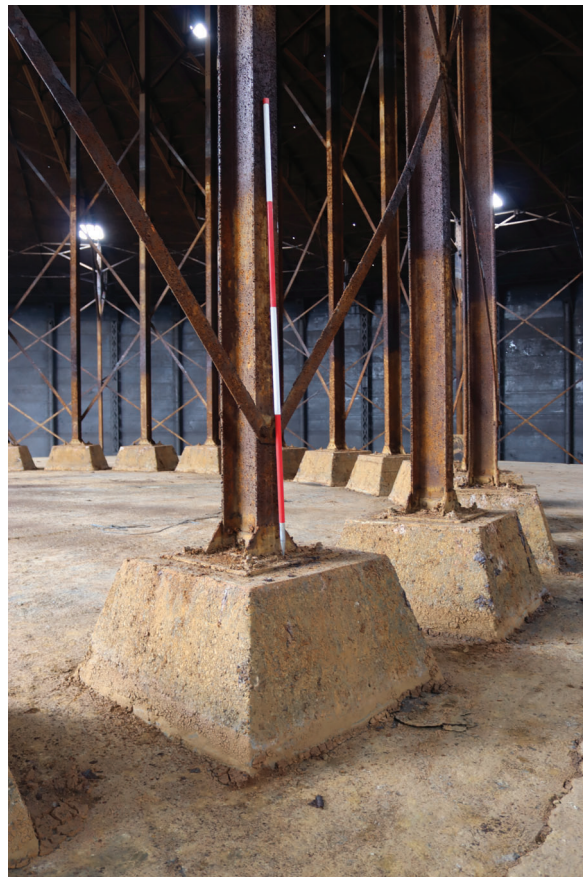
Plate 86: Gasholder No 5, general view of the concrete blocks beneath the vertical supports of the crown rest frame, from the north-east
