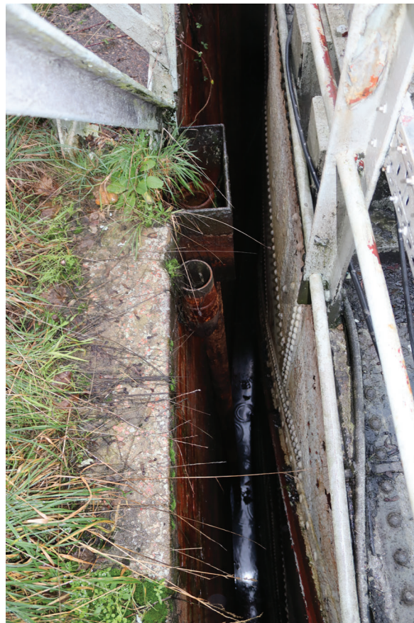
Plate 72: Gasholder No 4, detail view of overflow pipe discharge point, from the SSE
