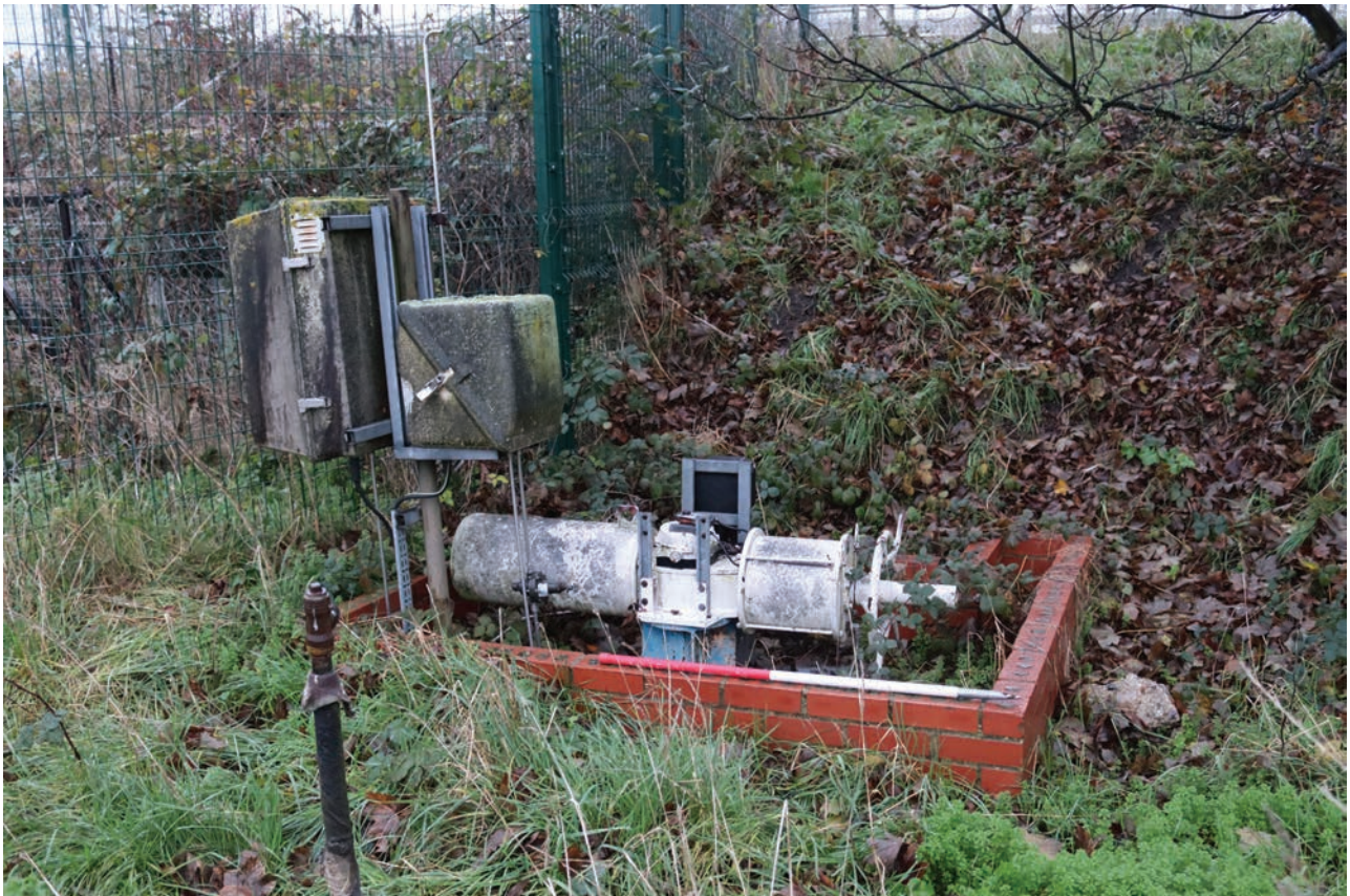
Plate 74: Gasholder No 4, detail view of unidentified electrical machinery within a brick setting, from the west
