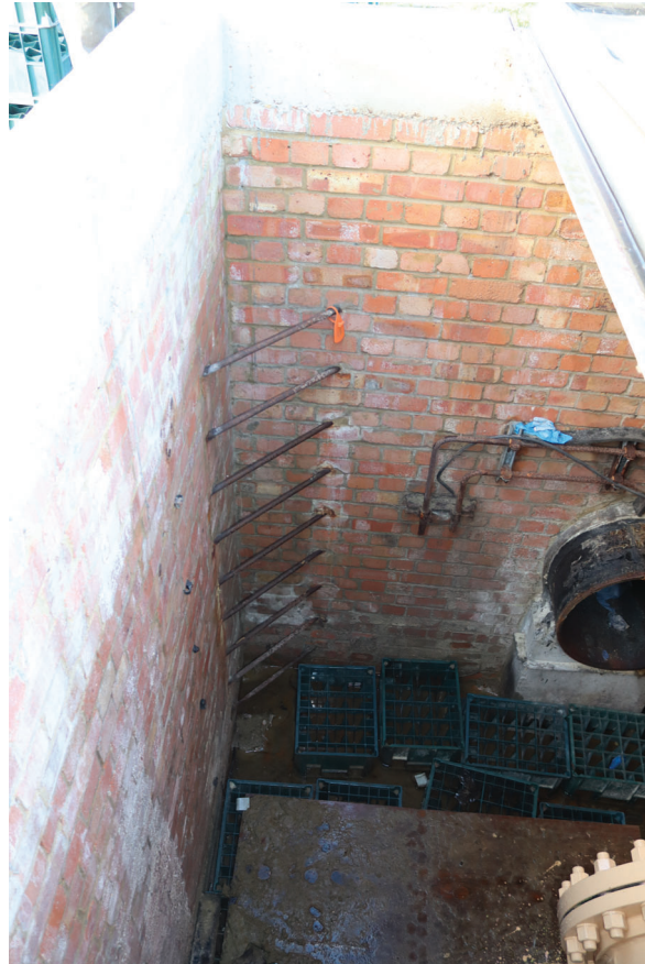
Plate 207: Valve pits, detail view of brick walled pit with access ladder, from the ESE
