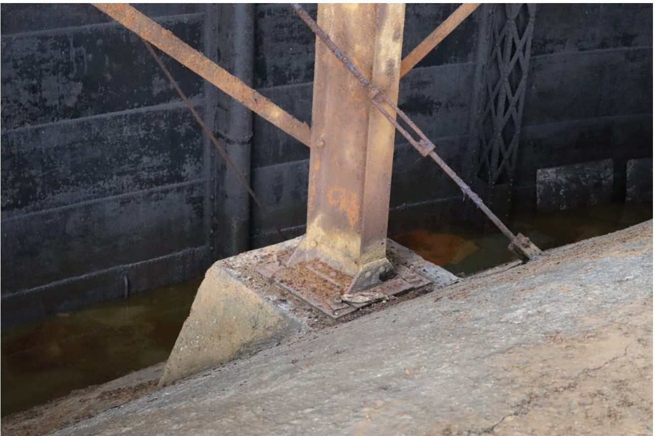
Plate 88: Gasholder No 5, detail view of the angled concrete blocks beneath the outer ring of steel supports of the crown rest frame, from the north-east
