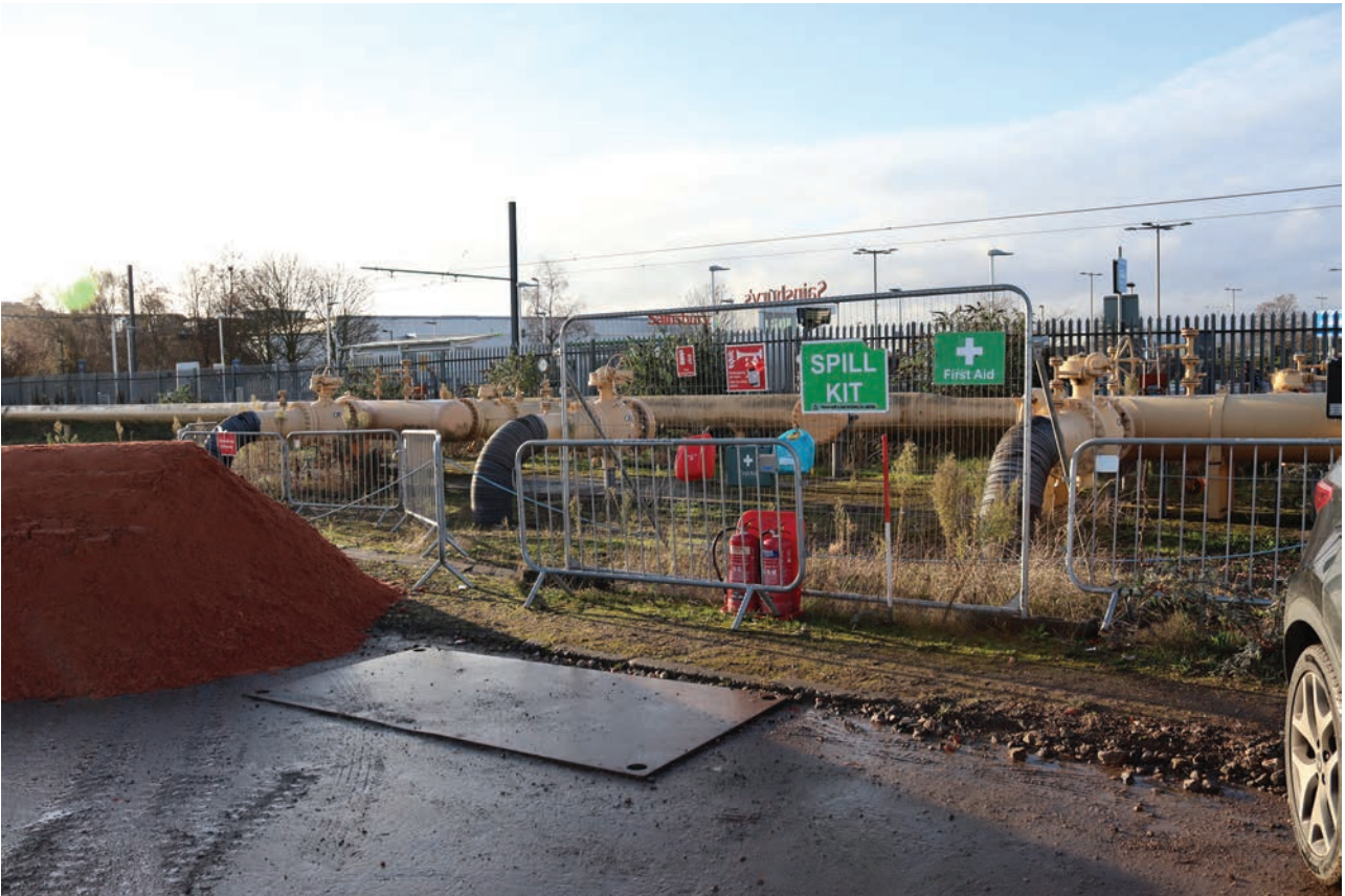
Plate 15: General view of pipework in parallel alignment with the south-west site boundary, from the north
