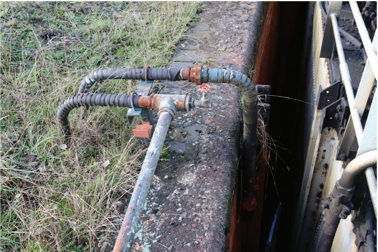
Plate 148: Gasholder No 5, detail view of pipework presumed related to the gas inlet and outlet, from the ESE
