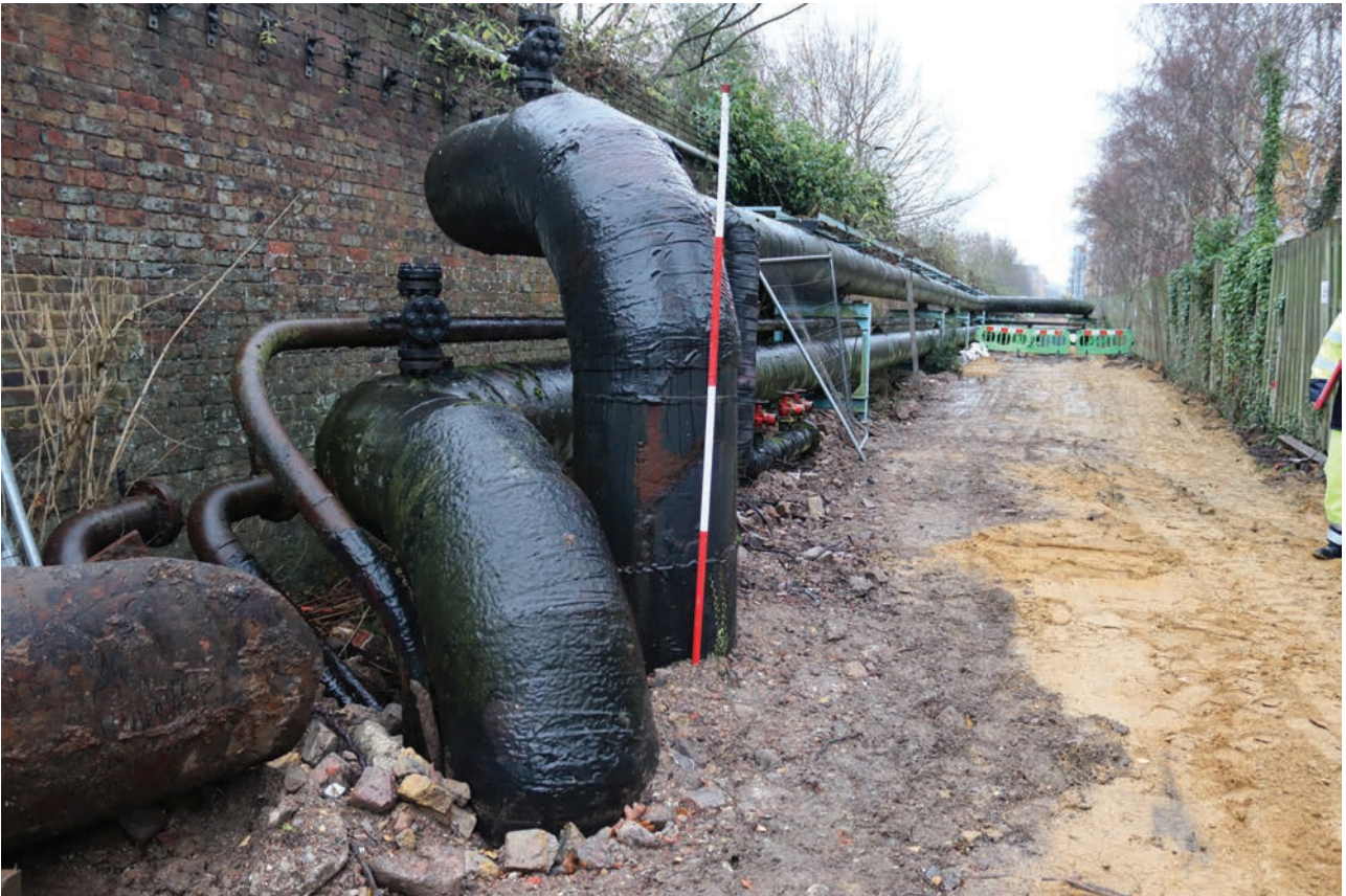
Plate 203: Pipework, general view of above ground pipework to the south of the site boundary, from the north-west
