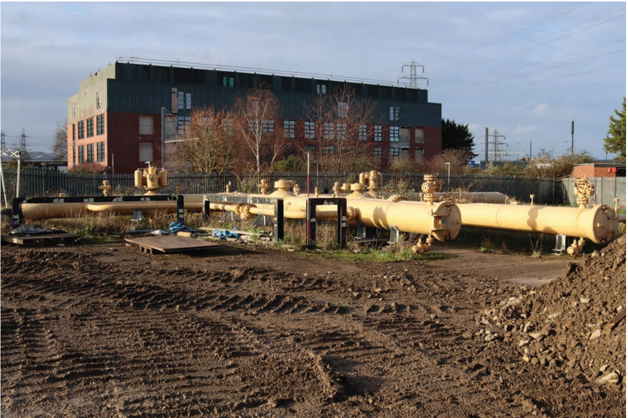
Plate 191: Pipework, general view of above ground pipework in the west corner of the side, from the east
