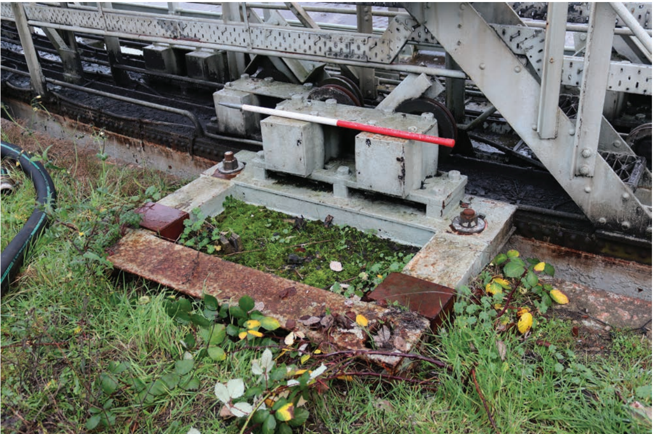
Plate 38: Gasholder No 4, detail view of steel structure supporting the bottom lift guide rollers, from the WSW
