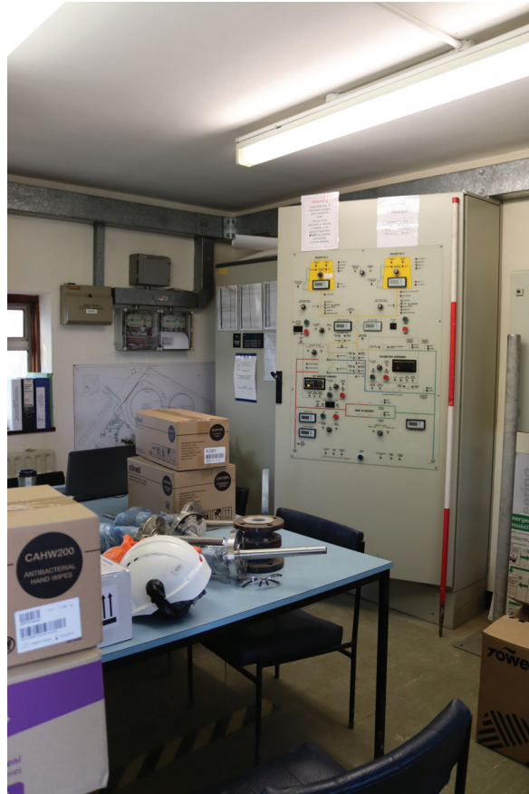
Plate 171: Structure 3, general view of gas monitoring panel for the holders within the Control Room, from the south
