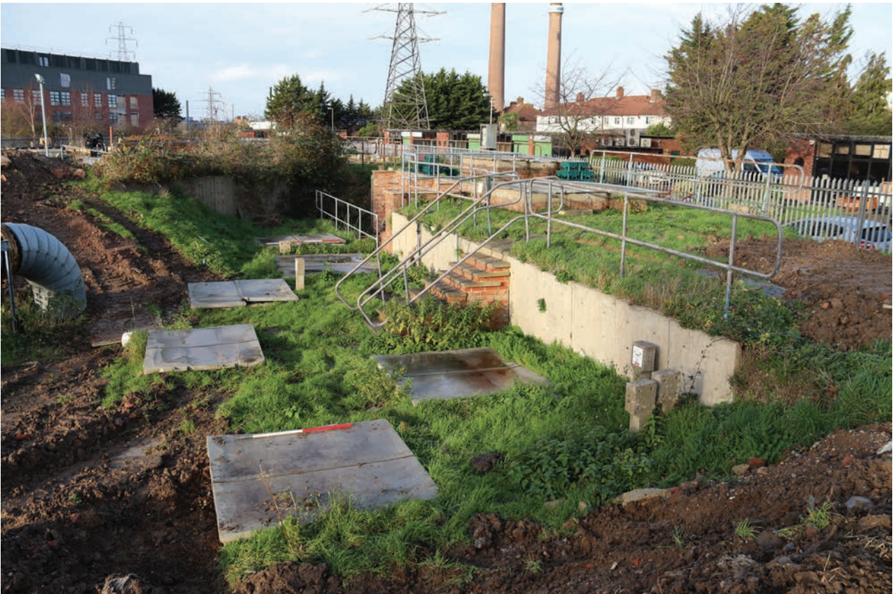
Plate 204: Valve pits, general view of north side double level valve pit area, from the ESE
