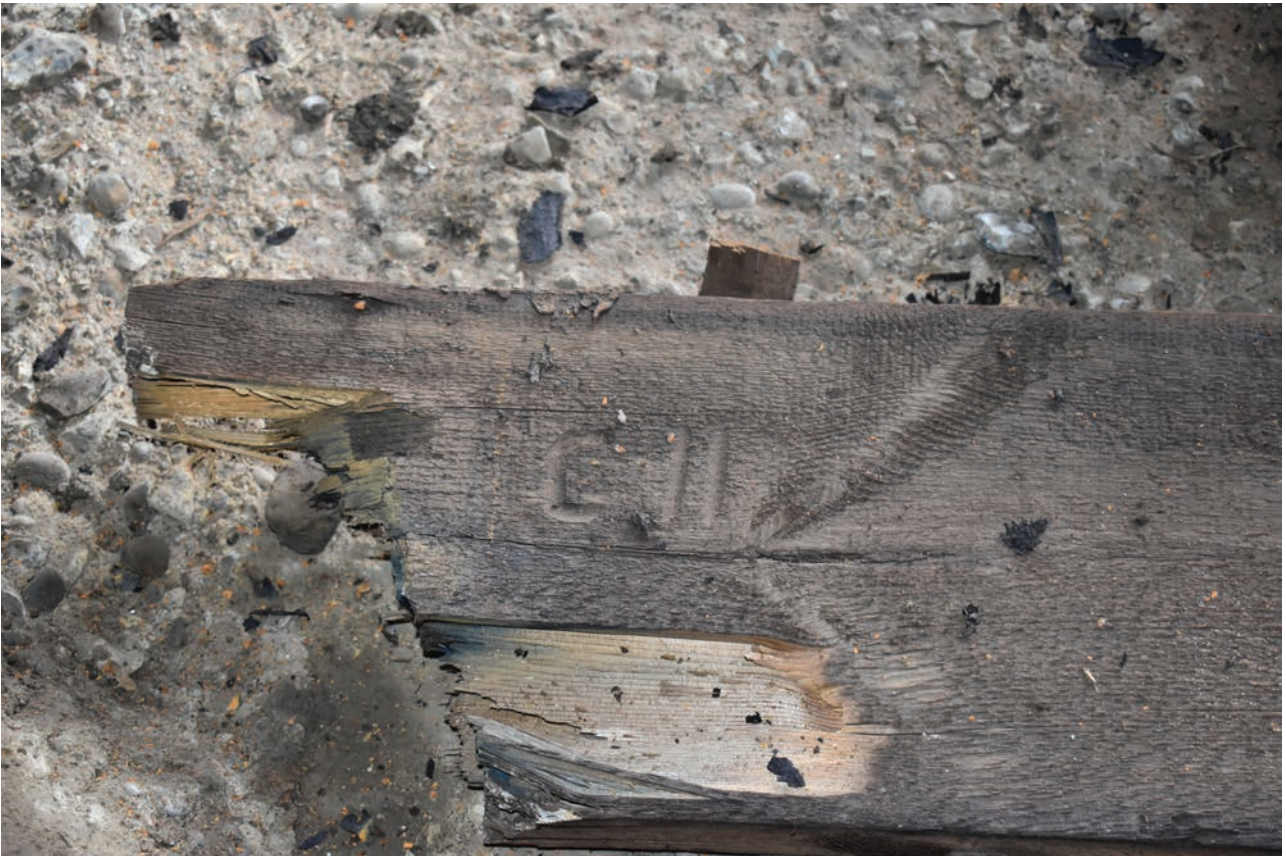
Plate 33: Gasholder No 4, detail view of carved letter and number on a timber associated with building the crown rest frame, not in situ
