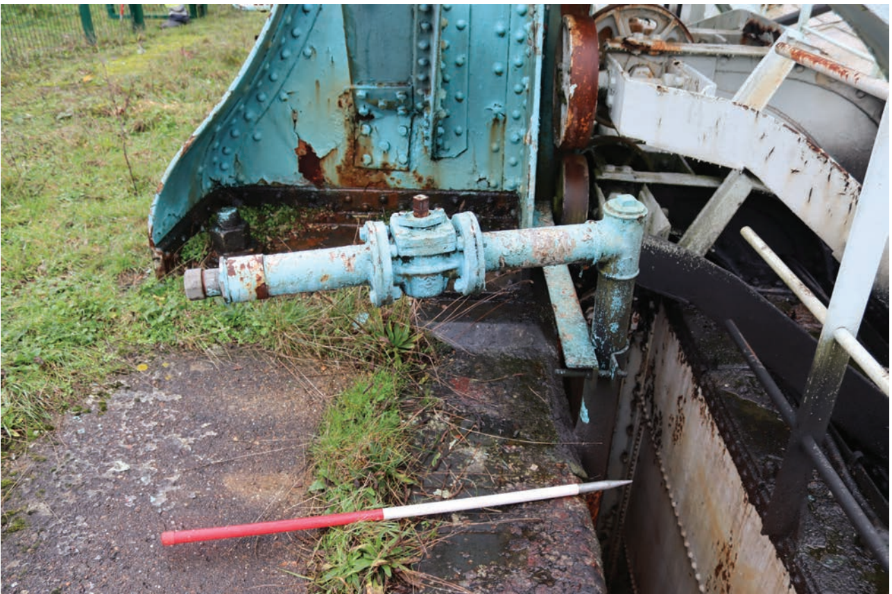
Plate 146: Gasholder No 5, detail view of oil pipe on the east side of standard 26, from the ENE
