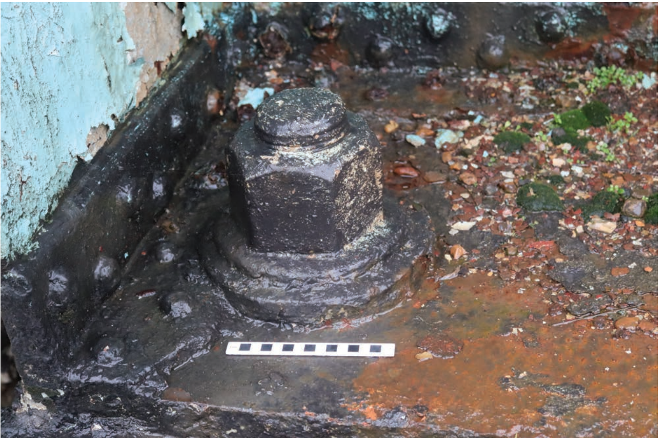
Plate 98: Gasholder No 5, detail view of 12cm diameter bolt at the base of standard 22, from the north
