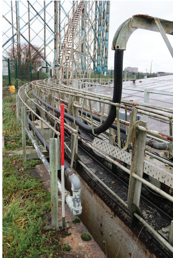
Plate 63: Gasholder No 4, detail view of rubber hose supported by cage and swan neck fixtures, from the SSW
