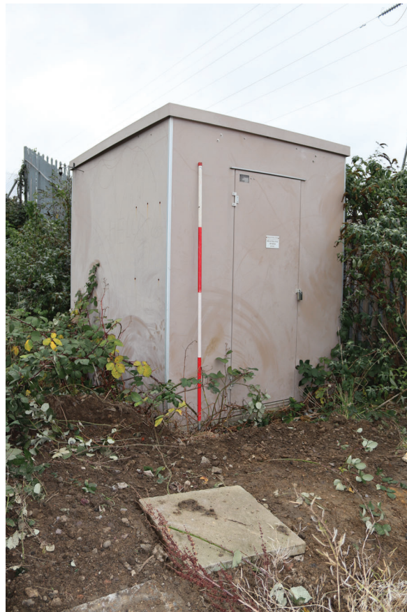
Plate 178: Structure 5, general view of the exterior of the Electrical Room, from the south-east
