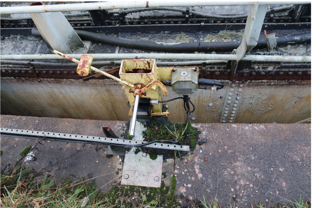
Plate 60: Gasholder No 4, detail view of sunstock knock-off switch located on the south-east side of the holder, from the SSE
