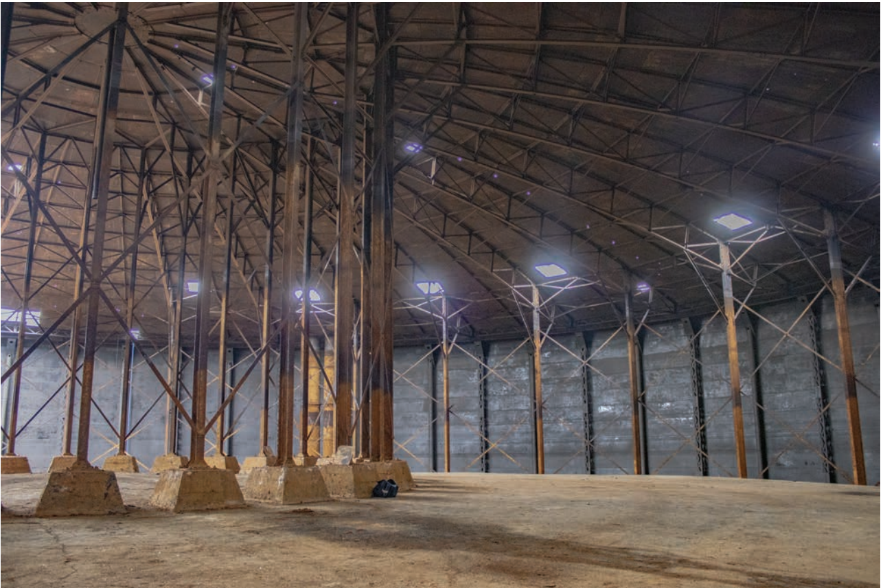
Plate 83: Gasholder No 5, general view of the tank interior showing vertical supports and dome of the crown support frame, from the NNW
