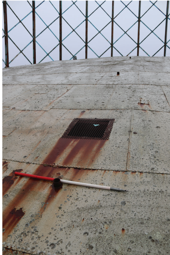
Plate 131: Gasholder No 5, detail view of holes and purge points added to the crown during decommissioning works, from the south-east
