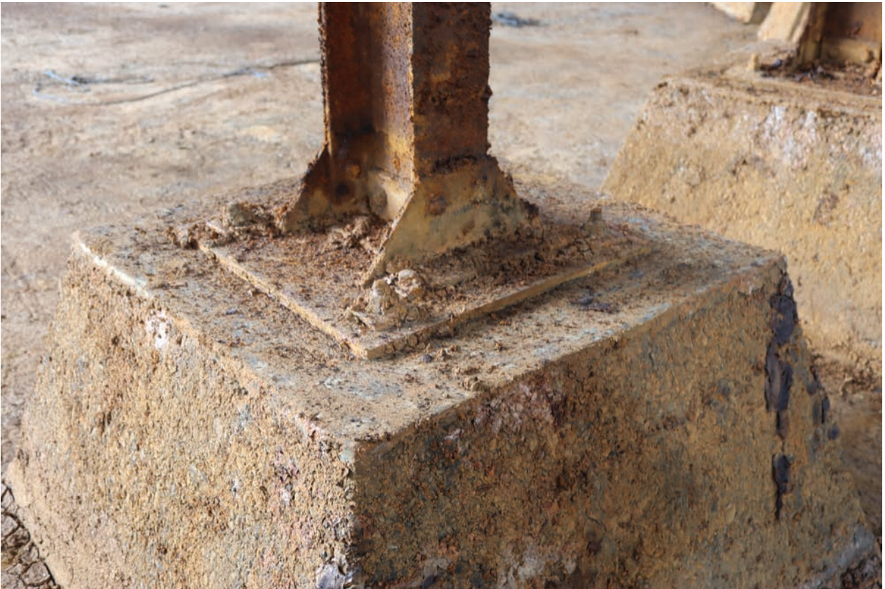
Plate 87: Gasholder No 5, detail view of the joint between the vertical steel support and concrete block beneath of the crown rest frame, from the north-east
