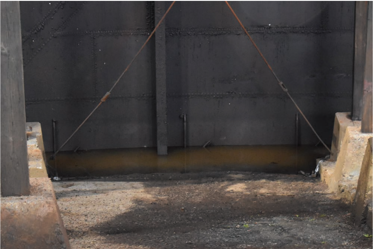
Plate 43: Gasholder No 4, detail view of grip water overflow pipes, from the west
