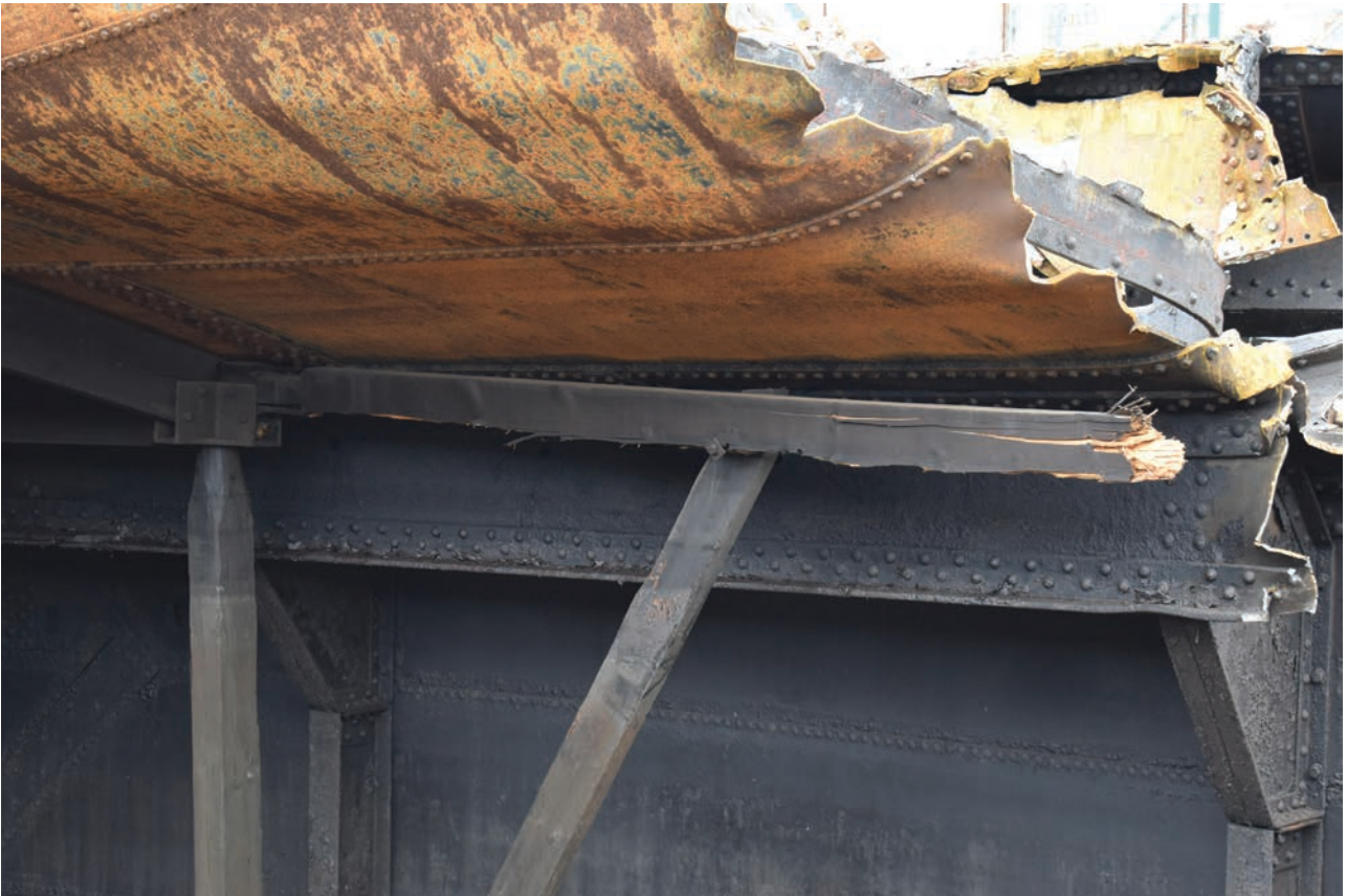
Plate 41: Gasholder No 4, detail view of steel sheet supporting the top curb of the bell, from the south-east
