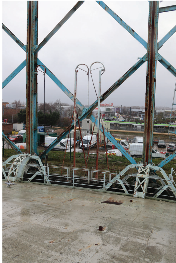
Plate 141: Gasholder No 5, detail view of swan neck fixture situated between standards 3 and 4, from the north
