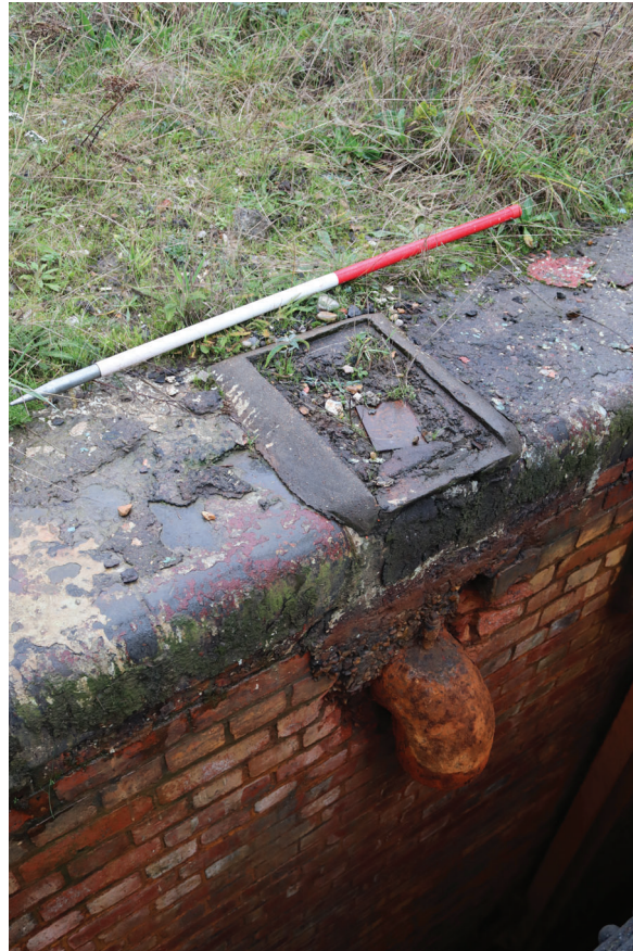
Plate 149: Gasholder No 5, detail view of possible water discharge point between standards 4 and 5, from the east
