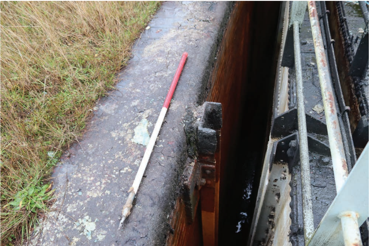
Plate 81: Gasholder No 5, detail view of guide rail set within the tank wall between neighbouring standards, from the WSW
