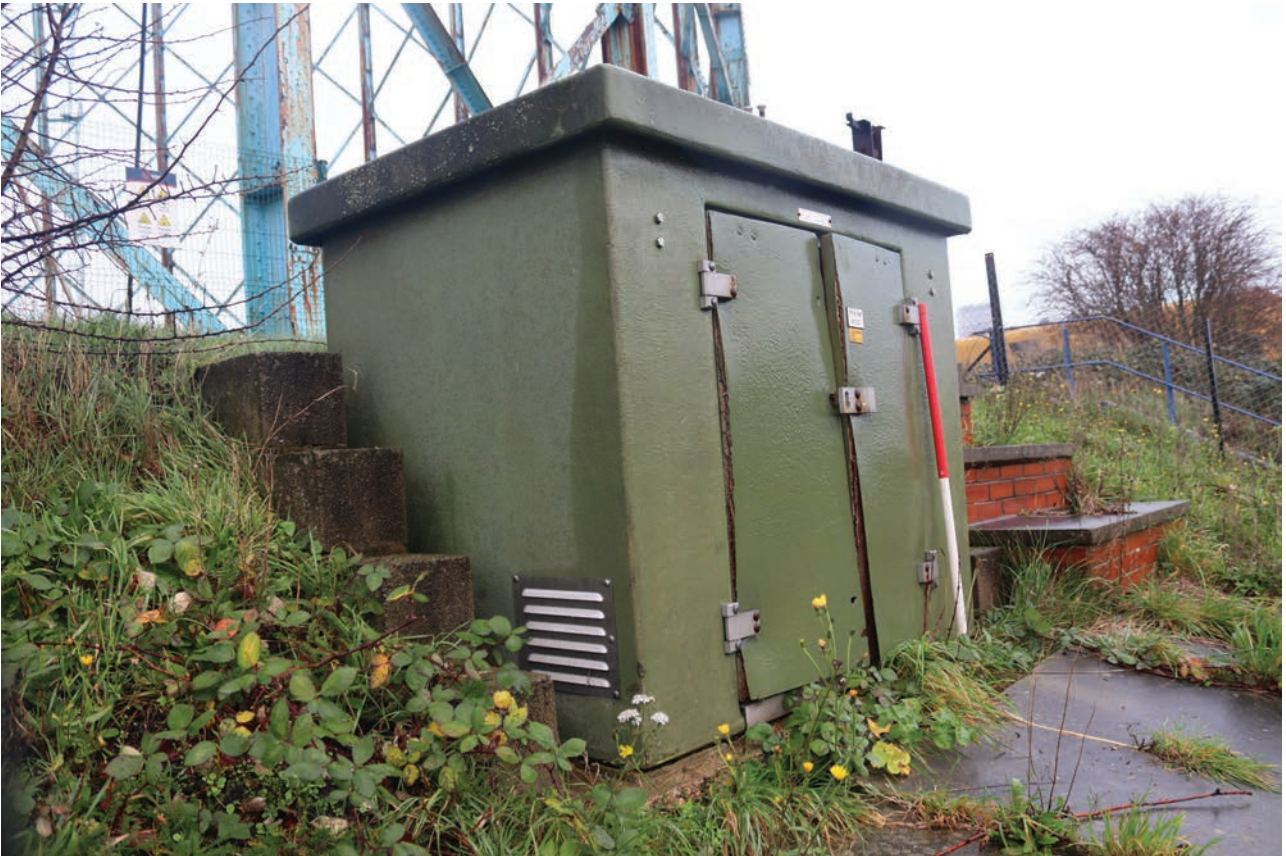
Plate 153: Gasholder No 5, detail view of top up pump hut, from the south-west
