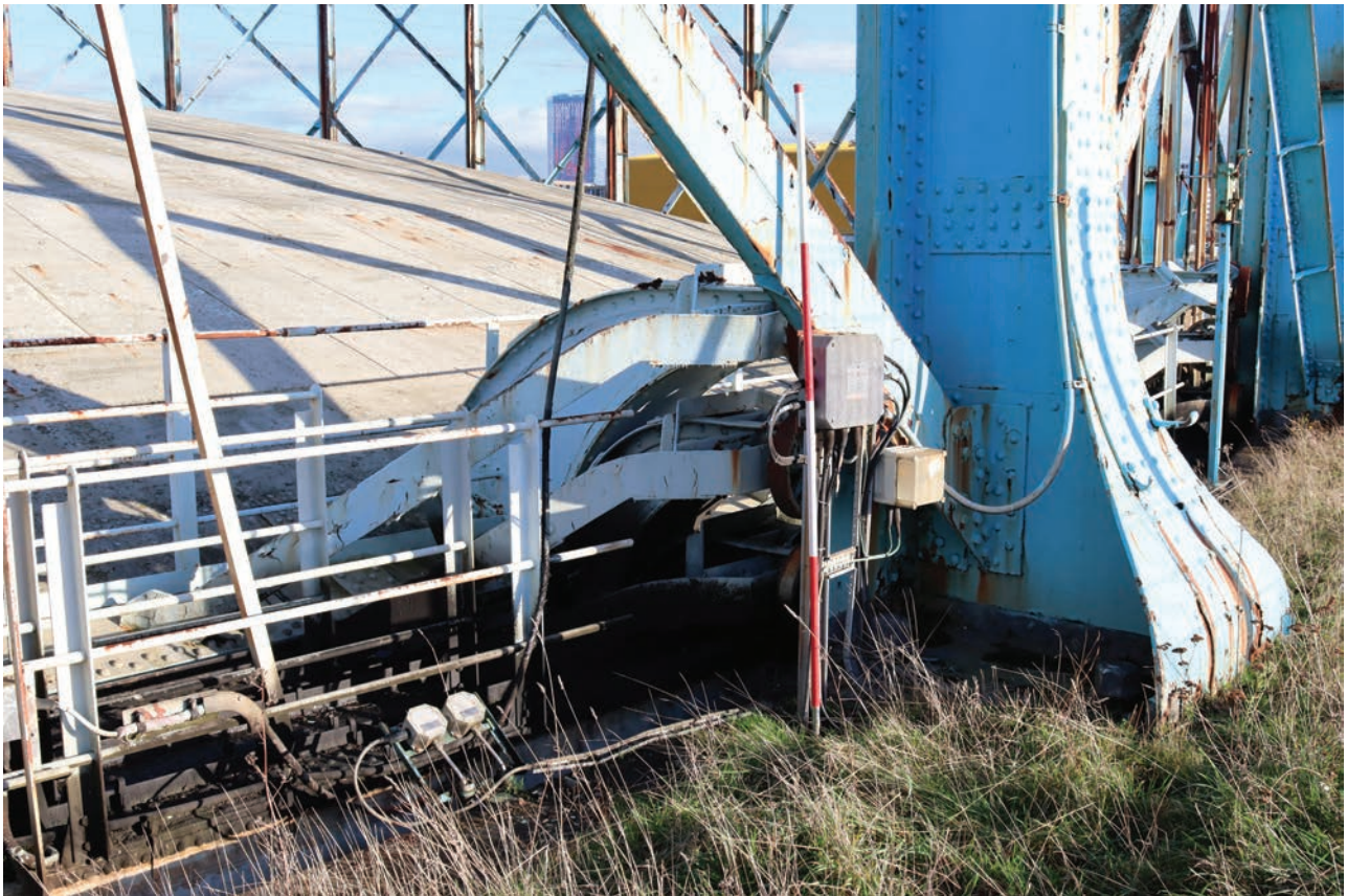
Plate 142: Gasholder No 5, detail view of electrical boxes and float switches on the west side of standard 3, from the WNW
