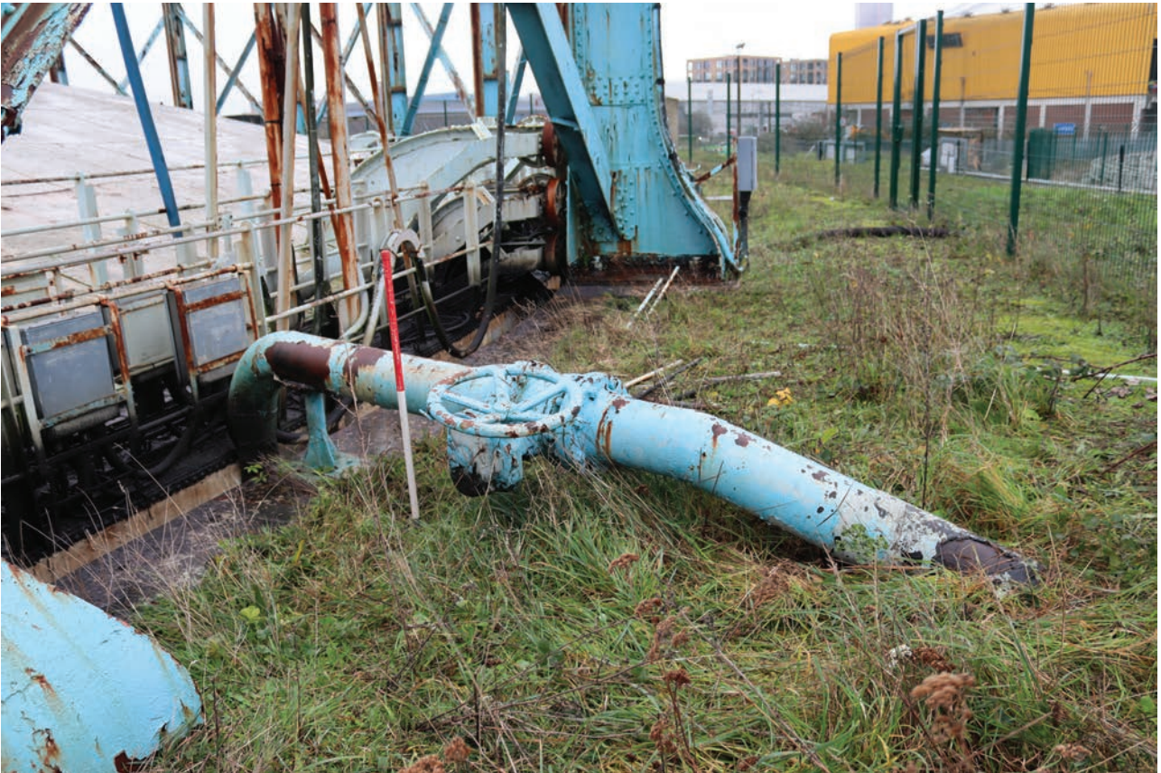
Plate 147: Gasholder No 5, detail view of water pipe between standards 27 and 28, from the south-west
