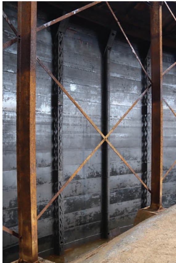
Plate 114: Gasholder No 5, general view of the two types of vertical support on the internal face of the crown lift wall, from the south-west
