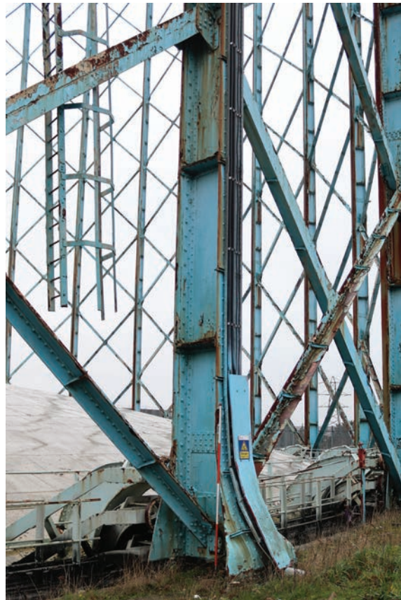
Plate 96: Gasholder No 5, detail view of solid standard design of standard 5, from the ENE
