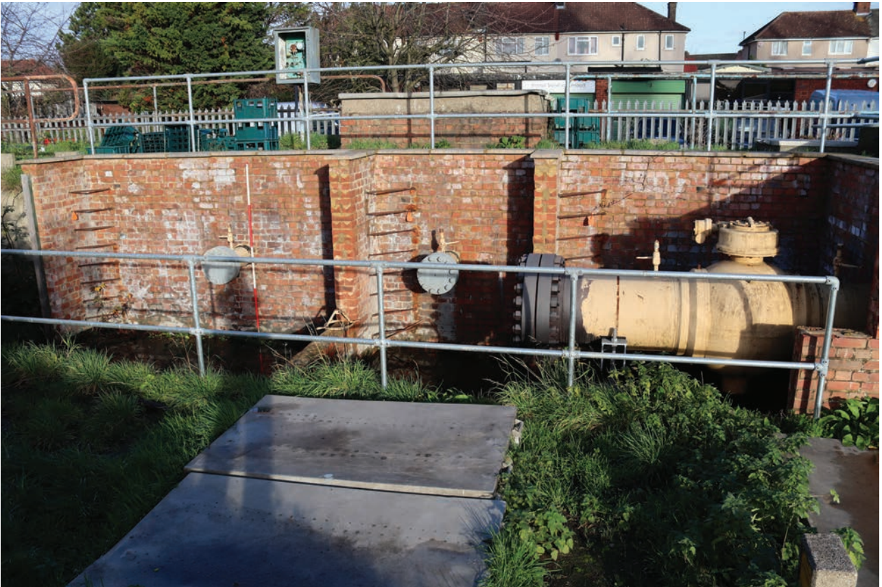
Plate 205: Valve pits, detail view of blanked pipework from the higher level valve pits, from the east
