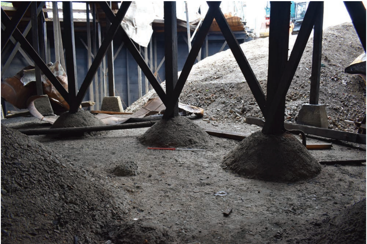
Plate 26: Gasholder No 4, general view of the uneven concrete mounds supporting the posts of ring 1, from the SSE
