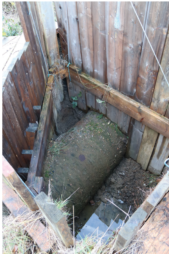
Plate 200: Pipework, detail view of exposed pipework with timber-banked hole supports, from the north
