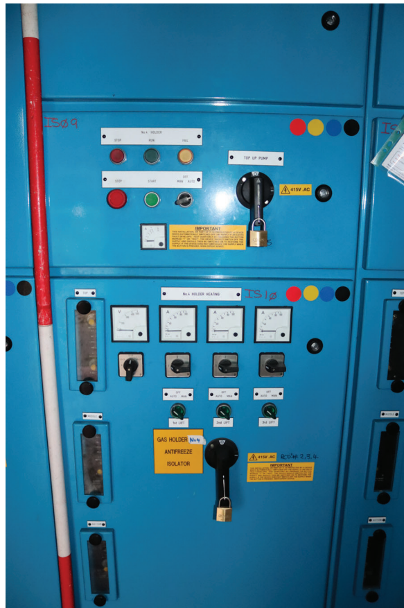
Plate 177: Structure 4, detail view of holder heating system control panel within the Switch Room, from the south-west
