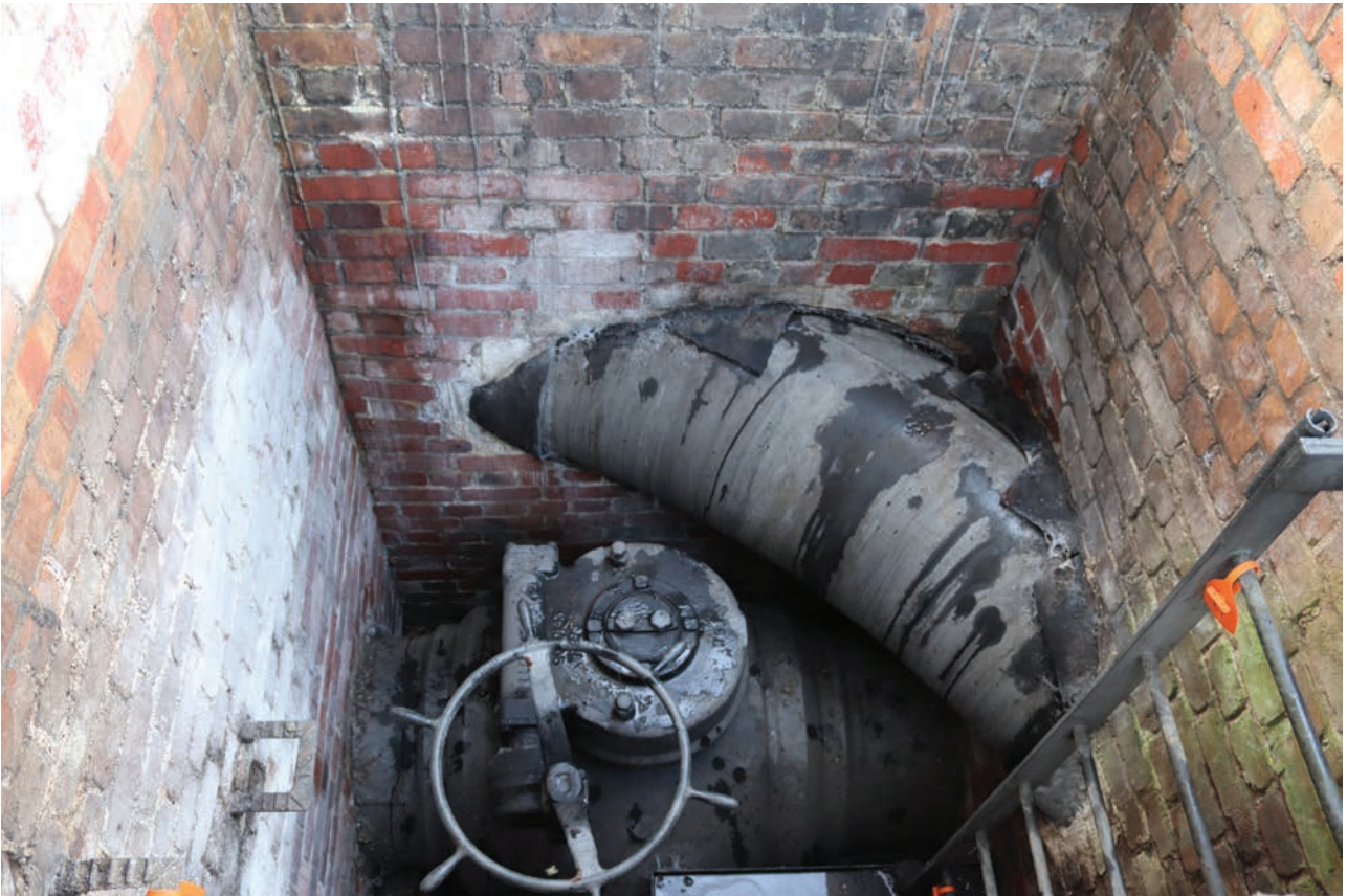
Plate 211: Valve pits, detail view of pits with two pipes, from the north-west
