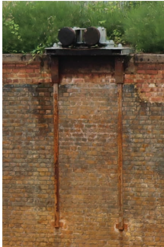
Plate 39: Gasholder No 4, detail view of vertical supports beneath the bottom lift guide rail structure, from the NNW
