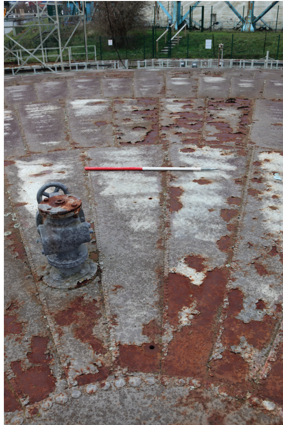
Plate 75: Gasholder No 4, detail view of poor condition rusting crown, from the south-east
