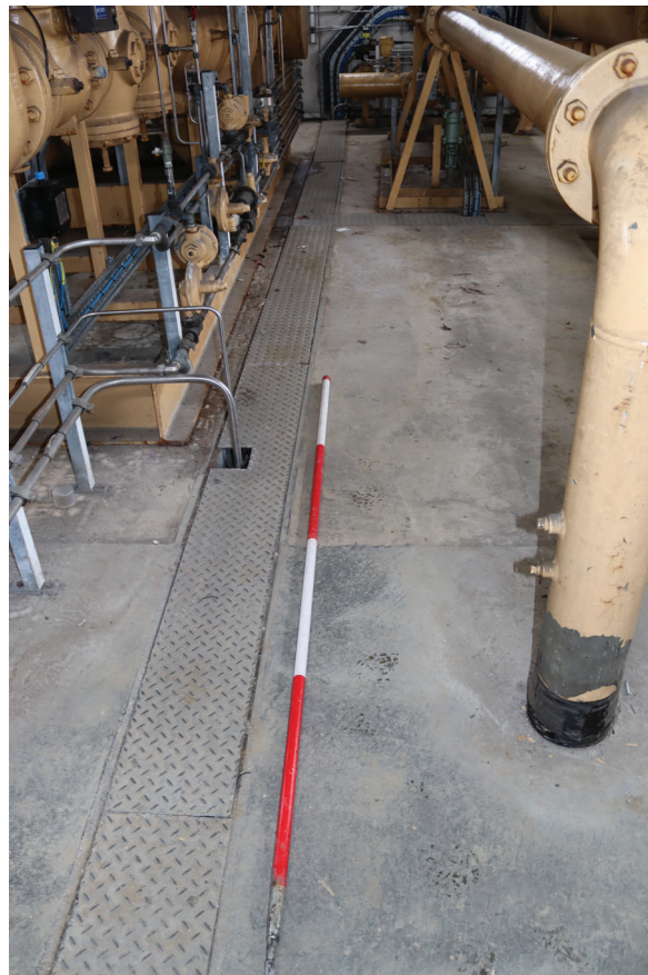
Plate 162: Structure 1, detail view of removeable steel plate in the concrete floor of the District Governor House, from the ENE
