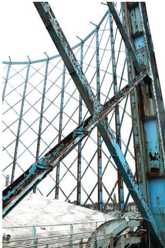
Plate 104: Gasholder No 5, detail view of T-shaped diagonal strut pair facing opposite directions, from the ENE
