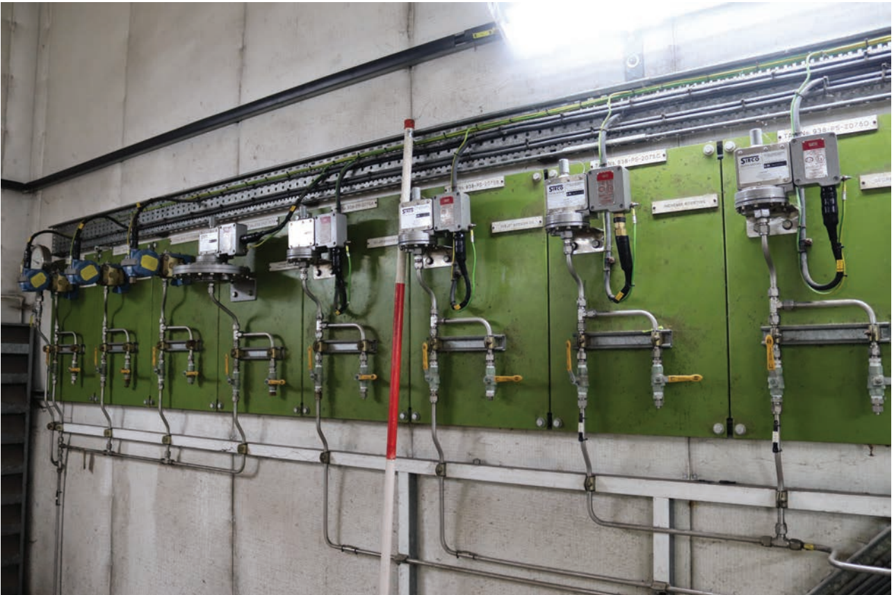
Plate 163: Structure 1, detail view of monitoring panels for boosters within the District Governor House, from the NNE
