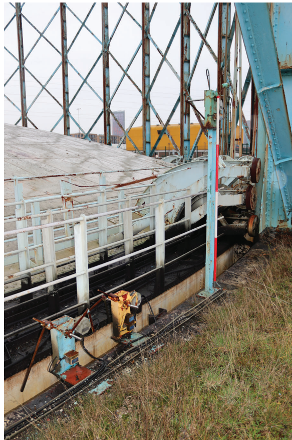
Plate 138: Gasholder No 5, detail view of low, high and sunstock knock-off switches between standards 2 and 3, from the west
