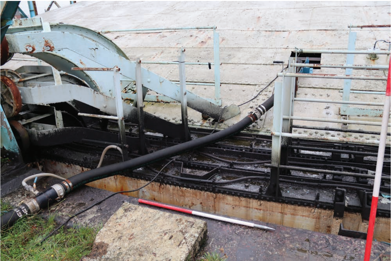
Plate 123: Gasholder No 5, detail view of cut handrails between standards 26 and 27 related to dewatering works, from the SSE
