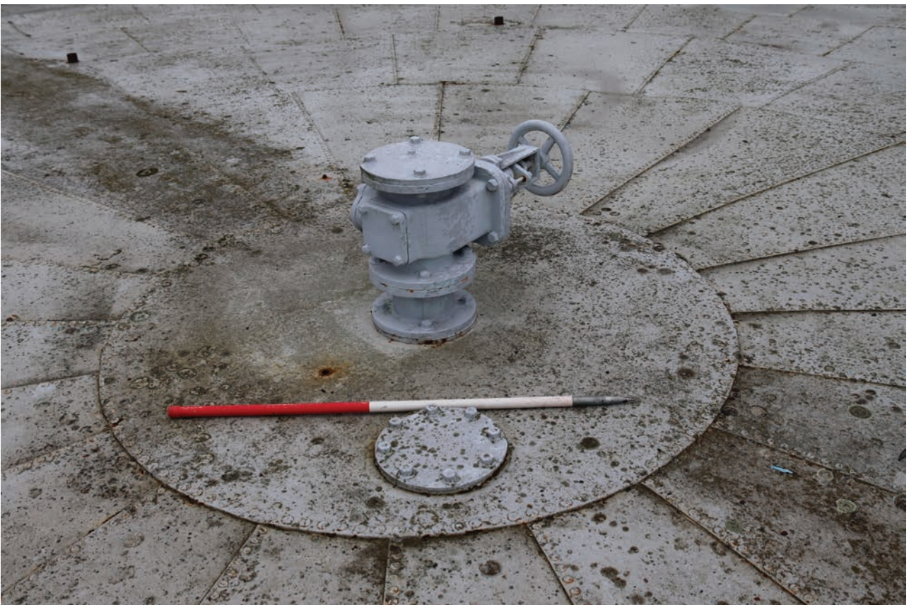
Plate 126: Gasholder No 5, detail view of the centre of the crown showing circular steel sheet and crown vent, from the west
