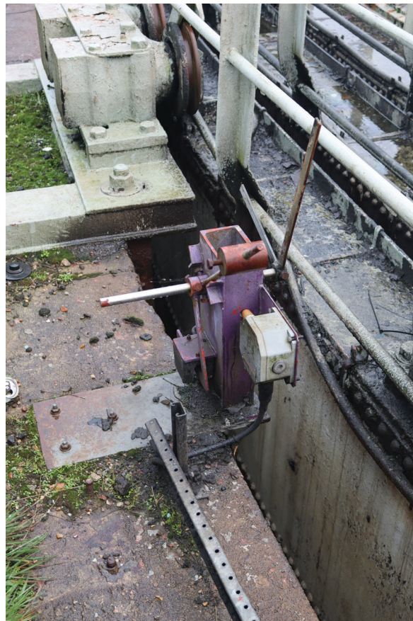
Plate 58: Gasholder No 4, detail view of low knock-off switch on the north-west side of the holder, from the west
