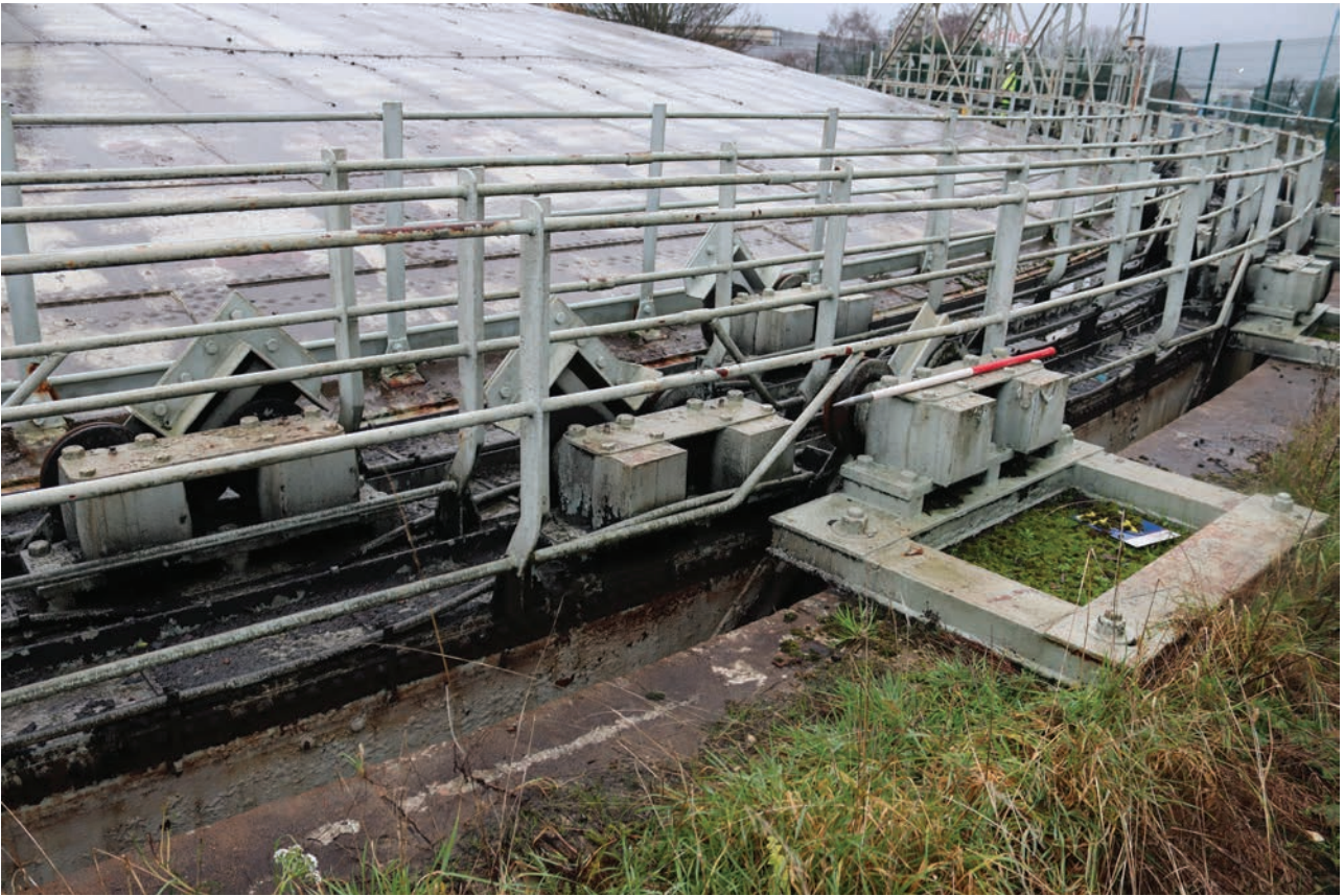
Plate 35: Gasholder No 4, detail view of pairs of tangential guide rollers bolted to the ground and lift tops, from the NNE
