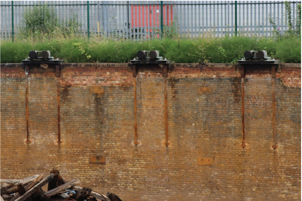
Plate 19: Gasholder No 4, detail view of replaced brick courses at the top of the tank and newer tangential guide roller pair additions, from the NNW
