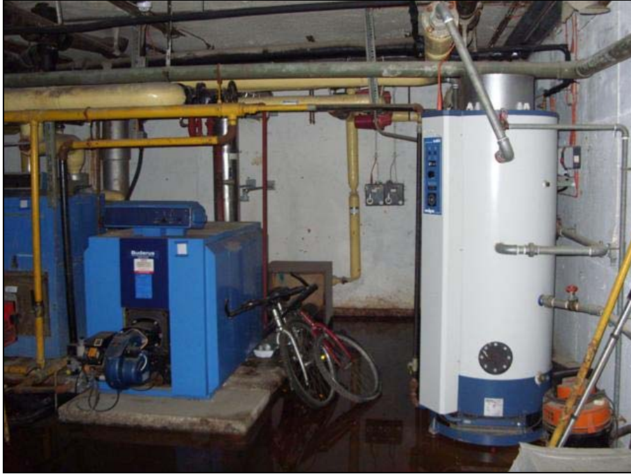
Plate 3: Boiler Room, basement
