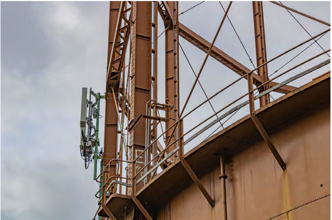
Plate 18 (BEL025): Gasholder No 1, detail of upper walkway on the south-east side of the gasholder from the ENE
