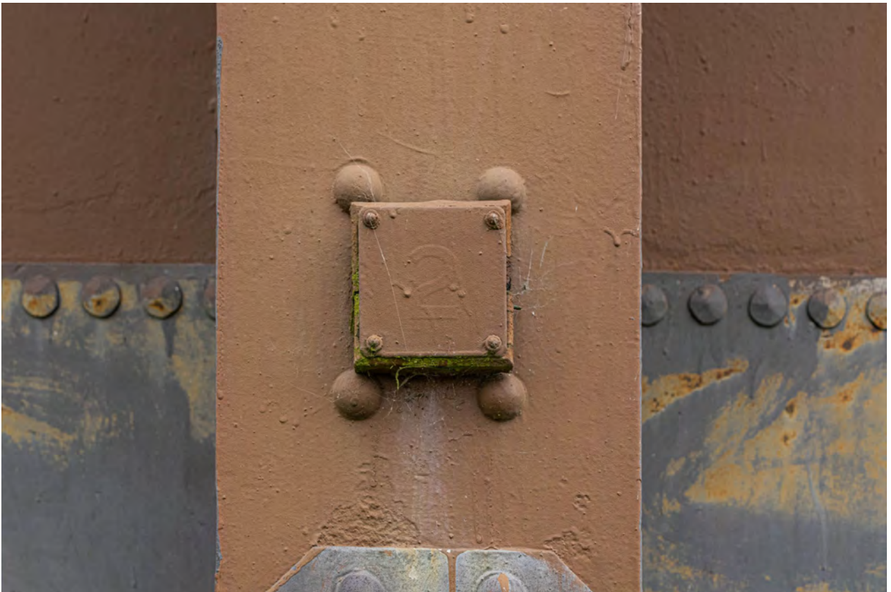
Plate 14 (BEL009): Gasholder No 1, close detail of original number plaque of standard 2 from the north-west
