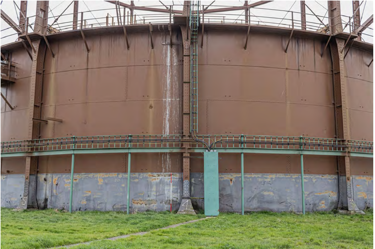
Plate 15 (BEL011): Gasholder No 1, general view of the north side of the gasholder showing above ground tank, from the north
