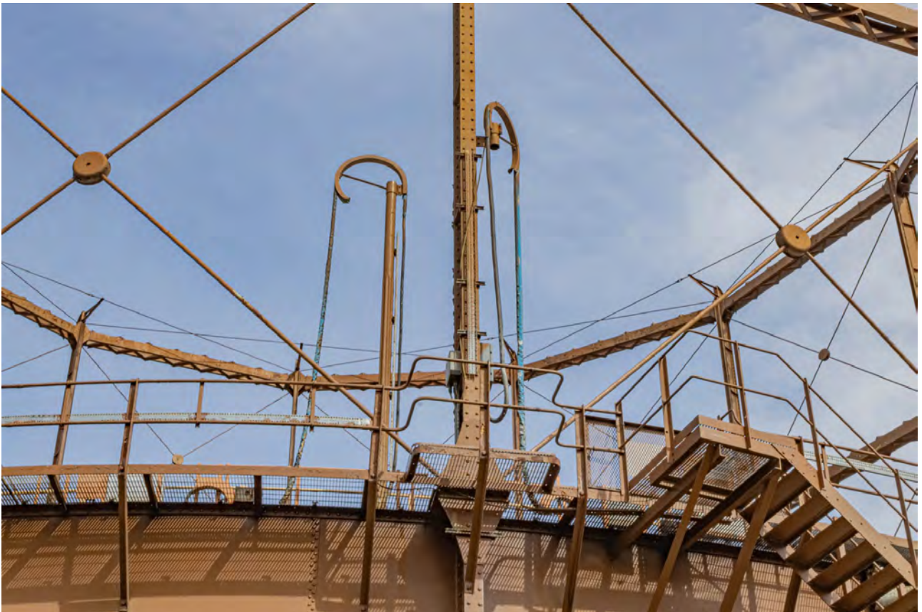
Plate 52 (BEL057): Gasholder No 2, detail of hoses on the south-west side of the gasholder above standard 9, from the south-west
