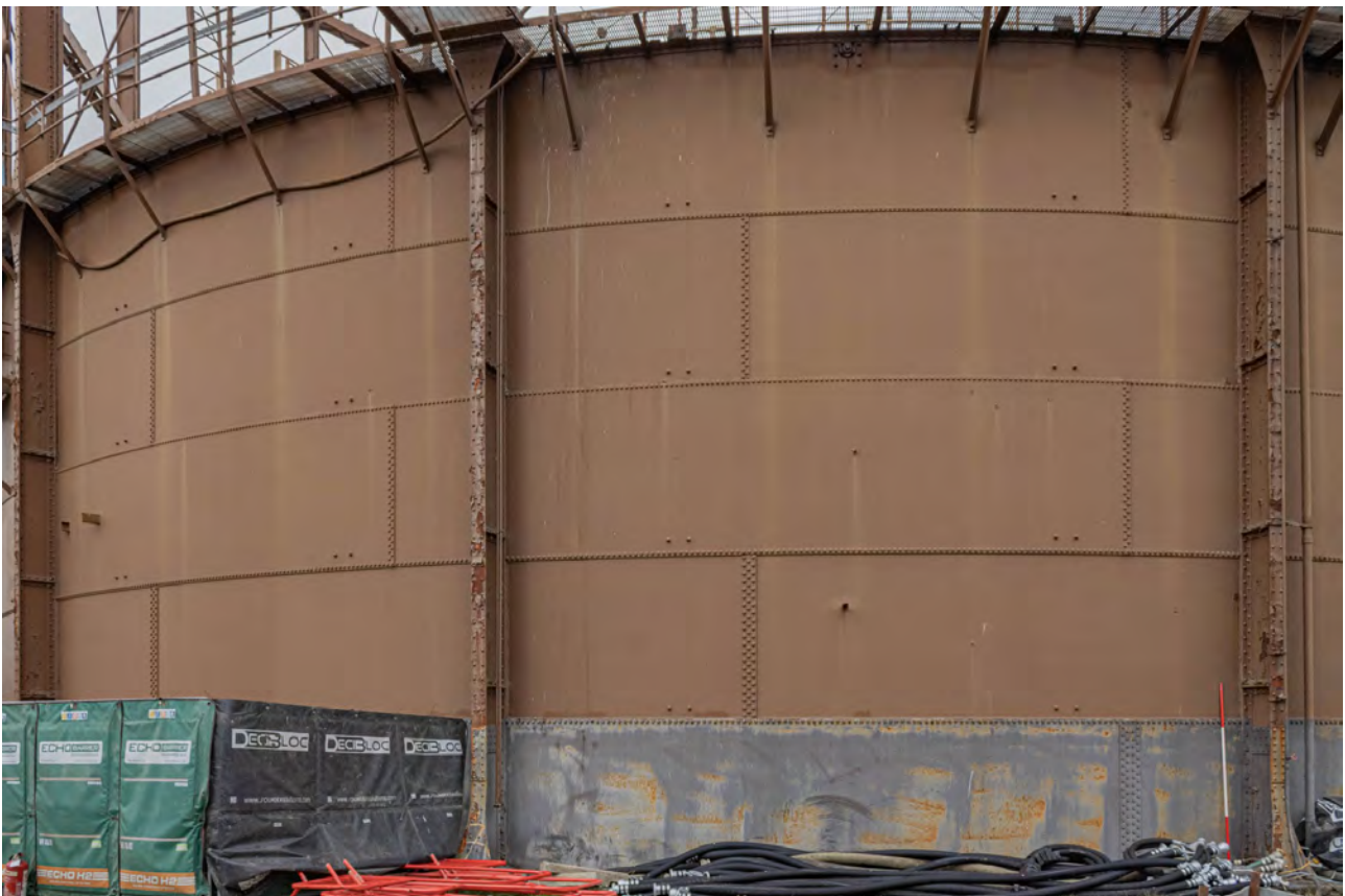
Plate 42 (BEL049): Gasholder No 2, general view of above ground tank between standards 6 and 8, from the SSE
