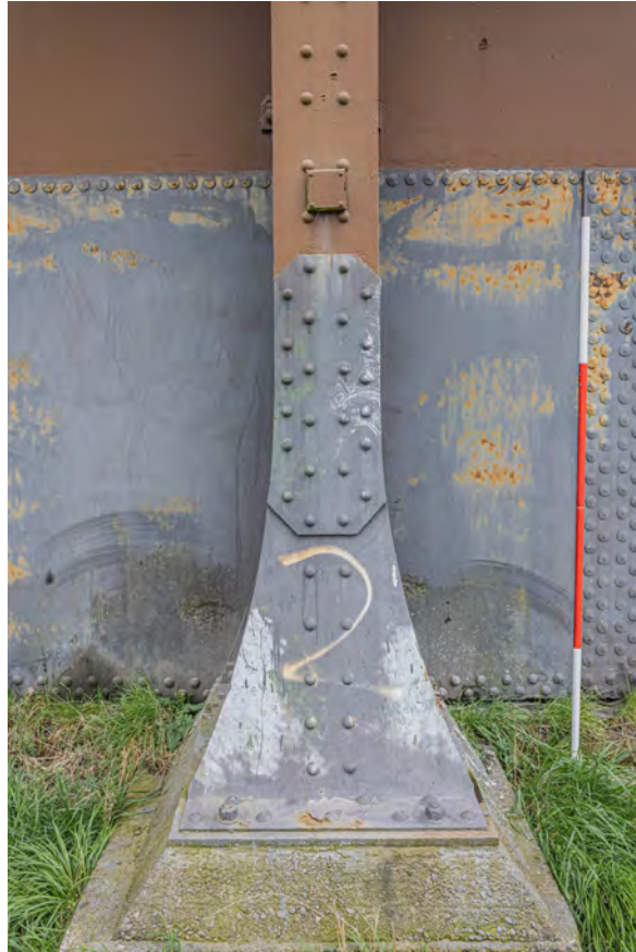
Plate 13 (BEL008): Gasholder No 1, detail of the base of standard 2 from the north-west
