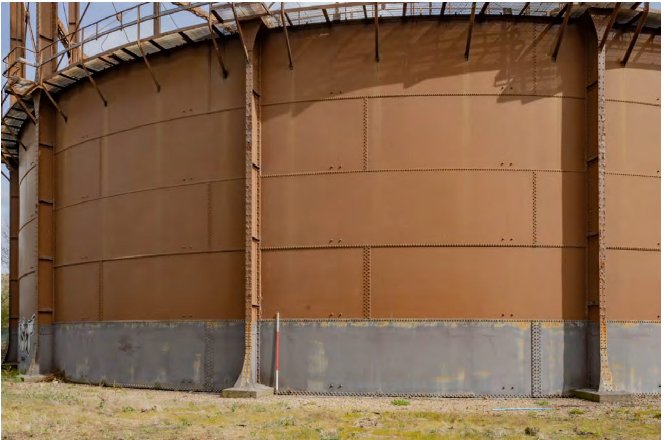
Plate 44 (BEL060): Gasholder No 2, general view of above ground tank between standards 10 and 12, from the SSW
