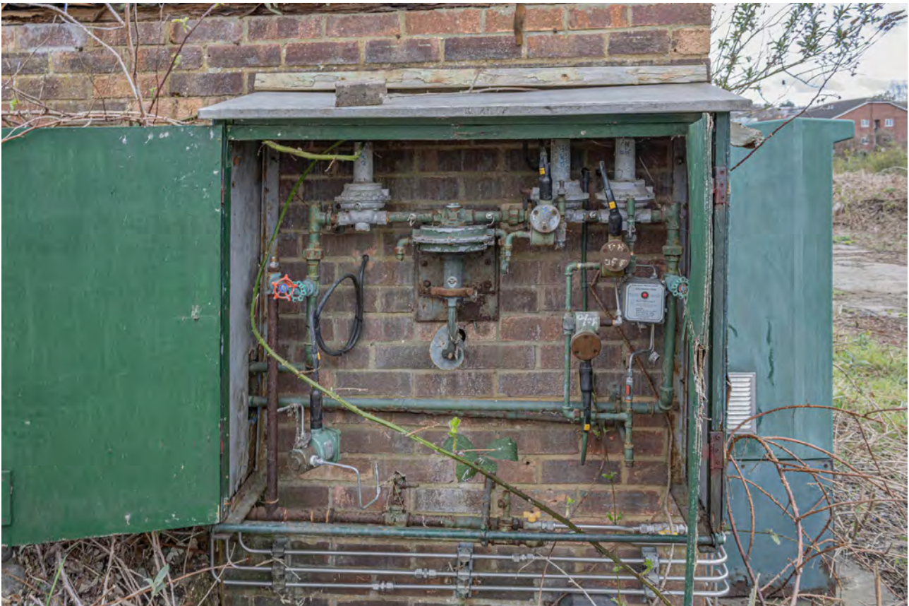
Plate 74 (BEL086): Building C, detail of cupboard on the north elevation, from the north
