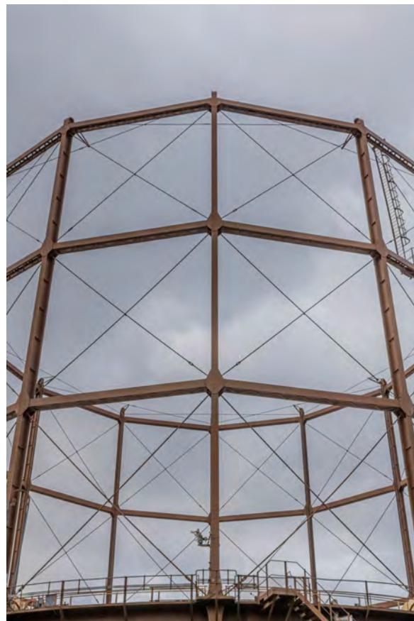
Plate 10 (BEL017): Gasholder No 1, general view of the guide framing from the north-east
