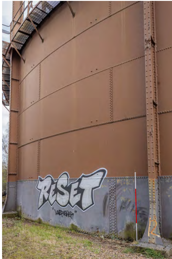
Plate 45 (BEL062): Gasholder No 2, general view of above ground tank between standards 12 and 13, from the WSW
