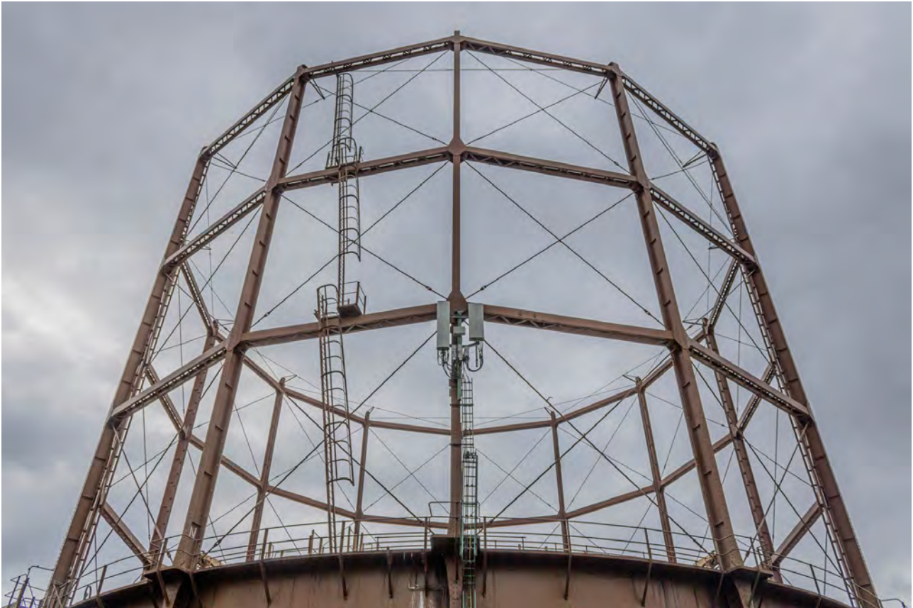
Plate 9 (BEL012): Gasholder No 1, general view of the guide framing from the north
