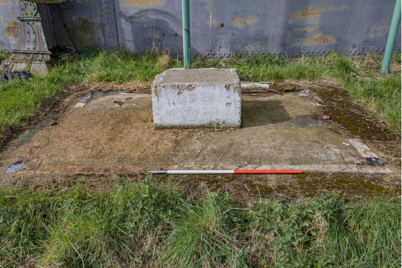
Plate 21 (BEL020): Gasholder No 1, detail of concrete platform and support for now-removed pipework between standards 6 and 7, from the north-east
