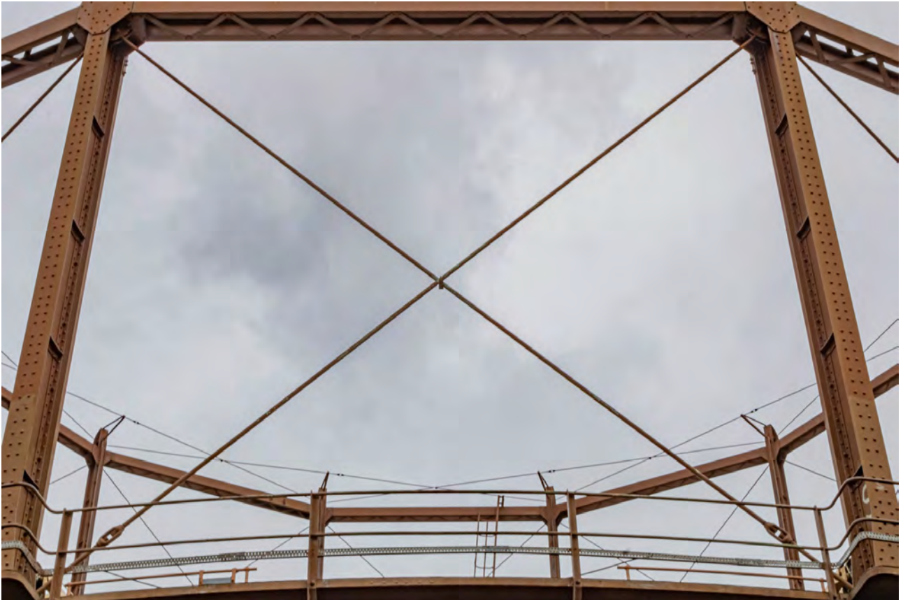
Plate 11 (BEL030): Gasholder No 1, detail of diagonal bracing of the guide framing from the south-west
