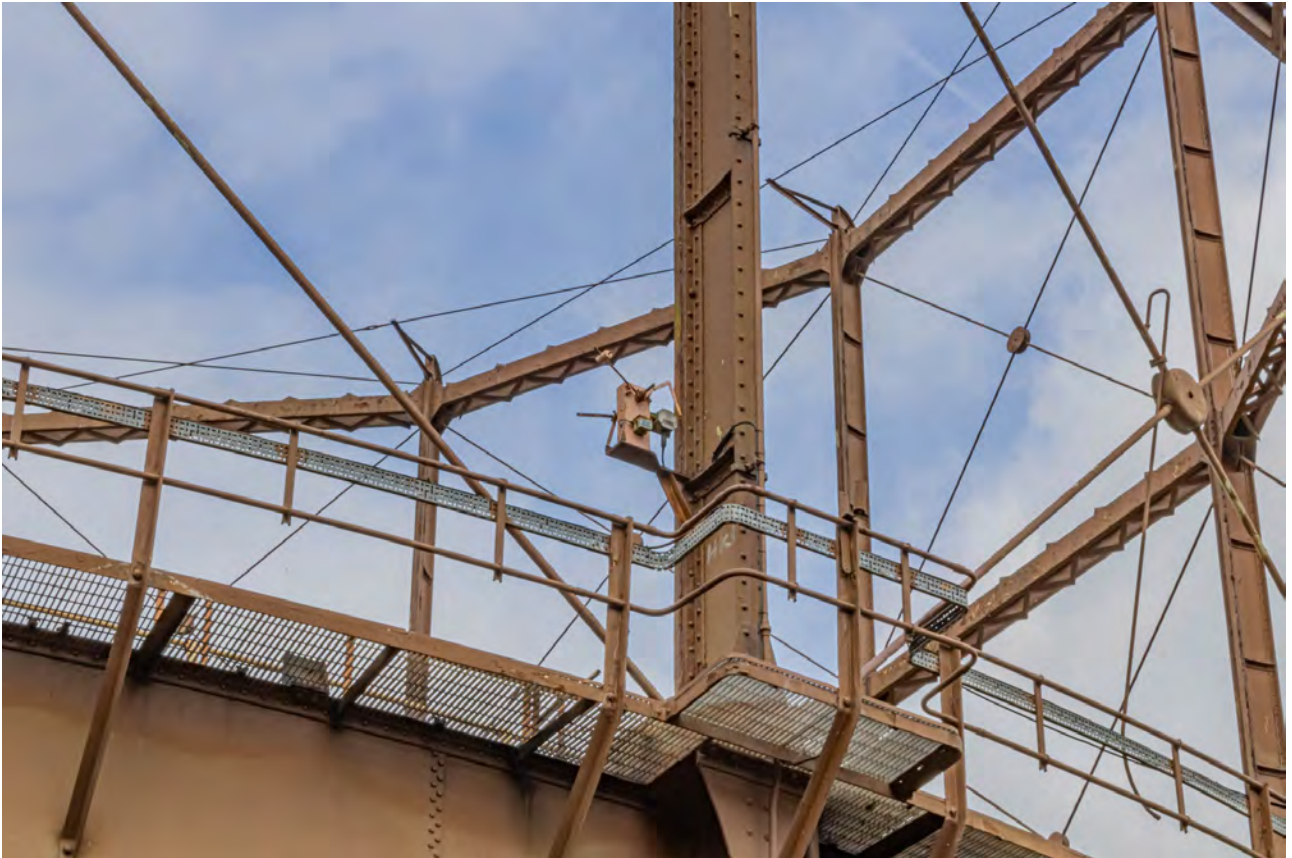
Plate 51 (BEL052): Gasholder No 2, detail of knock-off switch above standard 5 from the south-west
