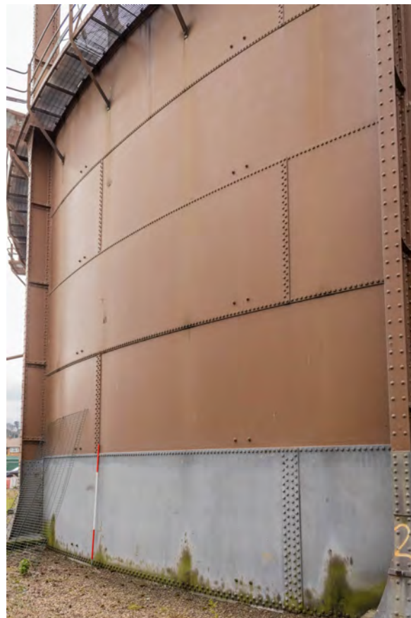
Plate 40 (BEL041): Gasholder No 2, general view of the above ground tank between standards 2 and 3, from the north
