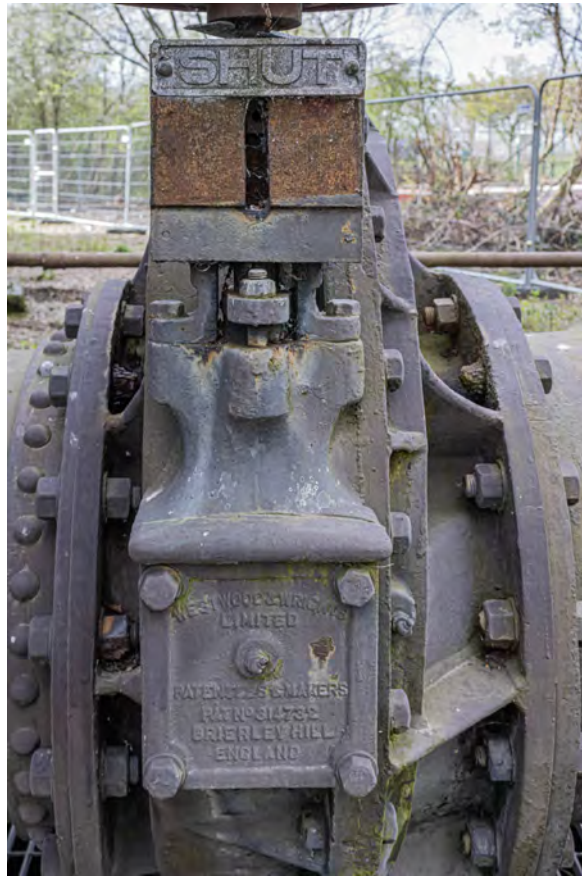
Plate 55 (BEL069): Gasholder No 2, detail of manufacturer's mark on the east side of the pipework on the north side of the gasholder, from the east
