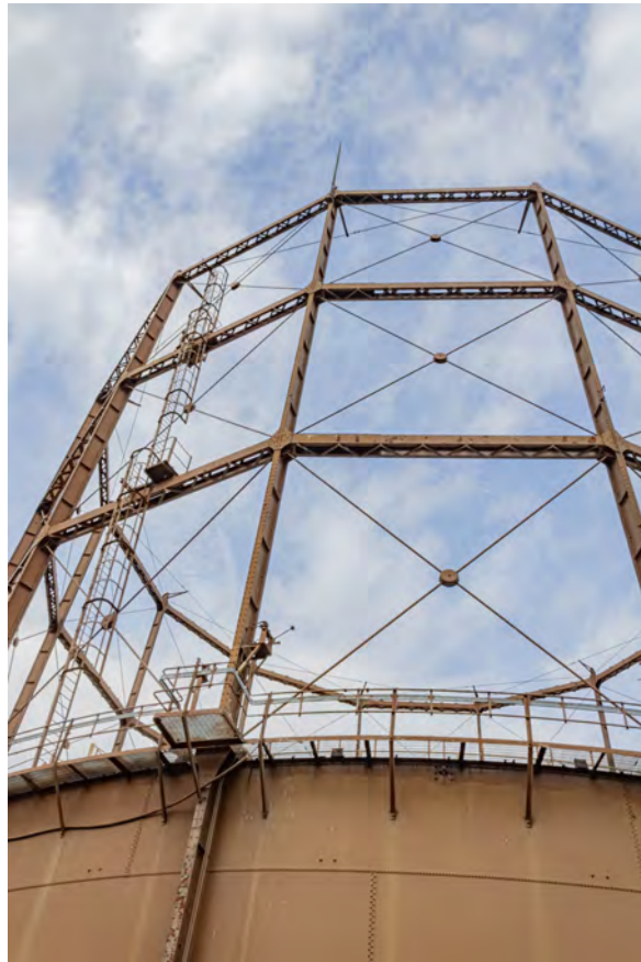
Plate 33 (BEL050): Gasholder No 2, general view of the guide frame from the SSE
