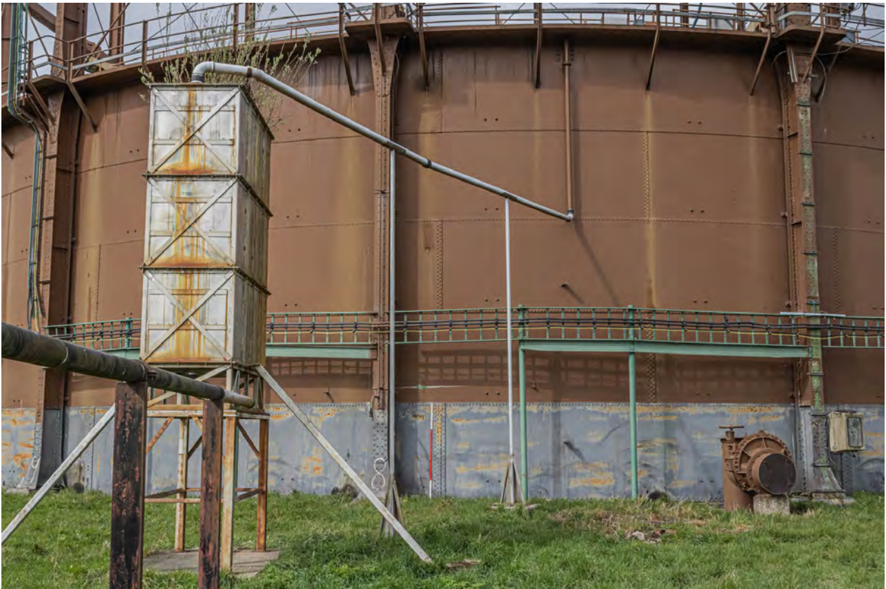
Plate 26 (BEL023): Gasholder No 1, detail of pipework and tank between standards 7 and 8, from the east
