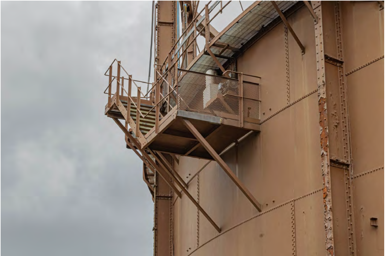
Plate 47 (BEL054): Gasholder No 2, detail of upper stair to the SSW of the gasholder, from the south-east
