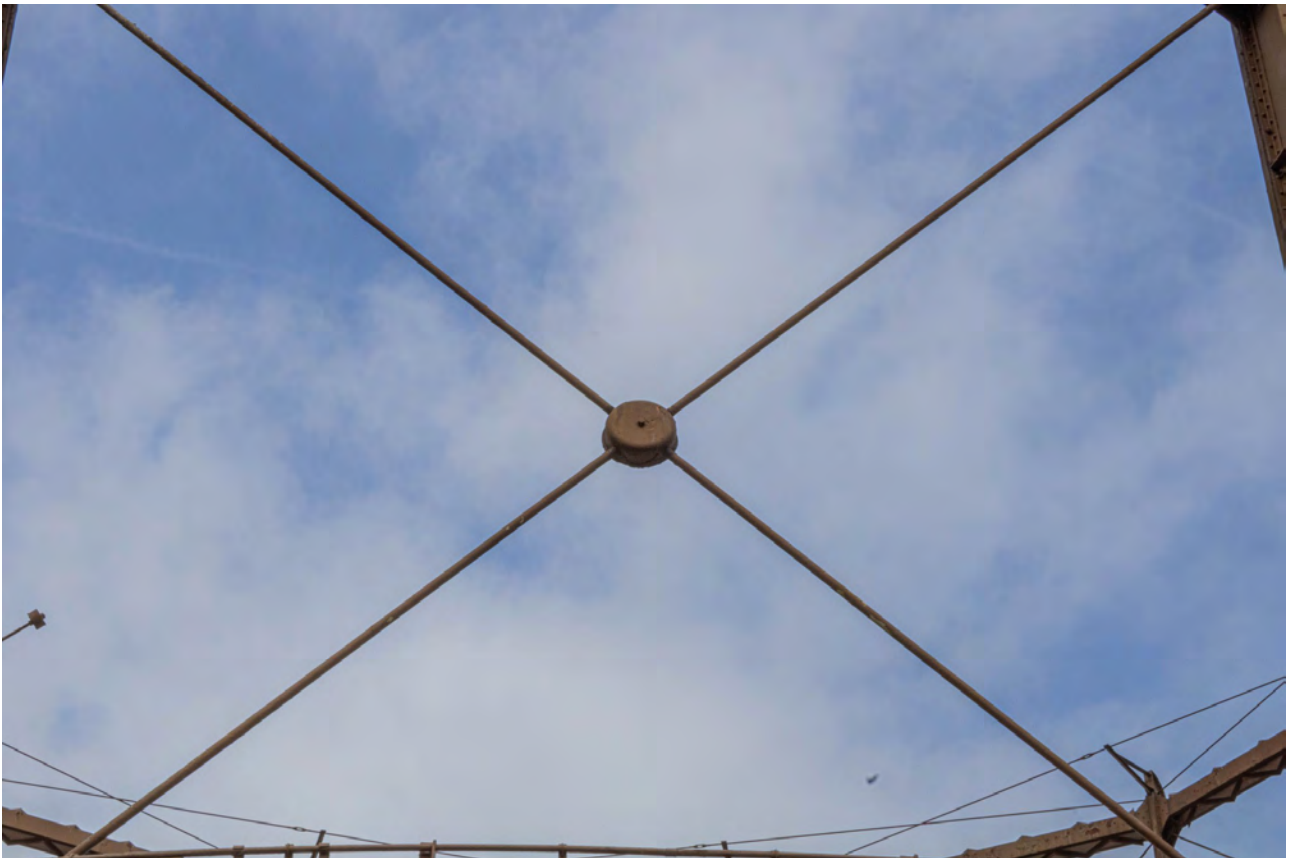
Plate 34 (BEL053): Gasholder No 2, detail of the diagonal bracing of the guide frame, from the south
