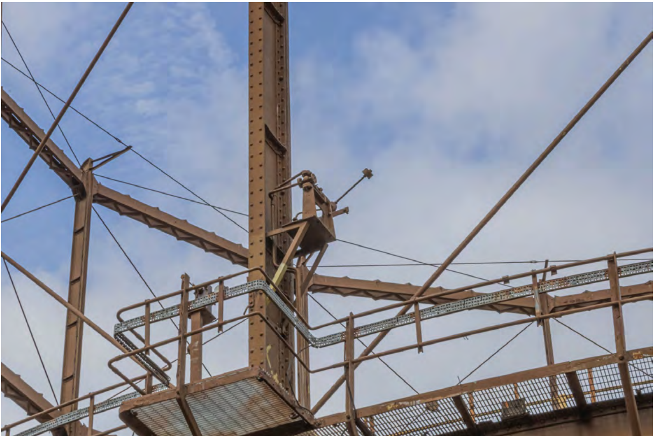
Plate 50 (BEL051): Gasholder No 2, detail of knock-off switch above standard 8, from the south-east
