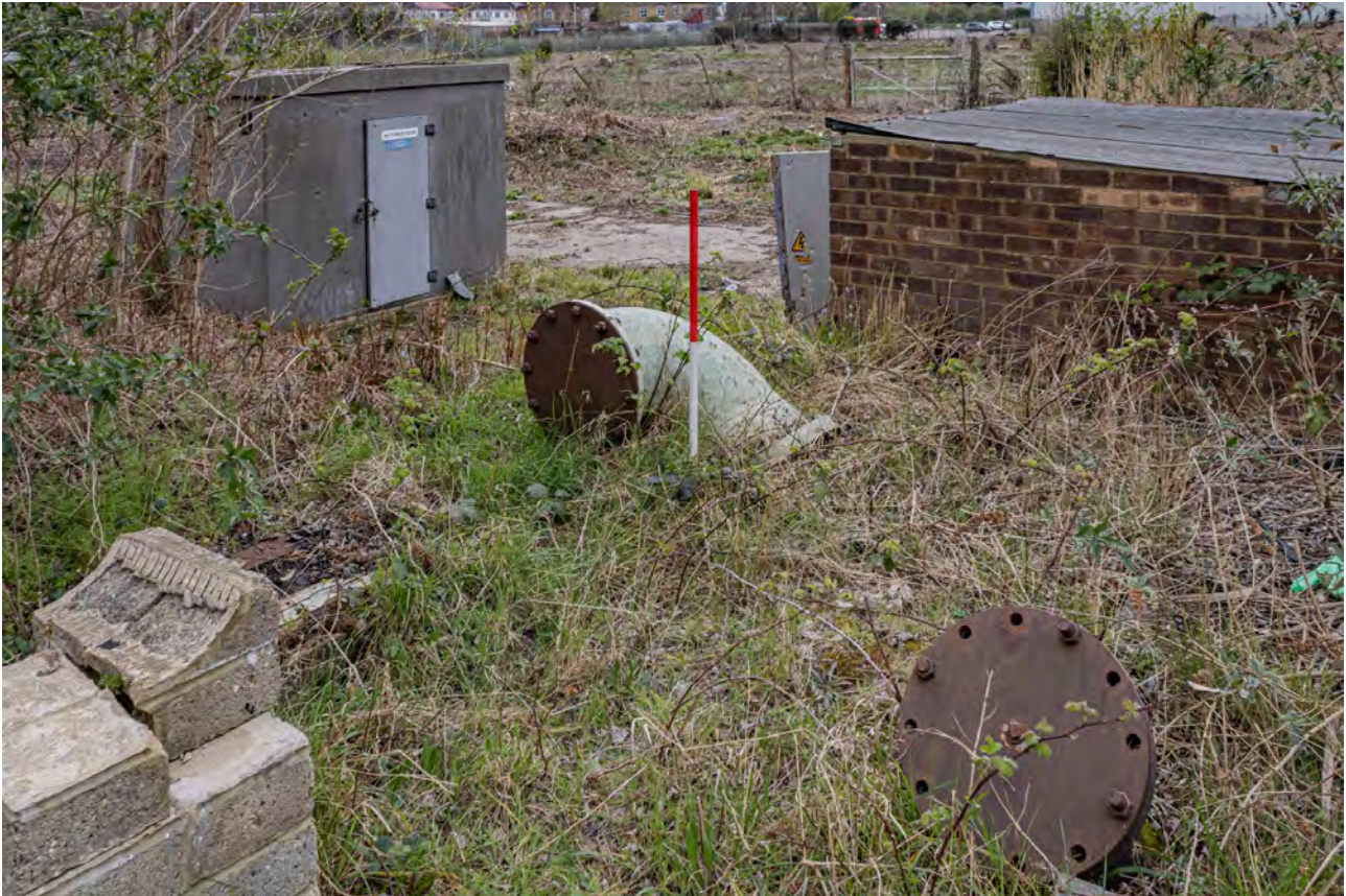
Plate 71 (BEL083): Detail of pipework from the north-east
