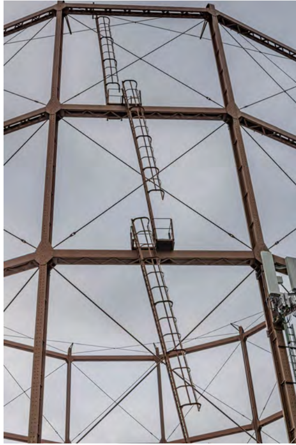
Plate 19 (BEL014): Gasholder No 1, detail of sequence of stairs for upper lifts, from the north
