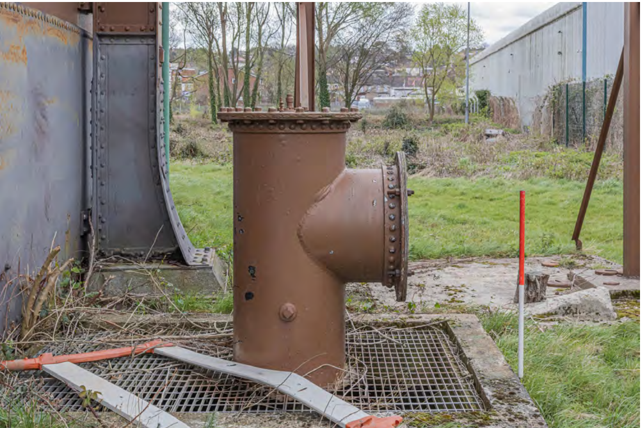
Plate 30 (BEL034): Gasholder No 1, detail of pipework between standards 1 and 14 from the north
