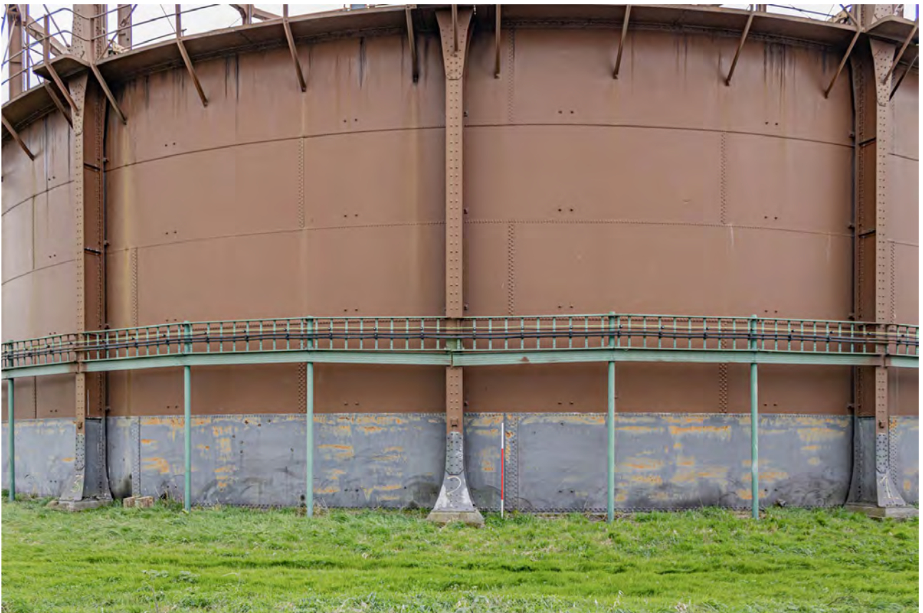
Plate 12 (BEL005): Gasholder No 1, general view of the north-west side of the gasholder and standard 2, from the north-west
