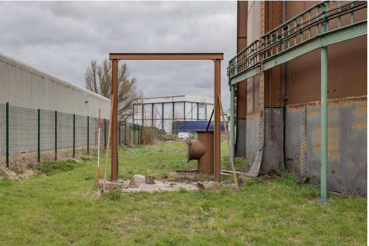
Plate 29 (BEL035): Gasholder No 1, detail of pipework and frame between standards 1 and 14 from the SSE
