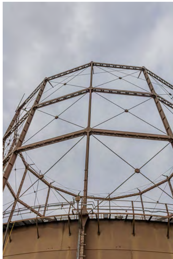
Plate 32 (BEL047): Gasholder No 2, general view of the guide frame from the south-east
