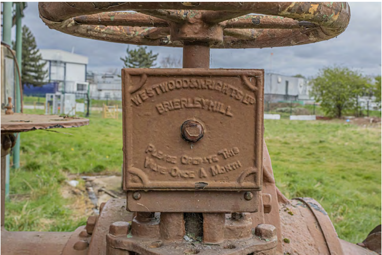
Plate 24 (BEL036): Gasholder No 1, detail of manufacturer's plaque on the pipework between standards 7 and 8 from the south
