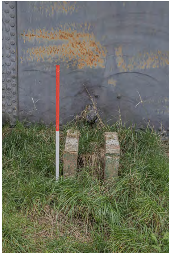
Plate 20 (BEL010): Gasholder No 1, detail of concrete support for now-removed pipework between standards 2 and 3, from the north-west
