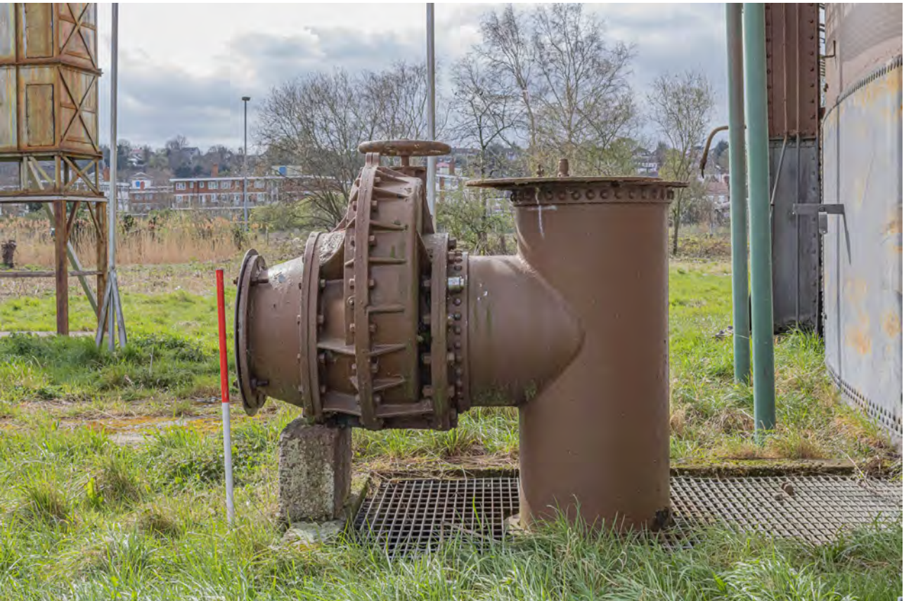
Plate 22 (BEL018): Gasholder No 1, detail of pipework between standards 7 and 8 from the north
