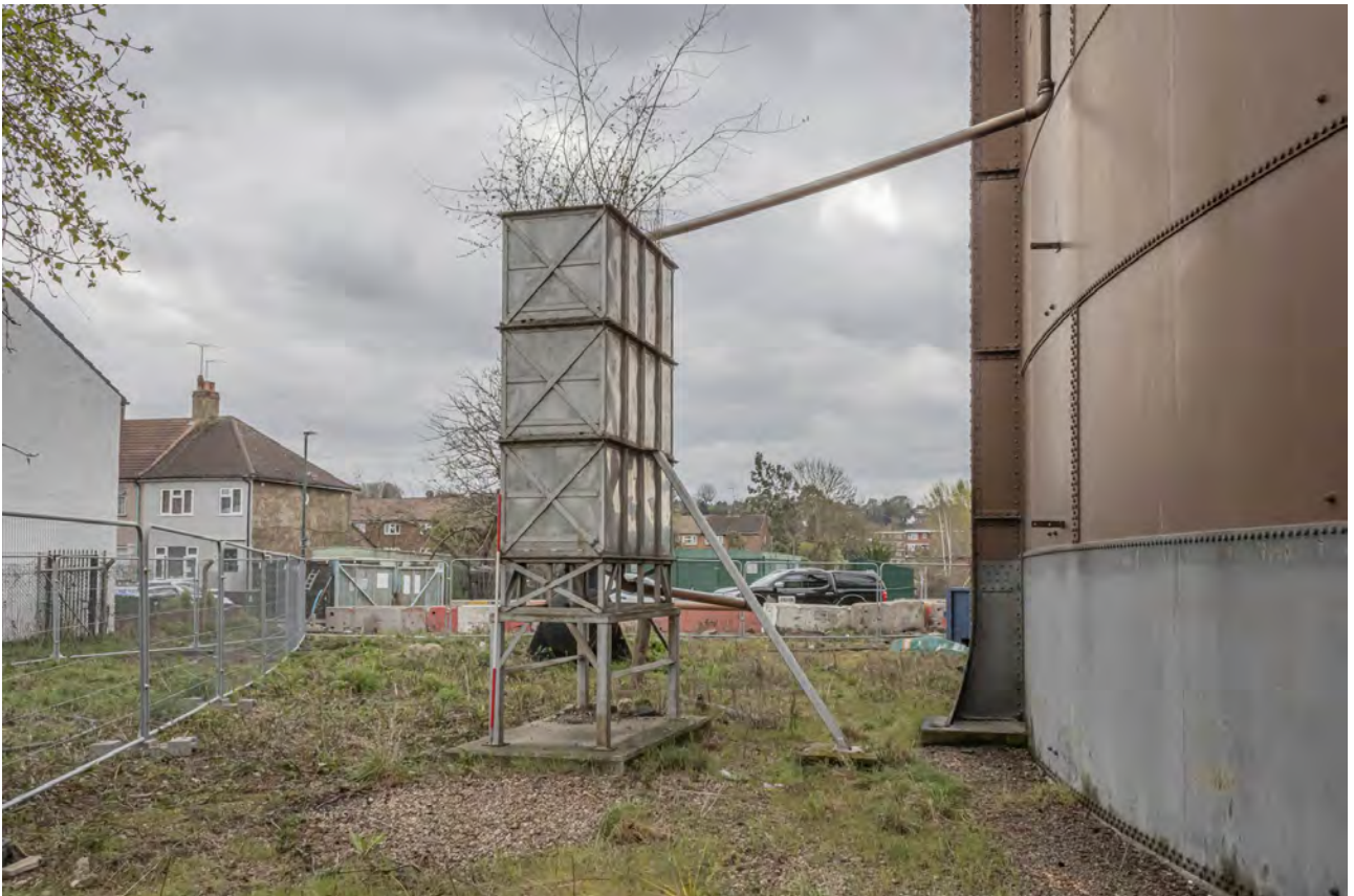
Plate 48 (BEL043): Gasholder No 2, detail of tank on the east side of the gasholder, from the north
