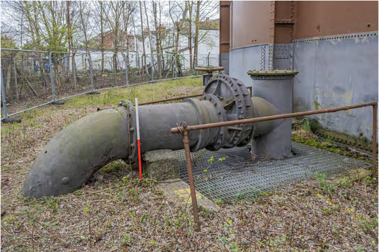
Plate 53 (BEL066): Gasholder No 2, detail of pipework on the north side of the gasholder, from the WNW
