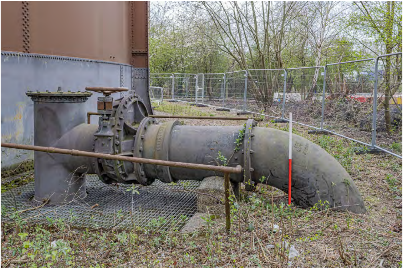
Plate 54 (BEL068): Gasholder No 2, detail of pipework on the north side of the gasholder, from the east
