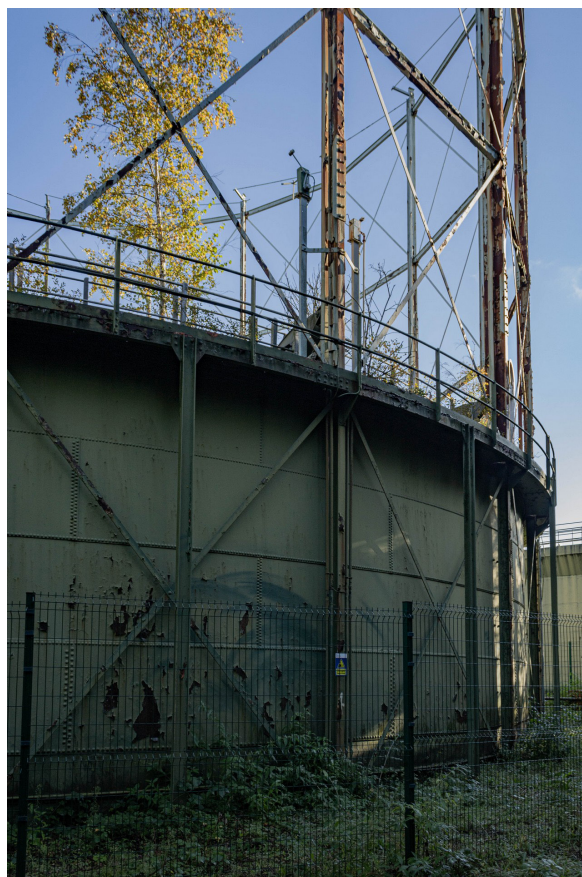
Plate 8: Gasholder No 3, general view at the location of Standard 4 (note the two knock-off switches to either side of the standard), from the west
