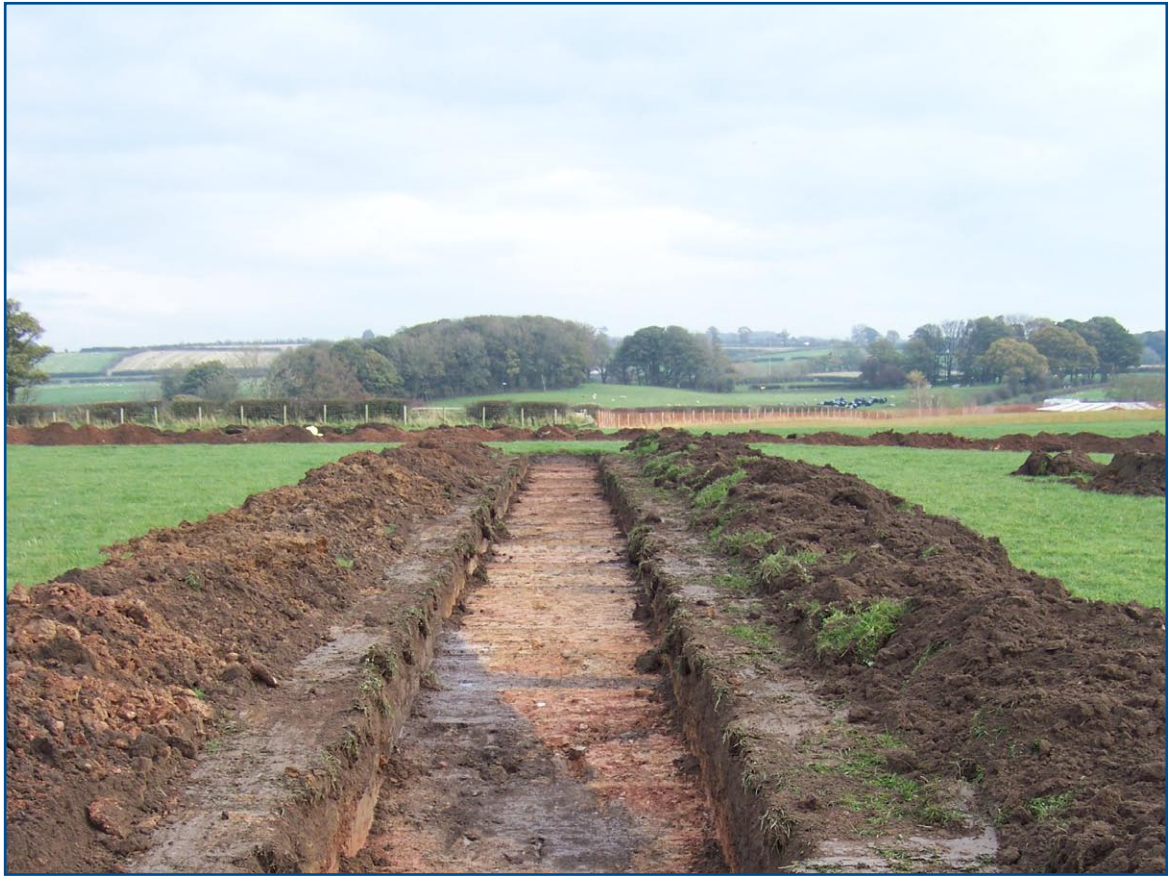
Plate 7: Modern drainage channel [1704] which truncates 19th-20th century field drains, from the west
