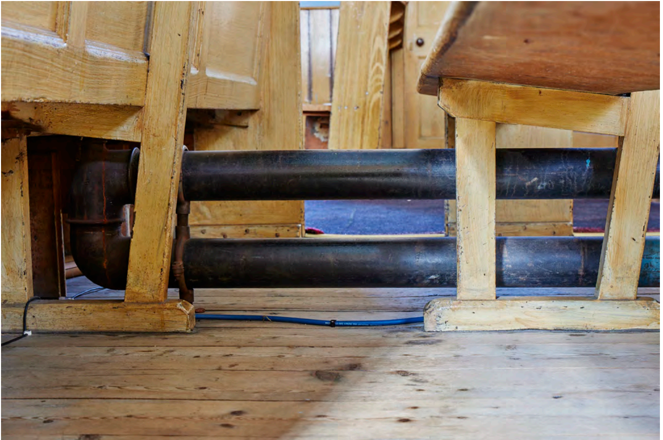
Plate 41: Cockenzie Old Parish Church, Room 1, detail of heating pipe beneath the pews
