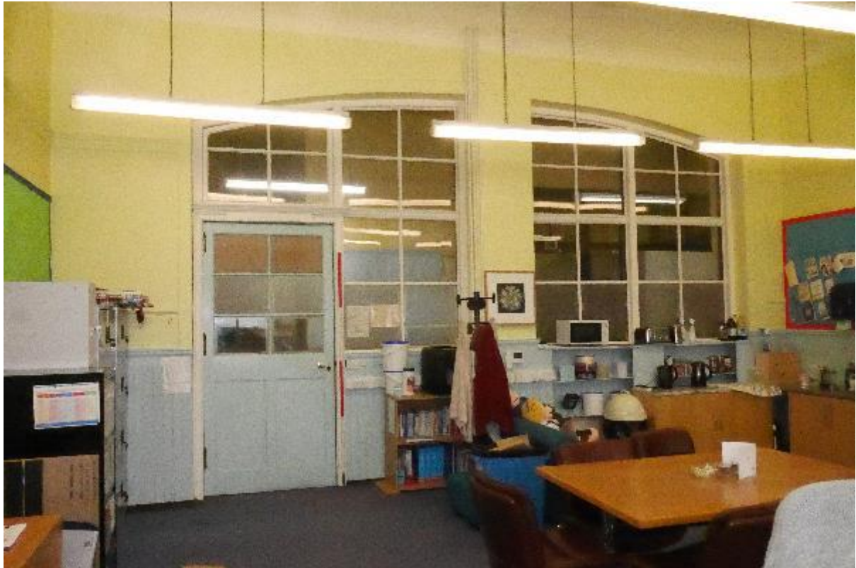
Illustration 85- Internal West facing elevation of Classroom (19) showing low arched glazed windows, doorway and half-timbered planked wall.
