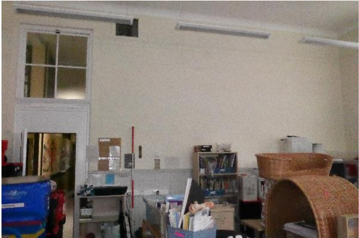
Illustration 60 - Internal South facing elevation of Classroom (13) showing doorway with glazed window above and half-timbered panelling on wall.
