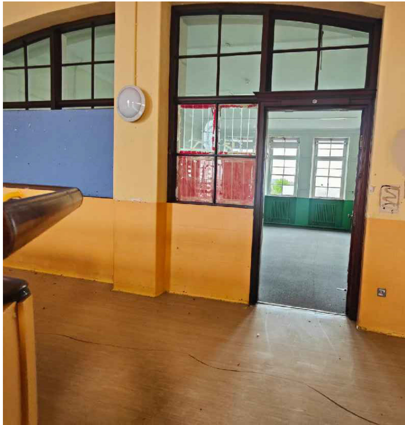
Plate 91: General view of entrance to Room 1/7 from Room 1/5, looking north-east (© Trail Architects 2024)
