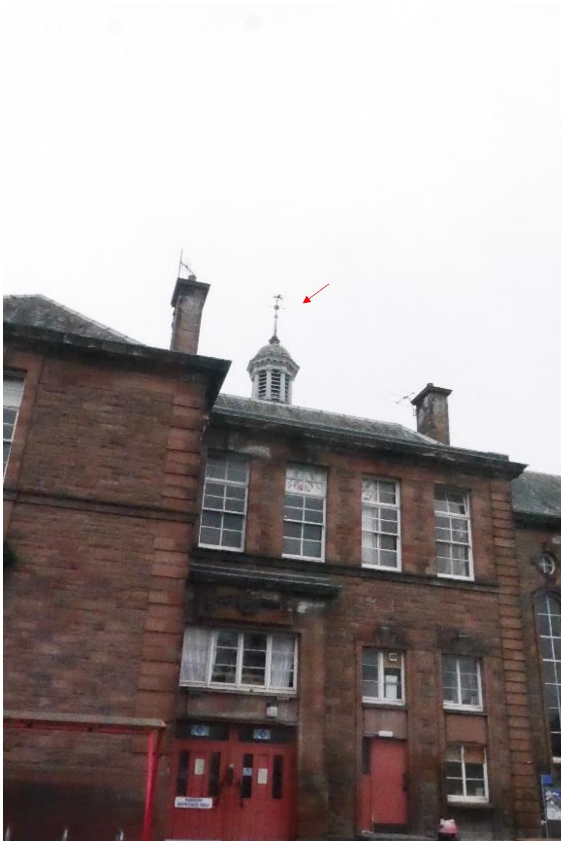
Illustration 126 – Roof ventilator at Eastern end of building, red arrow indicates weather van in the shape of a dragon.
