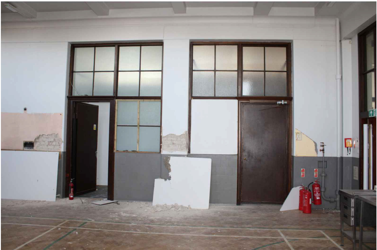
Plate 58: Detailed view of doors accessing Rooms 0/10 and 0/12 from Room 0/9, looking south-east (© Trail Architects 2024)
