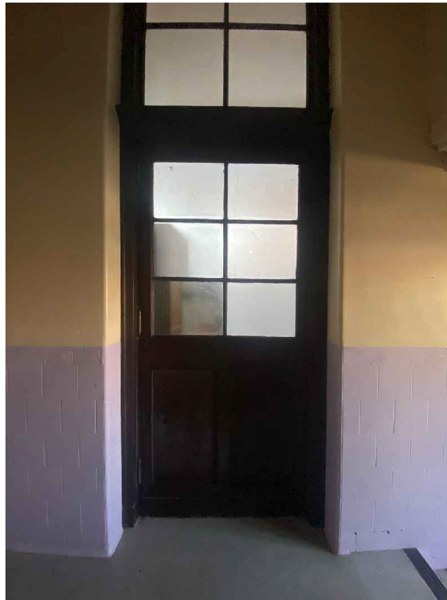
Plate 33: Detailed view of west door leading into Room 0/2, looking south-east (© Trail Architects 2024)
