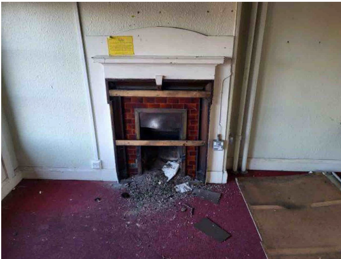
Plate 78: Detailed view of fireplace located on the north-east wall of Room M8 (© Graham & Sibbald 2025)
