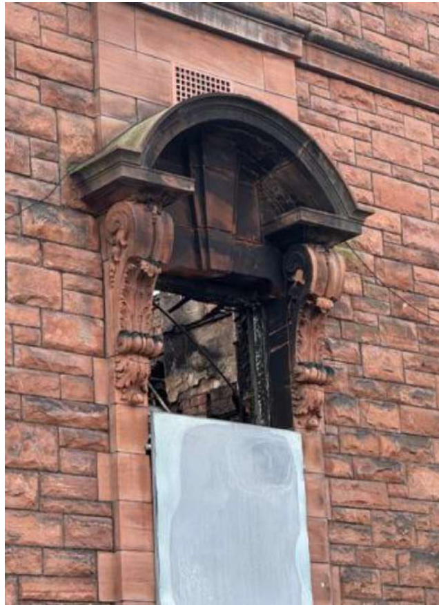
Plate 7: Detailed view of open segmental arched window in Bay 5 of the north-west facing elevation (© Perth and Kinross Council 2025b)
