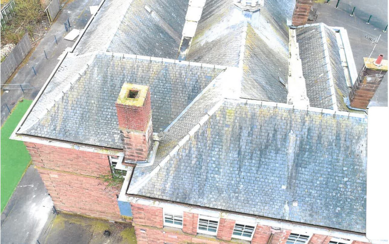
Plate 23: General view of the roof detailing towards the eastern extent of the building, looking WSW (© Conservation Masonry Ltd 2025)
