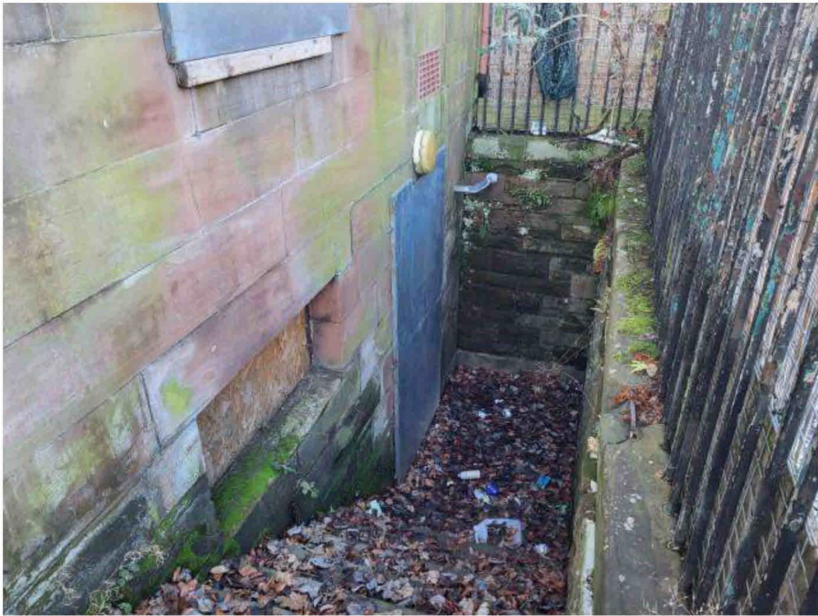
Plate 21: General view of the north-east elevation showing sets to basement, looking north-west (© G3 Consulting Engineers 2025)
