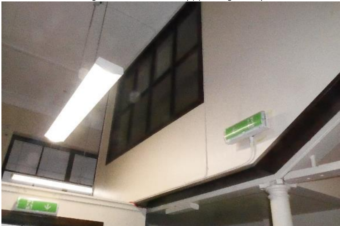
Illustration 31- Timber framed frosted glass window in elevation of stairs to Mezzanine floor (Upper section of South facing internal elevation of Lobby (5)).
