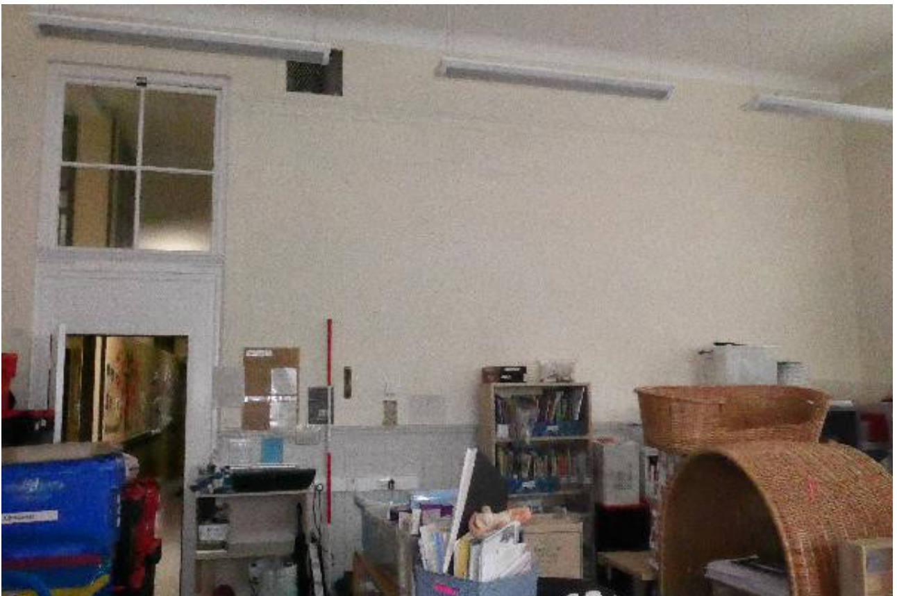
Plate 64: General view of the north-west wall in Room 0/17, looking north-west (© Derek Hall 2023)
