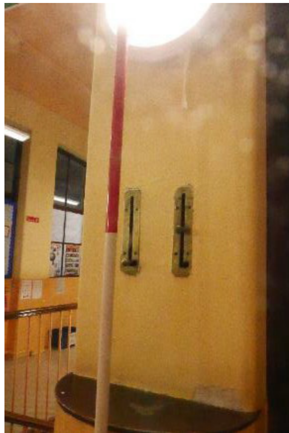
Plate 26: Detail of brass ventilation controls in Room 1/5 (© Derek Hall 2023)
