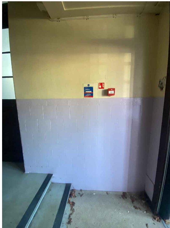
Plate 32: General view of south-east wall of porch area in Room 0/1 showing access steps (© Trail Architects 2024)
