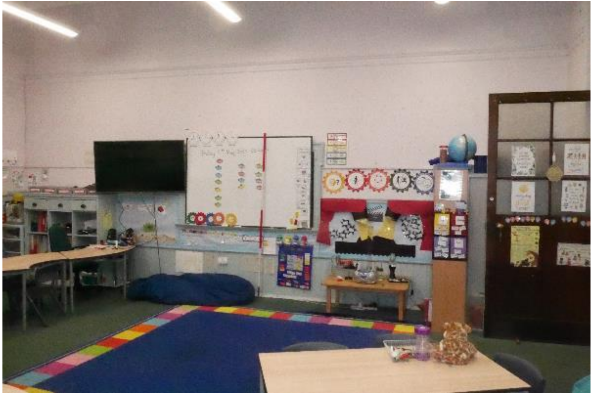
Illustration 96- Internal East facing elevation of Classroom (23) showing original black board behind whiteboard and half-timbered panelling.
