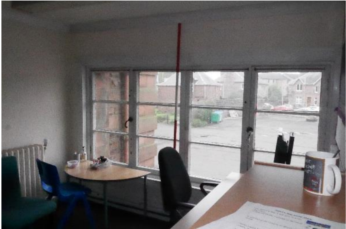
Illustration 75- Internal South facing elevation of the School Office (d) showing glazed windows.
