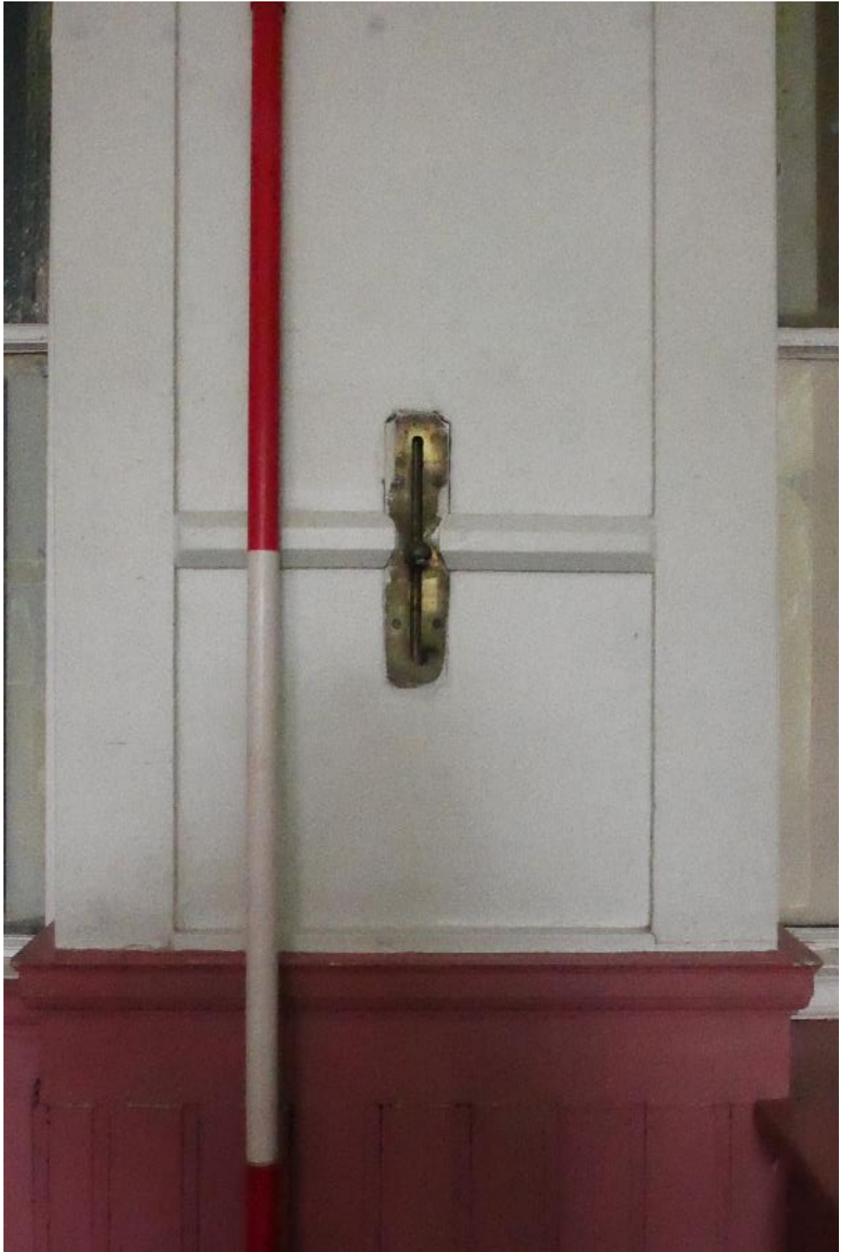
Illustration 37- Ventilation control (brass) in internal South facing elevation of Staff Room (6).
