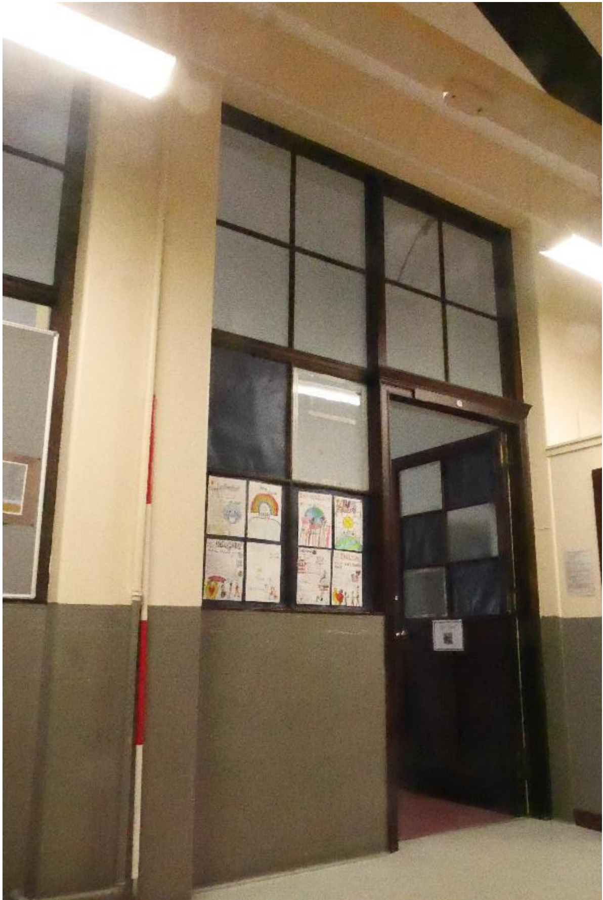
Illustration 29- Doorway into Staff Room (6) showing timber framed frosted glass windows in elevation.
