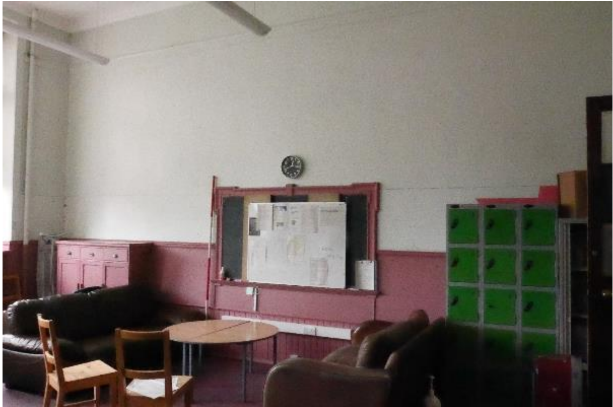
Illustration 33 - East facing internal elevation of Staff Room (6) showing original half-timbered panelling, blackboard and cupboard with drawers.
