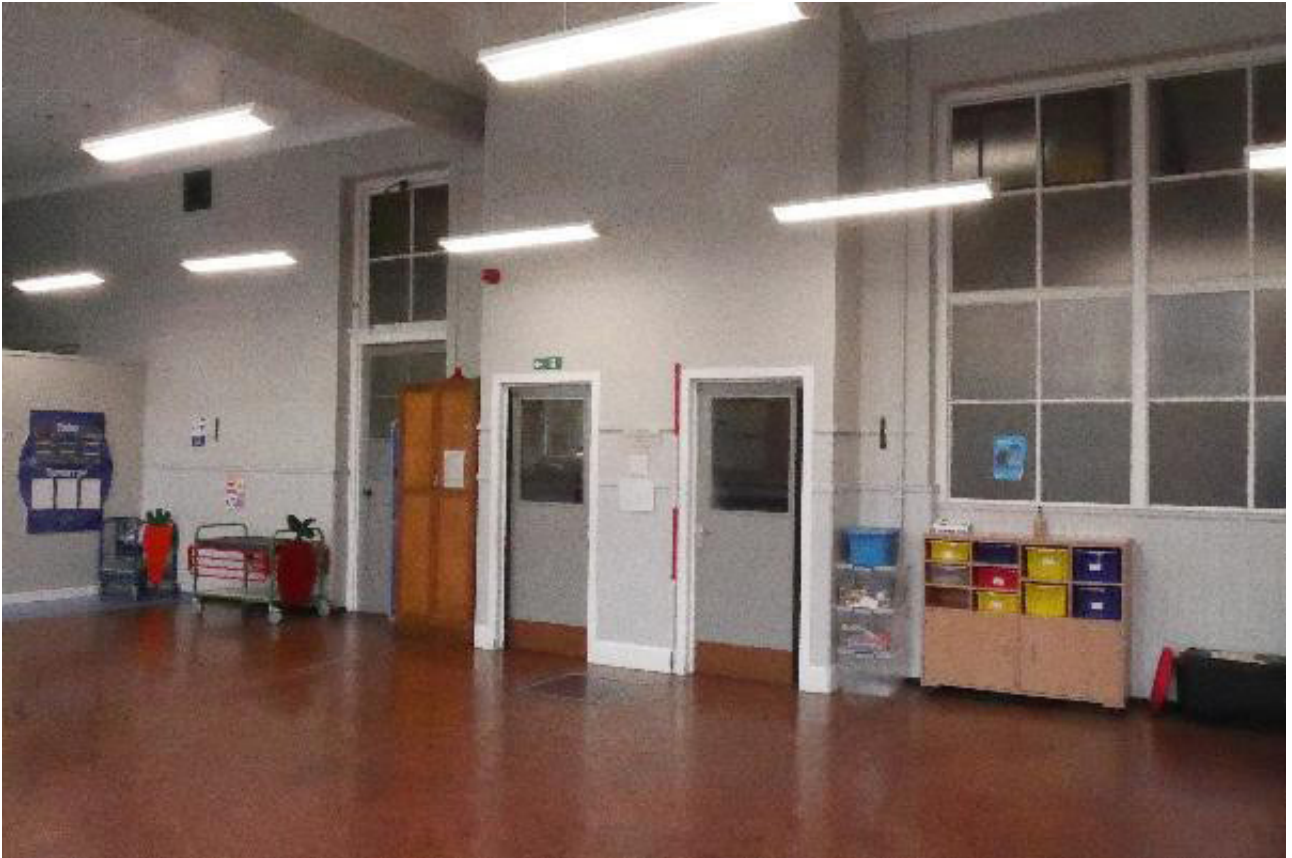
Plate 41: General view of the north-east wall of Room 0/2, looking NNE (© Derek Hall 2023)
