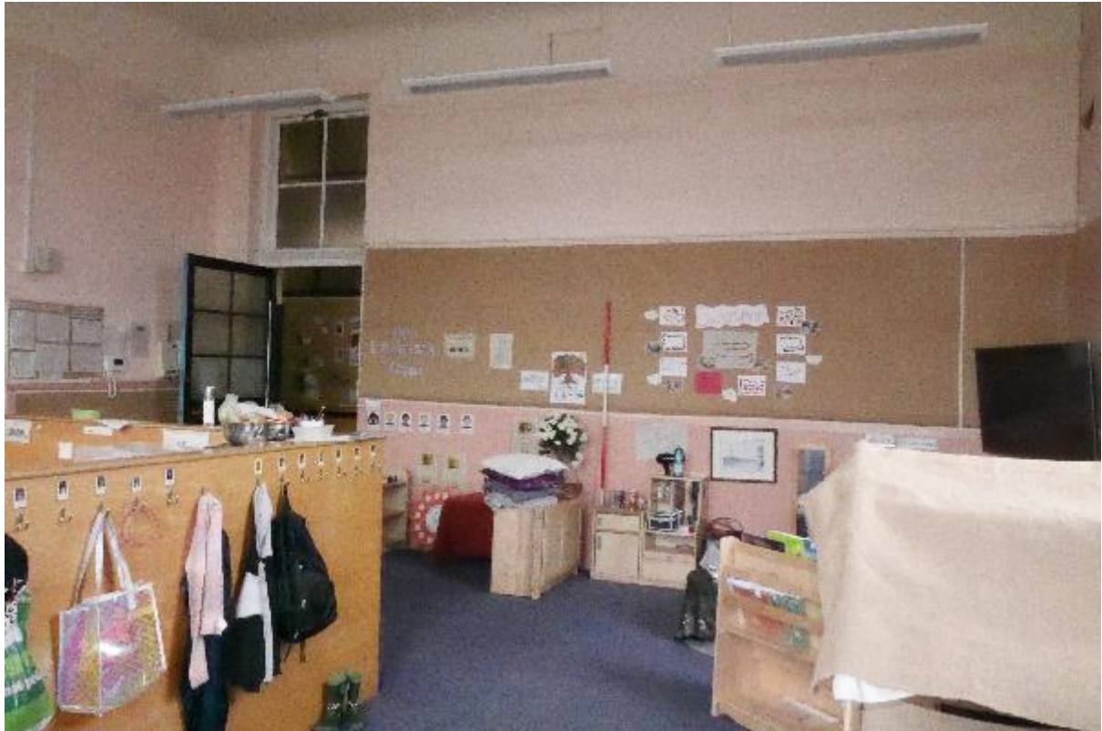
Illustration 68- Internal East facing elevation of Classroom (15) showing doorway with glazed window above and half-timbered panelling on wall.
