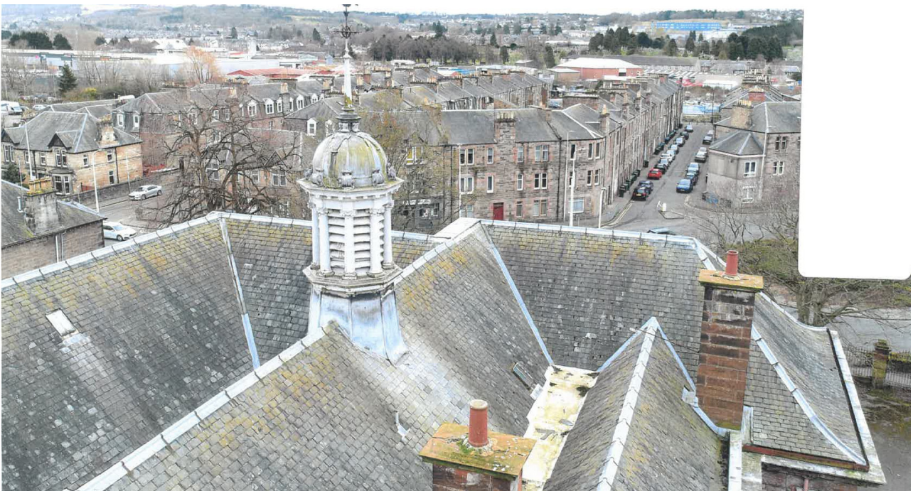
Plate 12: General view of the roof detailing toward the western extent of the building, looking WSW (© Conservation Masonry Ltd 2025)
