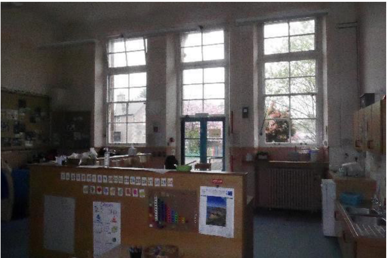
Plate 68: General view of north-east wall in Room 0/19 showing inserted double door, looking north (© Derek Hall 2023)
