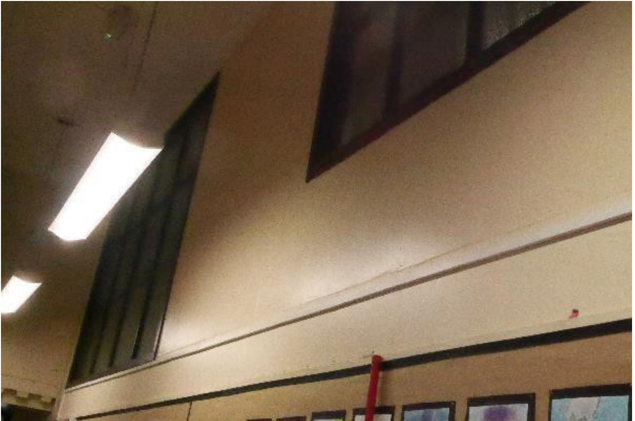
Plate 37: General view of windows on the north-east wall of Room 0/1 (© Derek Hall 2023)
