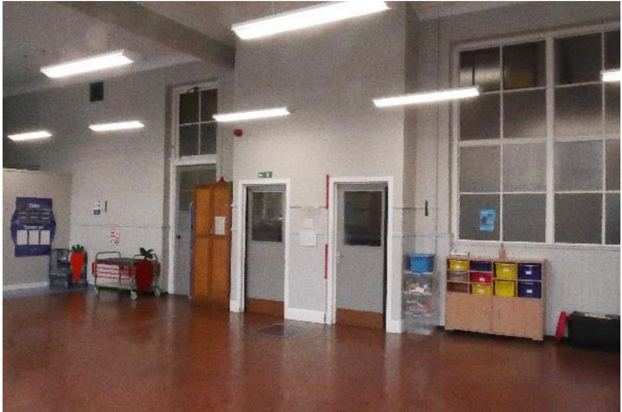
Illustration 22- Internal West facing elevation of Dining Room (2) showing entrance doors and frosted glass panelling.
