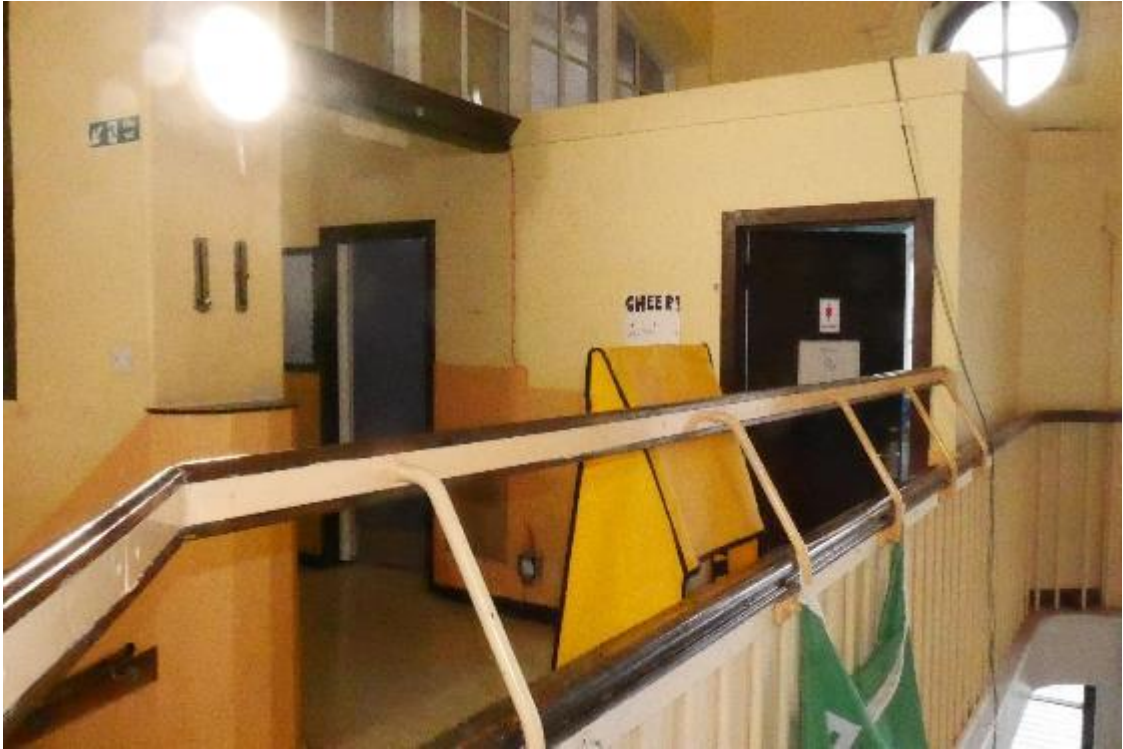
Illustration 90 - Access to lobby (21) showing entrance to toilets and first aid room. Red arrow indicates ventilation controls.
