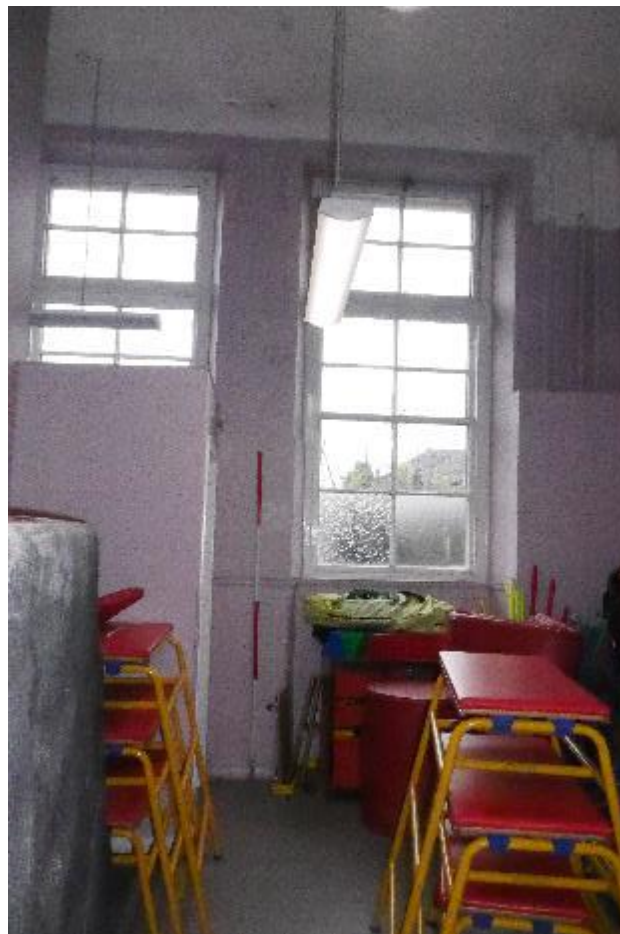
Illustration 44- Internal North facing elevation of Store (8) showing glazed windows and half-timber panelling.
