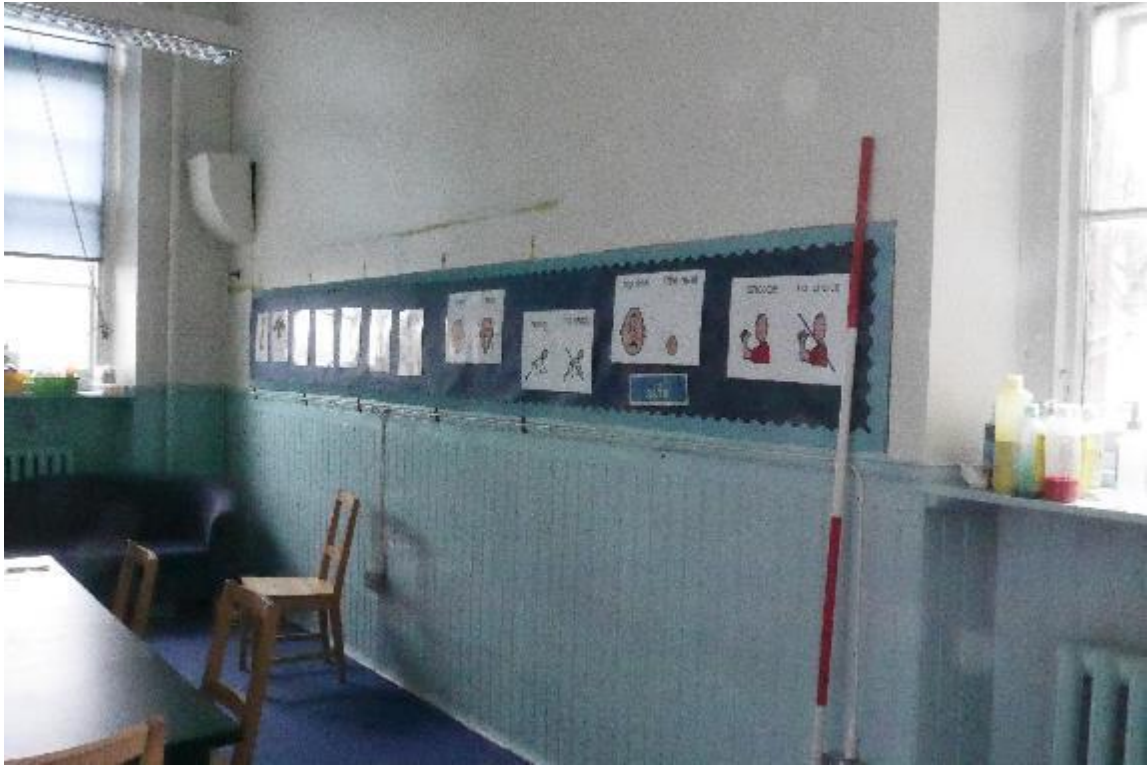
Illustration 26- Internal East facing elevation of Meeting Room (4) showing original half panelled wall.
