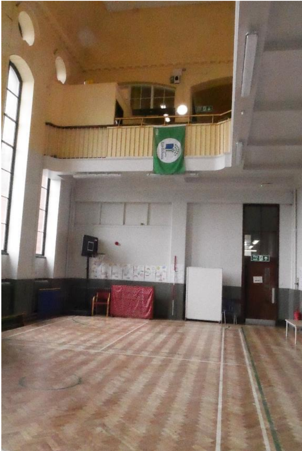
Illustration 38- Hall (7) looking East showing balustrade at upper floor level, parquet floor and doorway into Lobby (11). Moulding at start of ceiling vault and Eastern end of arched and circular windows in South facing internal elevation are also visible.
