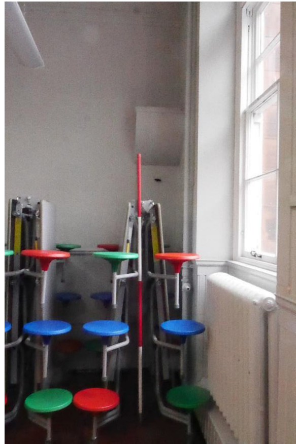
Plate 25: Control and part of ventilation system in south-western corner of Room 0/2 (© Derek Hall 2023)
