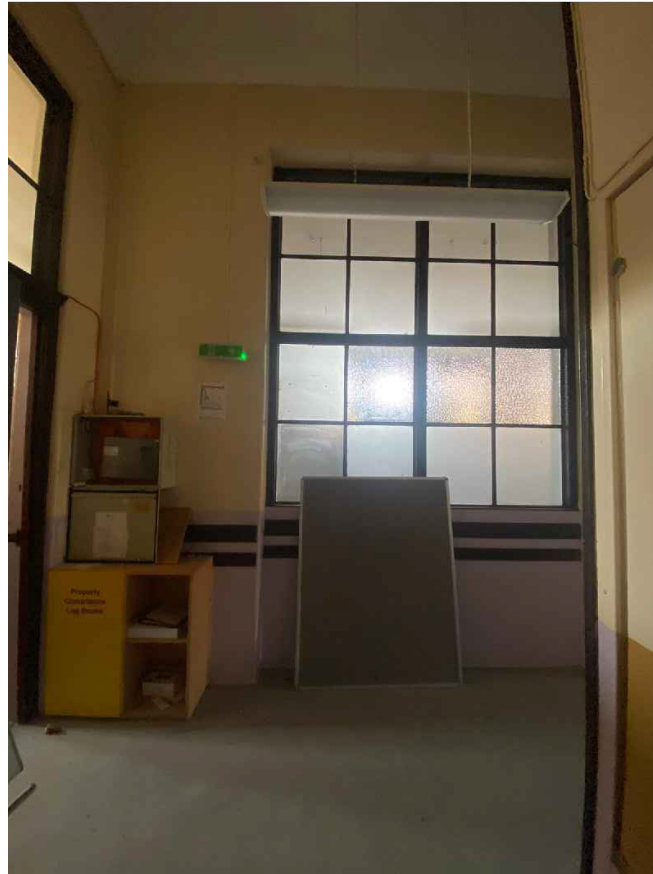
Plate 35: Detailed view of original classroom window for Room 0/2, looking south-east (© Trail Architects 2024)
