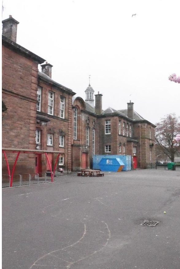
Illustration 5- North facing external elevation of Balhousie Primary School, top looking South East bottom looking South West (2023).
