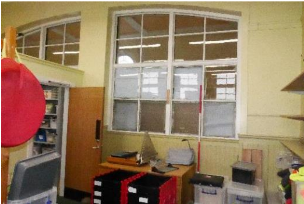
Illustration 105- Internal South facing elevation of Classroom (25) showing low arched windows and half-timbered planked wall.
