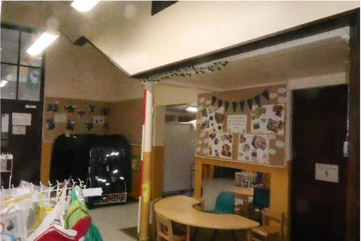
Illustration 51- Internal South facing elevation of Lobby (11) showing bottom of stairs to Mezzanine floor and doorways into store and toilet.
