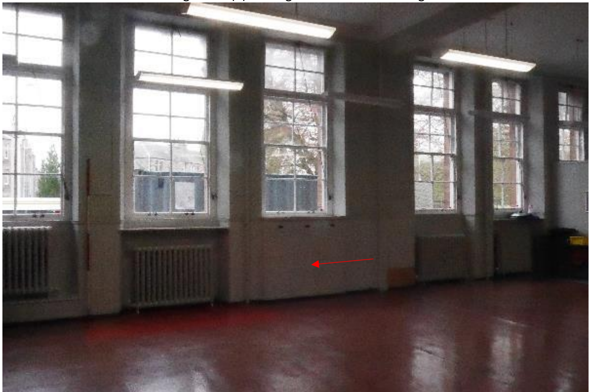
Illustration 19- Windows in East facing internal elevation of Dining Room (2), built in cupboards at red arrow (see next Illustration).
