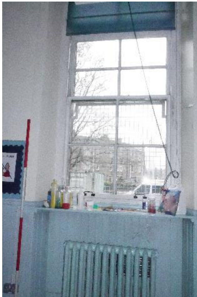
Illustration 27- Glazed window with shelf and radiator below in internal South facing elevation of Meeting Room (4).
