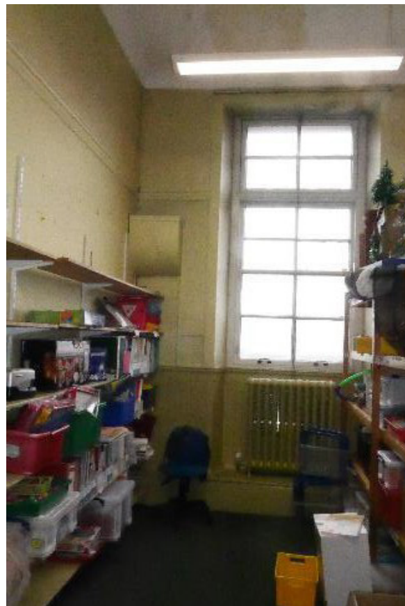
Plate 94: Detailed view of the north window in Room 1/8 showing adjacent ventilation system, looking south-east (© Derek Hall 2023)
