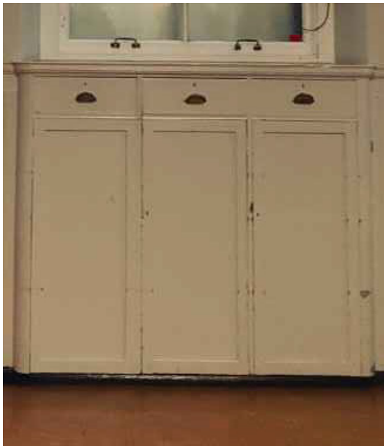
Plate 40: Detailed view of inbuilt cupboards in the south-west wall of Room 0/2 (© Trail Architects 2024)
