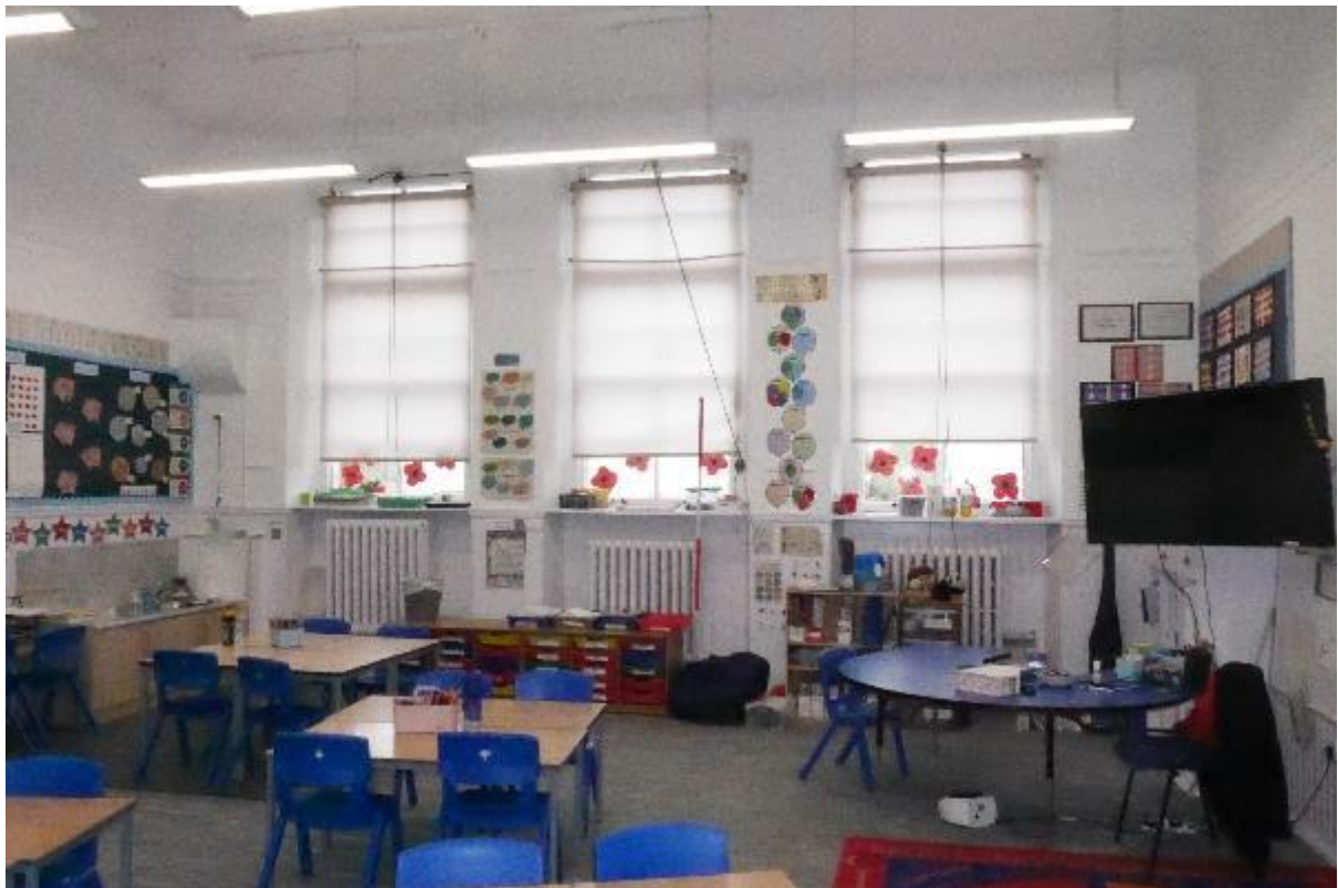
Illustration 115- Internal West facing elevation of Classroom (28) showing glazed windows and half-timbered planked wall.
