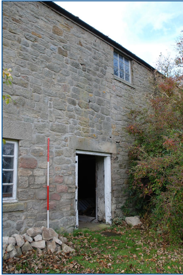
Plate 17: Detail of central door and edge of blocked door in east elevation of barn from east
