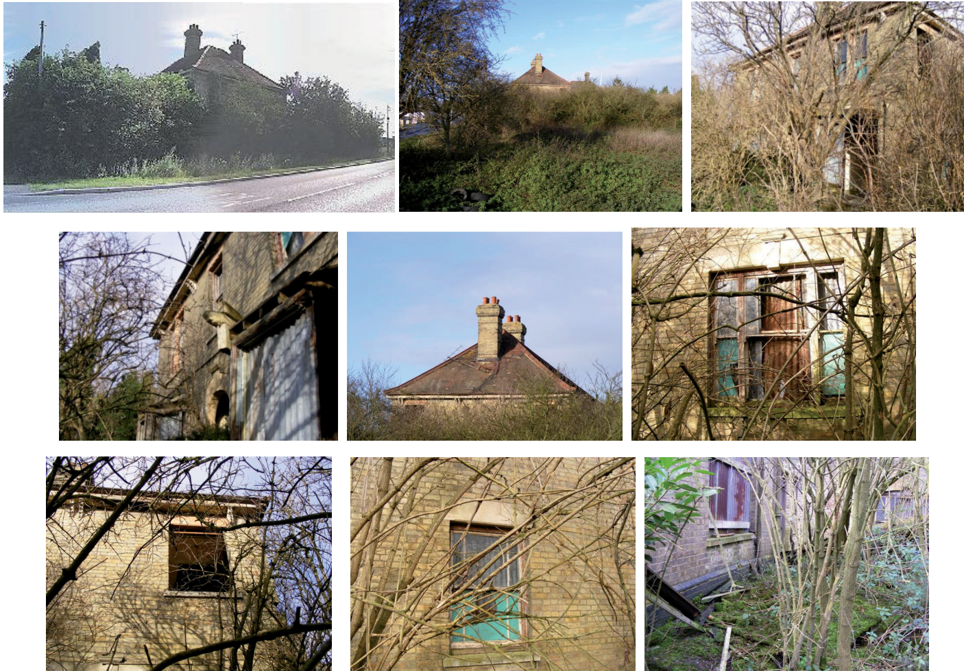
PLATE B: Views of the derelict two storey house (Preliminary House – AOC 62) in the south-west of the development site
