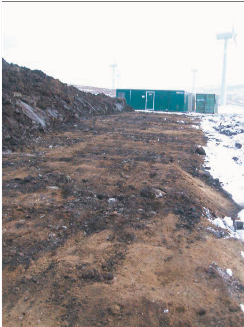
Plate 1: General view after peat stripping haul road and temporary lay down area, from the north
