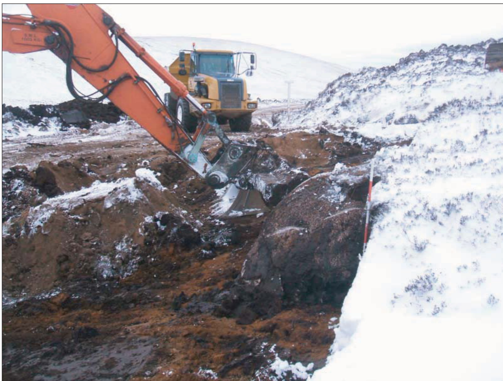
Plate 6: General view during peat stripping of the area and hard standing for turbine 1, A large glacial erratic is visible just below the turf horizon
