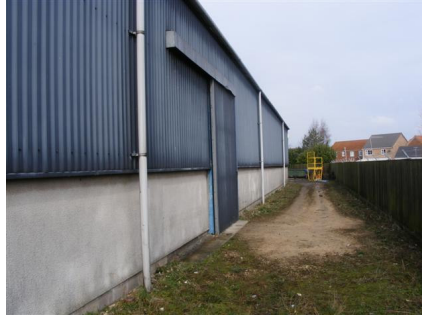
PLATE J: View of the eastern elevation of the main warehouse / assembly building
