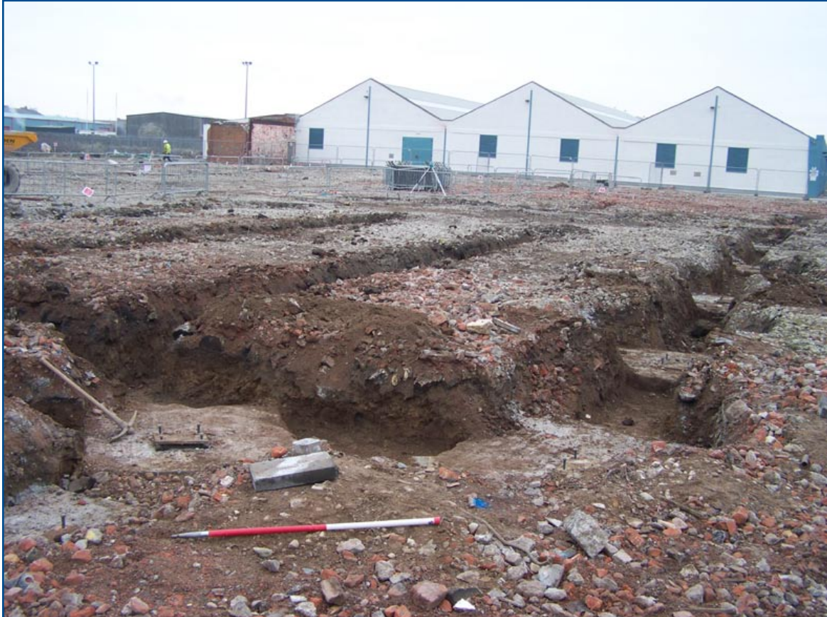
Plate 2: Strip foundations and pads for the building in the southern corner of the site, facing north.
