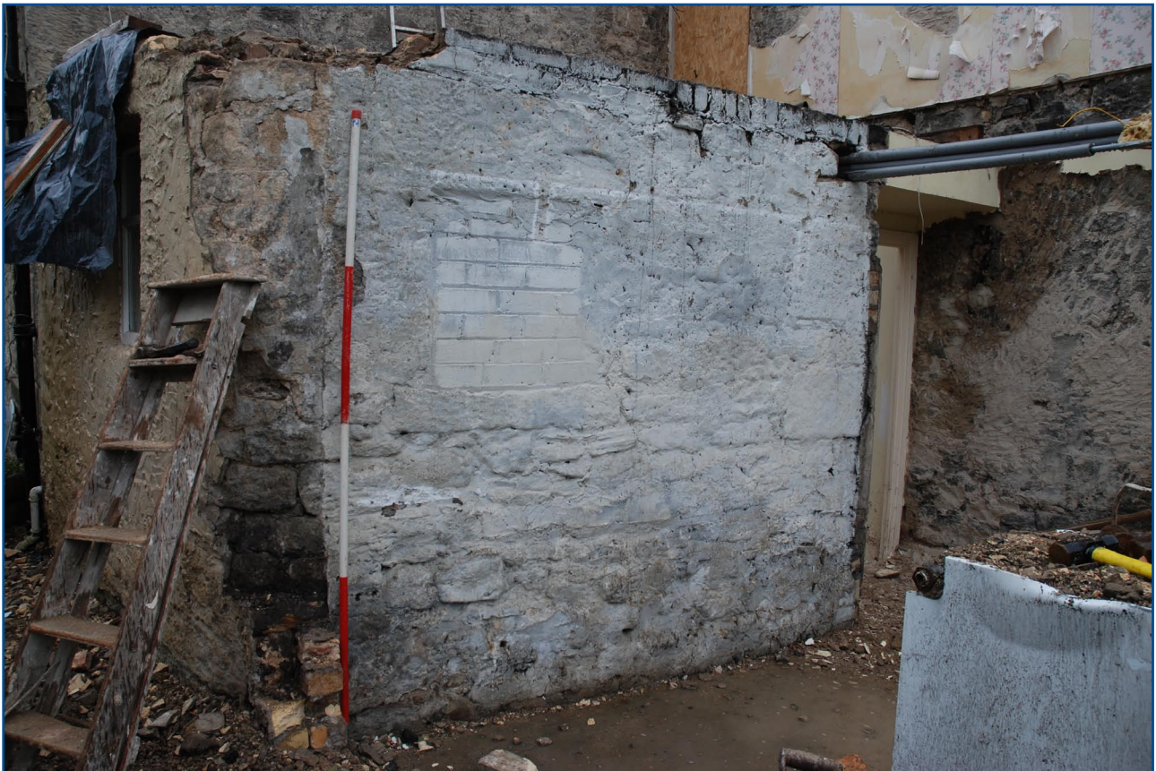
Plate 12: Detail of east wall on Room 0.3 during demolition of Manor House extension from west
