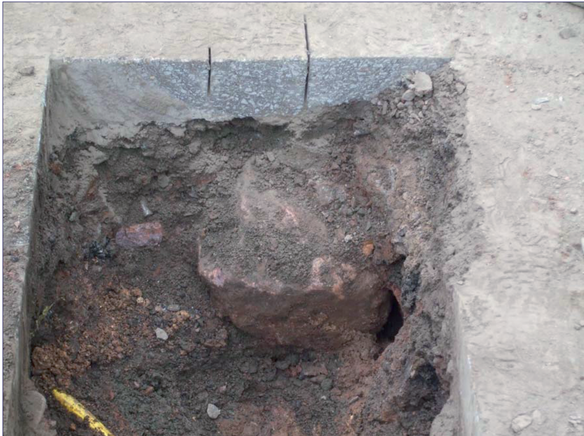
Plate 1: Sandstone block, forming part of the covered lade, with void below
