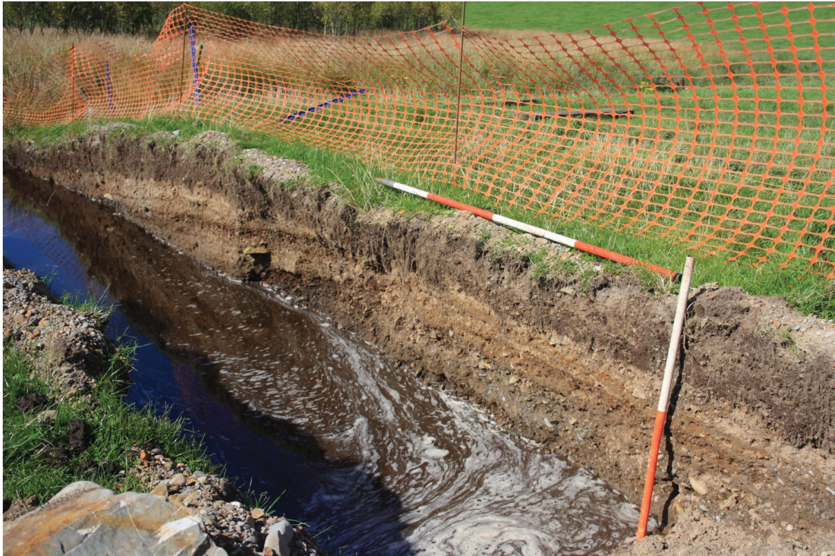
Plate 1: Gravel deposits overlying peats on the neck of the promontory, in trench 4.
