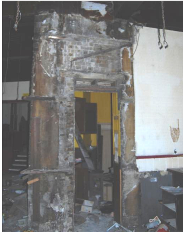
Plate 5: Stripped Area Behind Bar.
