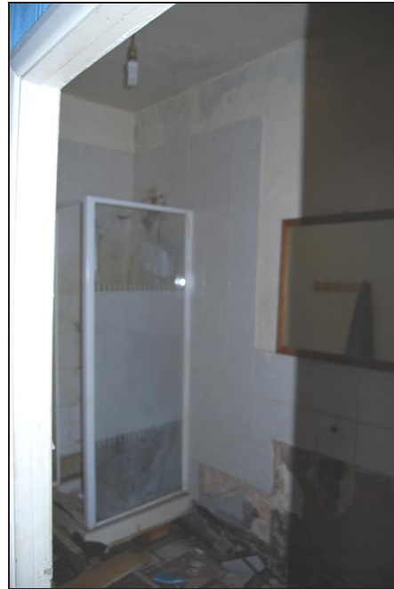
Plate 14: Bathroom S3 with Doorframe.
