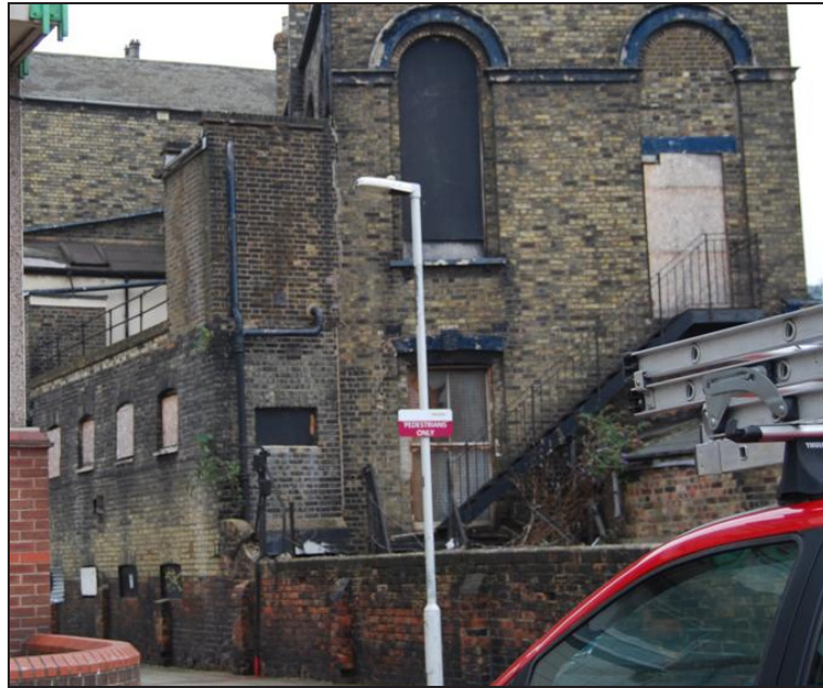
Plate 6: External View of Western End of Building, with Rooms G4 and M1, Red Brickwork with Yellow Brick Above.
