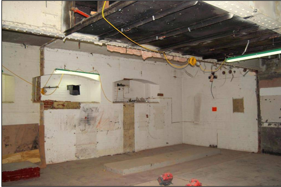
Plate 46: Blocked window in room T8G.9
