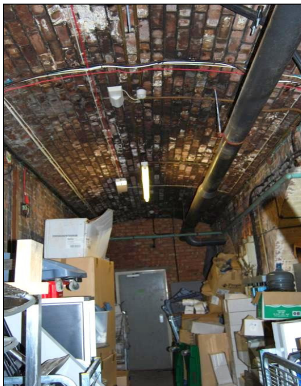
Plate 44: Storage Area with Stores.
