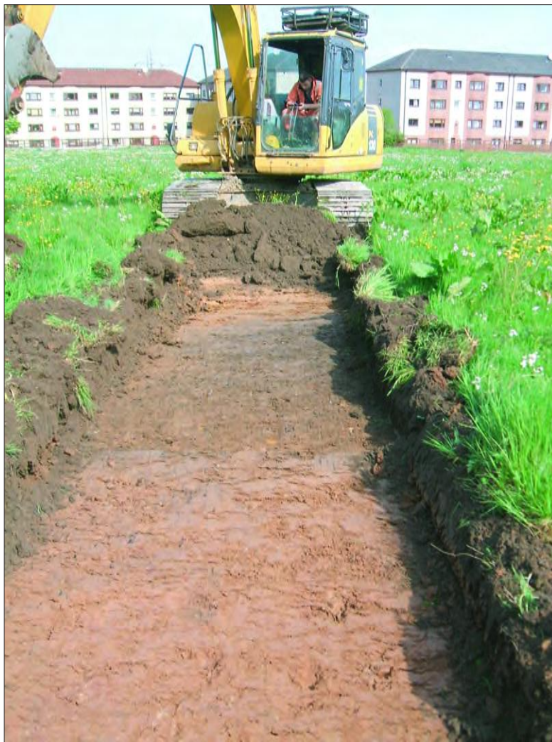
Plate 3: General view of broad rigg cultivation remnant in Trench 2 from the south-east
