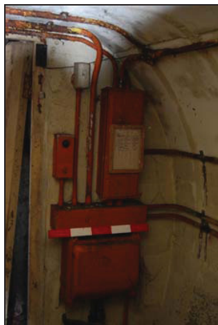
Plate 10: Western Shelter Fuse box
