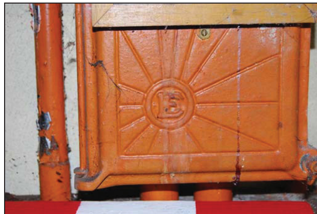
Plate 11: Sunburst on Fuse box
