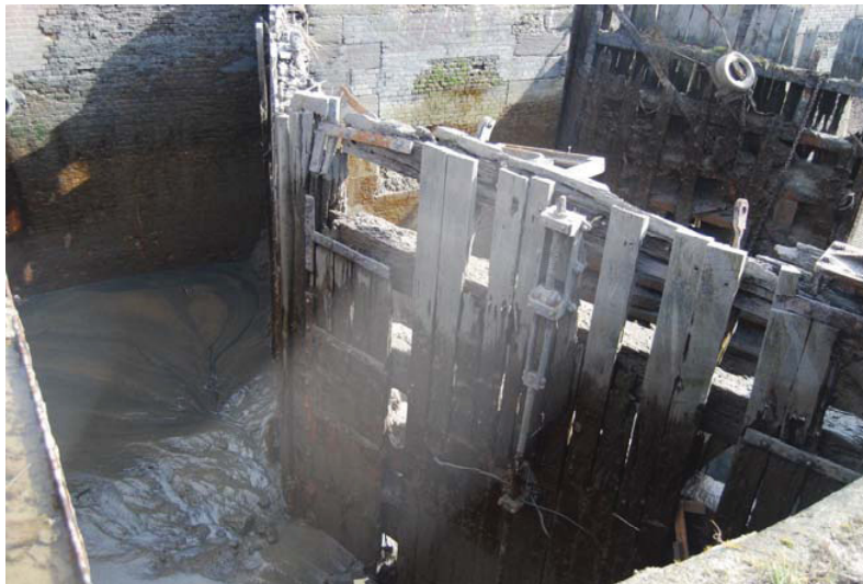
Plate E: Inner Lock Gates
