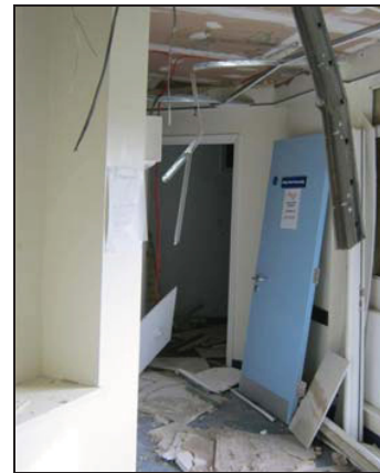
Plate 48: Room 7 Showing Disrepair
