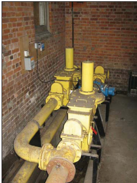
Plate 99: Plant in Building EHW 20
