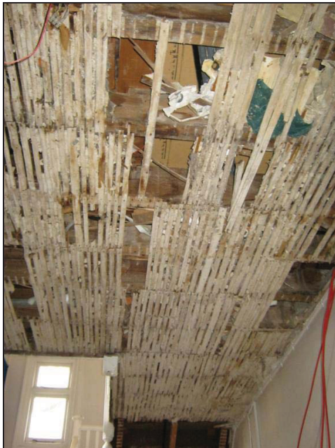
Plate 61: Ceiling Laths in Corridor
