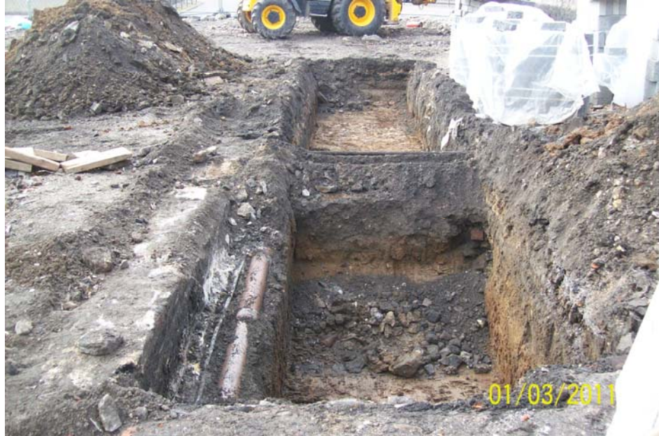
Plate 1: Trench 1, showing wall [106] along left side of the trench with an associated drainage pipe. Trench also crossed by a further service.
