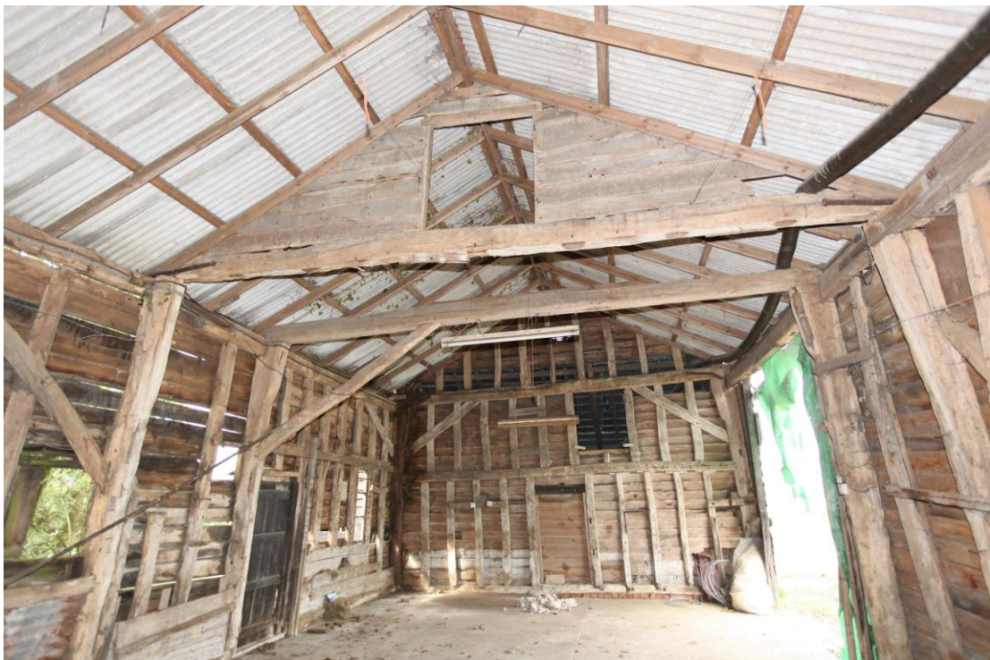
Illus. 12. The remains of the internal northern gable of the 16 th century barn (1) showing empty mortises for missing studs and corner braces but no mid-rail. The southern gable, in contrast, contained a mid-rail. The boarding above the tie-beam retains a loading hatch that served the missing hay loft of the stable bay (1b) beyond.
