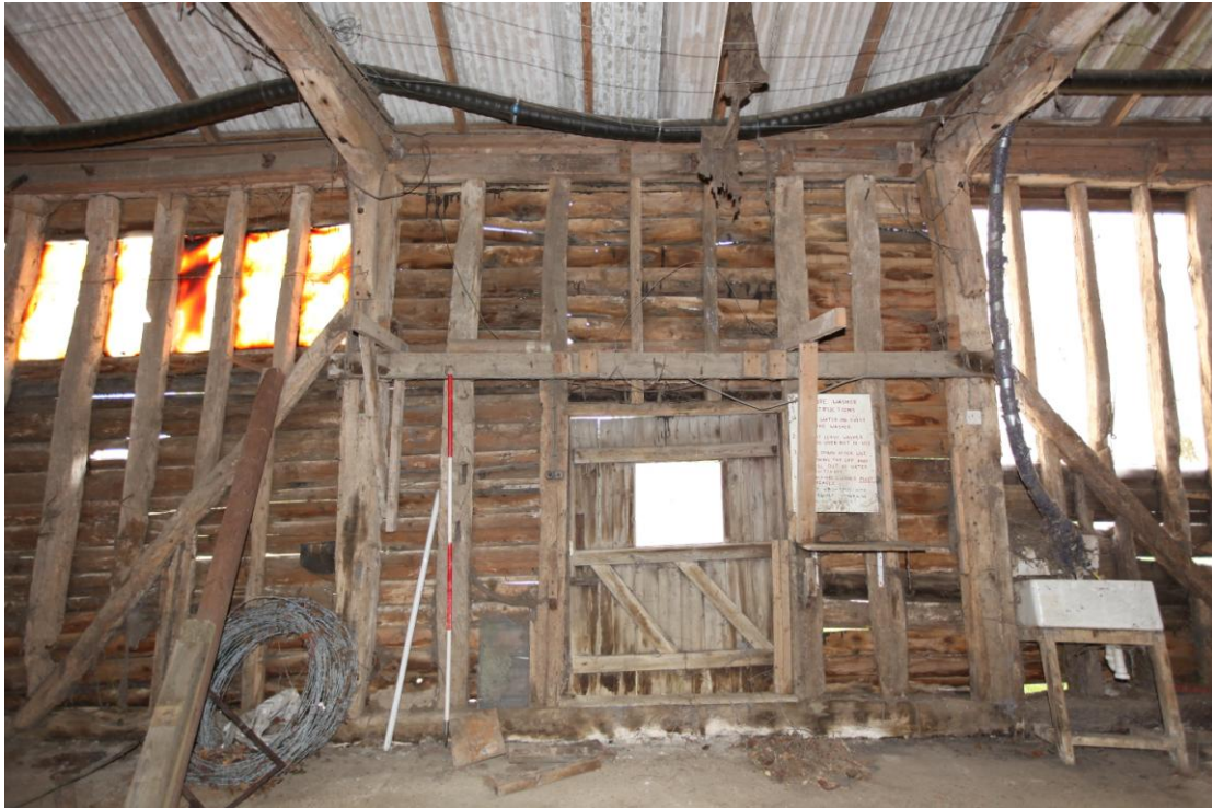
Illus. 11. The eastern interior of the central threshing bay of the barn (1) showing its rebuilt framing, including many re-used timbers, and a small 19 th century rear door. A similarly small doorway would have existed here in the original 16 th century structure.
