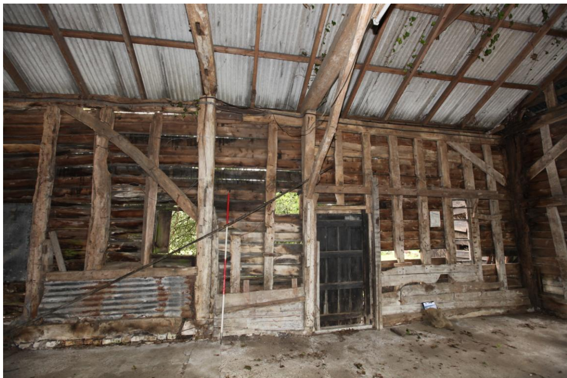
Illus. 8. The northern end of the western interior showing the early-17th century stable bay (1b) to the right and the corner post and tie-beam of the 16 th century barn (1) to the left. The internally trenched corner braces of the original barn are far larger than those of the stable. The position of the stable door appears to be original but this is not certain.
