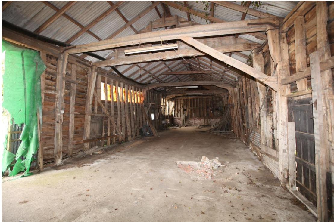
Illus. 5. General view of the interior of the barn from the north showing the intact arch-brace of the early-17 th century stable extension (1b) to the right. The left-hand brace has been removed. The right-hand (western) wall retains most of its original framing while the left-hand wall was largely rebuilt in the 19 th century.
