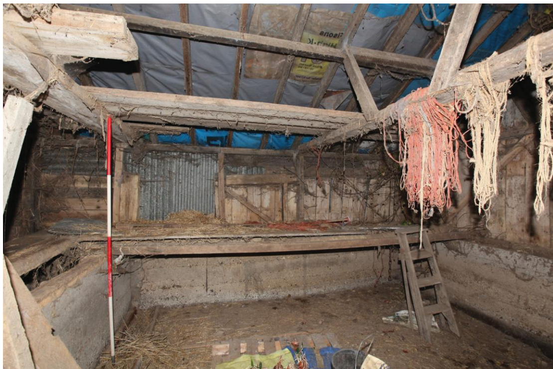
Illus. 10 The northern interior of the eastern boarded shed (2b) showing the storage shelf and a possible blocked doorway adjoining the low internal partition of shuttered concrete to the left.
