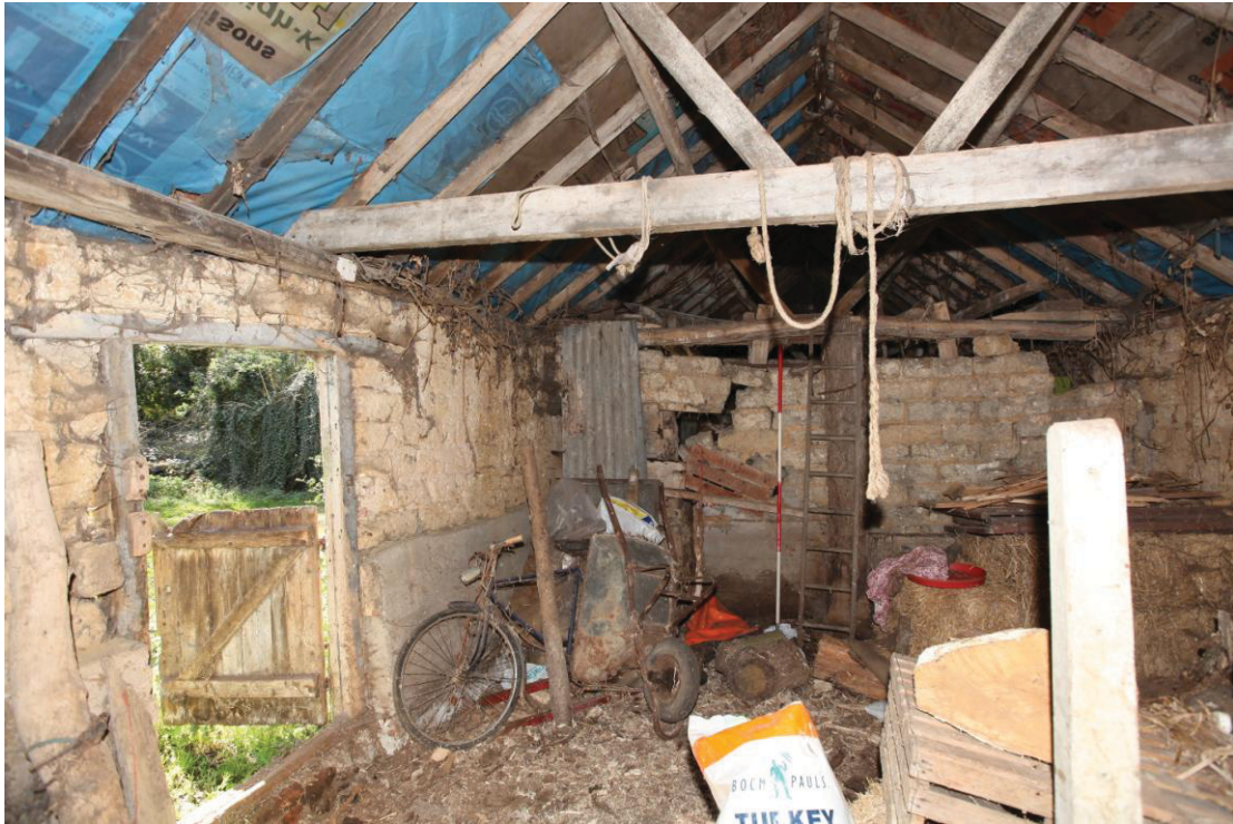
Illus. 7 The interior of the eastern clay-lump shed (1b) from the east showing its southern entrance to the left and the clay-lump internal partition to the western shed in rear (the latter rising only the tie-beam).
