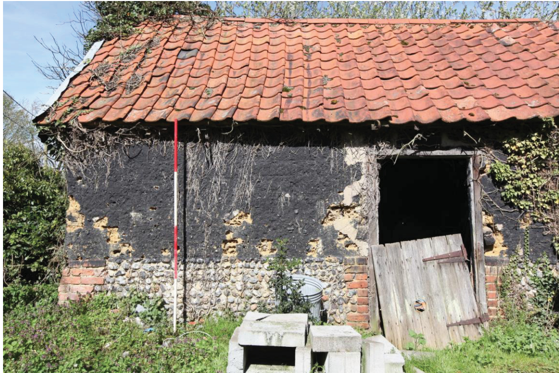
Illus. 3 The western end of the southern exterior of the clay-lump shed (1) showing the original doorway to the western compartment (1a) with red-brick dressing to the flint plinth. The clay-lump fabric has suffered damage from tunnelling bees where the tar is lacking.
