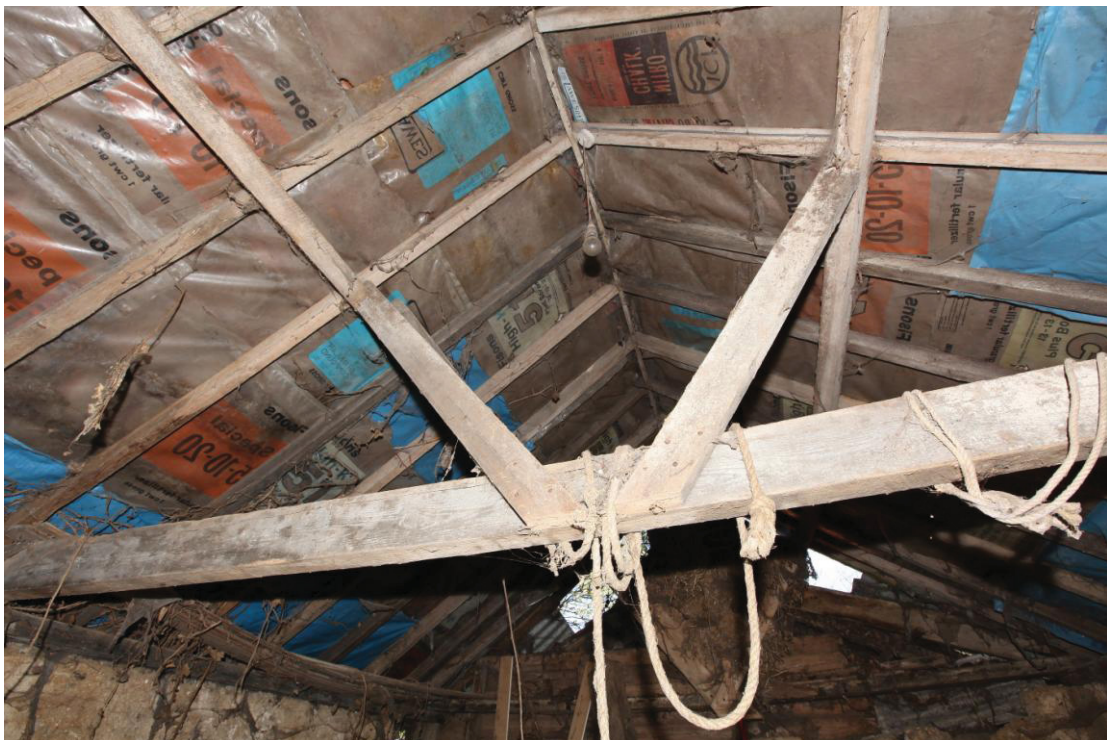
Illus. 8 Detail from the west of the rebuilt 20 th century roof structure in the eastern clay-lump shed (2b) showing its crudely nailed softwood struts and tie-beam.
