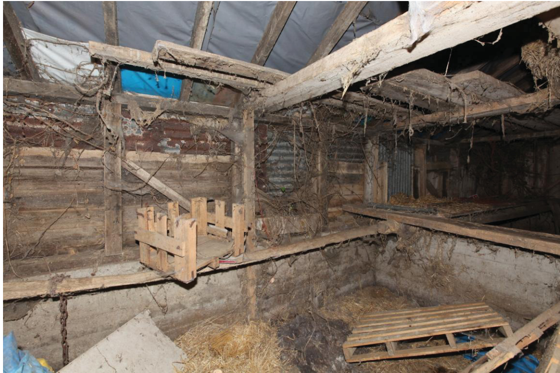
Illus. 9 The northern interior of the boarded shed (2) from the south-west showing the internal storage shelf and horizontal external weatherboarding beneath the later cladding of corrugated iron.
