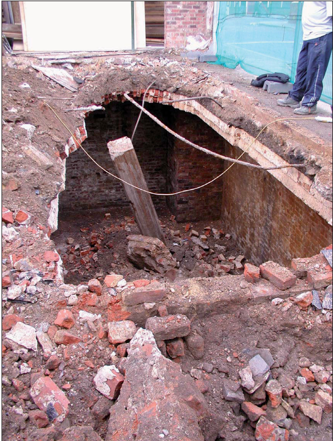
Plate III: Larger chamber of the cellar beneath No. 2, Fore Street. The smaller chamber is in the foreground but is yet to be excavated (11/2/2005)
