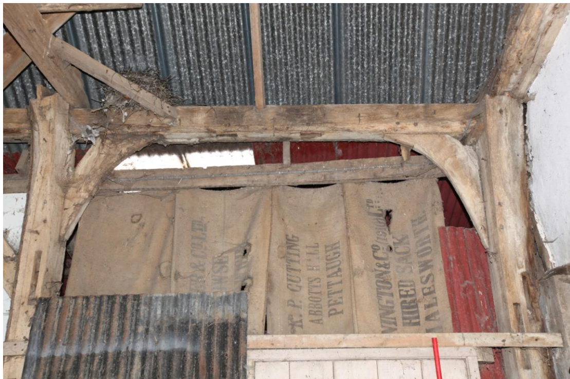
Illus. 12 Detail of the western roof-plate of the gateway (1a) showing its original corner brackets (fully tenoned and pegged to the frame) with a series of mortises for later studs which have since been removed.
