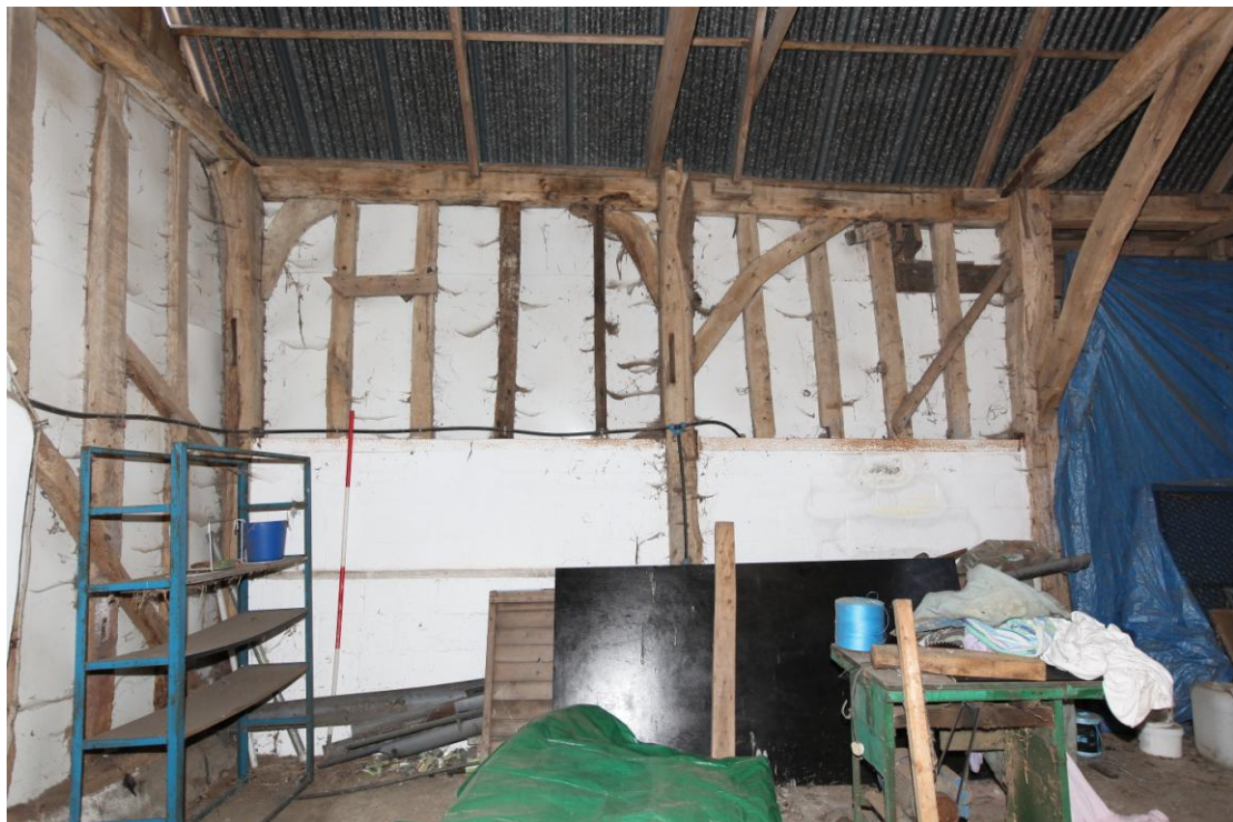
Illus. 8 The eastern interior of the barn (1) showing the original corner brackets and later studs of northern gateway (1a) to the left and the main entrance to the threshing barn behind the blue tarpaulin to the right. The arched gateway was divided by the barn by a missing partition at the central post from which the studs and tie-beam have been removed, and contained a high loft as indicated by joist mortises in the gable tie.
