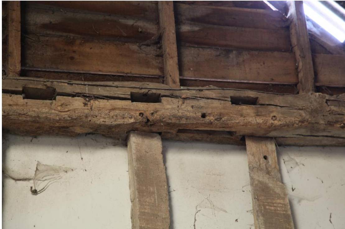
Illus. 11 Detail of the tie-beam of the northern gable of the barn (1) showing a series of 11 original pegged mortises for the missing joists of a loft above the gateway (1a). The studs are also original, with an empty mortise and trench for an internal wall brace.
