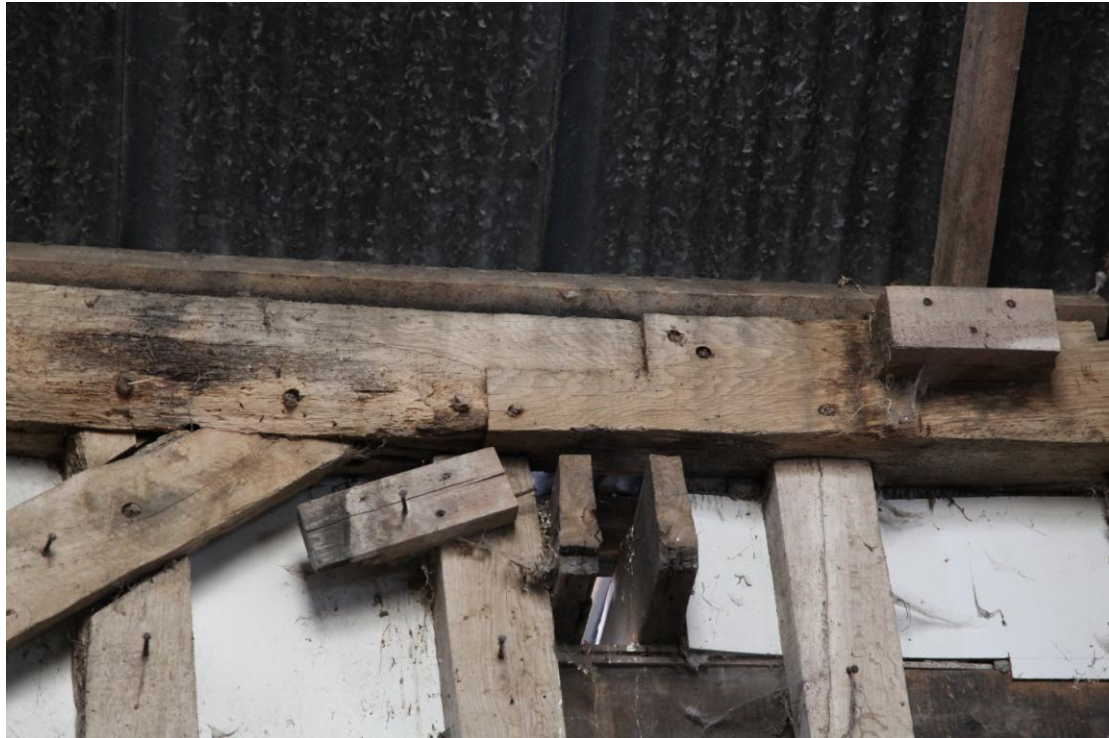
Illus. 9 Detail of the 16th century type edge-halved and bridled scarf joint in penultimate bay of the eastern roof plate of the barn (1) as shown to the right in illus. 8 above.
