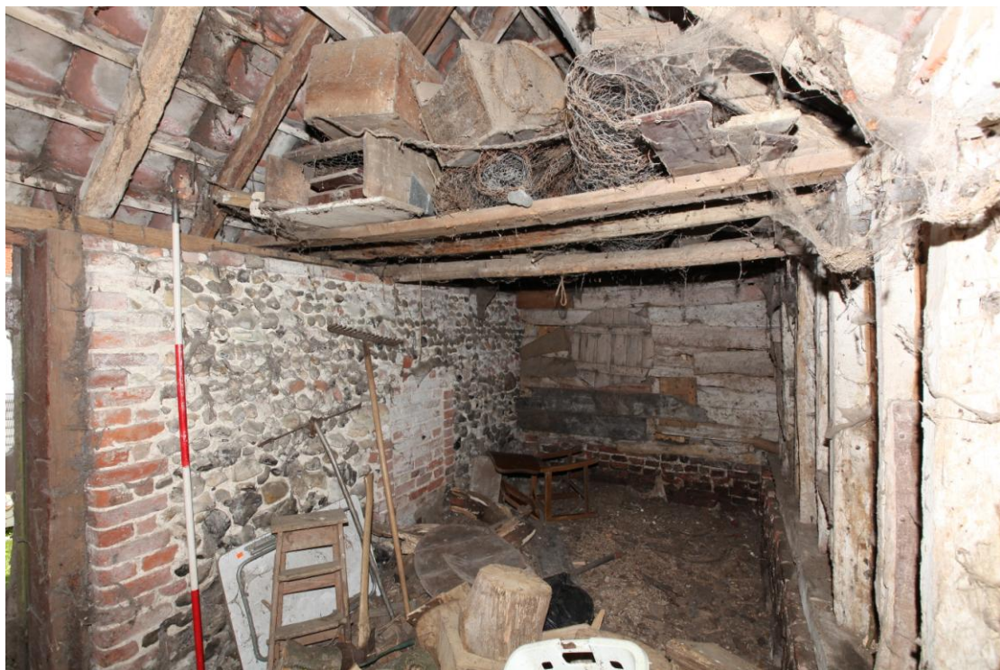
Illus. 8 General internal view of the central shed (1b) from the west showing its original cross-entry in the foreground and the opposing small doorways (now blocked) in the rear. The boarded partition to the eastern shed (1a) includes a re-used circular copper lid.
