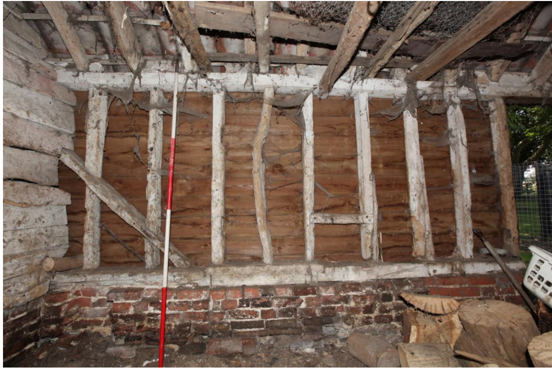
Illus. 9 The southern interior of the central shed (1b) showing its original studwork with a later stud blocking the original narrow entrance (indicated by the crooked secondary stud in the centre and by corresponding straight joints in the brick plinth).
