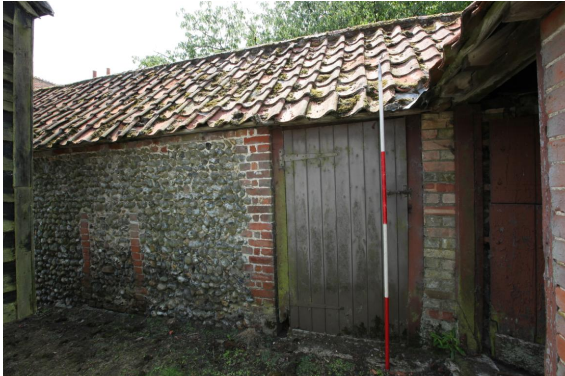
Illus. 5 The northern exterior of the original shed (1) showing the original doorway opening onto the central area (1b) with the door of the later brew-house (3) to the right and the brick jambs of a blocked narrow entrance (just 2 ft wide by 3.5 ft high) to the left.
