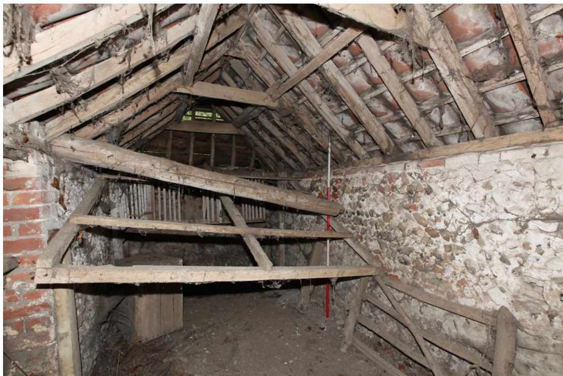
Illus. 10 The interior of the later flint-rubble extension (2b) seen from the east, showing its collapsed tie-beam and joists with a slatted chicken coop attached to the western gable in the rear.
