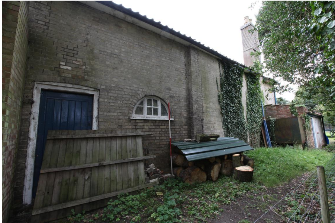
Illus. 5 The rear (north-eastern) exterior showing the original door and arched window to the probable former stable (1d) to the left and the projecting central bay to right. The straight vertical joint in the latter's brickwork suggests the right-hand half of the structure has been remodelled (i.e. the domestic cottage 1a and 1b).
