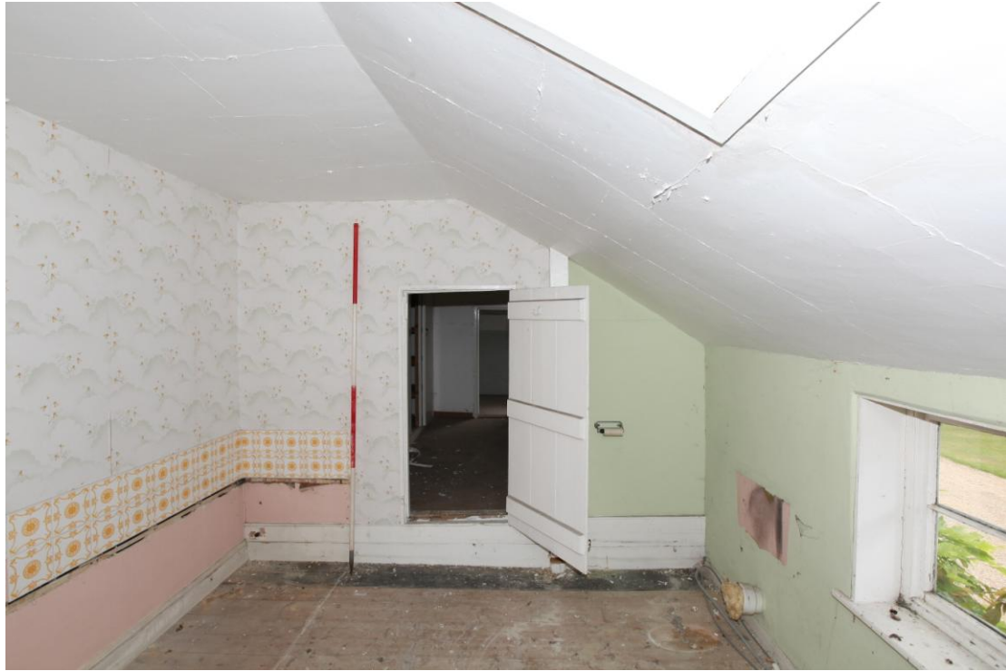
Illus. 11 The front (south-western) bedroom above the cottage sitting room (1b) showing the door to the raised area above the central shed (1c).
