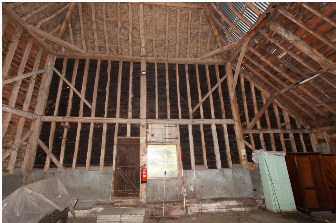
Illus. 6 The internal eastern gable showing its nailed primary wall braces (interrupting the narrow unpegged studs) with the rear aisle to the right. The tie-beam abuts the wall-plate and arcade-plate in a manner not found before the 19 th century - before which the tie-beam would have been dovetailed to the respective plates above jowled corner posts. The door is secondary but the ventilation hatch above the modern window is original.
