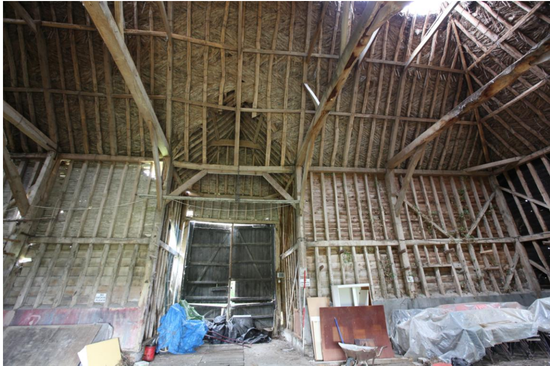
Illus. 11 The eastern end of the northern interior showing the entrance to the eastern porch (1a) with the original framed doorway in bay A to the right. The roof-plate above the porch contains empty mortises for studwork above an original lintel at the same level as the secondary corner braces, and the reed fleaking beneath the thatch is laid in a herringbone pattern.
