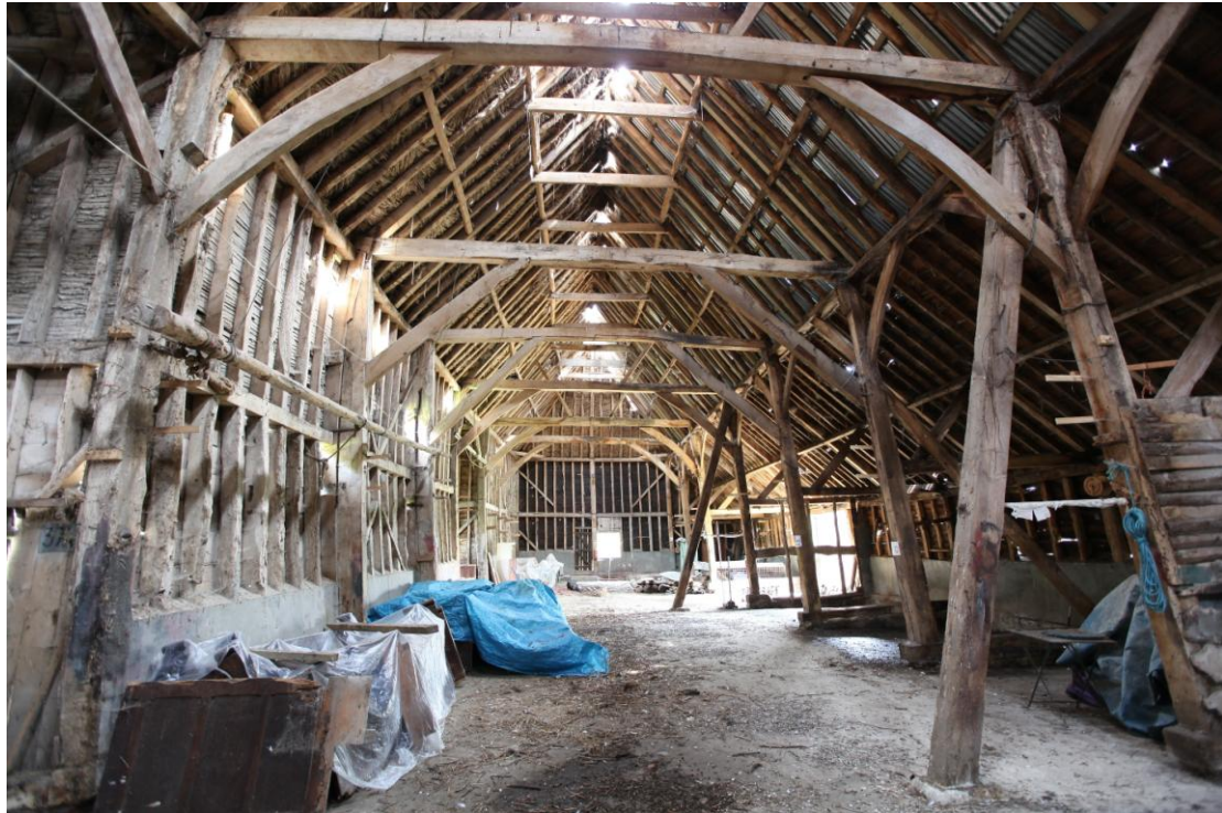
Illus. 5 A general view of the barn interior from the west showing its largely intact roof structure and arch-braces with the original rear aisle to the right. The diagonal props are secondary insertions, as are the inner storey posts of the northern elevation to left.
