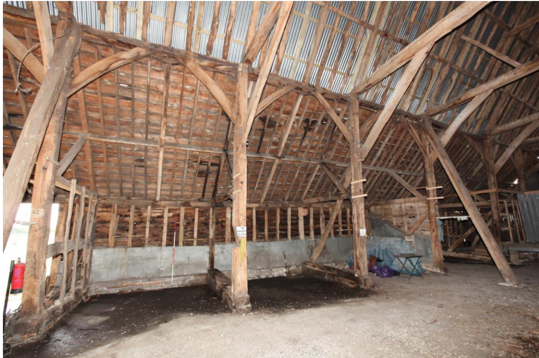
Illus. 7 The central bays (D, F and G) of the southern aisle showing the intact arch-braces to the arcade plate and the renewed tall-sectioned softwood rafters of the aisle roof.
