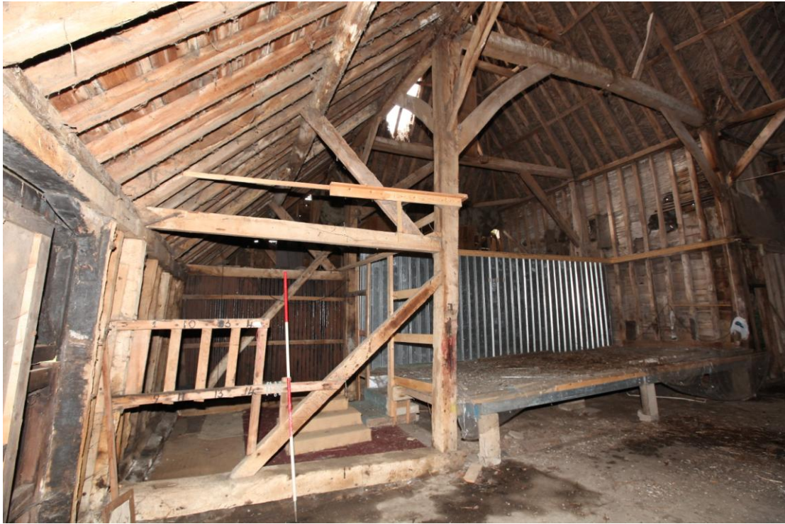
Illus. 9 The well-preserved lateral truss to the west of bay H showing an original down-brace in the foreground and a secondary strut in the rear.
