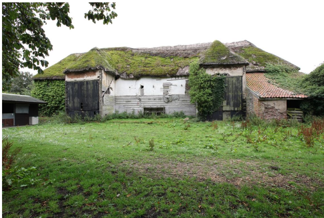
Illus. 2 The northern facade of the barn showing its original 'two-tier' cladding of render above horizontal boarding and thatched roof with twin hipped porches (1a and 1b) to left and right respectively. The secondary pantiled flint-rubble lean-to (2) is visible to the extreme right. A similar lean-to between the porches has been demolished.
