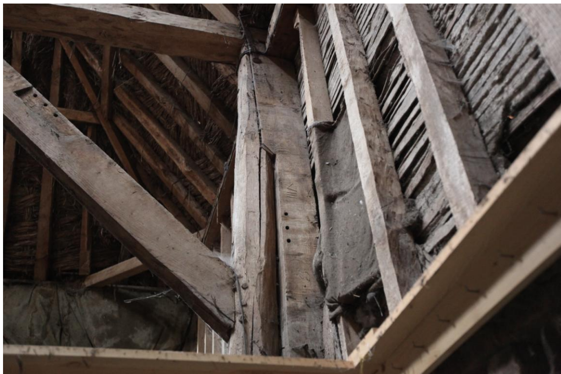
Illus. 12 A detail from the east of the northern storey post between bays J & I showing an inserted support post obstructing the jowl and mortise of the original arch-brace. The latter is numbered VIII.
