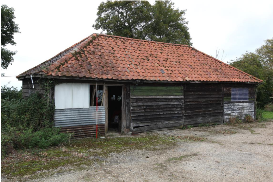
Illus. 3. The exterior of the cart lodge from the south-east showing its originally open eastern elevation (now enclosed by 20 th century boarding) with the weatherboarded southern gable to the left.
