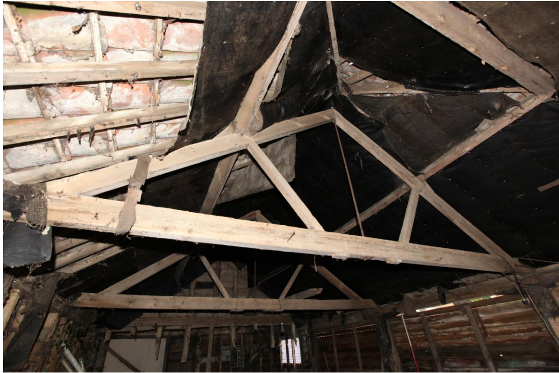
Illus. 7. Detail of the pre-fabricated softwood roof trusses from the south showing a central iron suspension bar.
