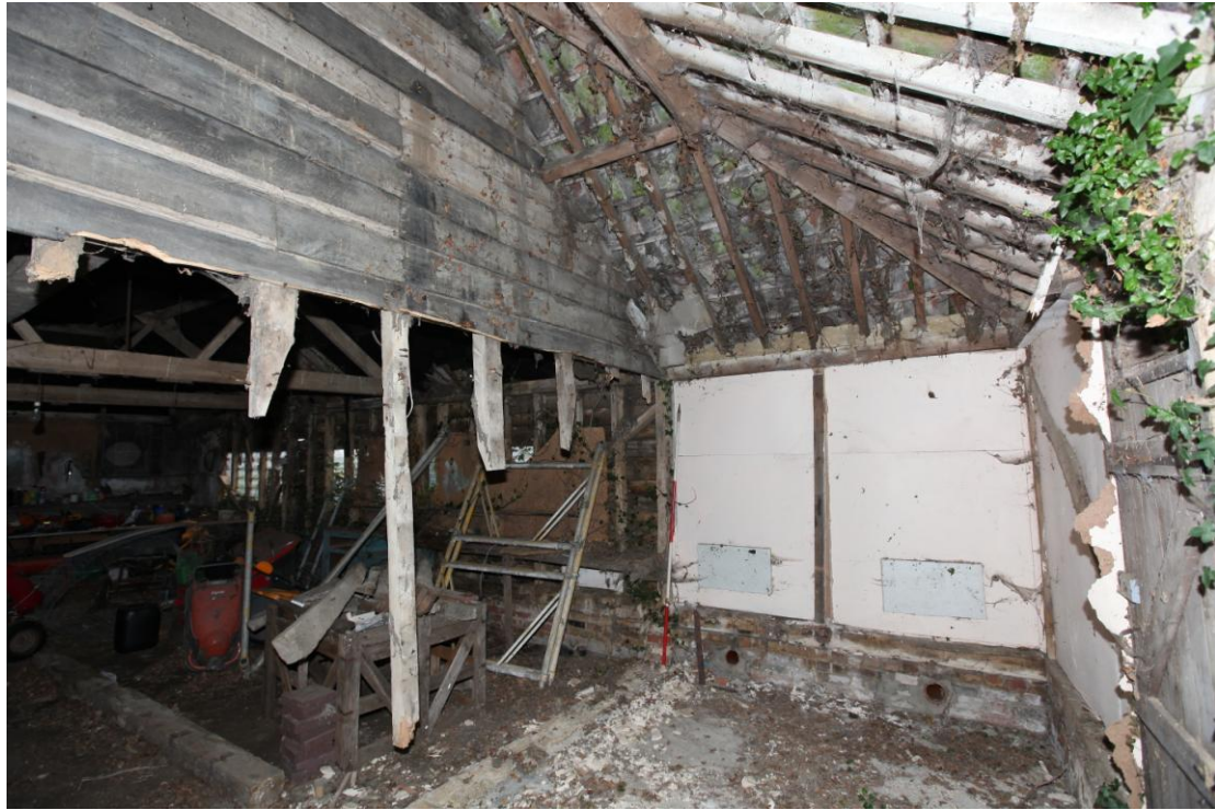
Illus. 5. The interior of the northern bay from the east showing the remains of the boarded internal partition to the left and the northern gable to the right.
