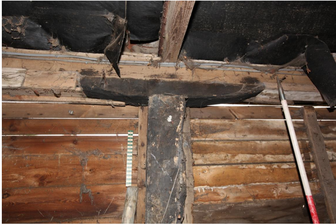
Illus. 9. Detail of the chamfered and nailed lintel to the northern arcade post of the eastern interior.
