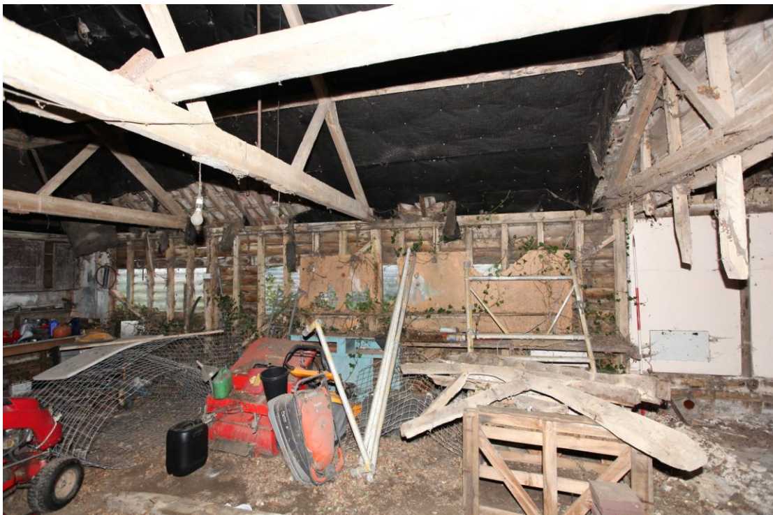
Illus. 4. The rear (western) internal elevation showing its narrow studs with nailed primary braces and deal roof-plate. The remains of the original boarded partition on a brick plinth to the northern bay are visible to the right.
