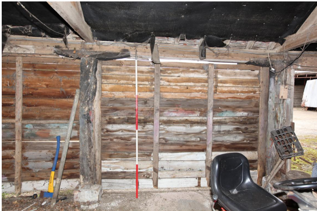
Illus. 8. Detail of the black-painted arcade posts and lintels to the original open eastern interior.
