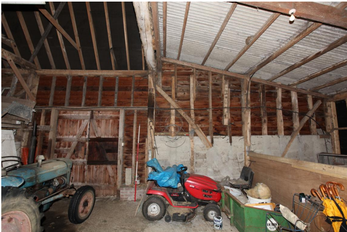
Illus. 10 The eastern end of the barn's northern interior showing the 20 th century doors in bay C to the left and the largely original framing of bays D and E to the right beneath the truncated roof. There is no evidence of tie-beam braces or loft joists in the jowled storey posts.
