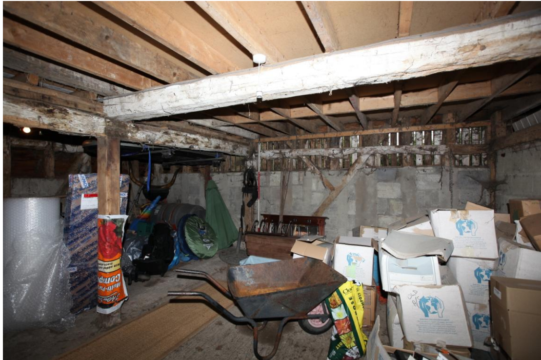
Illus. 7 The northern interior of bay B showing the original axial and binding joists of the loft with recently renewed softwood common joists & cement block-work between the original studs of the external wall.
