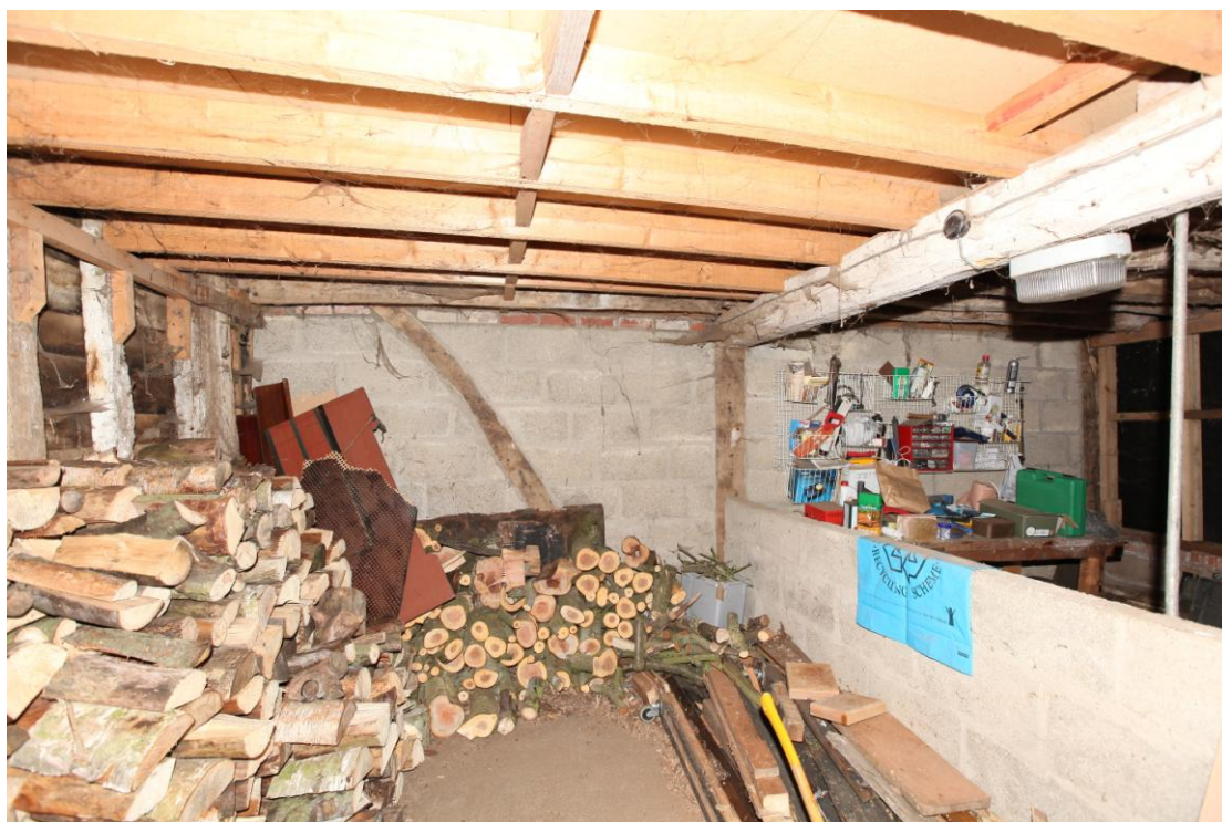
Illus. 12 The interior of the southern shed (F) from the south showing the cement-block partition to the main barn with a single original primary brace. The whitewashed axial joist to the right is also original but the common joists of the loft have been renewed in softwood.
