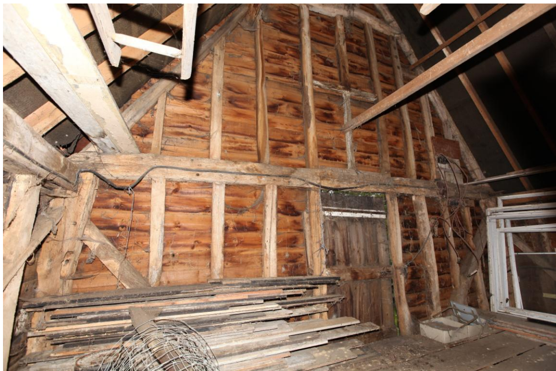
Illus. 8 The largely intact interior of the western roof gable (seen from the loft in bay A) showing the original rafters and pegged primary wall braces with copious re-used timber. The horizontal timber above the tie-beam appears to have been the lintel of a blocked window.
