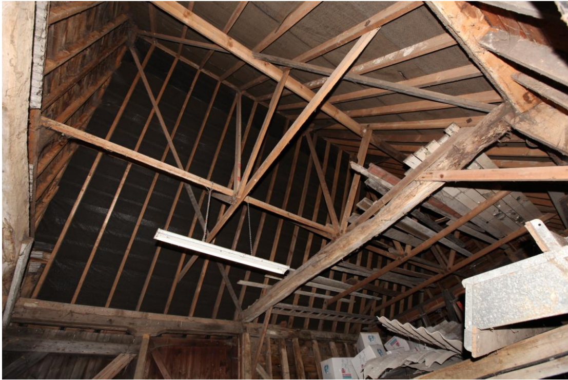
Illus. 9 The interior of the open barn from the north showing the recently rebuilt softwood roof structure with the two-bay loft to the right & the central entrance doors in bay C to the left.
