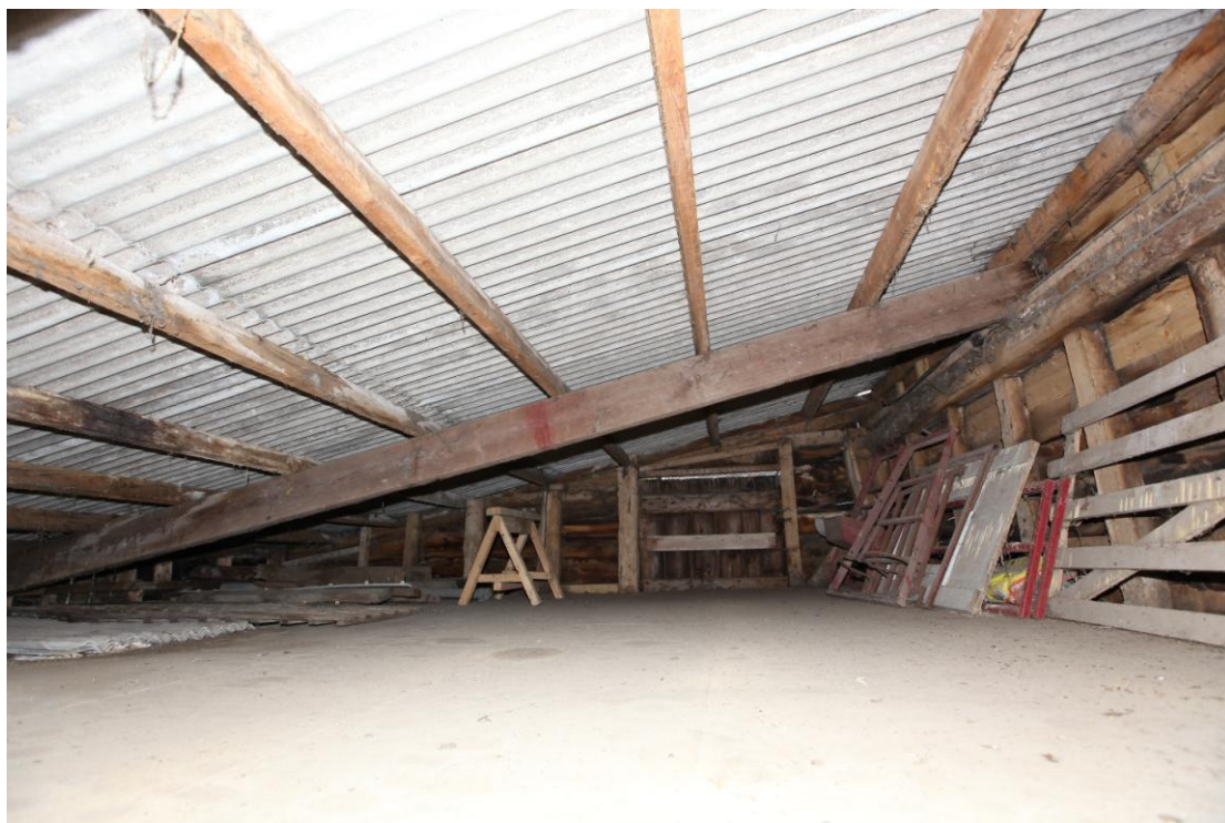
Illus. 11 The truncated loft of the southern shed (F) seen from the open barn to the north showing the original studwork and jowled storey posts of the intact western elevation to the right.
