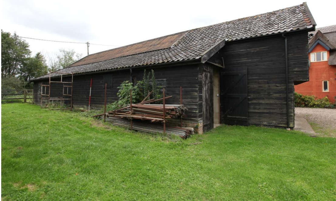
Illus. 1 The exterior of the barn from the north showing the glazed pantiles of the modern (1980s) garage with overhanging upper storey to the right and the lean-to shed (3) to the left. The corrugated iron roof of the main barn (1) is visible to the rear.
