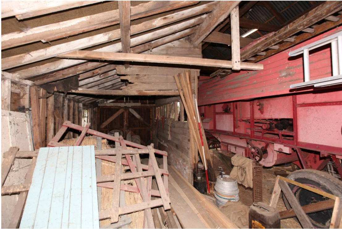
Illus. 7 The interior of the lean-to shed (3a) from the west showing the entrance to the central bay of the barn (1) to the right and the fragmentary remains of the boarded partition which originally divided the area adjoining the threshing floor from the eastern shed beyond.
