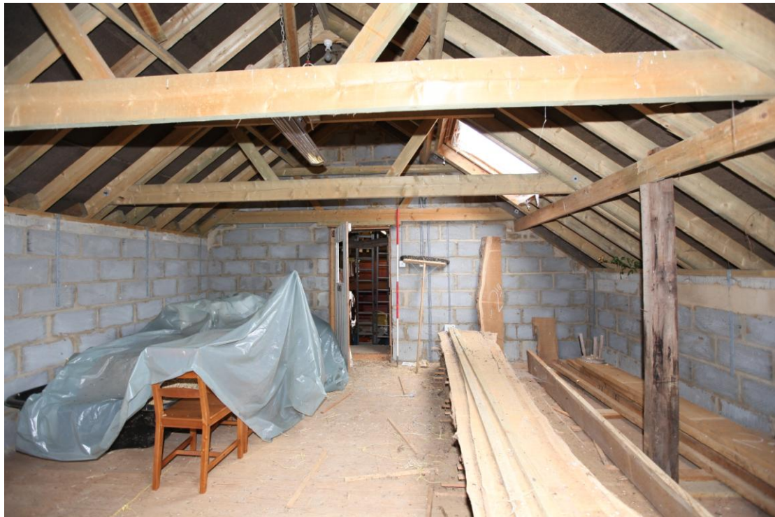
Illus. 6 The interior of the loft above the 20th century garage (2) from the west showing its cement-block fabric (hidden by weatherboarding to the exterior) and the door to the barn (1).
