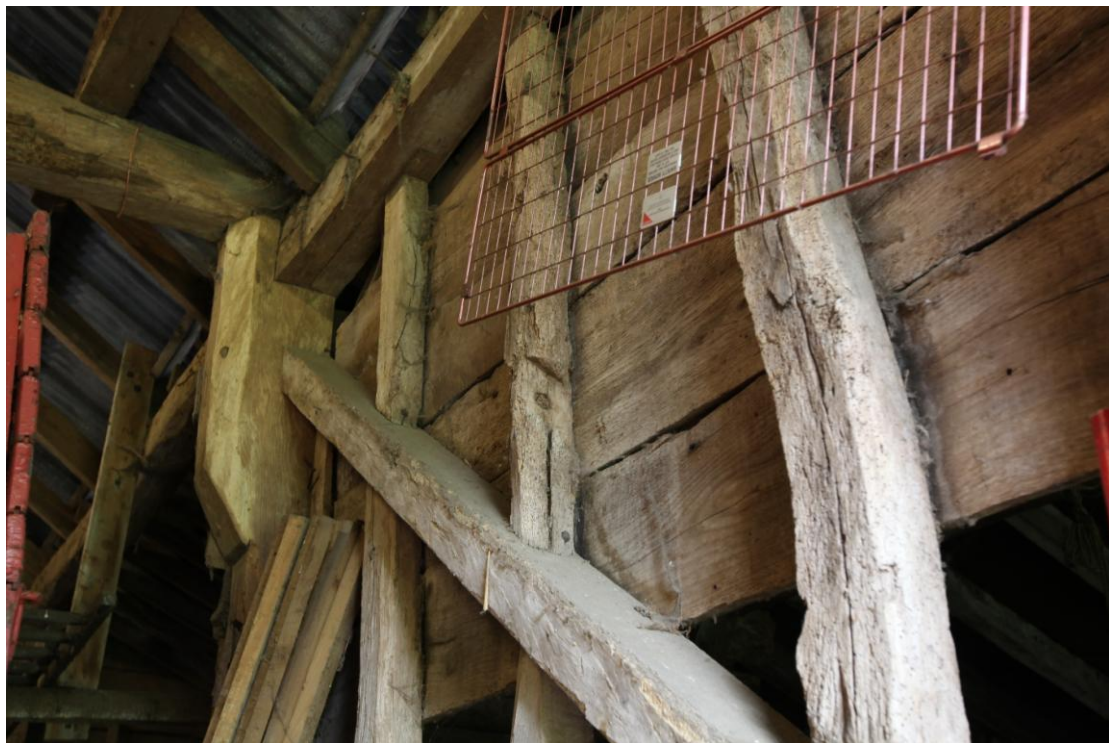
Illus. 10 A detail from the east of the northern jowled storey post to the east of the central bay showing a face-halved and bladed scarf joint in the roof-plate and copious evidence of re-used timber. The butted external boards shown here suggest the rear lean-to is an original feature.
