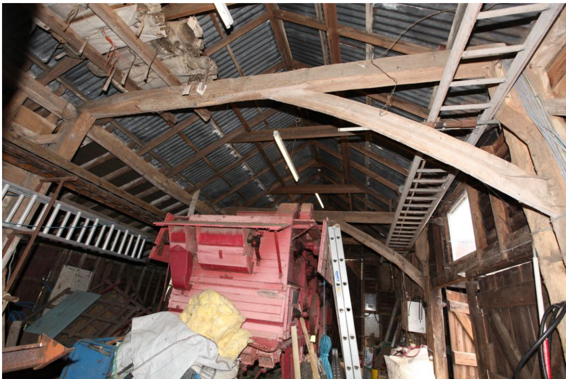
Illus. 8 The late-20th century softwood roof structure of the barn (1) from the west, showing the two original arch-braces tie-beams flanking the central bay to the right and the positions of the removed northern arch-braces to the left.
