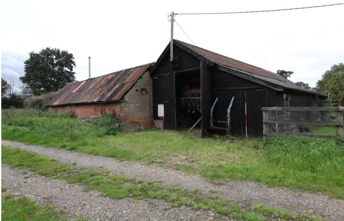
Illus. 2 The exterior from the east showing the inserted vehicle doors in the gables of the barn (1, centre) and the lean-to shed (3a, right) with the brick shelter-shed (4) to the left.
