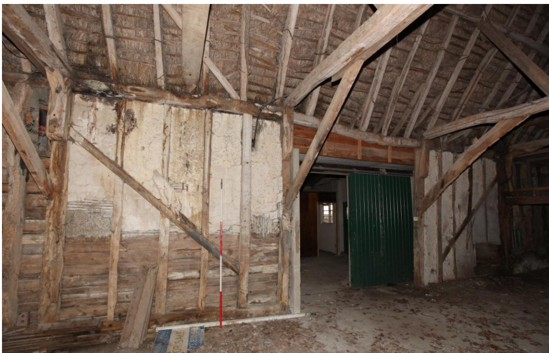
Illus. 8. The northern interior of the original three-bay threshing barn of circa 1800 barn showing its largely intact framing with pegged primary braces and the position of the northern entrance in its central bay. This entrance appears to have opened onto a rear porch (possibly with a lean-to roof structure rather than a vertical gable).
