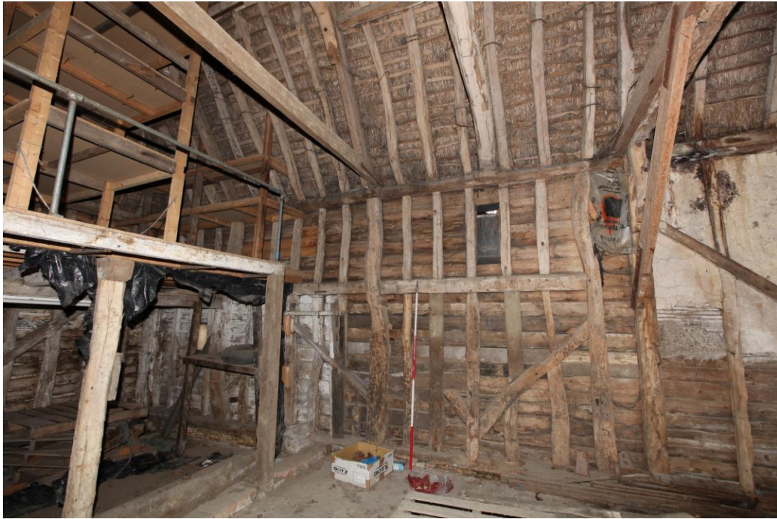
Illus. 7. The northern interior of the three-bay stable (1c) showing evidence of re-used timber with nailed diagonal primary braces and unusually distorted storey posts linked by mid-rails. The original tie-beam of the removed western gable of the three-bay barn is visible to the right (with some extant lath-and-plaster to its western bay). The remaining fragment of the original loft to the left has been largely rebuilt in modern softwood and supports a series of modern storage shelves.
