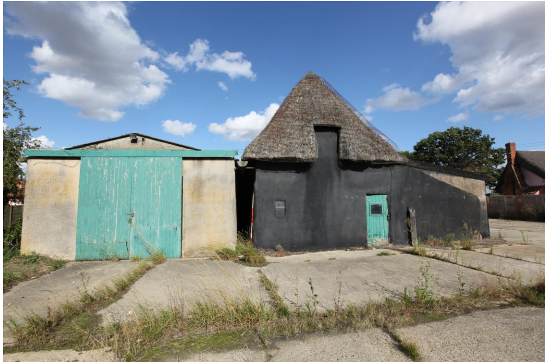
Illus. 3. The external western gable showing the sliding doors of the garage shed (3) to the left and evidence of a blocked window or loading hatch in the thatch of the hipped gable above the former stable (1c). Note the tarred external render and the profile of an earlier southern lean-to shed to the right.
