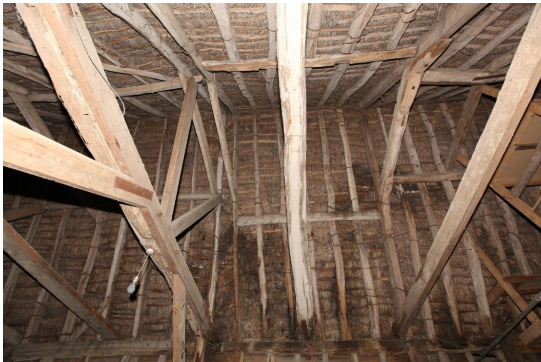
Illus. 12. The southern roof structure of the three-bay stable (1c) showing its triangular butt-purlins and the junction with the clasped-purlin roof of the barn (1a) to the left.
