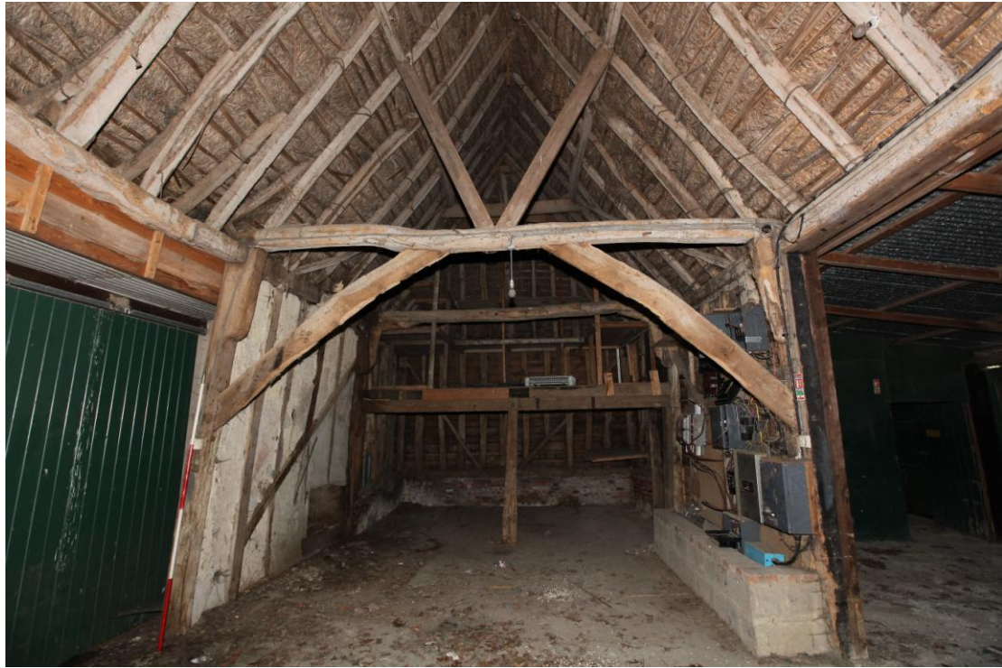
Illus. 9. The interior of the concreted central threshing floor of the three-bay barn (1a) seen from the west, showing the intact open-truss of the steeply-pitched clasped-purlin roof structure with later (V-shaped) queen-struts above its tie-beam.
