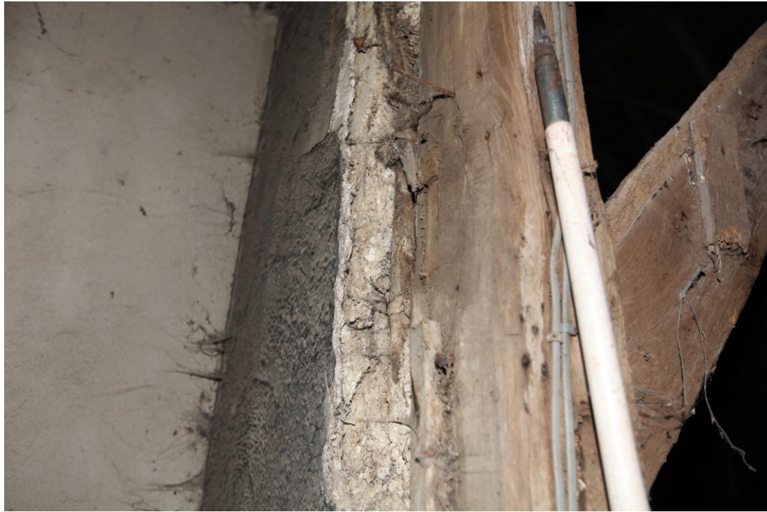
Illus. 11. The eastern truss of the central bay of the barn (1a) seen from the west, showing the narrow exposed section of original external roughcast clay daub with a skim of tarred lime plaster. The mortise of the demolished rear 'porch' which this daub abutted is also visible.
