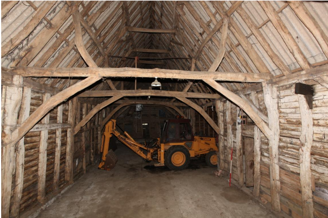
Illus. 5. A general view of the main barn (C-G) from the south, showing the distinctive profile of its roof trusses. The original mid-rail in bay F is visible to the left – apparently a device to allow the re-use of short lengths of timber.
