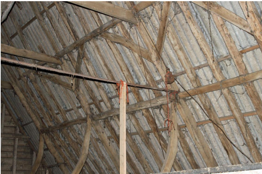
Illus. 6. The roof structure seen from the north-east, showing the exceptionally intact array of curved wind-braces to the upper tier of clasped-purlins and the lower tier of butt-purlins.
