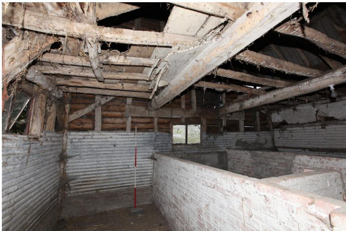
Illus. 8. The internal gable of the northern stable (bays A and B) showing the twin axial joists of the hay loft with remnants of lath-and-plaster. The mid-20 th century brick partitions and wainscot of corrugated asbestos were probably designed to form loose boxes for calves.
