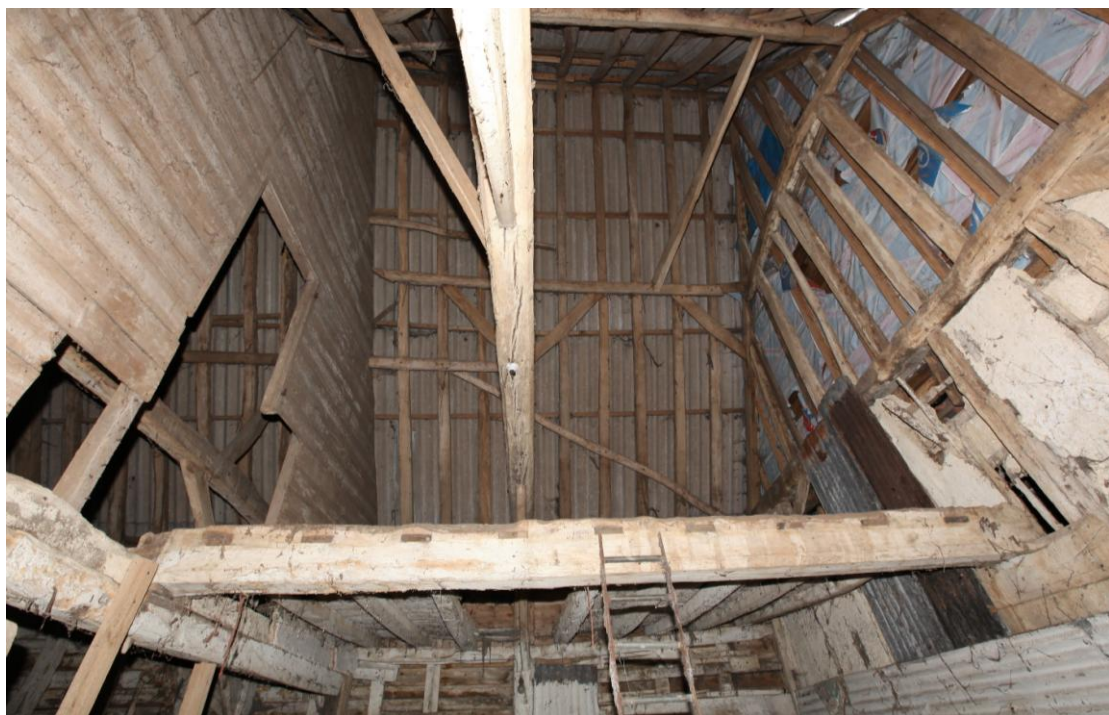
Illus. 12. The southern stable (bays H and I) from the west, showing the empty soffitenon mortises in the axial joist for the missing western half of the hay loft. Note the junction with the different roof of the main barn: The clasped and butt purlins of the latter project through the boarded loft partition to the left and are nailed to the rafters. This roof consists only of clasped-purlins and lacks queen-struts. This end of the building also differs in the absence of re-used timber and appears to pre-date the rest of the barn.
