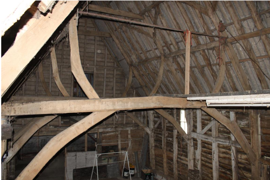
Illus. 7. The highly unusual cranked queen-struts between the tie-beams and principal rafters, seen from the north-east. These are tenoned and pegged to the tie-beams but nailed to the rafters and may possibly be secondary insertions.
