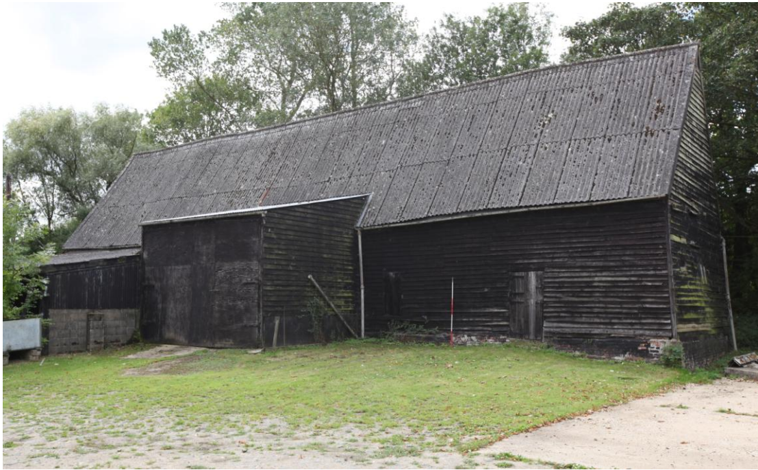
Illus. 1. The eastern exterior showing the corrugated asbestos roof (steeply pitched for its original thatch) with a late-20th century lean-to porch adjoining bay E to the left (on the site of an earlier, narrower gabled porch) and the half-hung entrance door to the northern stable in bays A and B to the right.
